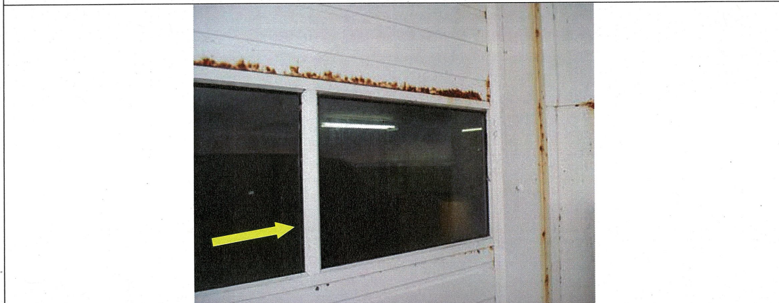
Typical asbestos-containing black window putty applied to glazing of the exterior overhead sectional doors.
