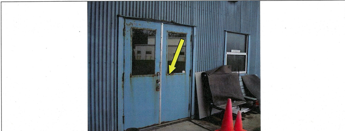
Typical asbestos-containing black window putty applied to glazing of the exterior man doors.
