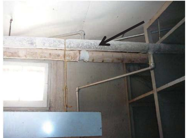
#2 Administration Office - Basement Suspected mould growth on asbestos pipe insulation
