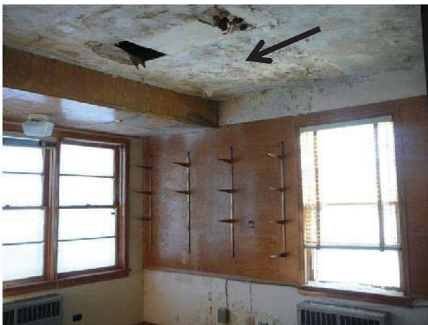
#2 Administration Office – Main Floor Water damage and failure of the main floor ceiling
