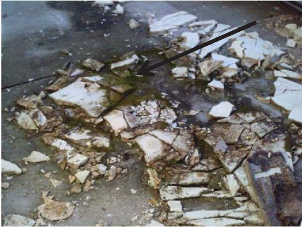
#2 Administration Office – 2 nd Floor Ceiling material on the floor with biological growth
