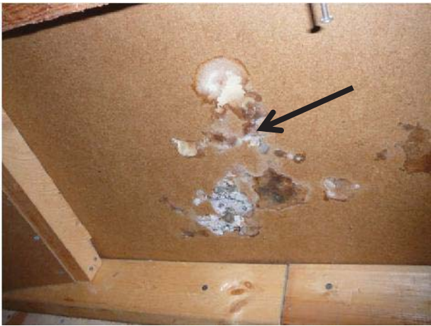
#33 Processing & Carpenter Shop Attic with some suspect mould growth
