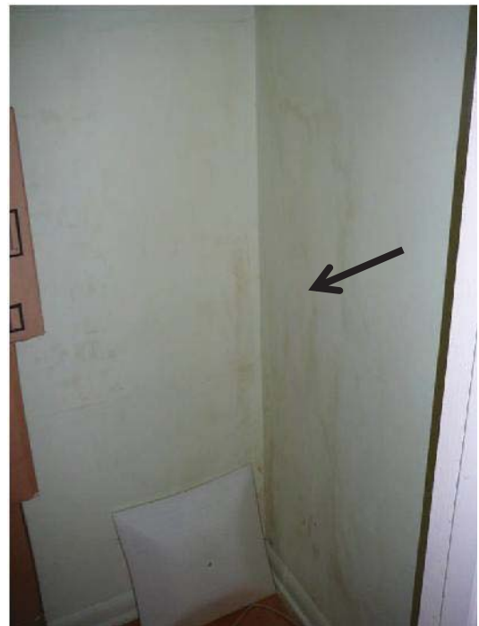
#60 Duplex House – North Unit Water damage in the conference room closet
