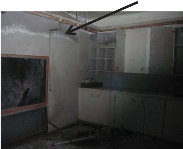
#2 Administration Office - Basement Suspected high water mark from flooding
