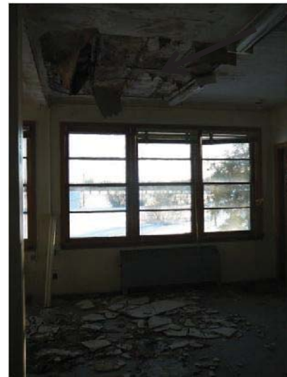
#2 Administration Office – 2 nd Floor Water Damage and debris from failure of the 2 nd floor ceiling
