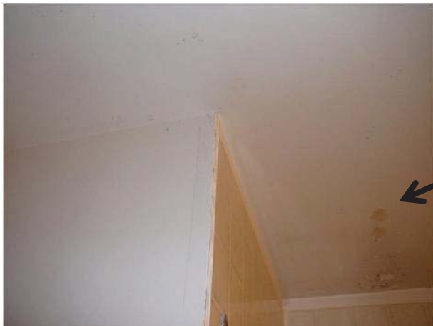
#60 Duplex House – North Unit Water damage in the washroom
