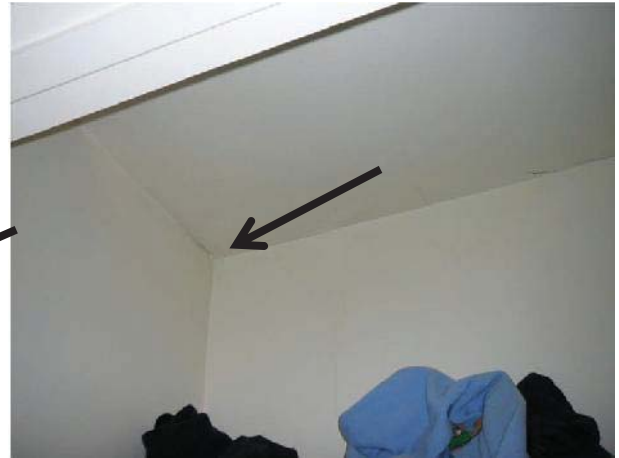
#60 Duplex House – South Unit Water damage in the northwest bedroom closet
