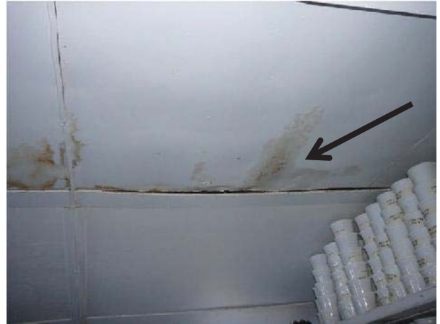
#14 Drying and Threshing Shed Water damaged ceiling
