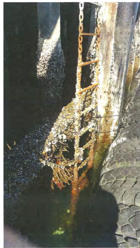
14. CHAIN LADDER AT NORTH BERTH
