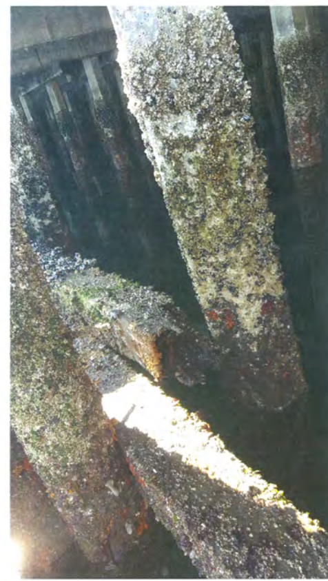
9. HEAVY MARINE GROWTH, BROKEN LOWER WALER BEAM AT THE WEST END OF THE NORTH BERTH
