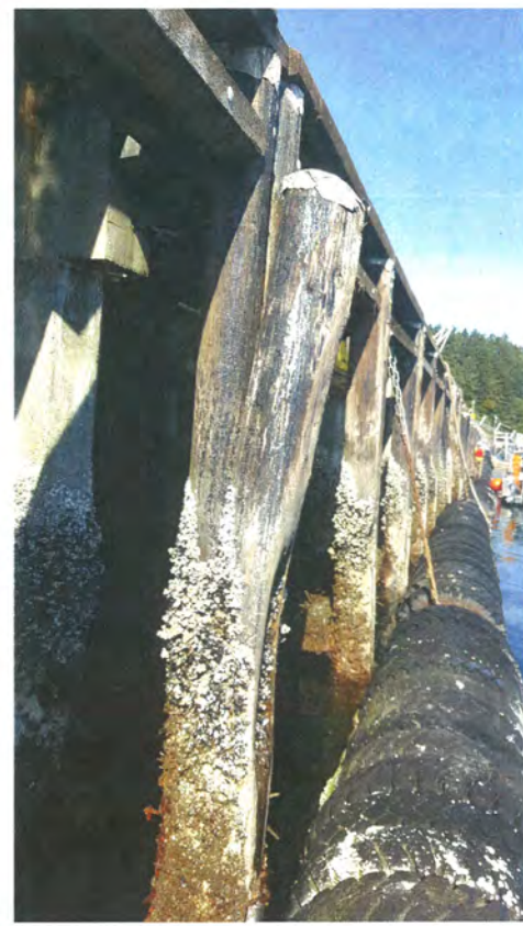
10. HEAVY WEAR ON RUBBING POLES AT NORTH BERTH
