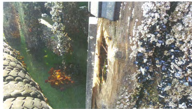
5. HEAVILY WORN TIMBER RUBBING POLE AT NORTH BERTH
