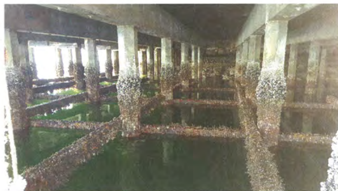
4. LATERAL BRACING (NE CORNER) VISIBLE AT LOW TIDE
