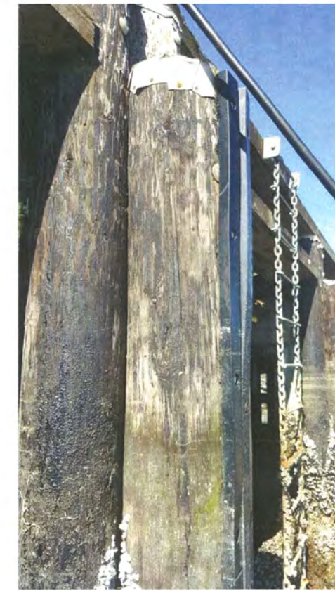
16. WEAR STRIPS ON RUBBING POLES AT EAST BERTH
