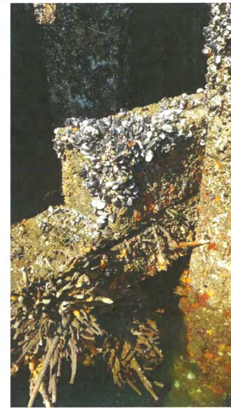
15. HEAVY MARINE GROWTH ON LOWER TIMBER WALER
