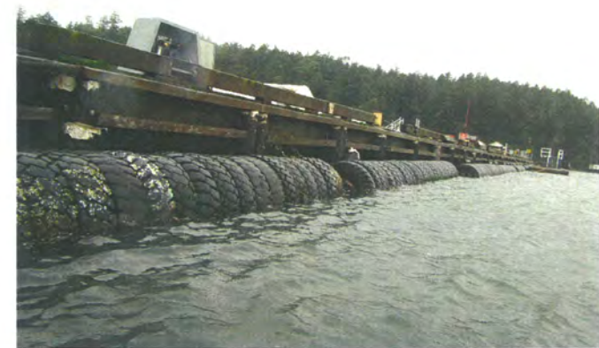
1. NORTH BERTH FENDER SYSTEM
