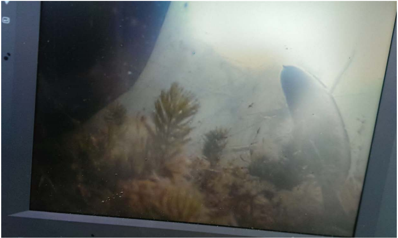
Photo 45: Underwater camera to assess placement of geotextile curtain on bottom of marsh.
