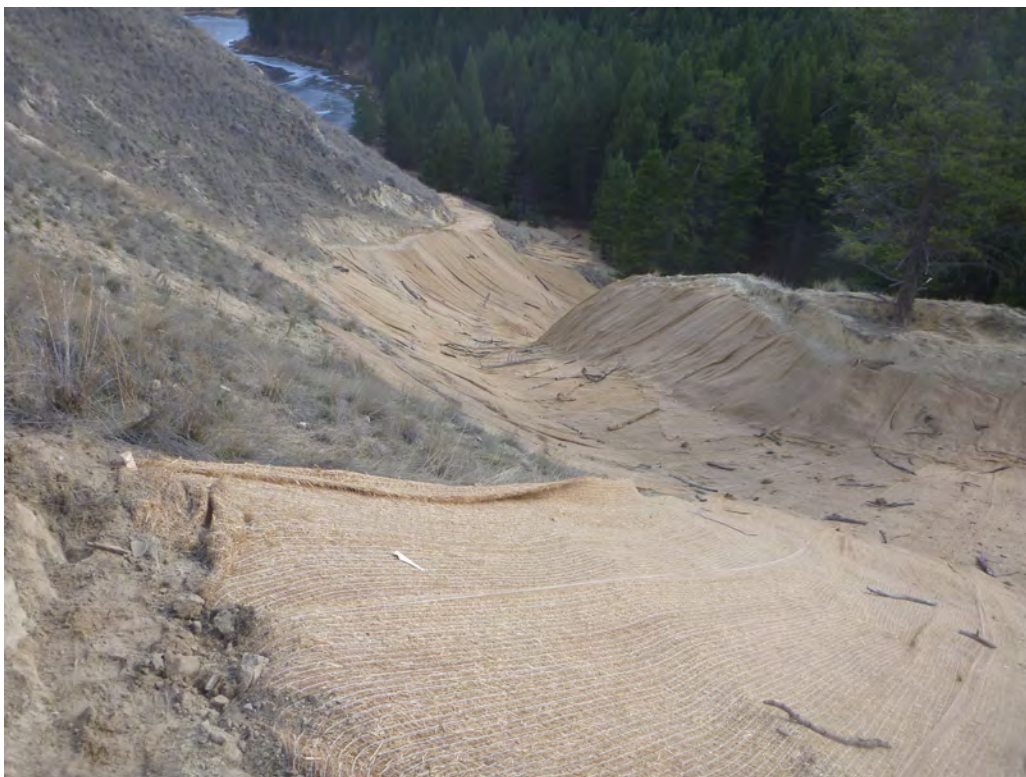
Photo 8: Final site completion with installed Erosion Control Blanket and Coarse Woody Debris (Mar. 13, 2015)
