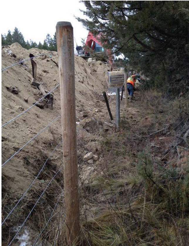
Photo 83: Cleanup of material that had moved from the stockpile back onto the NWA.
