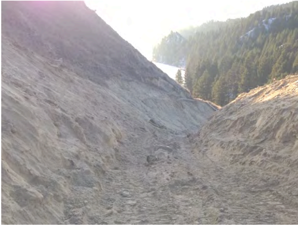
Photo 3: MDZ excavation developed a gully feature between the trees (exclusion zone) and the north slope. (Mar. 5, 2015).
