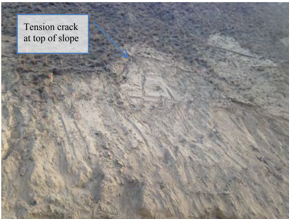
Photo 4: View of tension crack that developed along the north slope on Mar. 5, 2015
