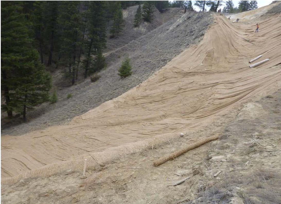
Photo 99: Erosion control blanket keyed in at top of excavation and sloping downward to channel water to lower gully.
