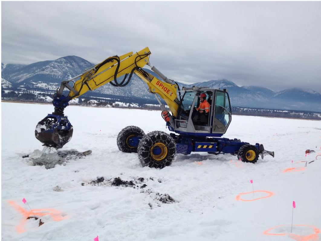
Photo 59: Debris removal on ice by spider hoe at locations identified by electromagnetic survey.
