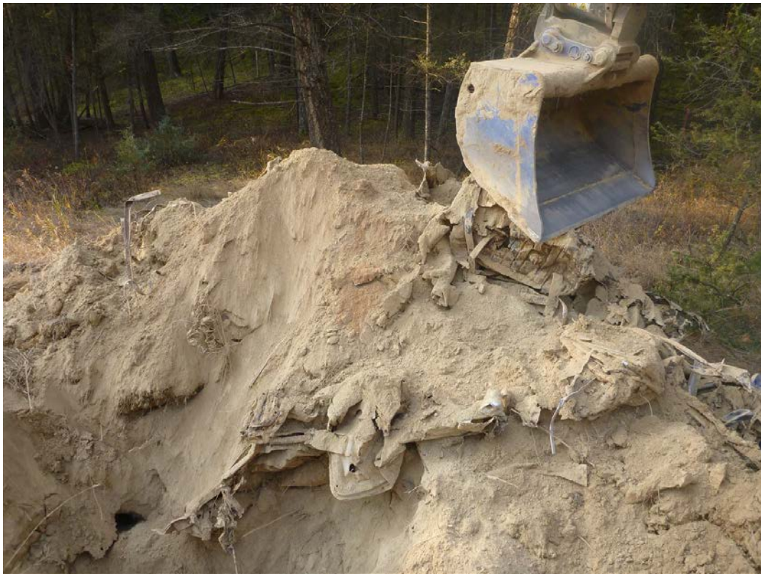
Photo 30: TP11 – Debris removed from test pit.
