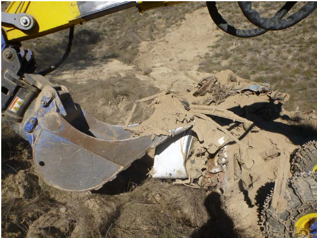
Photo 15: TP7 - Metal debris observed throughout excavation.
