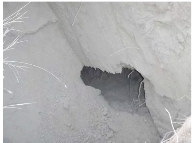
Photo 5: Lower view of void encountered along outslope of lower trail
