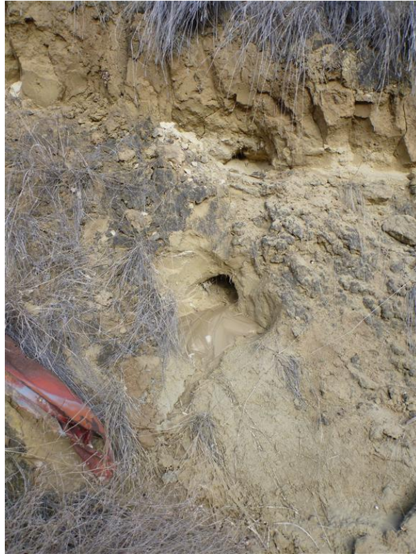
Photo 57: Void outlet and saturated soil (March 2014)
