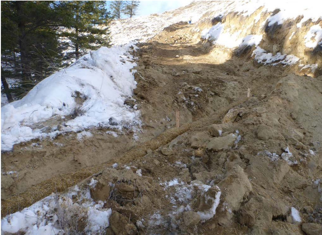
Photo 71: Temporary diversion ditches and wattles placed along lower trail until re-contouring work complete.
