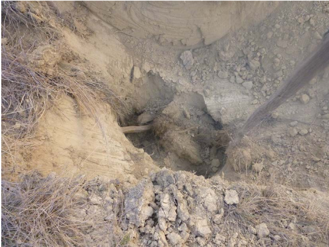
Photo 24: Excavation in area of cavity and water flow – found deep cavity in trail.
