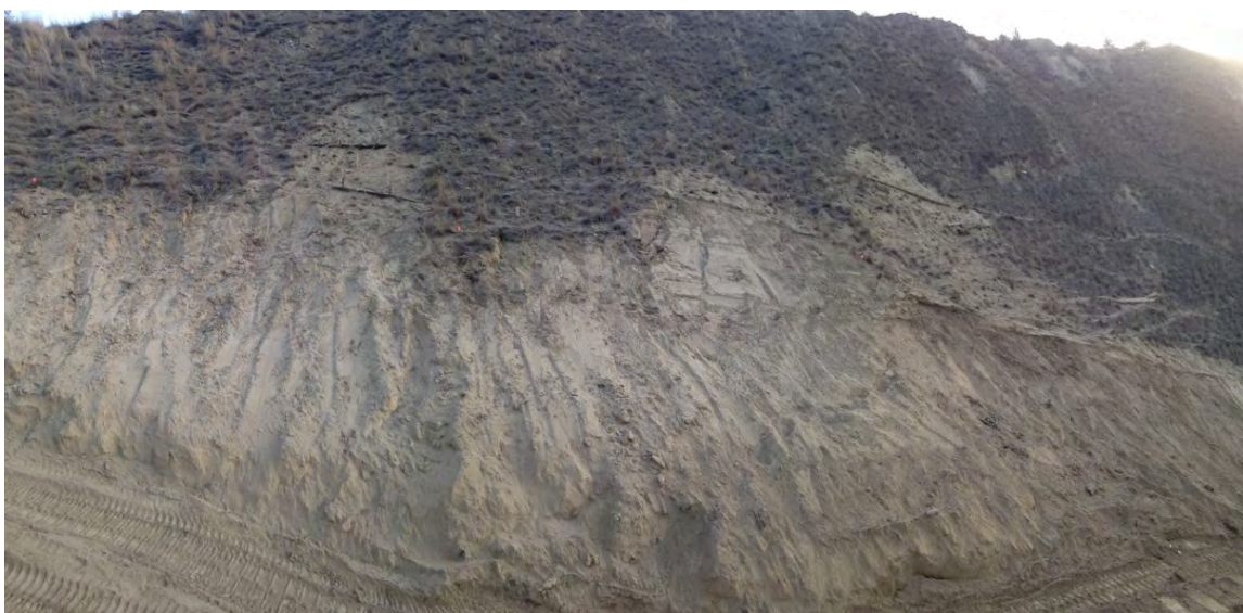
Photo 2: View of the north slope of the MDZ excavation, showing 1H:1V slopes approximating the upslope grade. (Mar. 5, 2015).
