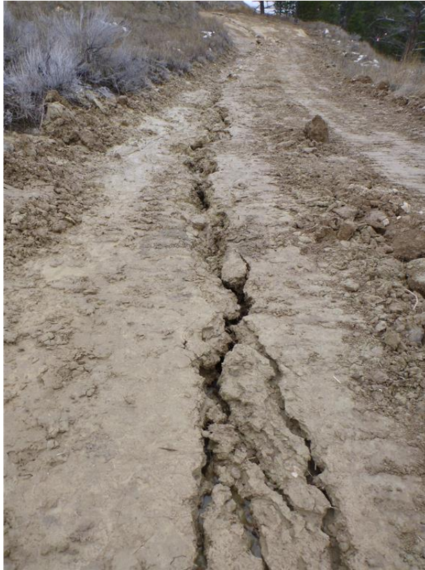
Photo 75: Erosion channels following rapid snowmelt.
