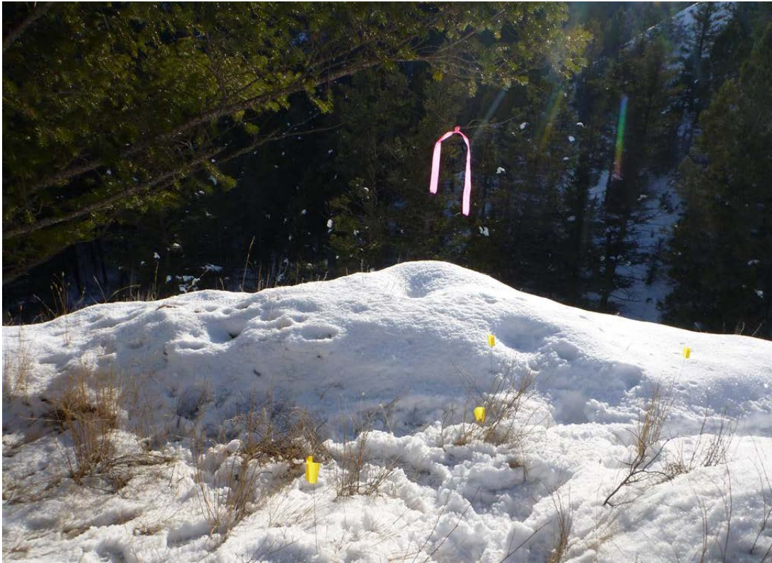
Photo 57: Prior to remedial works, wildlife trees marked with pink flagging and exclusion zones with yellow flagging.
