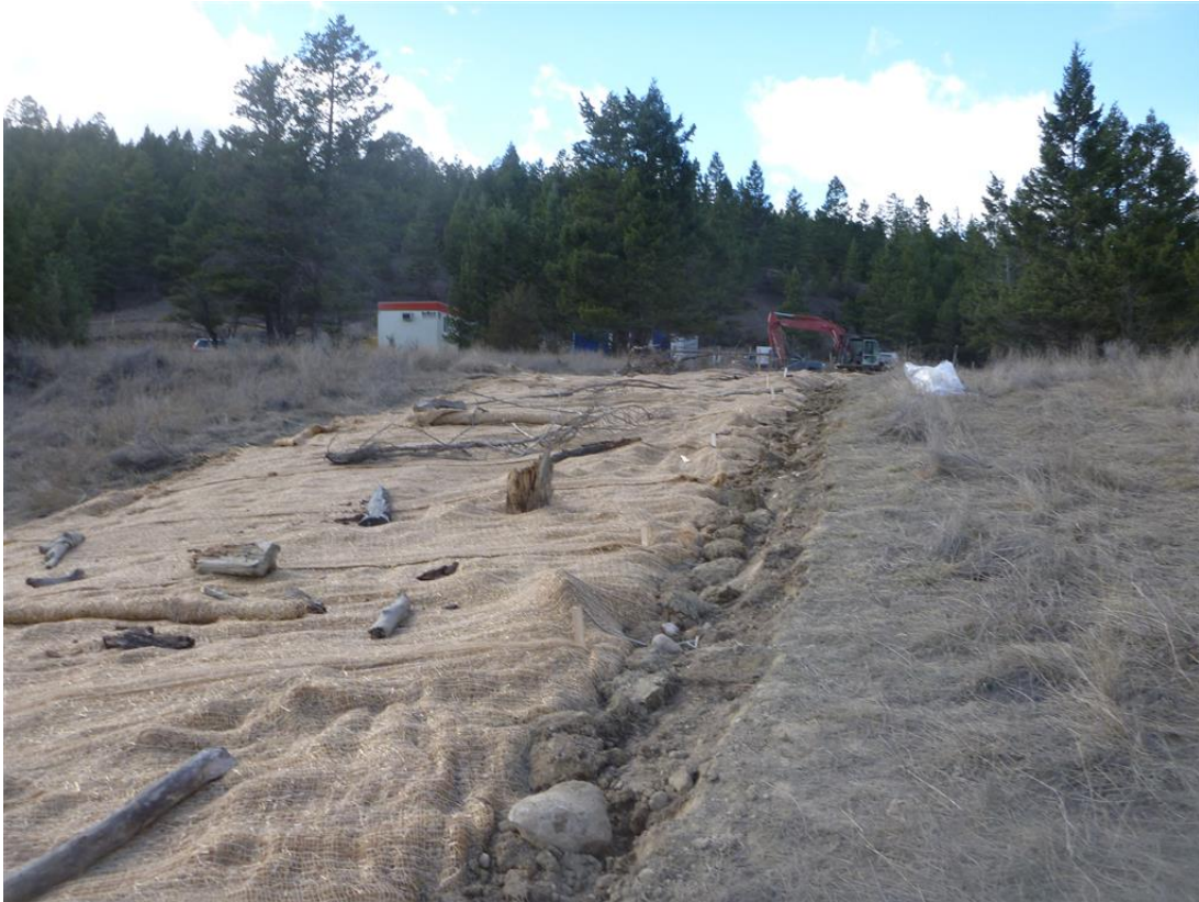
Photo 105: Trail area restored to fence line. Keyed in at north side of trail and staked at south side.
