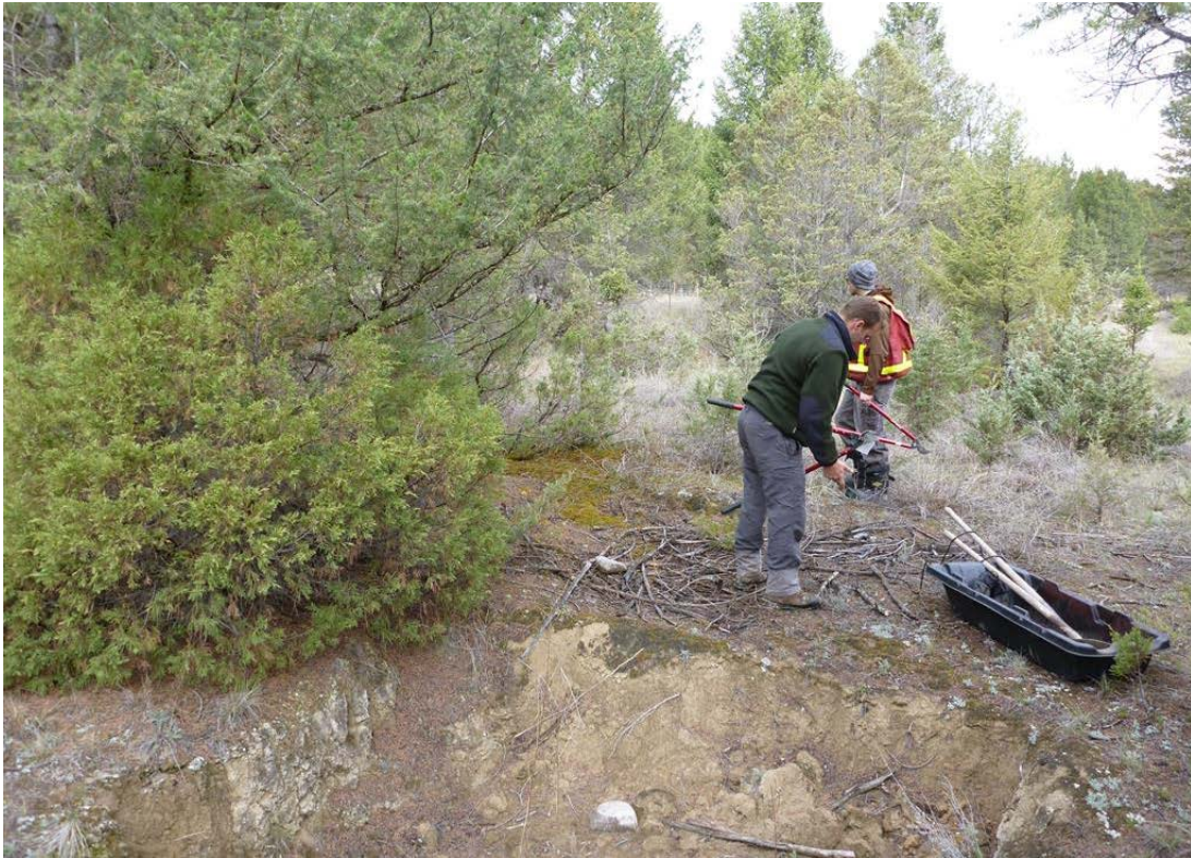
Photo 1: Collection of woody debris to be used as stakes for installation of coir matting.
