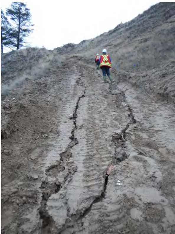
Photo 1: Erosional gullies that formed along the trail after the runoff event of Feb. 6, 2015 (Feb. 7, 2015)
