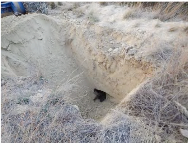
Photo 4: Upper view of void encountered along access trail
