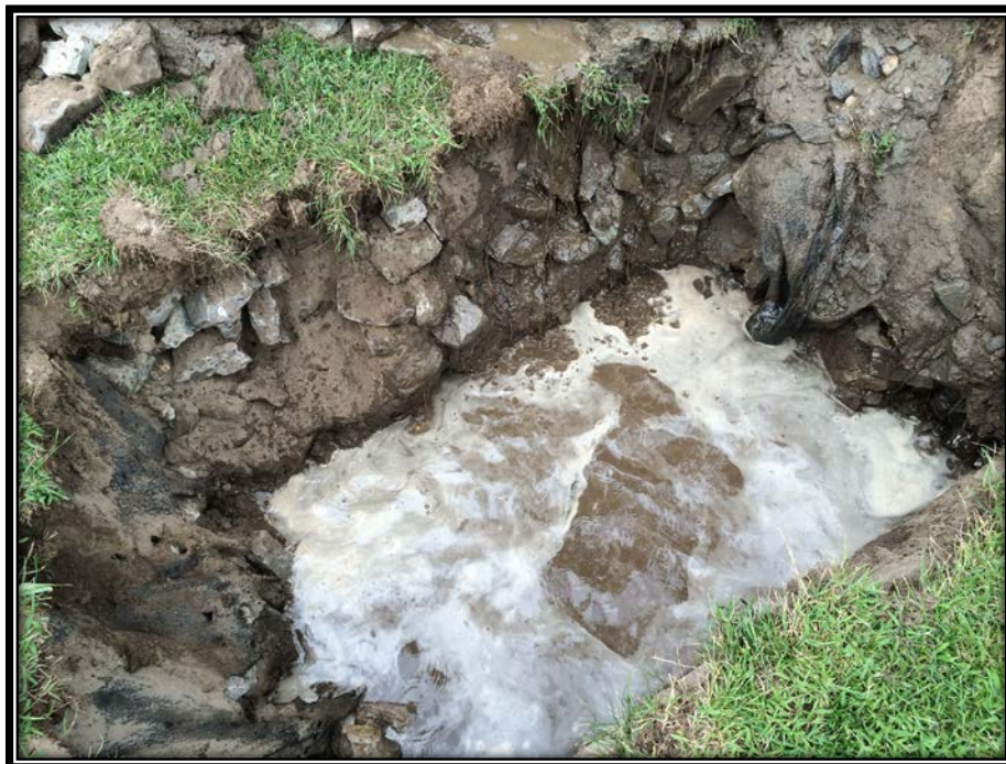
Figure 14 –TP7-N, overburden material, geotextile fabric – note geotextile fabric on edges of test pit
