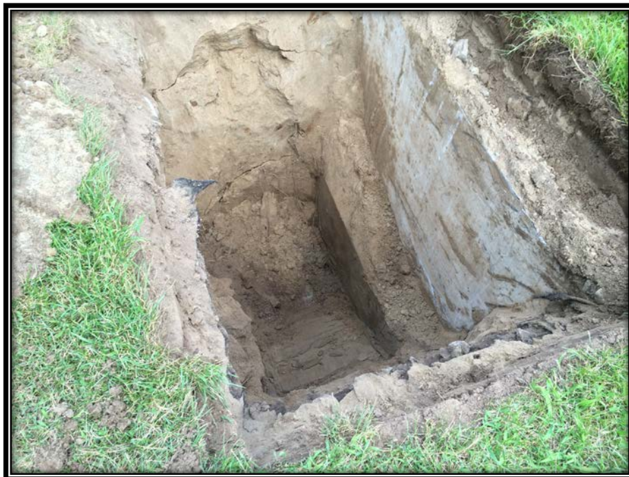
Figure 16 – TP8-N, concrete retaining wall and overburden, termination on bedrock – note geotextile fabric on edges of test pit
