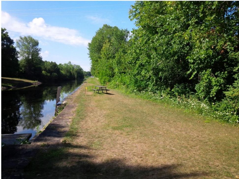
Photo 1. Earth dam and masonry/concrete wall at Upper Nicholsons – looking towards the weir from the lock (July 2016).
