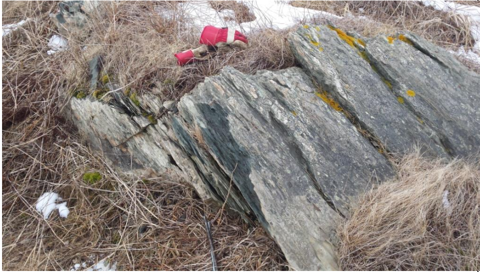
Photo 17: Outcrop F located ~ 35 m NE of approximate location of Turbine 14-03. Note close spacing of cleavage planes with some surface fracturing.
