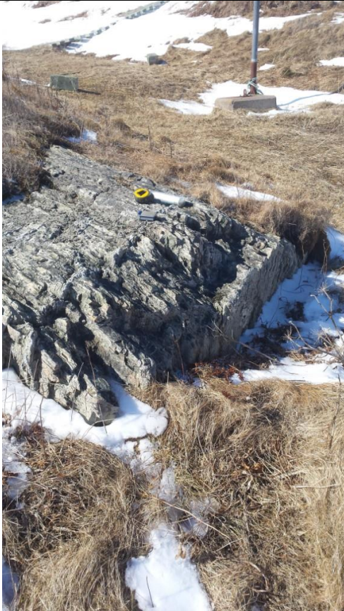
Photo 5: Outcrop B – near proposed location of Turbine 14-01. Located ~ 3 m west of the existing west anchor block. Note close spacing of joints / cleavage planes with some surface fracturing.
