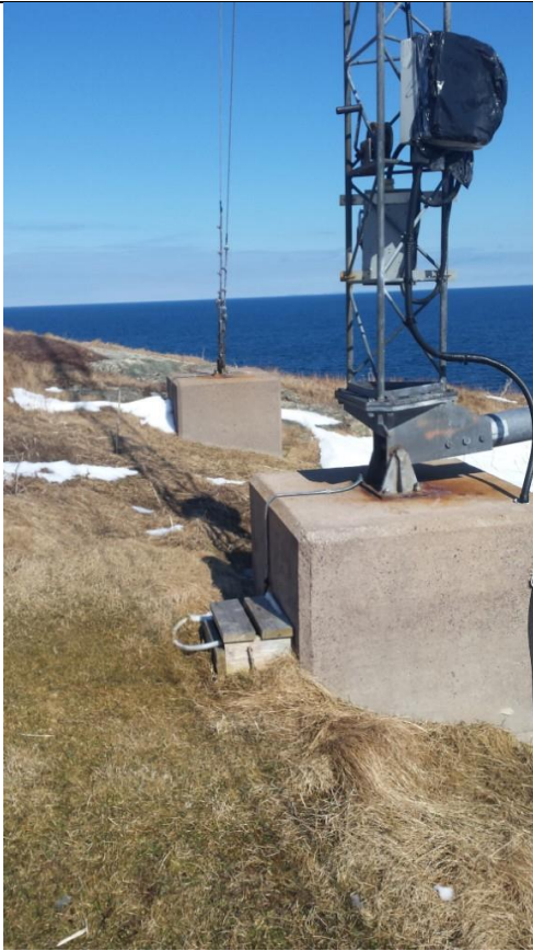
Photo 1: Existing Turbine & Concrete Support Blocking. Existing Turbine to be decommissioned and replaced with Turbine 14-01.
