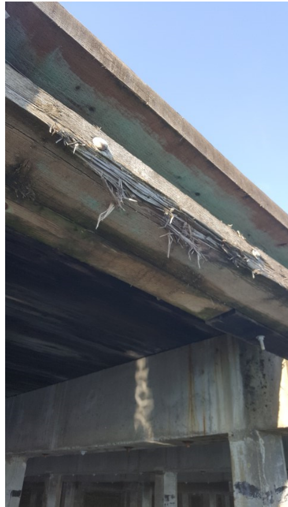
Photo 6: Abrasion damage on timber chock beam
