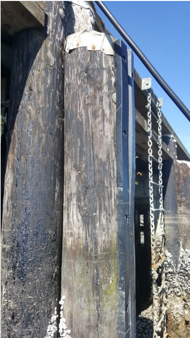
Photo 3: Fender pile in excellent condition
