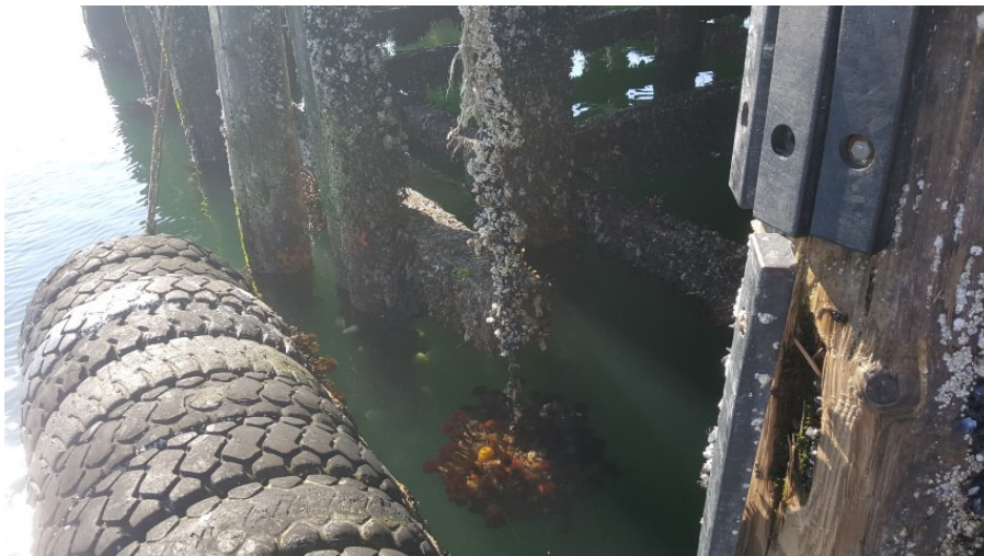
Photo 2: Lower waler missing at North Berth – Pile Group 3, abrasion damage, rubbing strip partially dislodged
