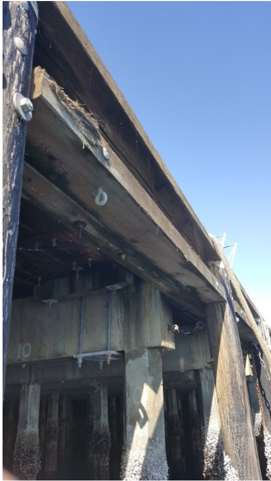
Photo 3: Minor damage to chock beam
