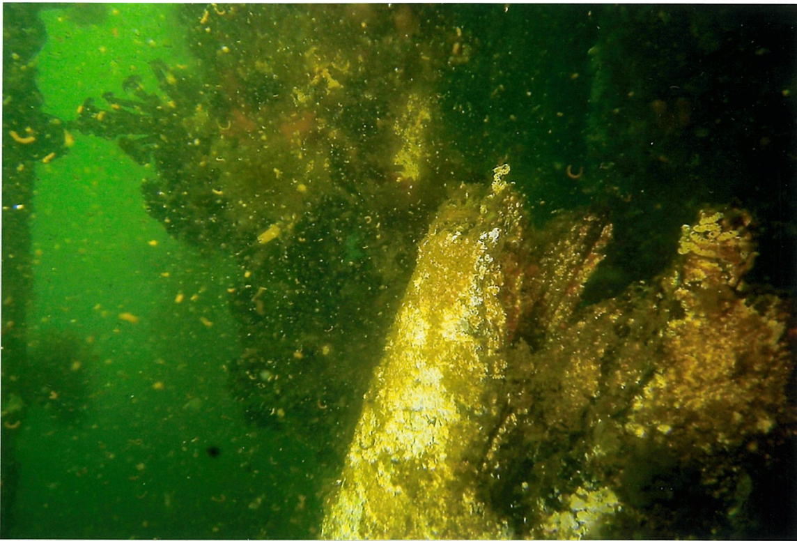
PILE GROUP 17A PILE #1 SEVERED PILE
