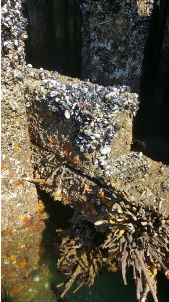
Photo 5: Longitudinal cracking in lower water
