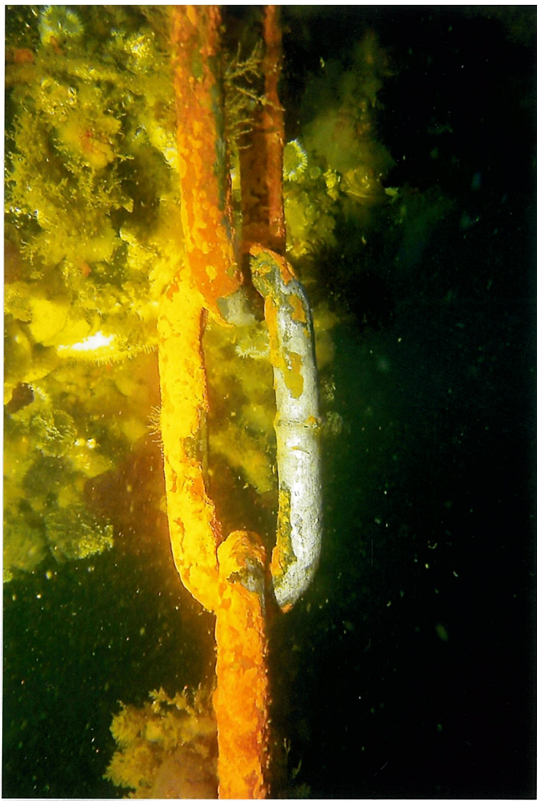
OVERALL TREE SAVER MOORING CHAIN CONDITION
