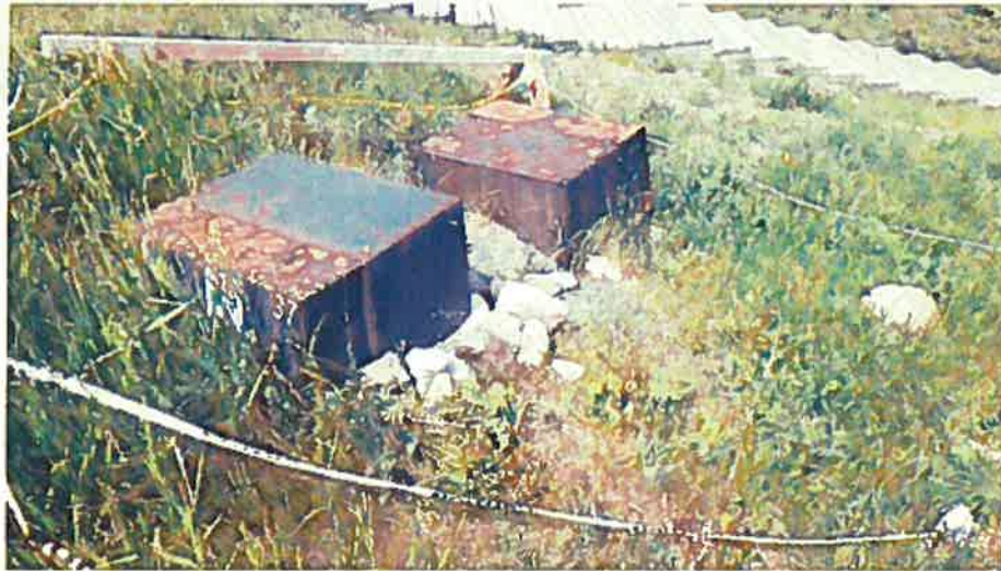
Figure 2 Transformers to be Decommissioned and Replaced
