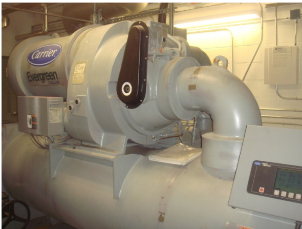
Figure 8: Chiller Plant, 300 ton Carrier Chiller M-1 Mechanical room
