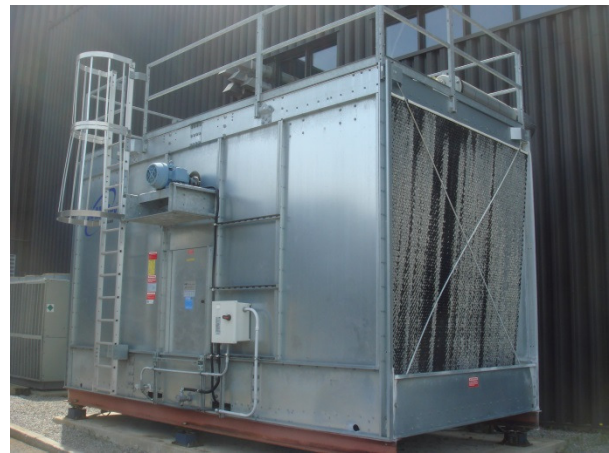
Figure 9: Chiller Plant, Cooling Tower
