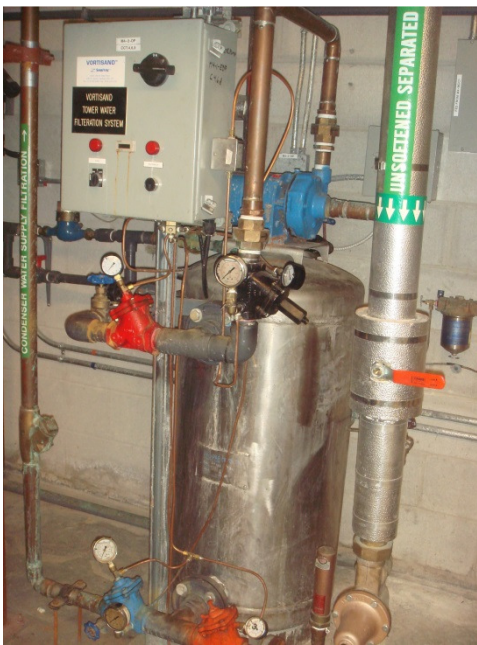
Figure 13: Vortisand Filtration System (S/N MR161) in Mechanical room M4
