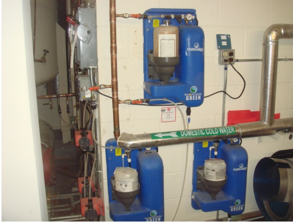
Figure 11: Chemical Treatment Station in M-1 Mechanical room
