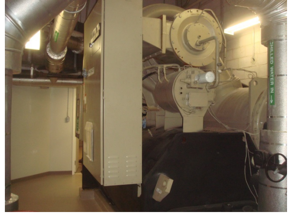
Figure 7: Chiller Plant, 500 ton TRANE CVHE Chiller in M-4 Mechanical room
