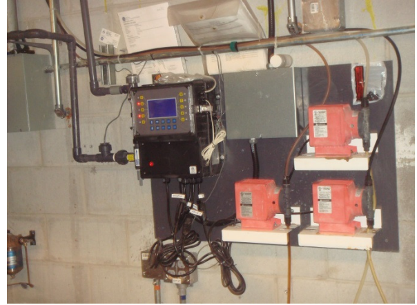
Figure 12: Chemical Treatment Station in M-4 Mechanical room
