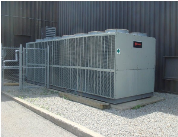
Figure 10: Chiller Plant, 200 ton RTAA dry-cooler
