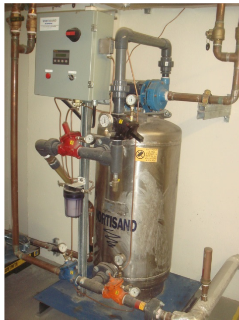
Figure 14: Vortisand Filtration System (S/N MR431, standby) in Mechanical room M1
