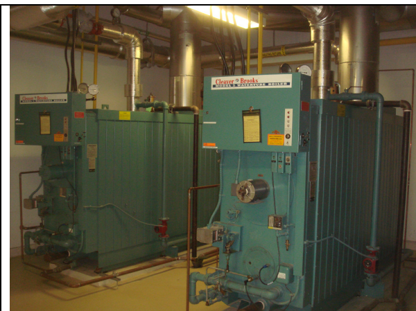
Figure 6 : Installation de chauffage
