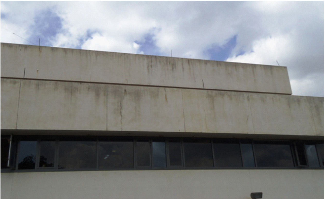
S-11: Vertical Cracks on Parapet Walls
