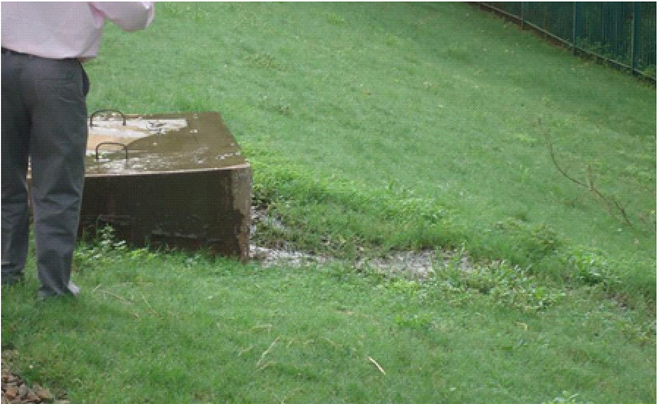
BG-3: Overflowing septic at the back area
