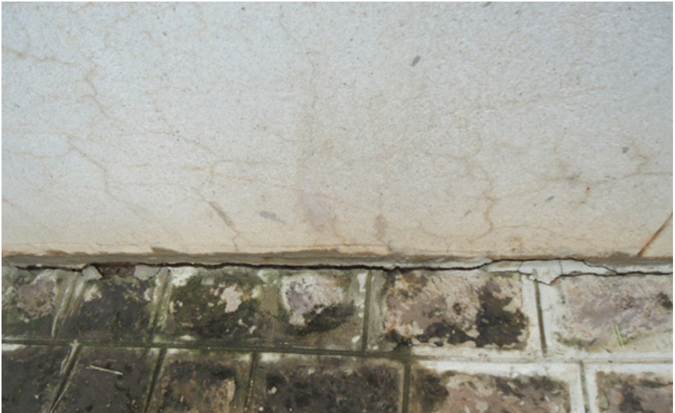
S-23: Separation of Retaining wall from floor
