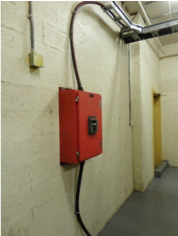
ES-8: Fire Pump Disconnect
