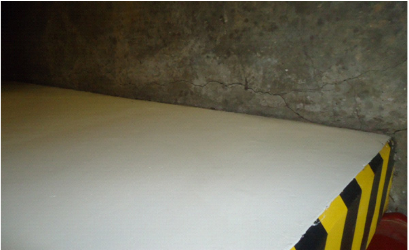
S-2: Cracks on Basement floor slab
