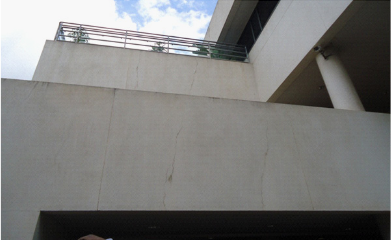
S-27: Cracks on exterior walls
