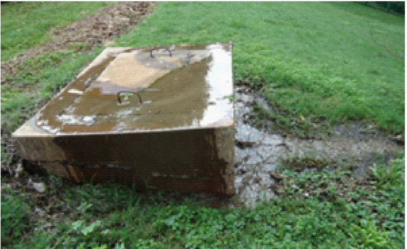
MS-20: Overflowing septic tank
