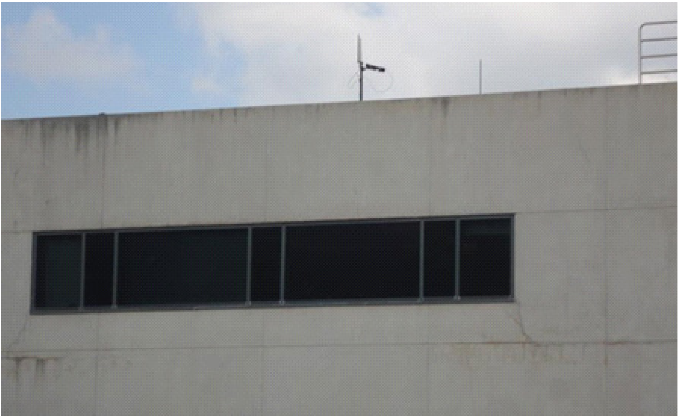
BE-4: Wall without copping drip
