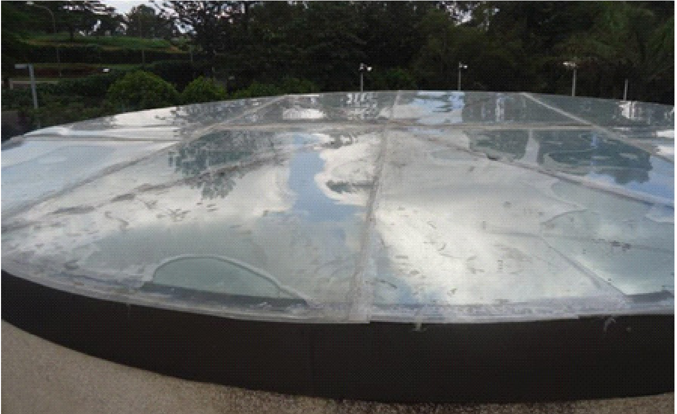
BE-5: Sky light, damaged glass roof assembly which requires replacement
