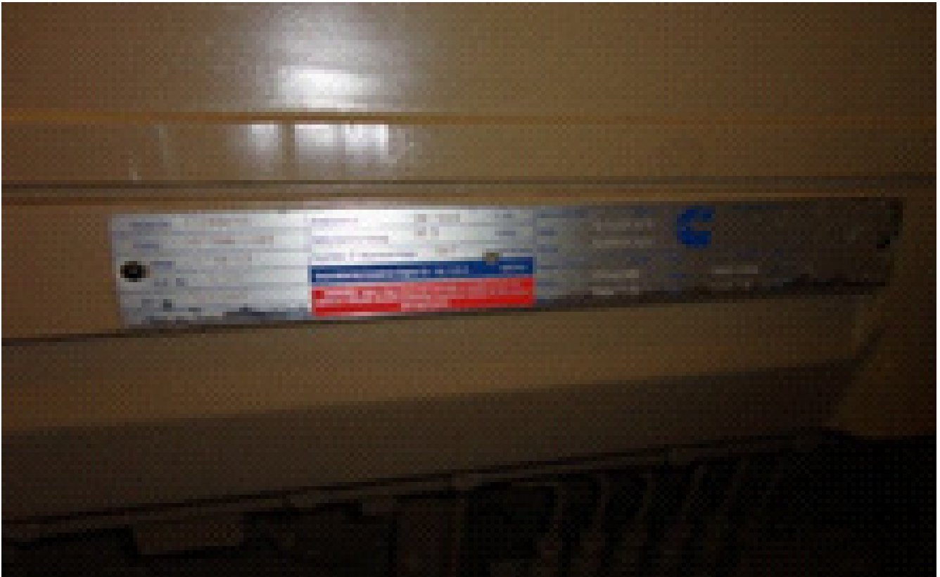
ES-7: Generator Nameplate
