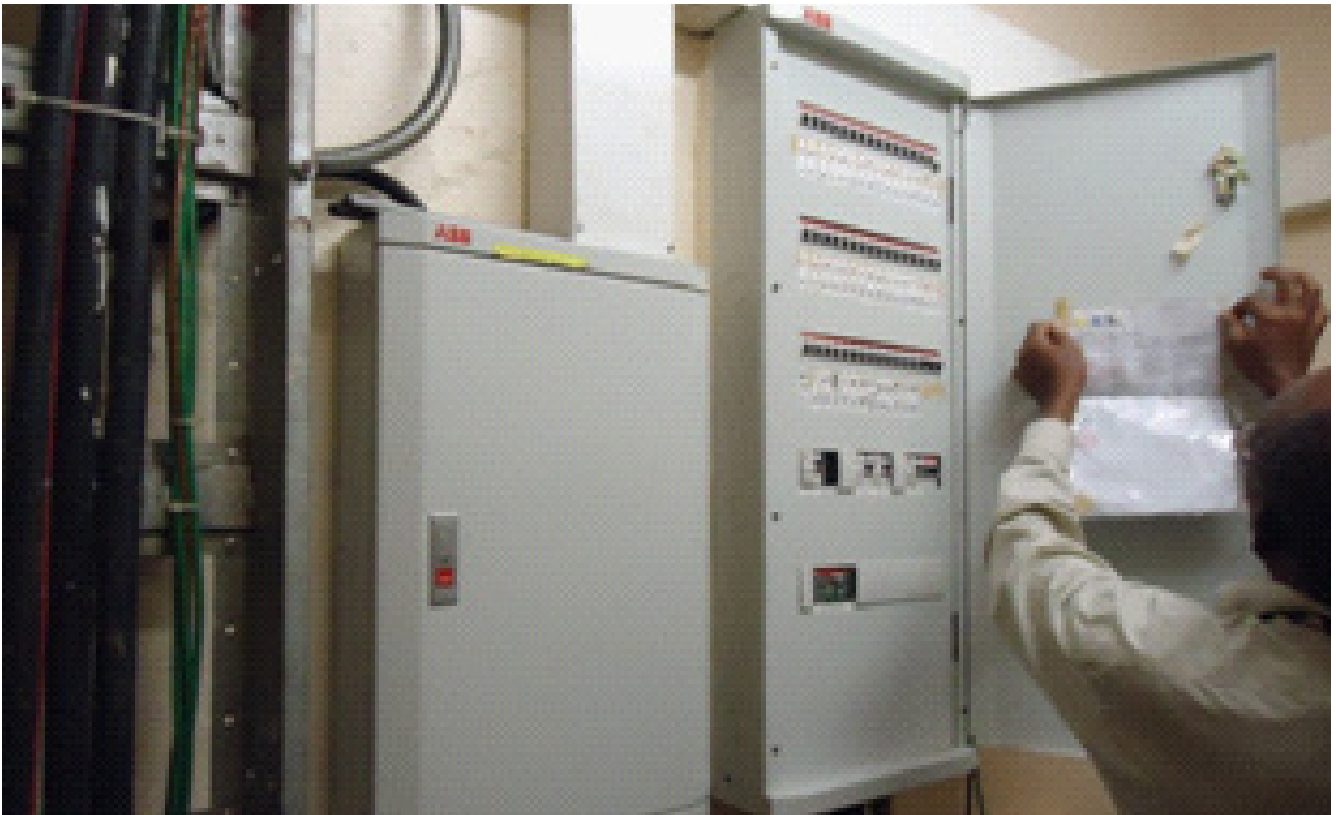
ES-14: Inside Distribution Panel
