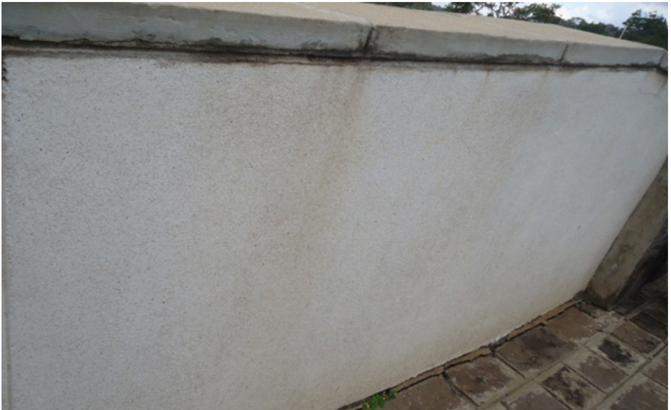
S-22: Separation of wall capping from wall
