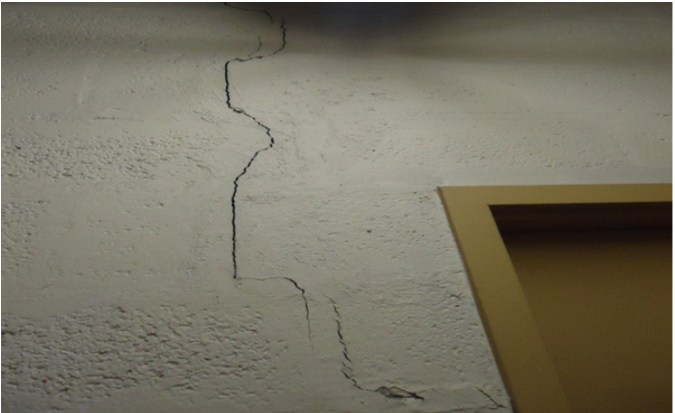
S-18: Crack on masonry wall
