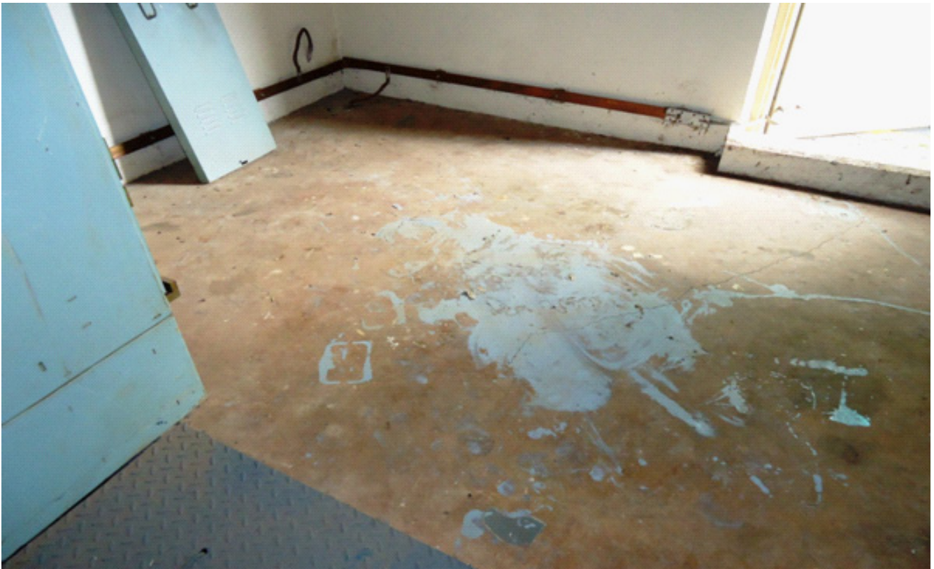
S-6: Crack on Floor Slab in Basement Electrical Transformer Room
