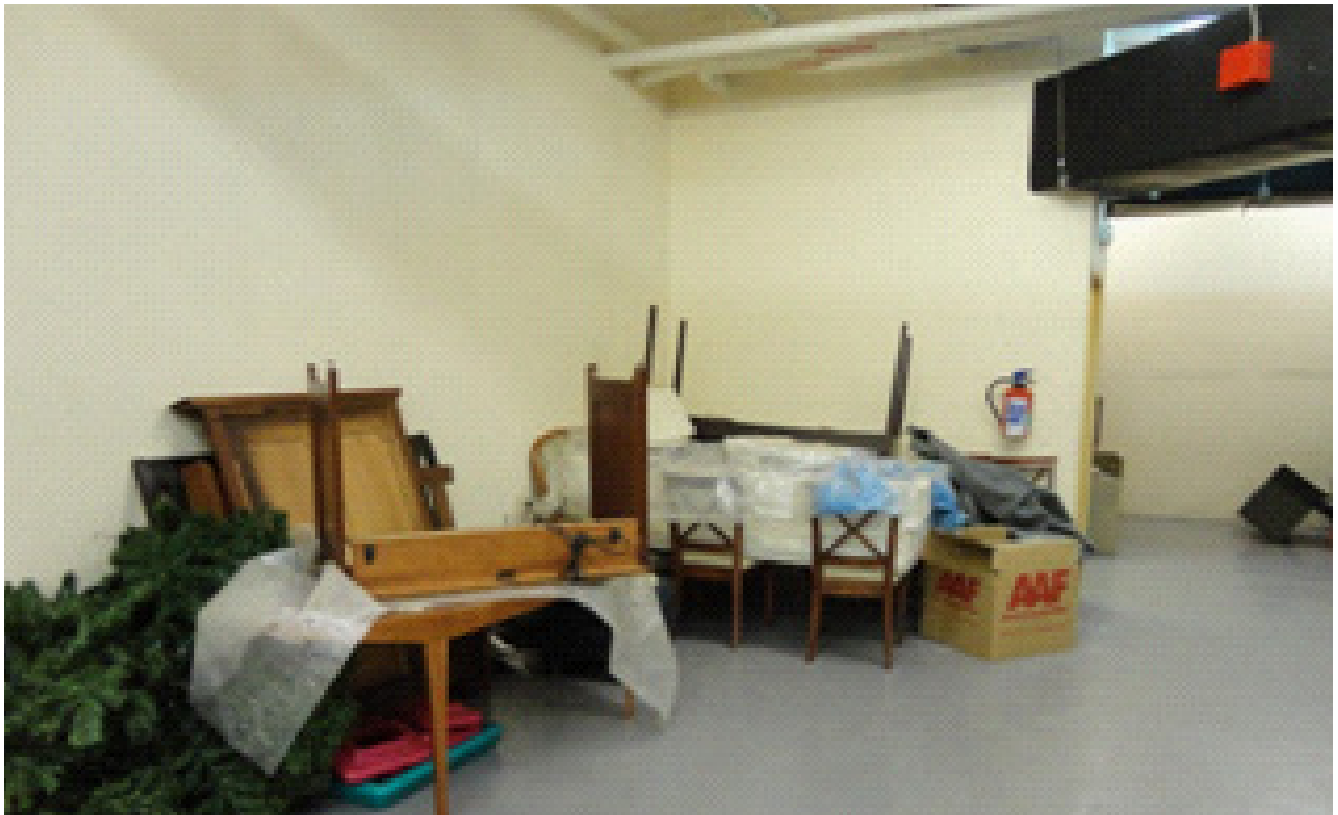
MS-4: Storage in AHU Room
