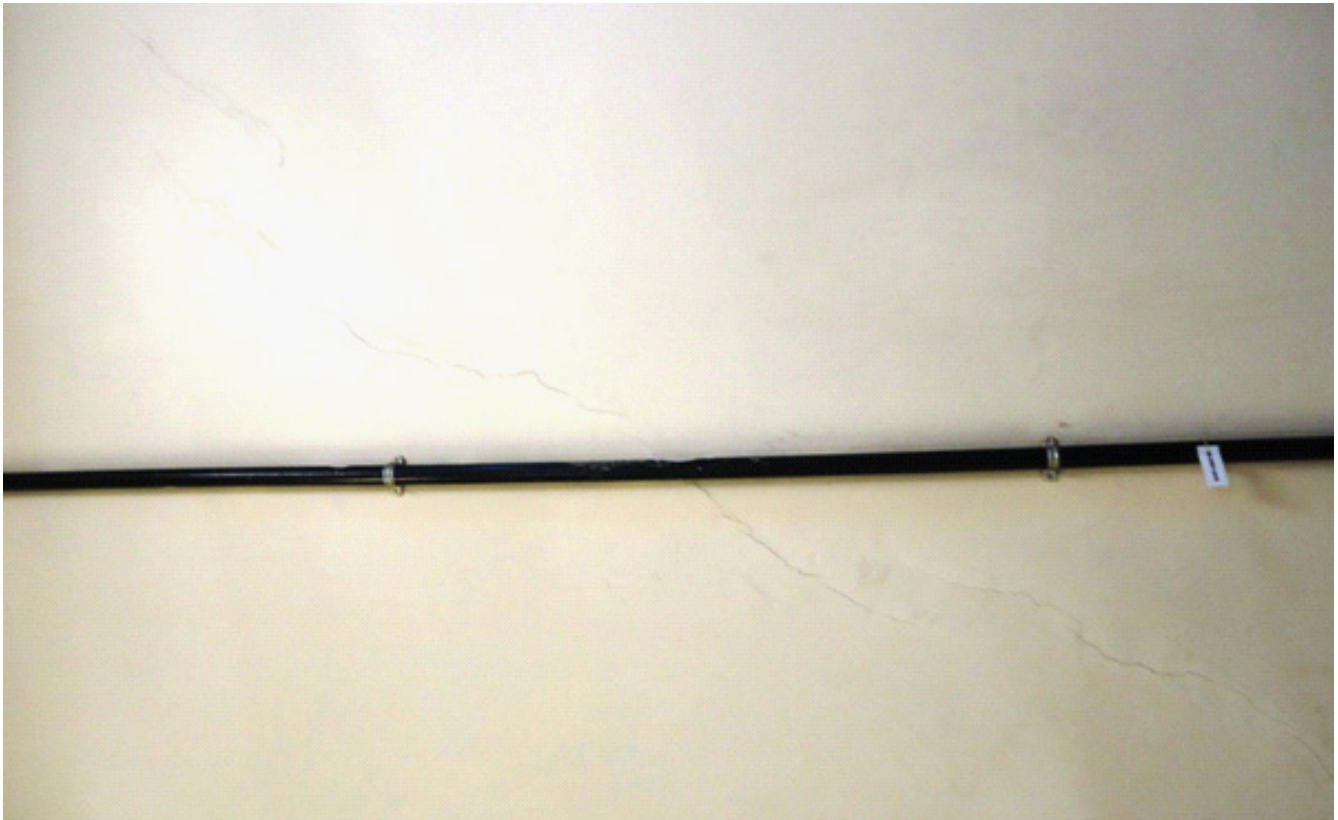
S-13: Cracks on Slab soffit on Sub-Basement Storage Area
