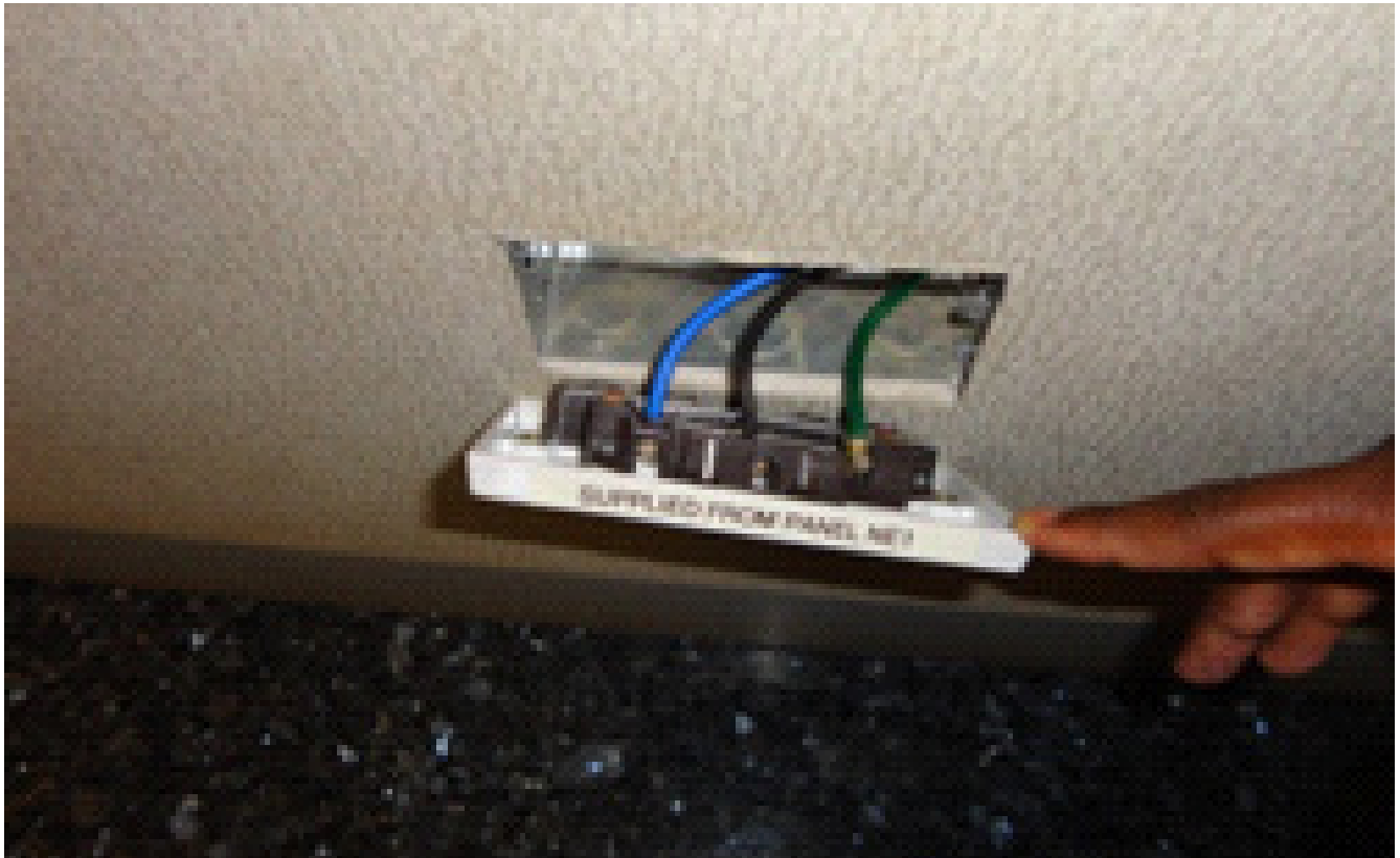
ES-3: Distribution Wiring to Socket (Receptacle), Blue Phase
