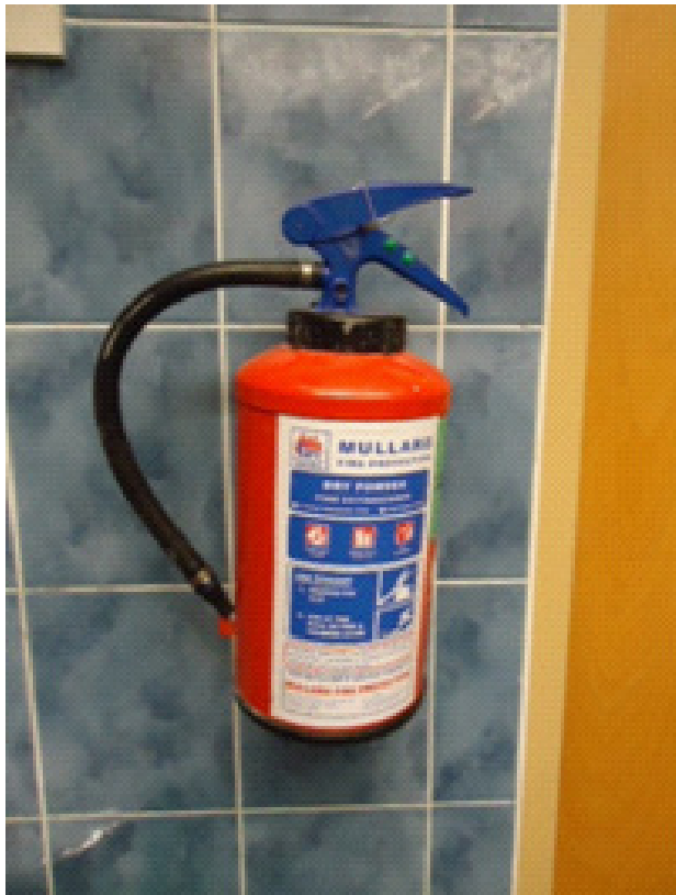
MS-24: Fire Extinguisher
