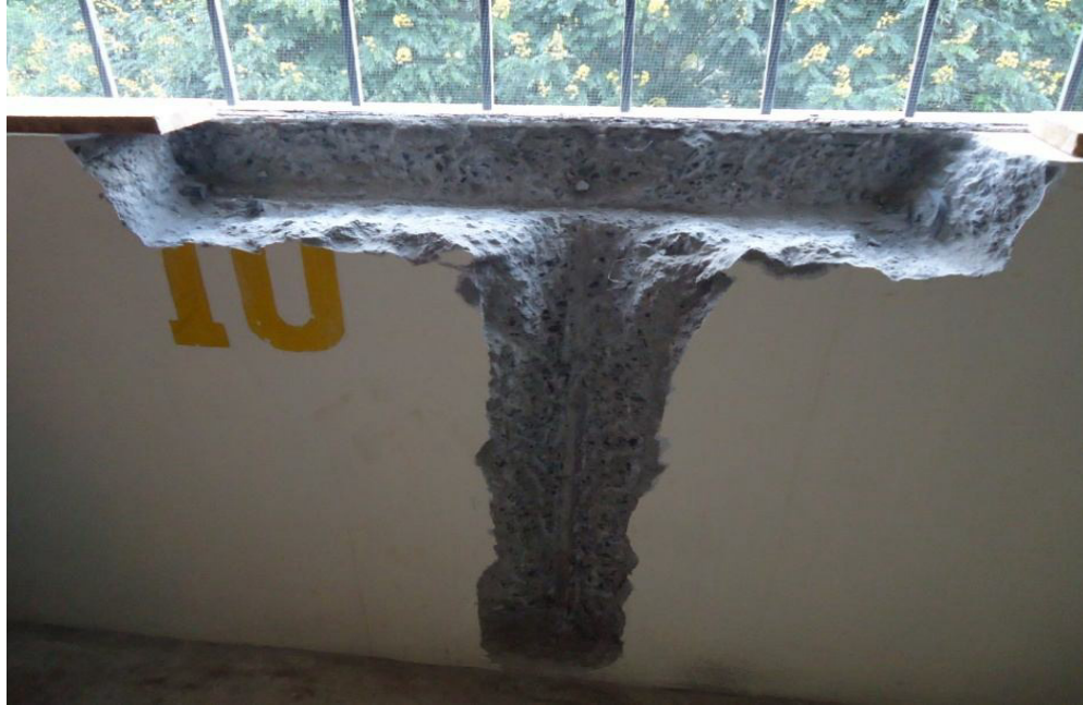
Photograph 1:- Exposed area after reinforcement bar extraction at basement level.
