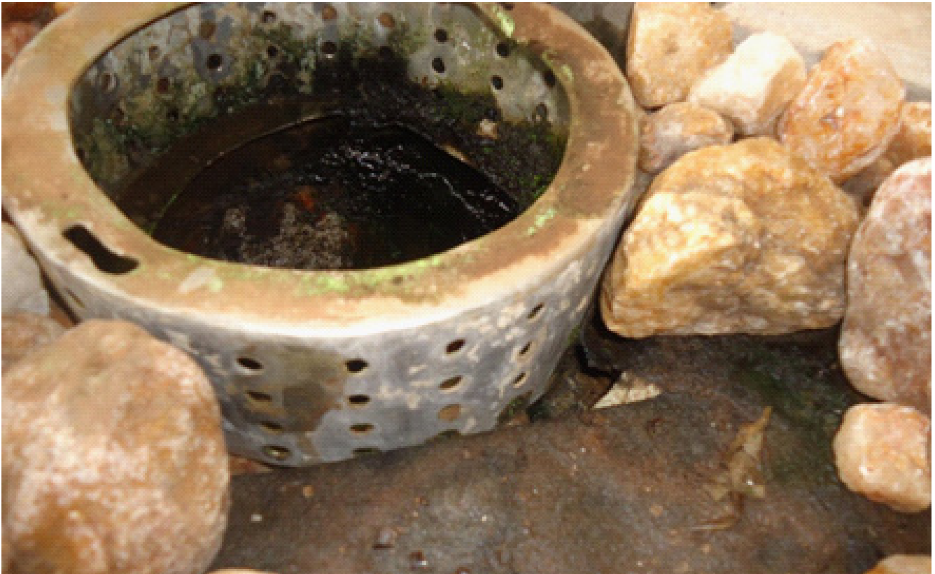
BE-1: Exposed Insulation
