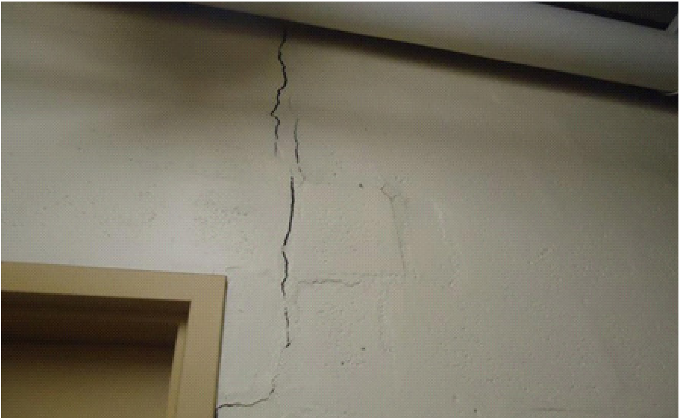
BE-13: Crack on the block work at the basement
