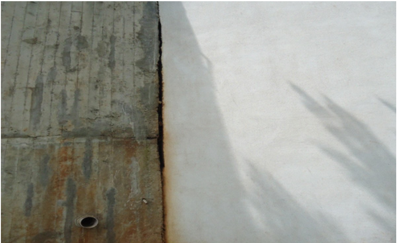
S-24: Separation of Two Retaining walls
