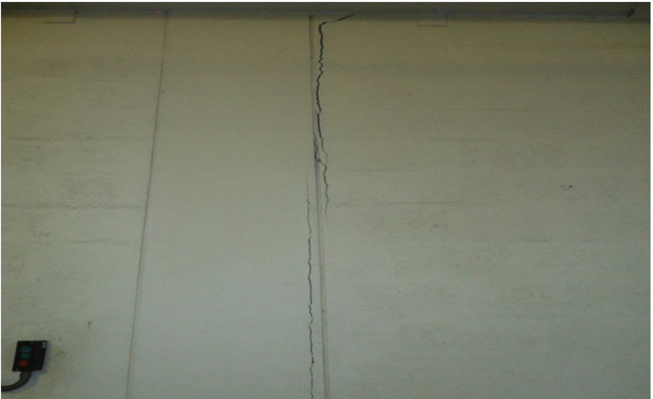
S-16: Crack on junction between masonry wall and concrete
