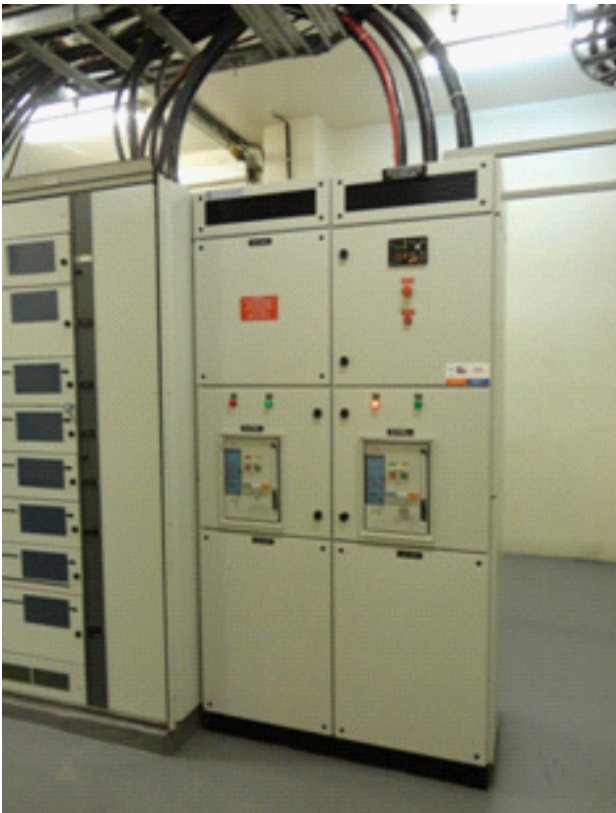
ES-2: Main Switchpanel, Additional Section
