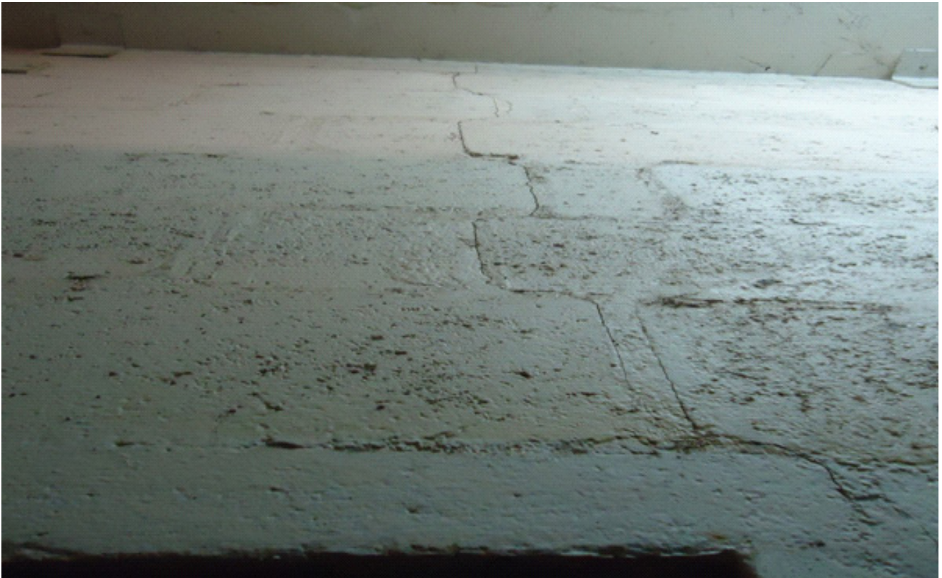
S-17: Cracks on masonry wall
