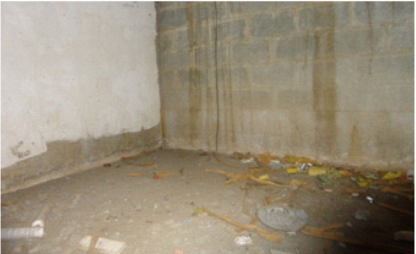
MS-6: Debris in Return Air Shaft
