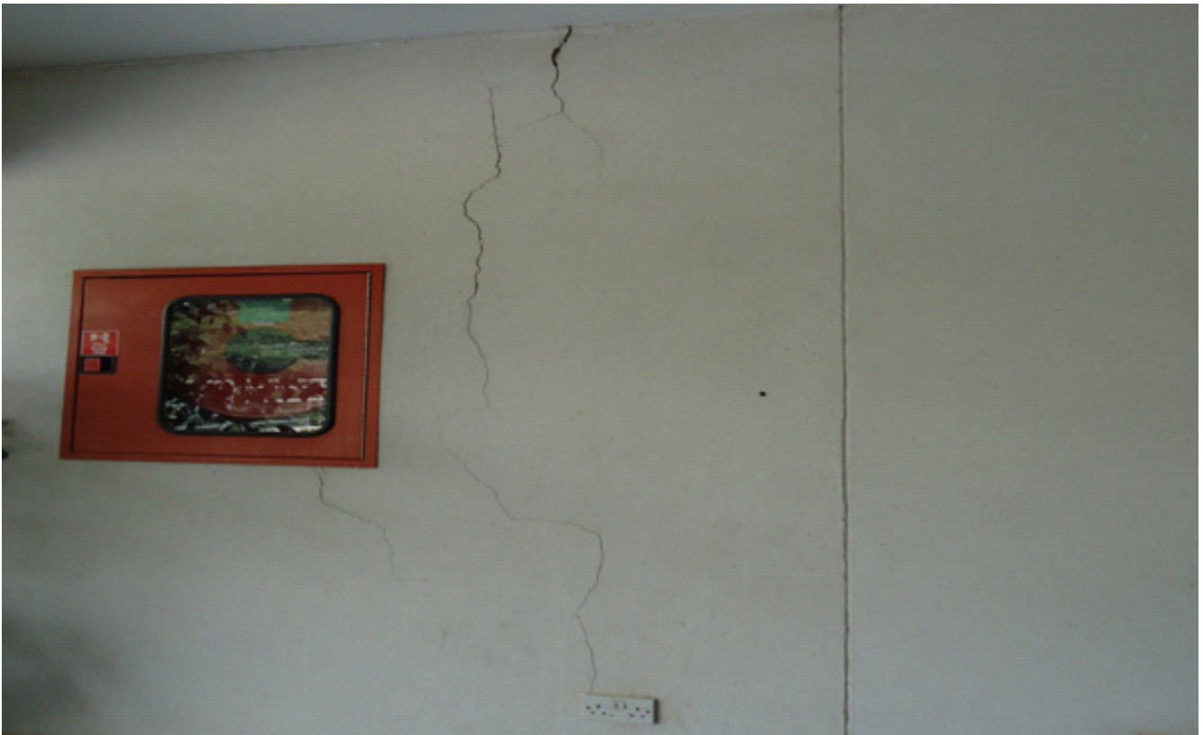
S-28: Cracks on exterior walls
