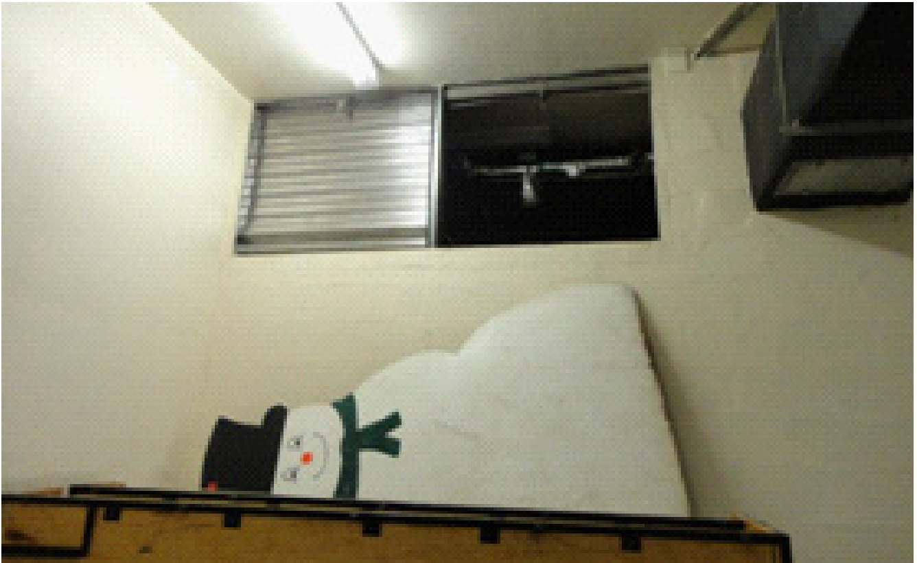
MS-7: Return Air Route with Fire Damper over Elevator Machine Room
