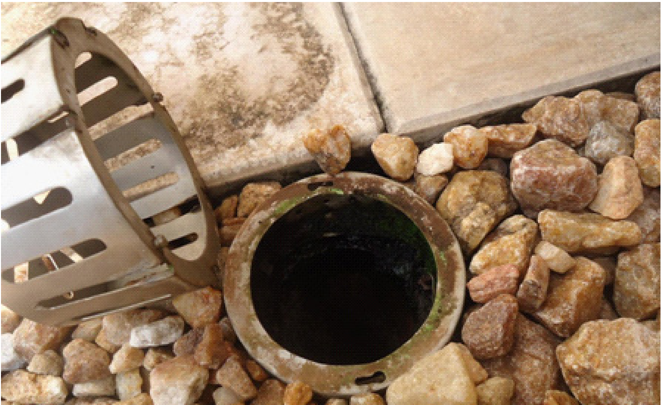
BE-2: Existing Roof Drain to be raised
