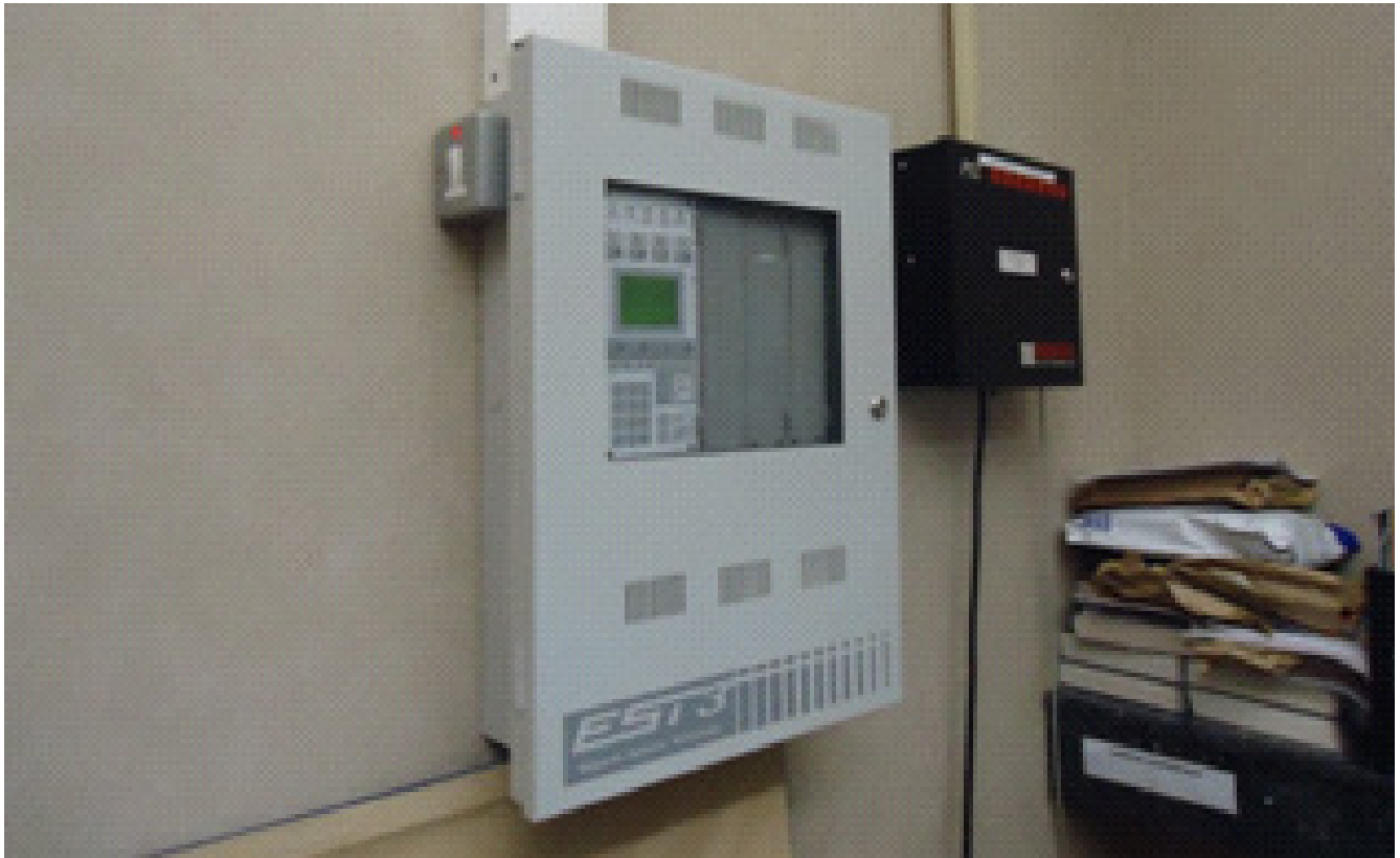
ES-15: Fire Alarm Panel
