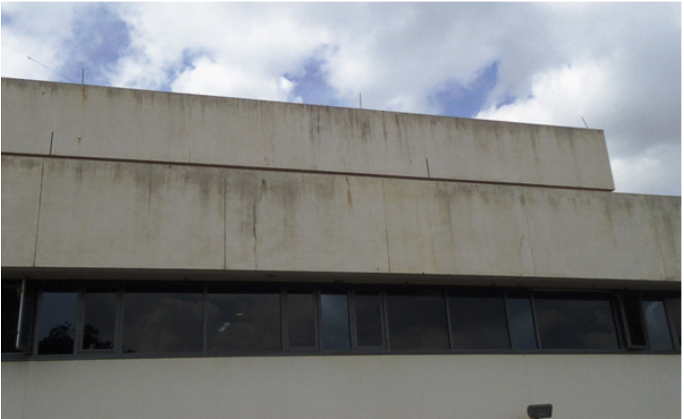
S-25: Cracks on Exterior walls
