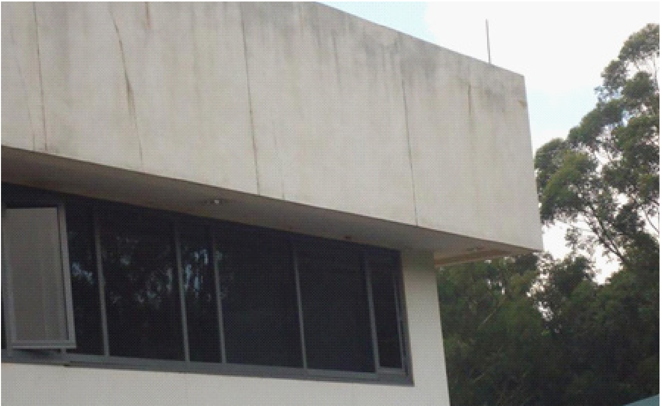
BE-3: Wall without copping drip
