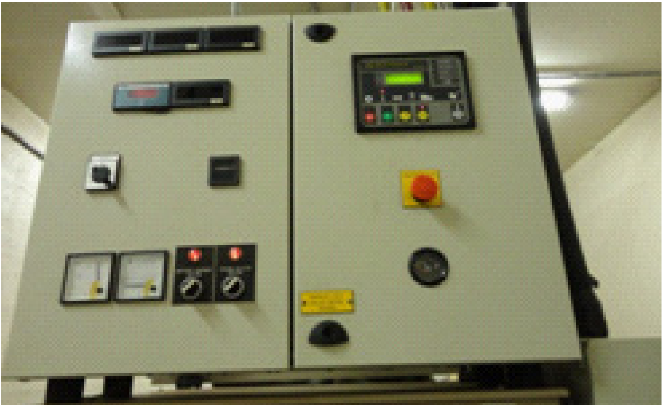
ES-6: Generator Control Panel
