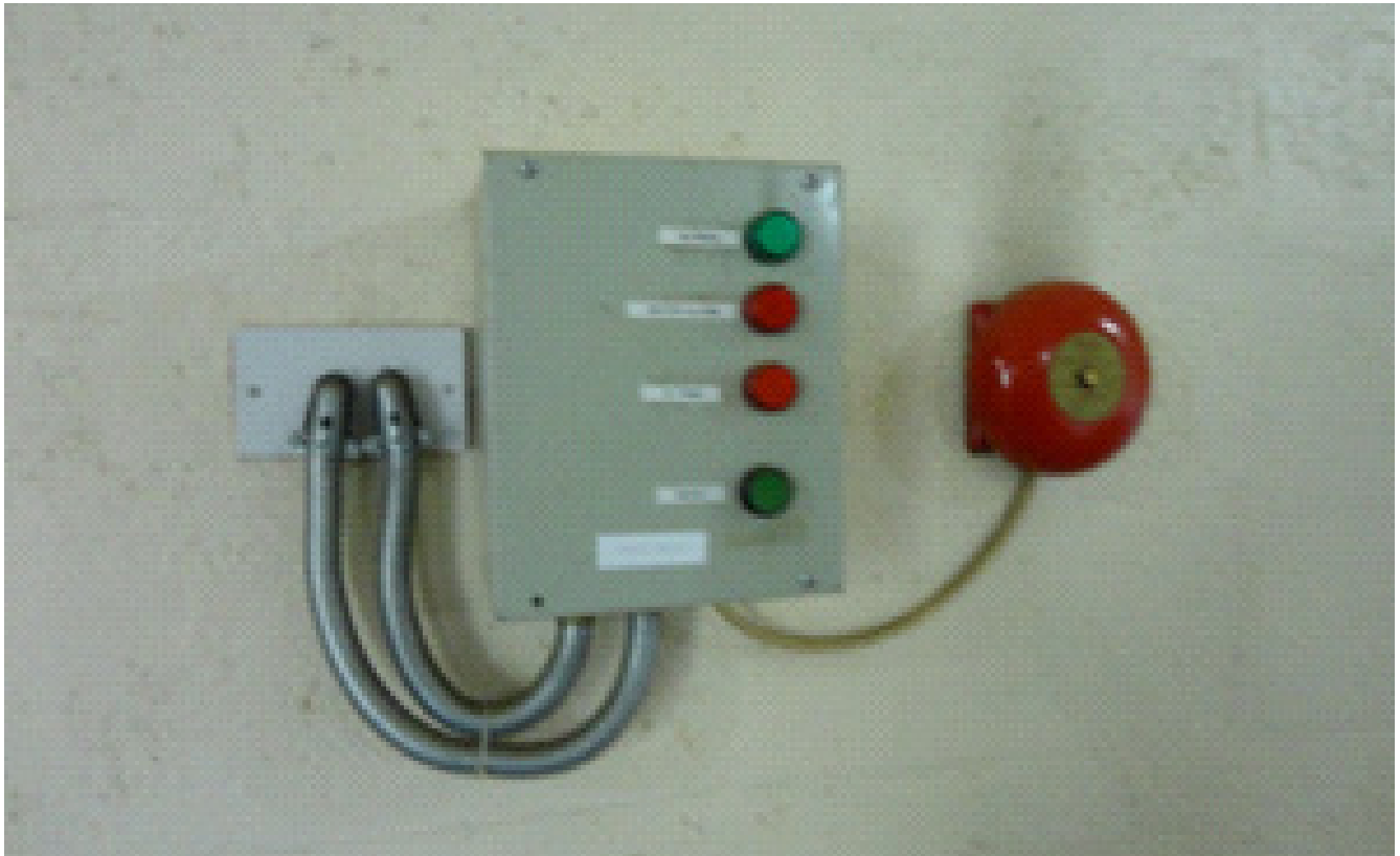
ES-11: Transformer Temperature Alarm and Bell
