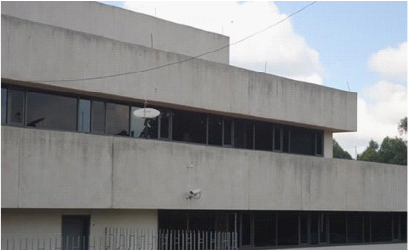
BE-9: External Elevation finishes which require upgrading
