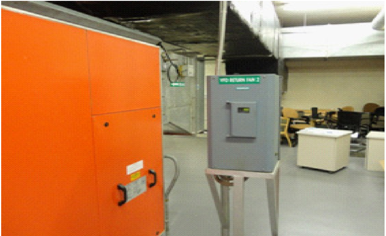
MS-1: AHU #2; VFD
