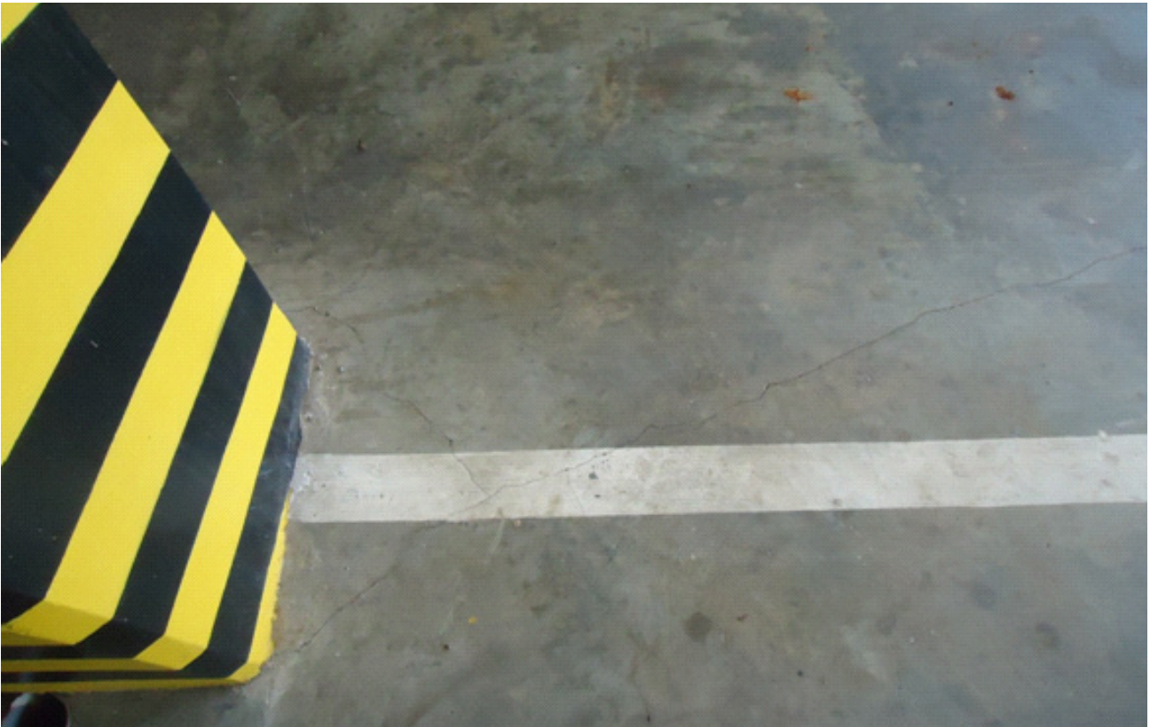
S-9: Radial Cracks on Floor Slab in Basement Columns
