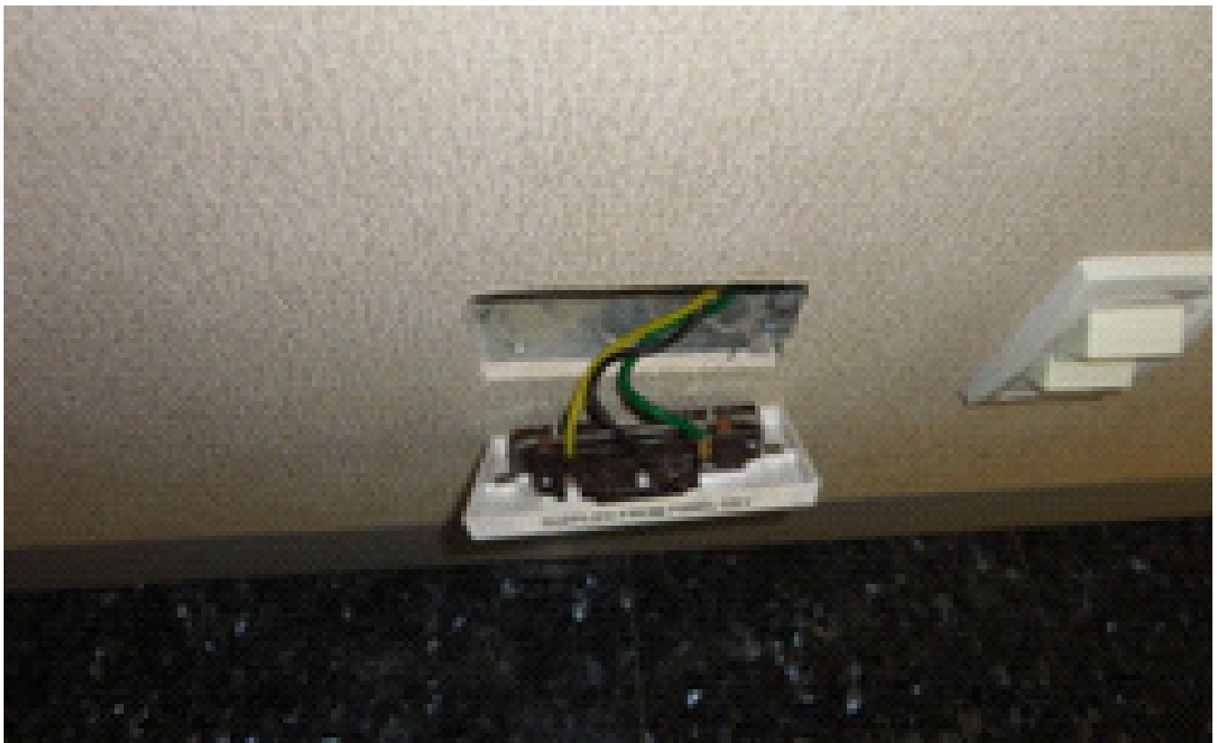
ES-4: Distribution Wiring to Socket (Receptacle), Yellow Phase
