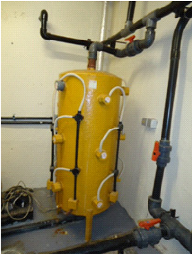
MS-16: Pool Water Heater
