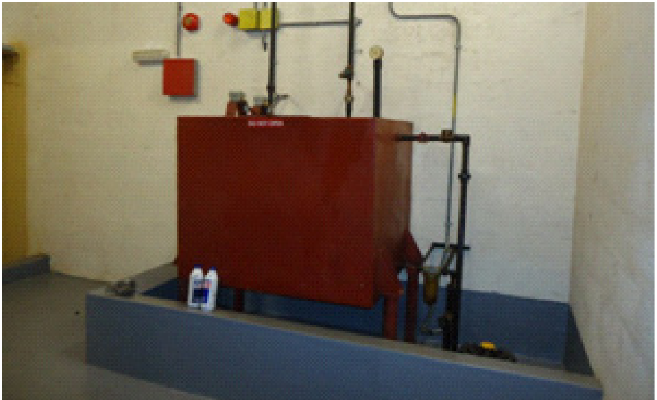
ES-20: Stand-by Generator Daytank
