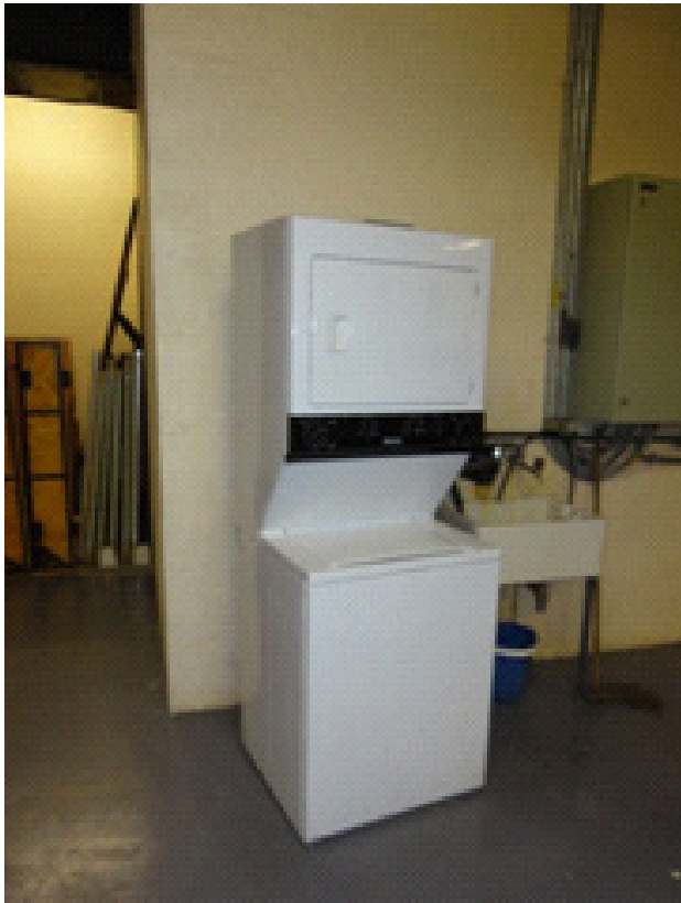
MS-3: Washing Machine in AHU Room
