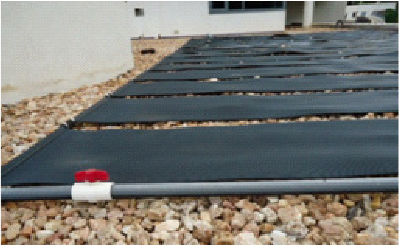
MS-17: Solar Hot Water Panels
