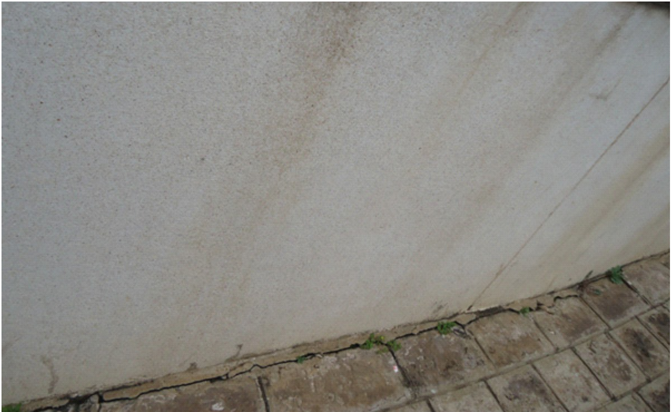
S-21: Separation of ramp wall from floor
