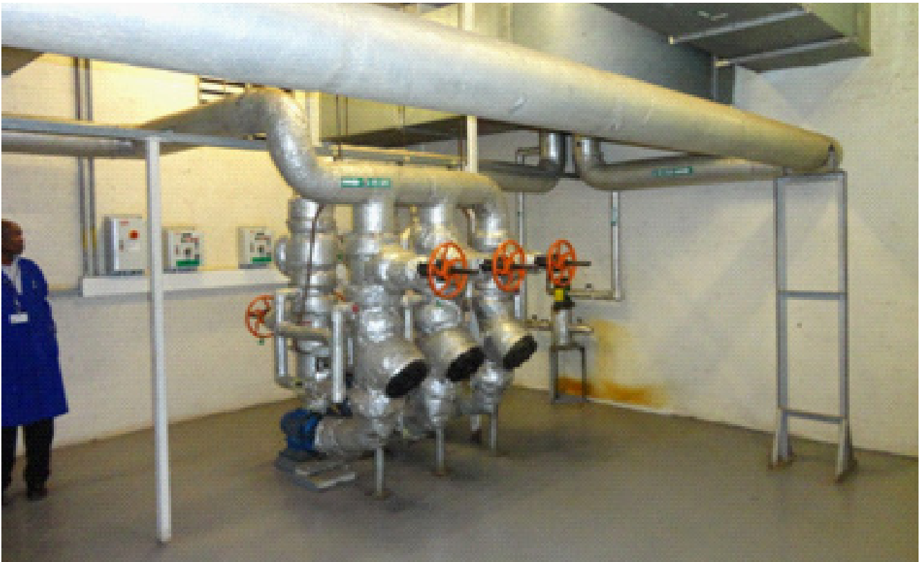
MS-22: Chilled water Manifold
