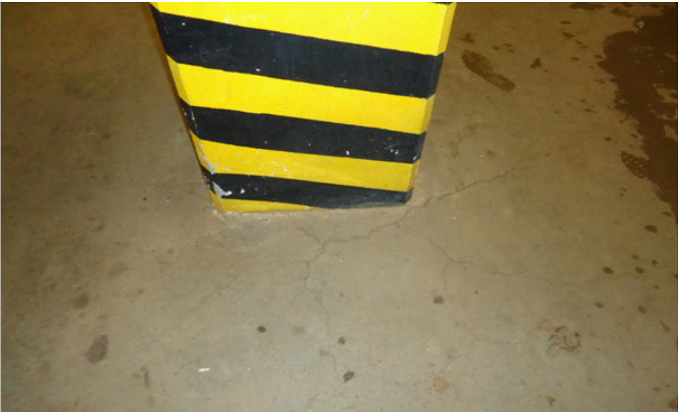
S-10: Radial Cracks on Floor Slab in Basement Columns
