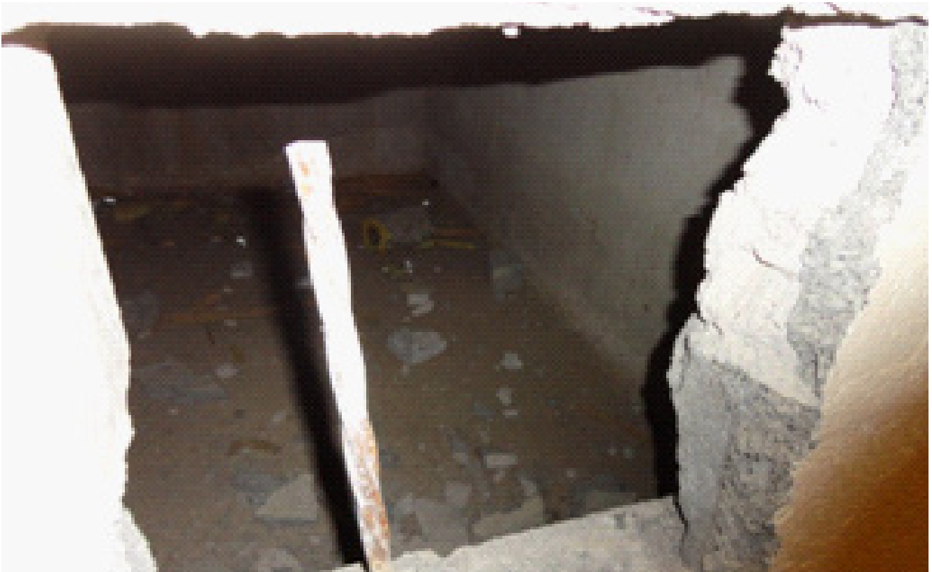
MS-9: Debris in Return Air Shaft (hole from electrical cupboard with broken fan)
