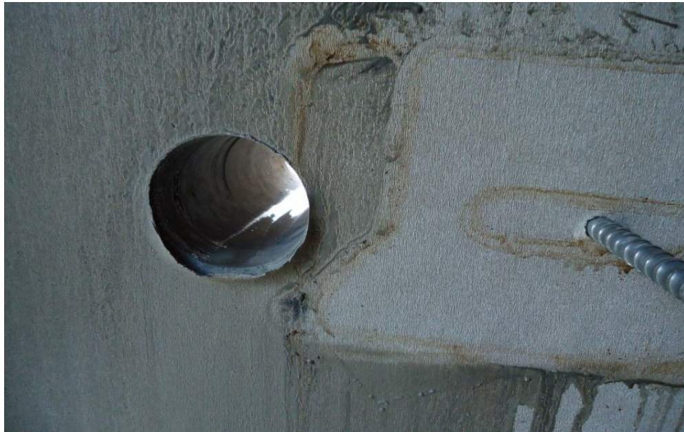
Photograph 2:- Exposed area after concrete core cutting at the staircase landing on the 2 nd Floor.
