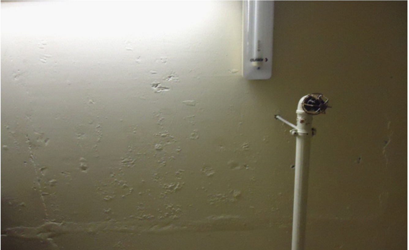
S-3: Spalling on slab soffit below swimming pool
