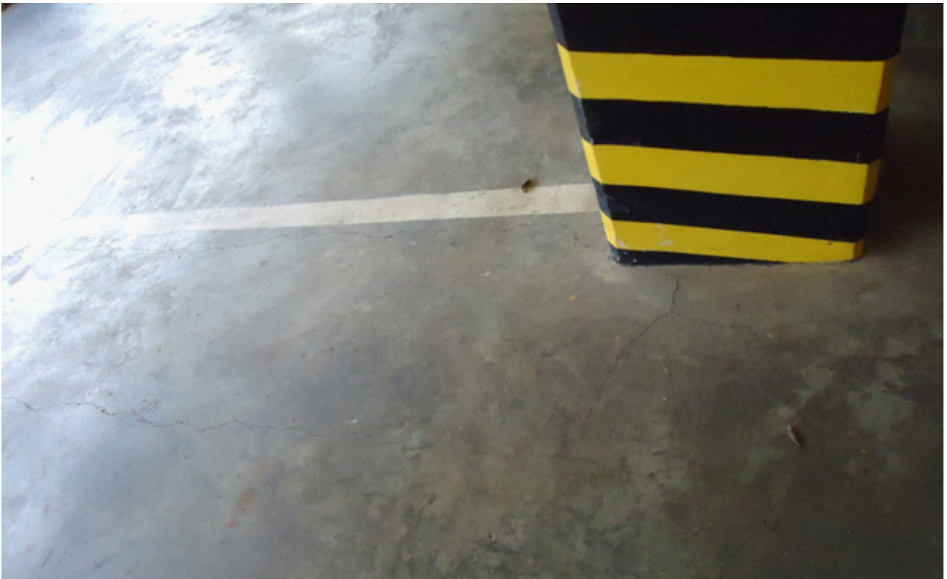
S-8: Radial Cracks on Floor Slab in Basement Columns
