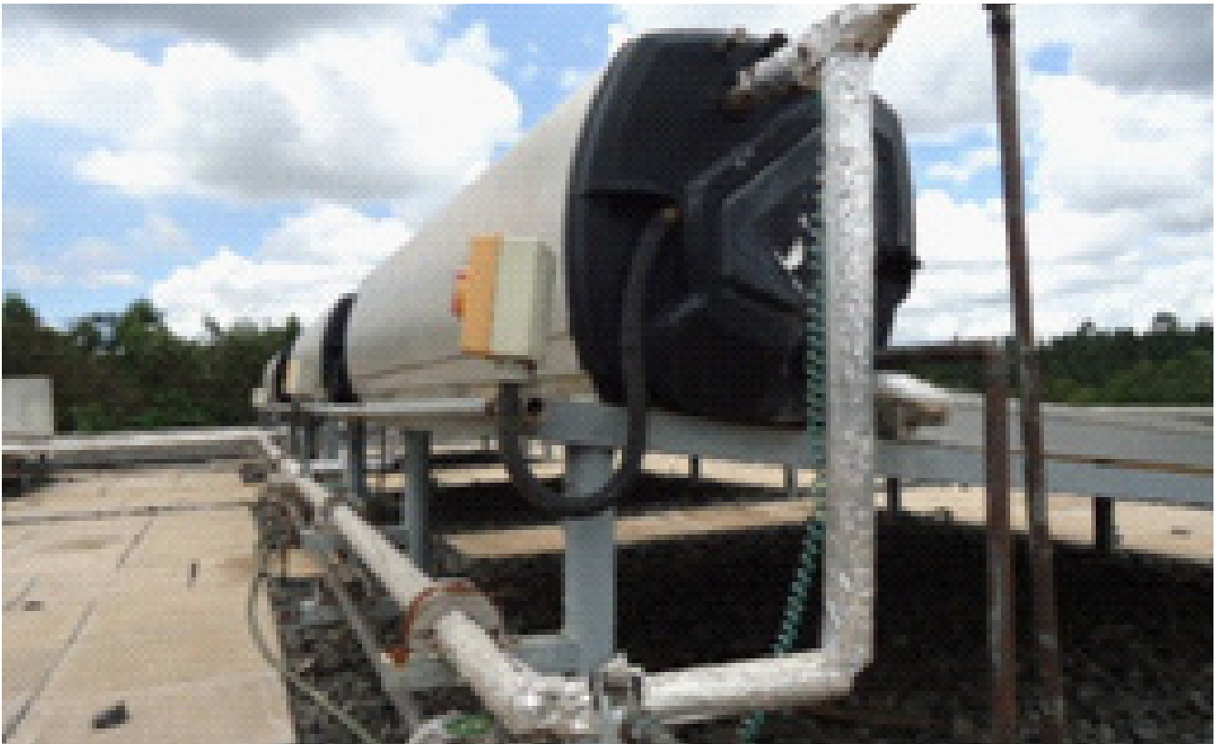
MS-18: Solar Hot Water Header
