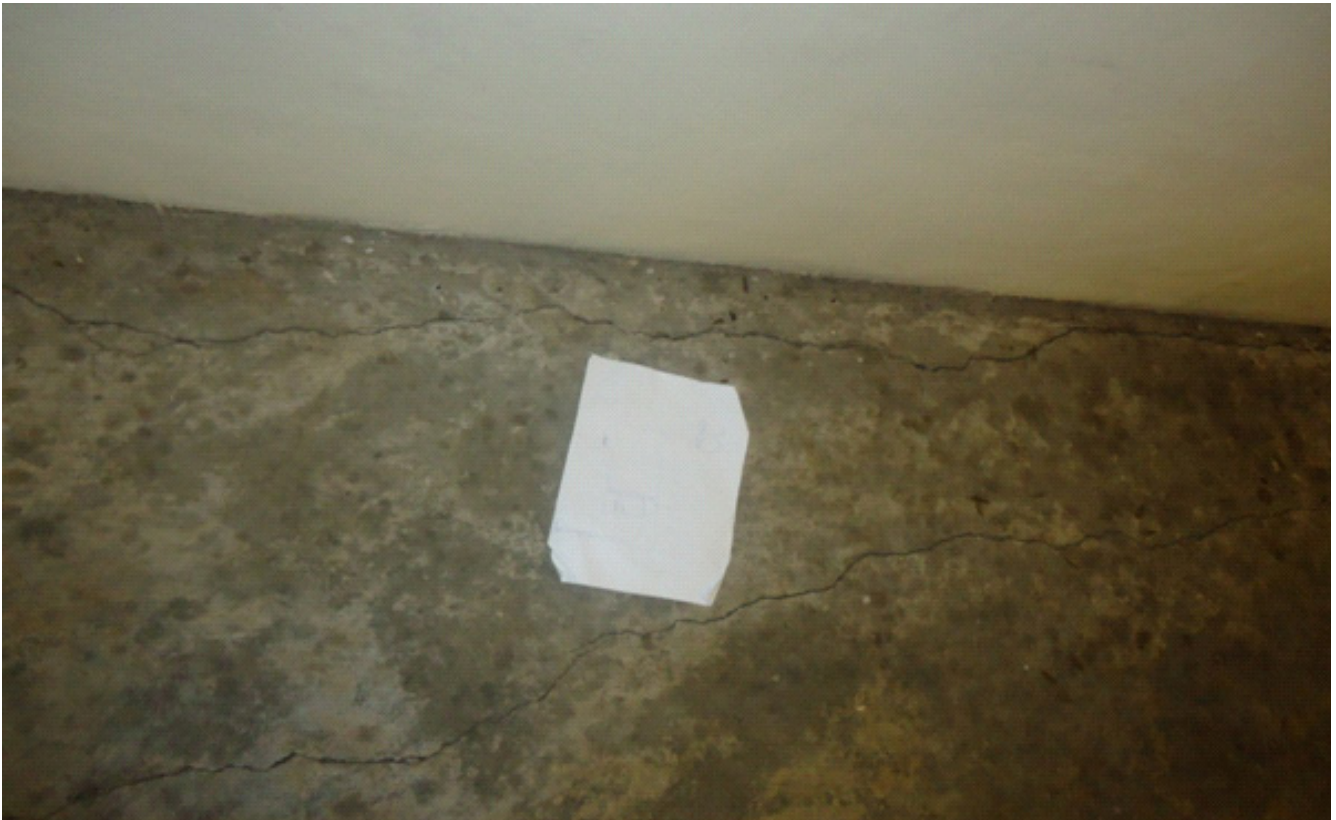
S-1: Cracks on Basement floor slab
