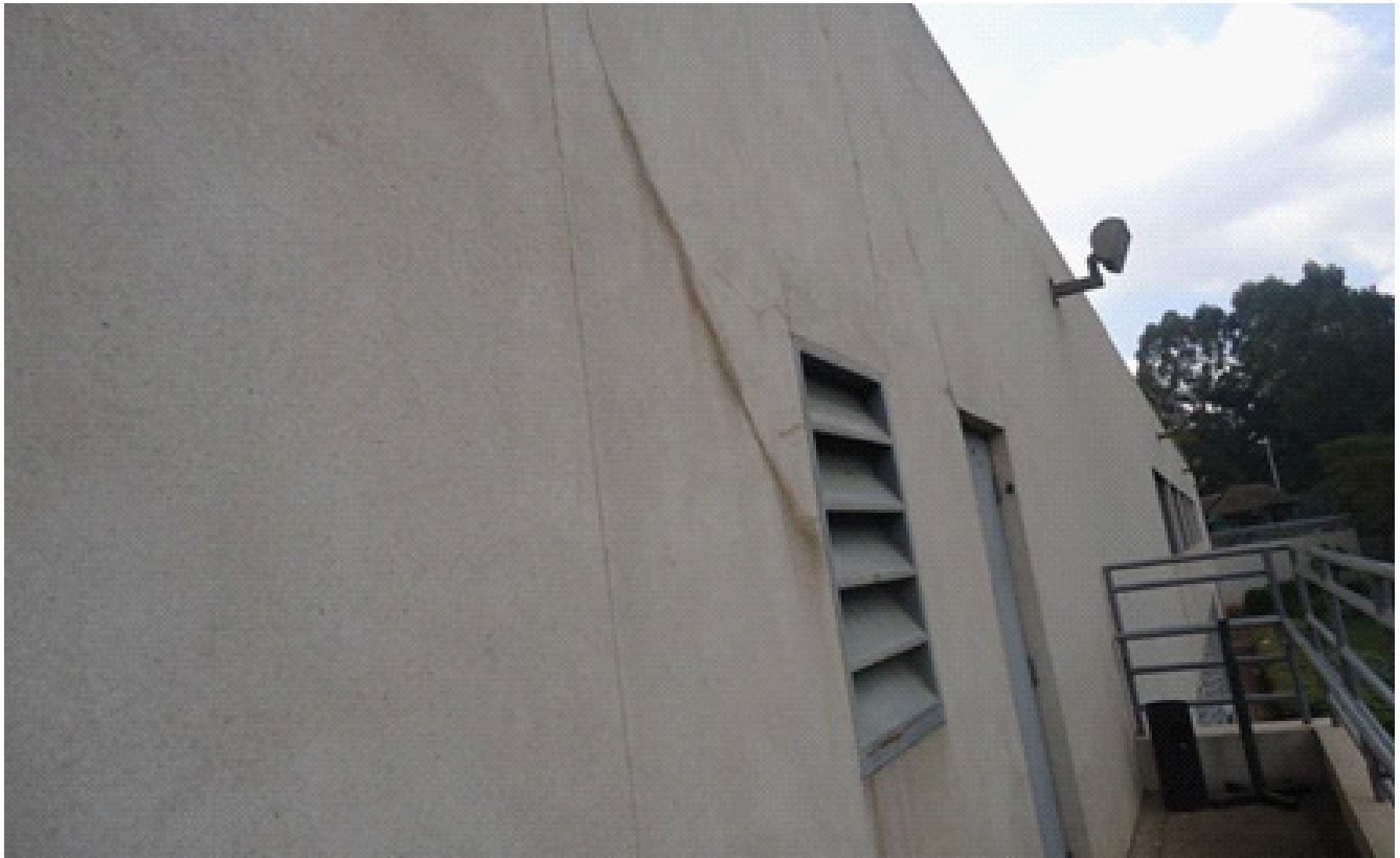
BE-11: Diagonal cracks on the wall which require rectification
