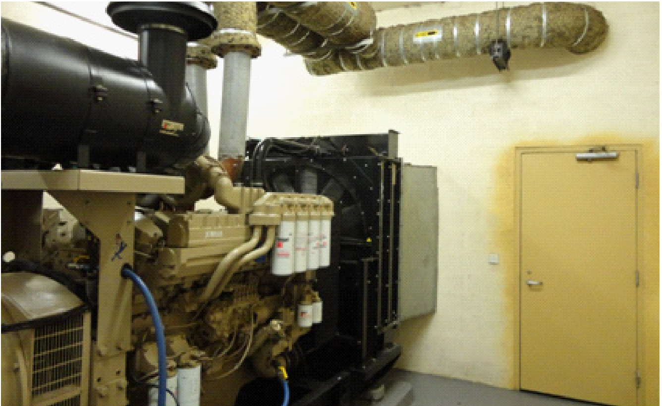
ES-5: Stand-by Generator
