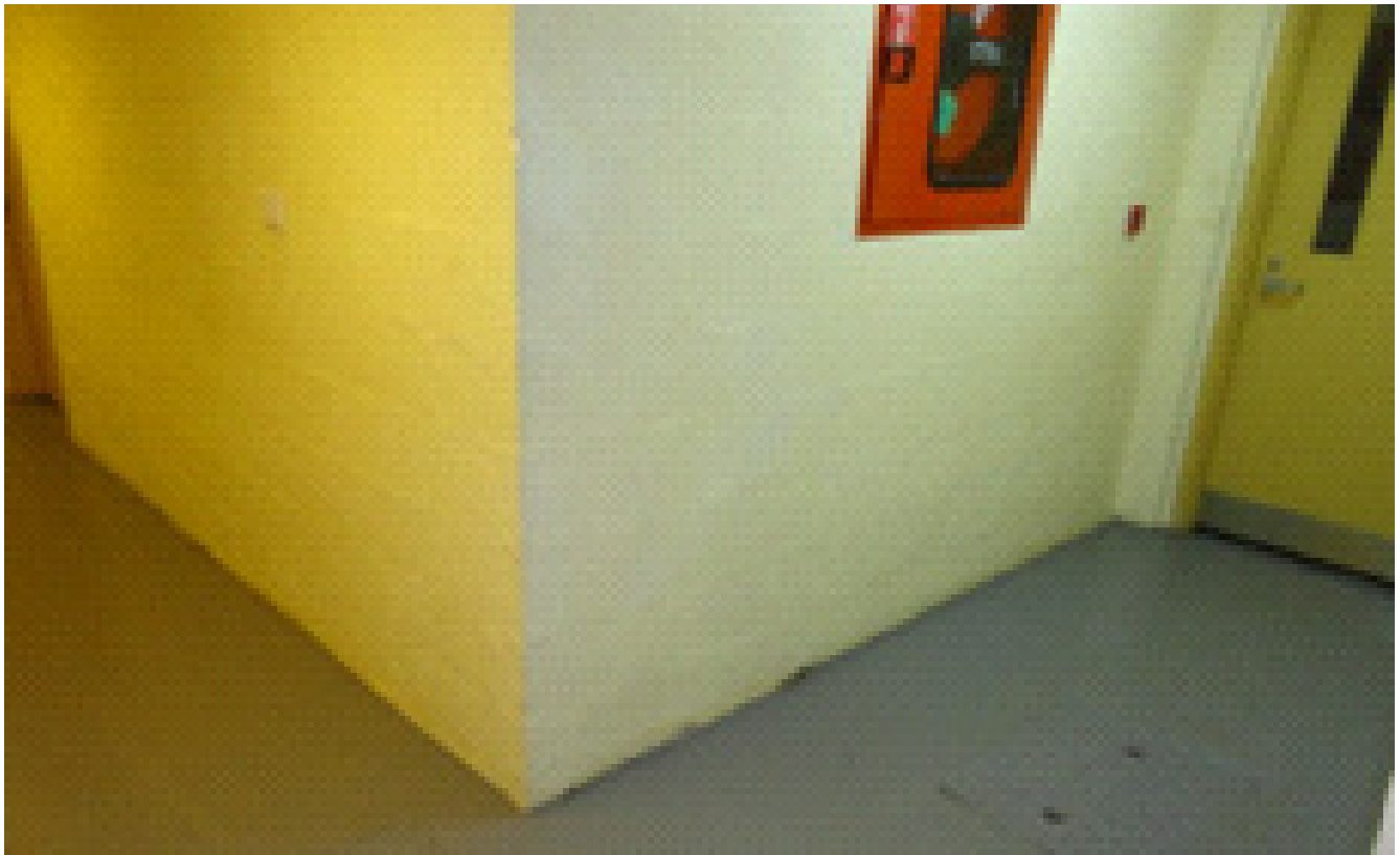
ES-16: Hose reel and Fire Alarm Callpoint
