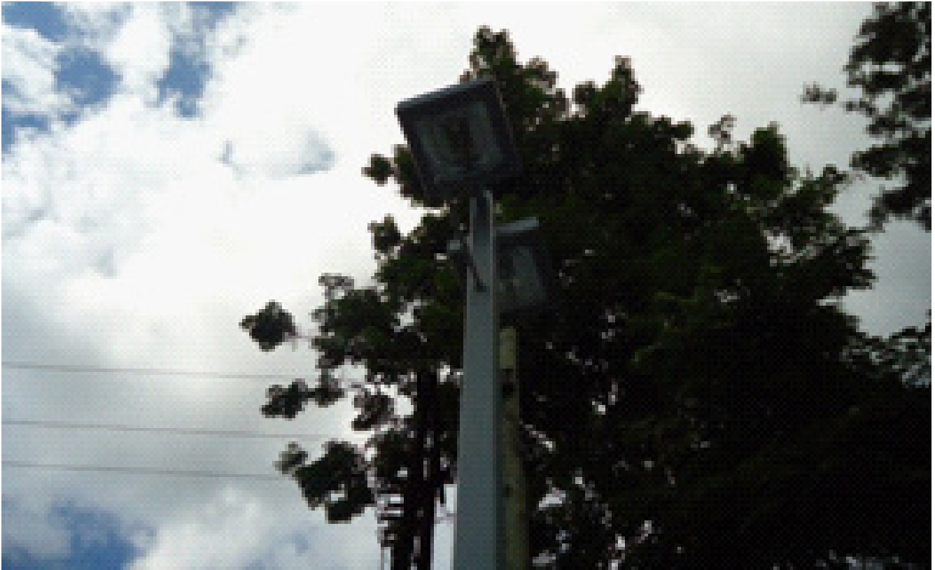
ES-18: External Lighting Pole
