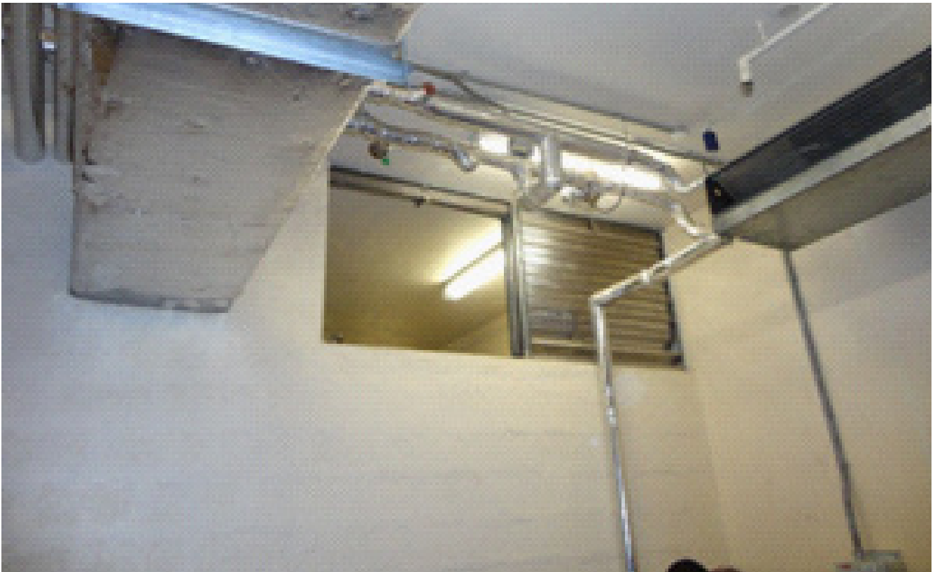
MS-8: Return Air Route with Fire Damper over Elevator Machine Room (view from Elevator Machine Room)
