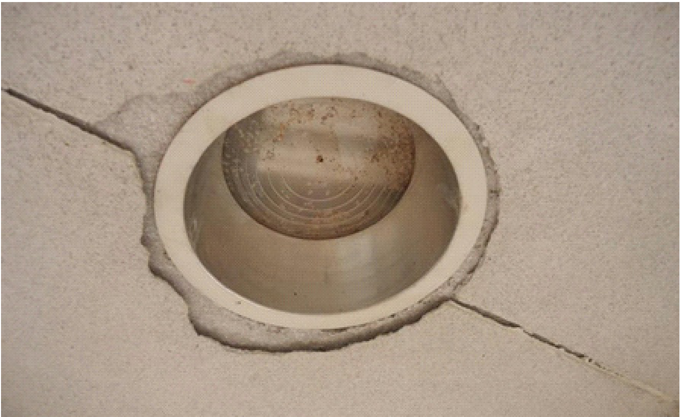
BE-14: Soffits with cracked
