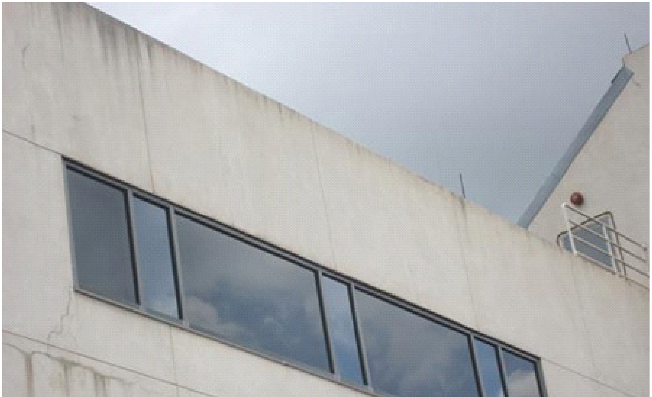
BE-12: Cracks on the edges of the windows with structural concerns
