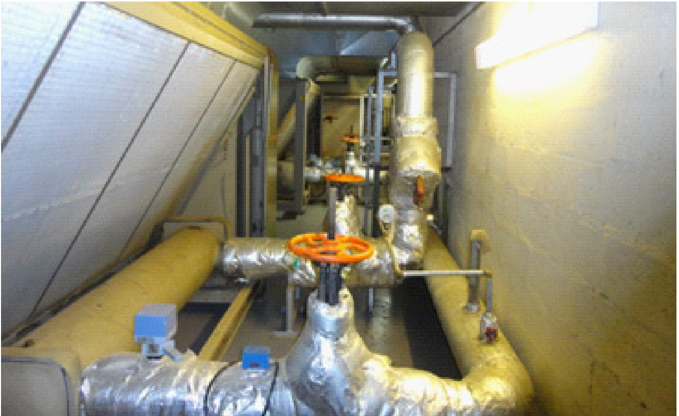
MS-21: Chiller (at left) in plantroom
