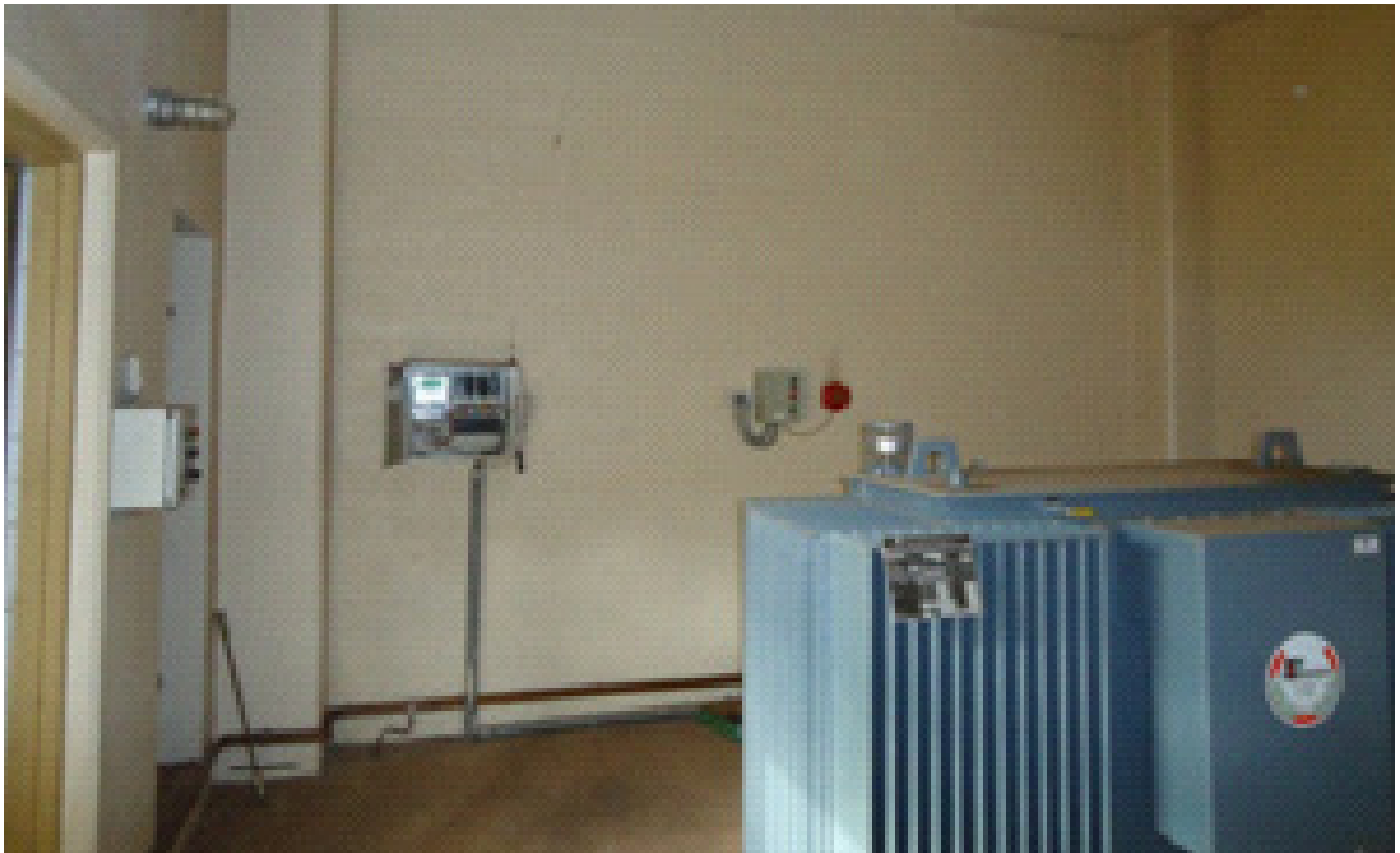
ES-12: Electrical Intake room (showing Wellglass-type light)
