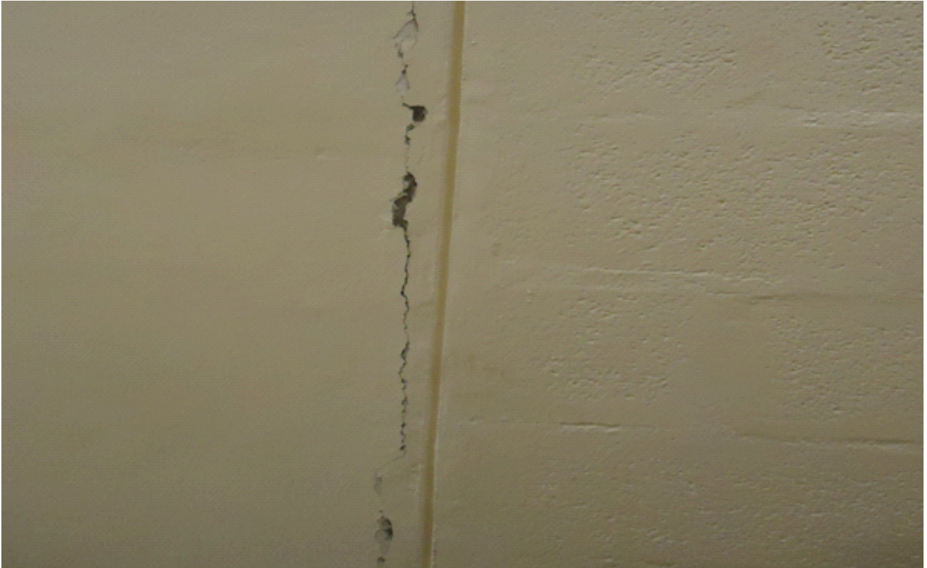
S-15: Crack on junction between masonry wall and concrete
