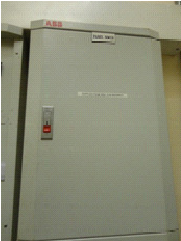
ES-13: Typical Distribution Panel
