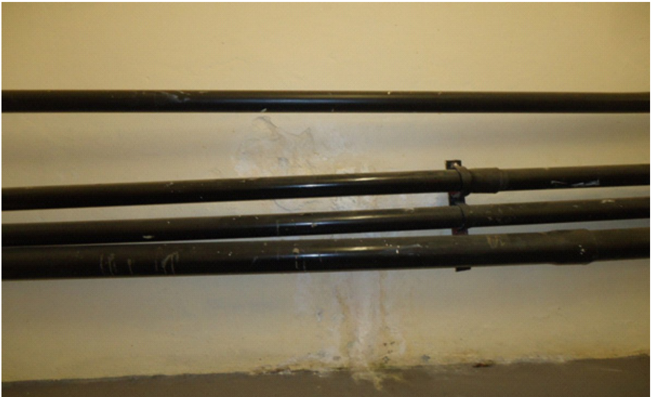
S-14: Efflorescence in pump room below swimming pool
