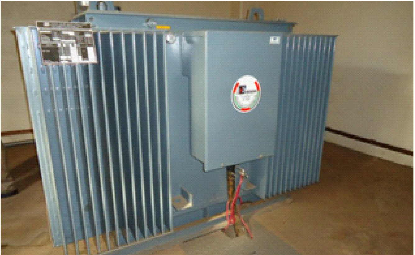
ES-9: Main Transformer
