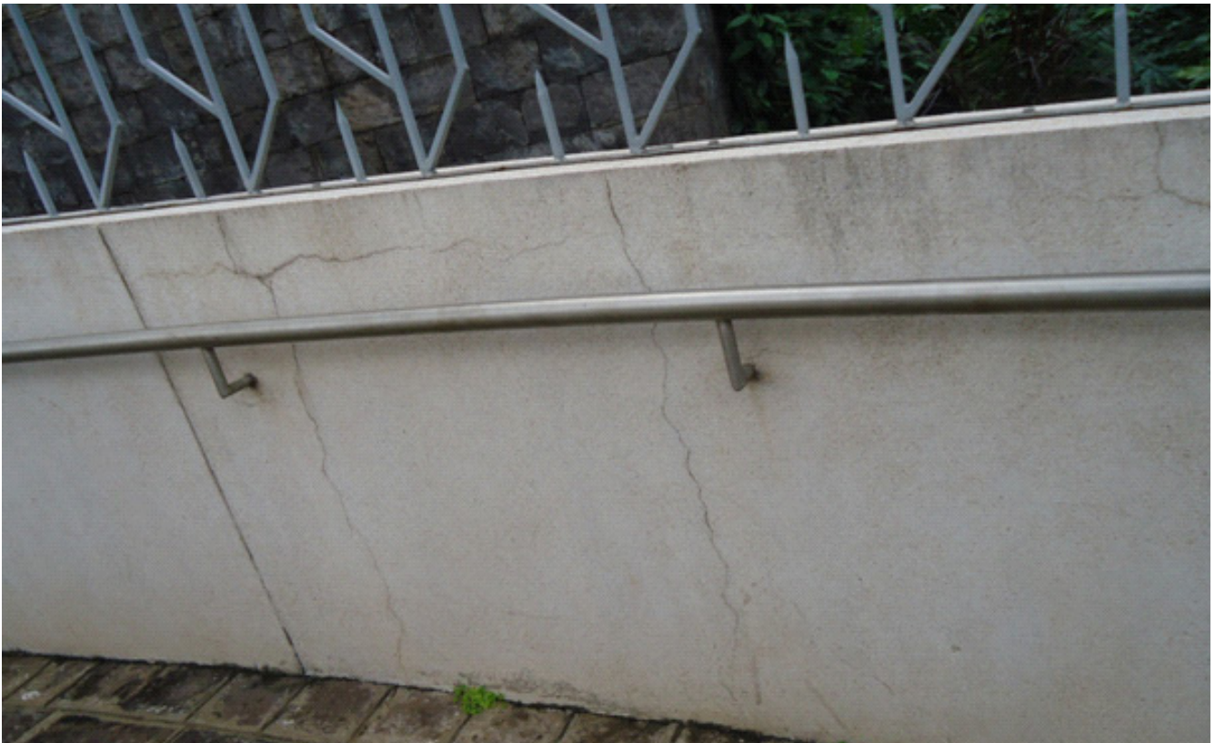
S-20: Cracks on ramp wall
