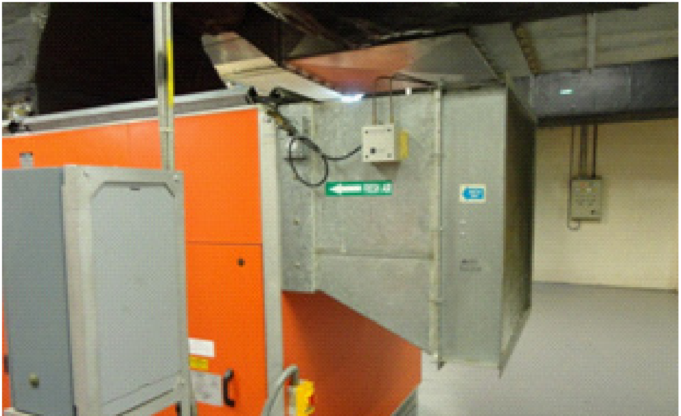
MS-2: AHU #2; Return Air intake
