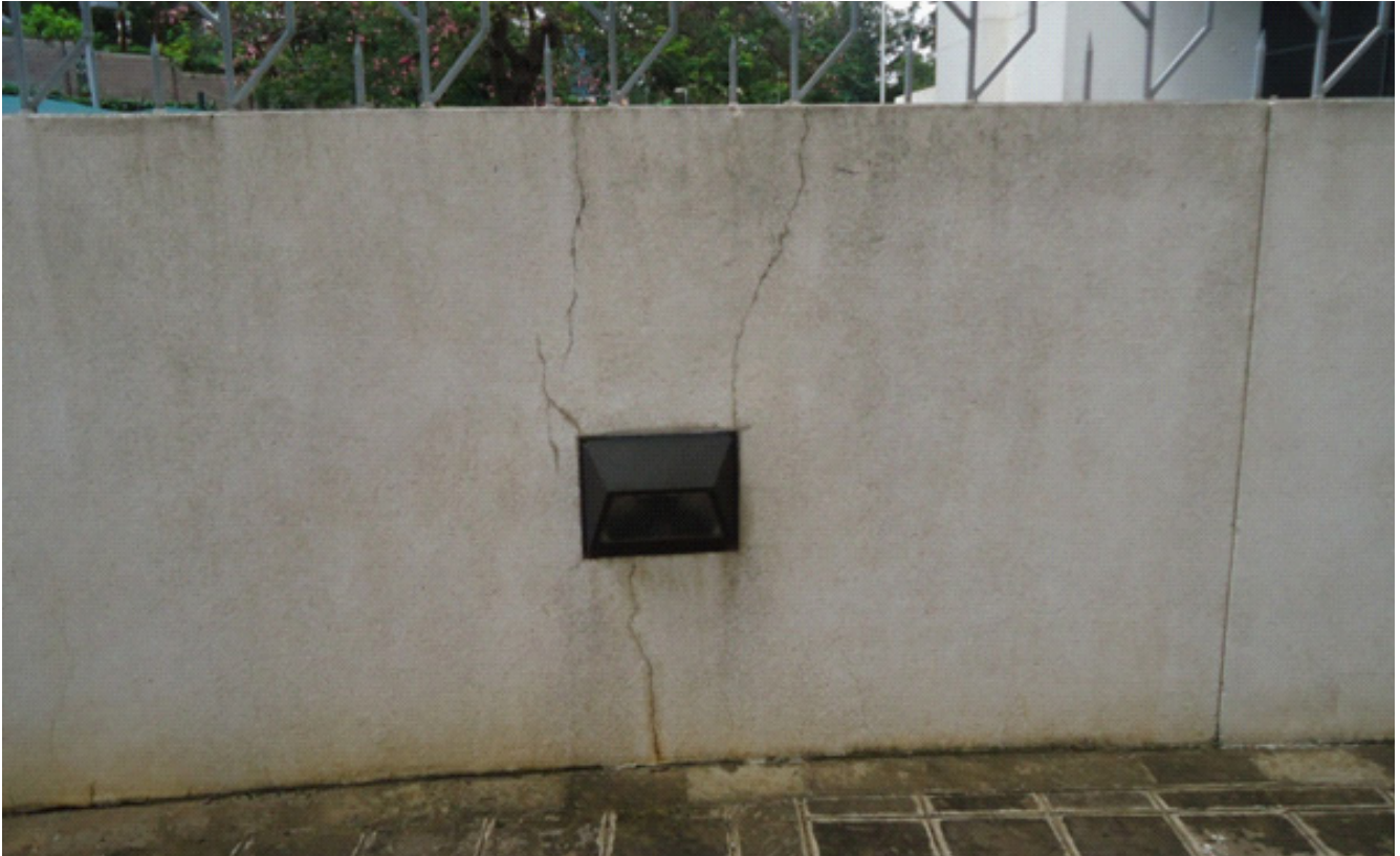
S-19: Cracks on ramp wall
