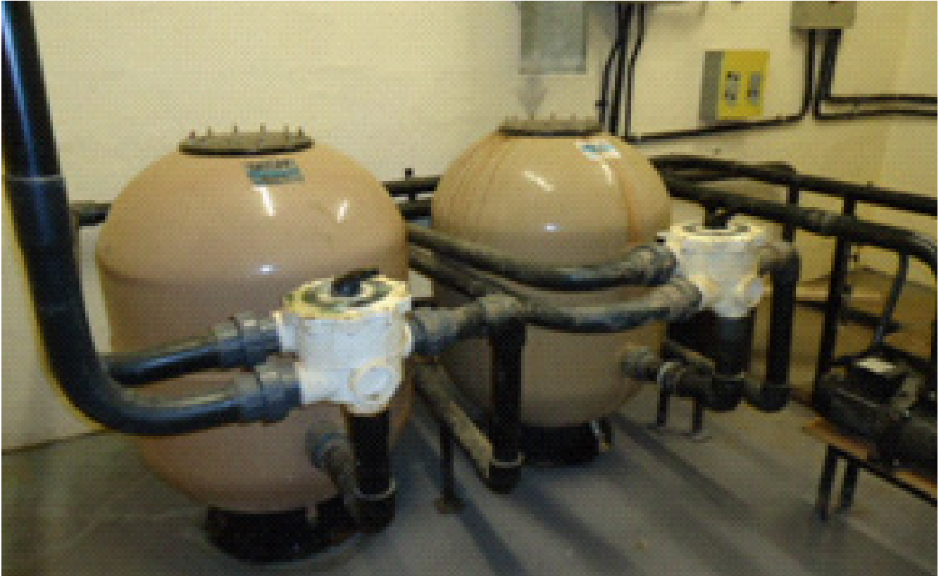
MS-15: Swimming Pool Plant
