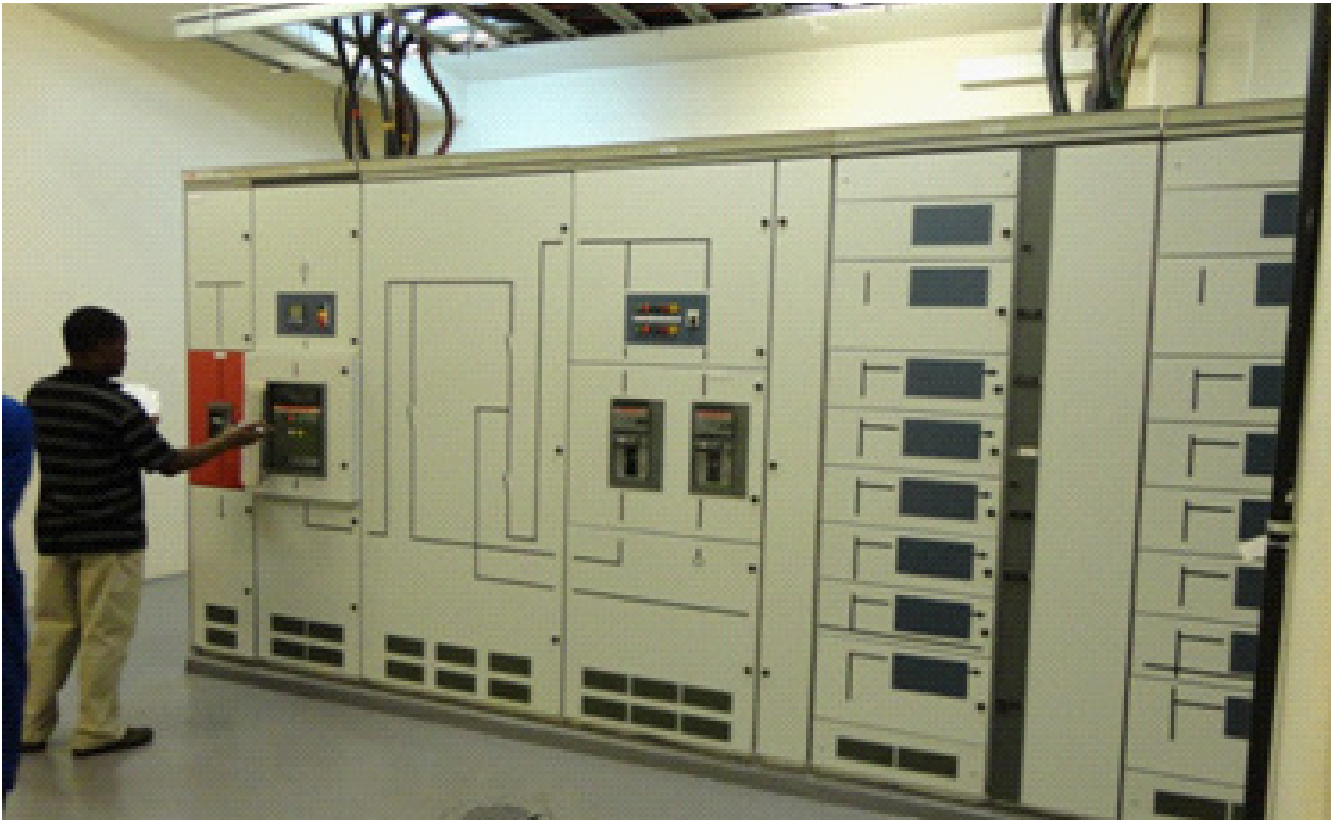
ES-1: Main Switchpanel
