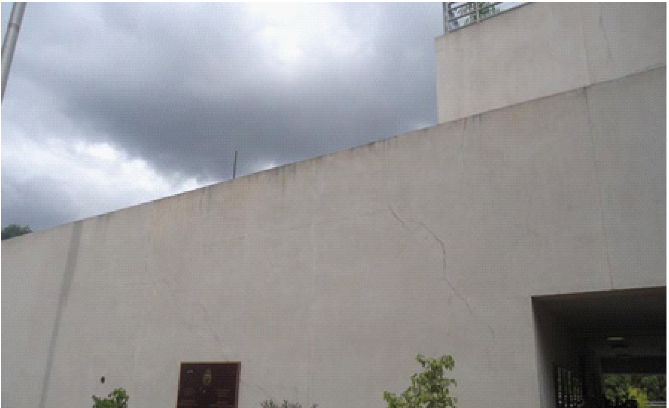
BE-10: Cracks on top of the wall finish
