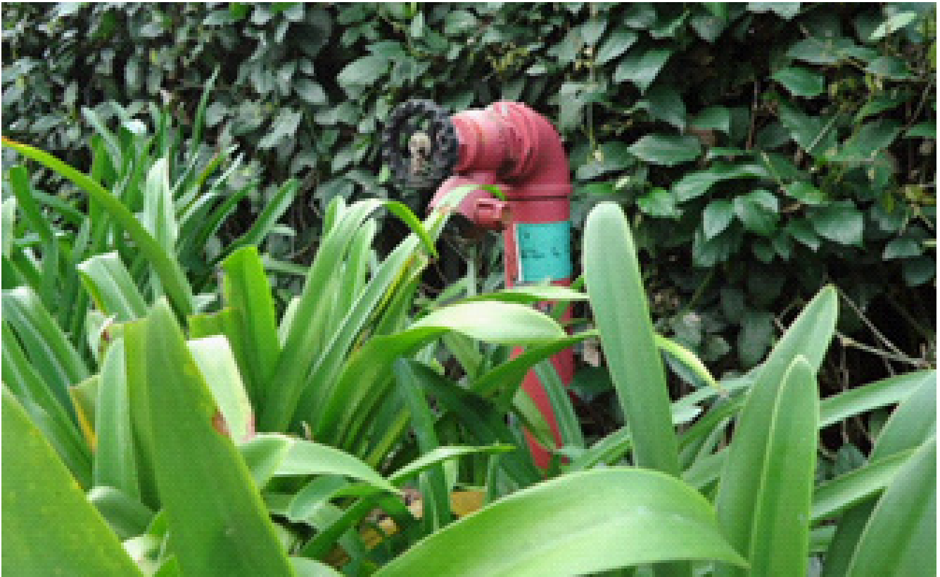
MS-19: Fire Hydrant
