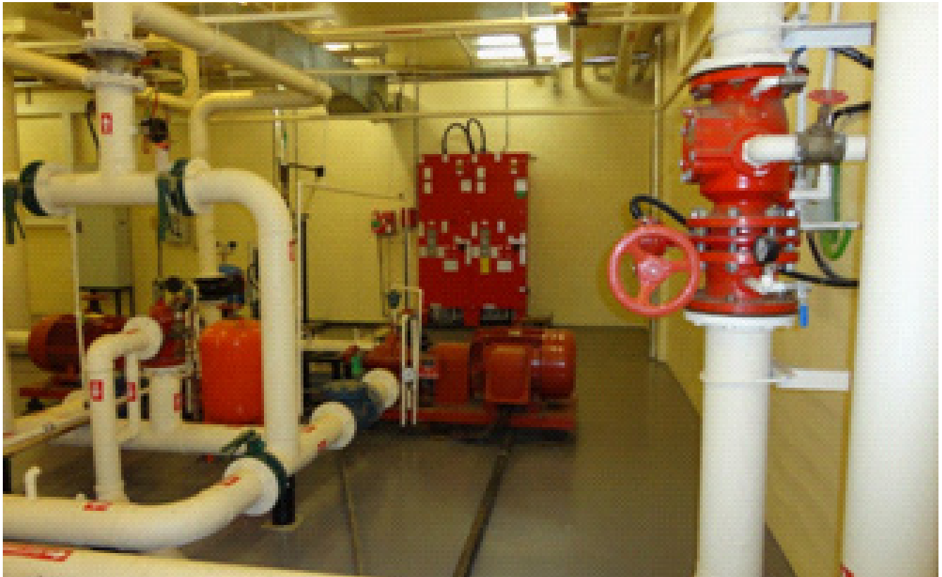
MS-13: Fire Pump Room
