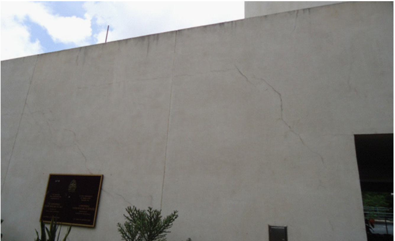
S-26: Crack on Exterior walls
