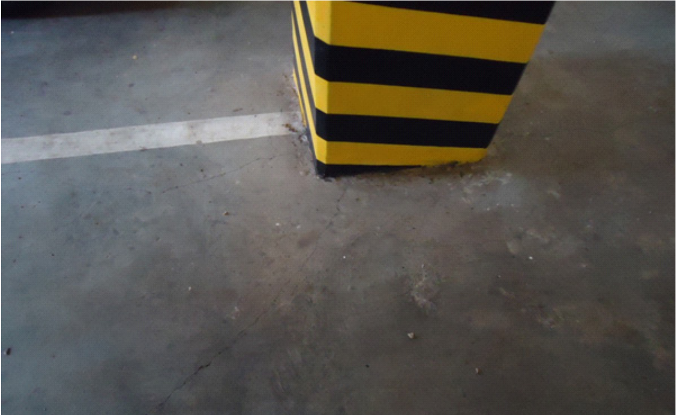
S-7: Radial Cracks of Floor Slab in Basement Columns
