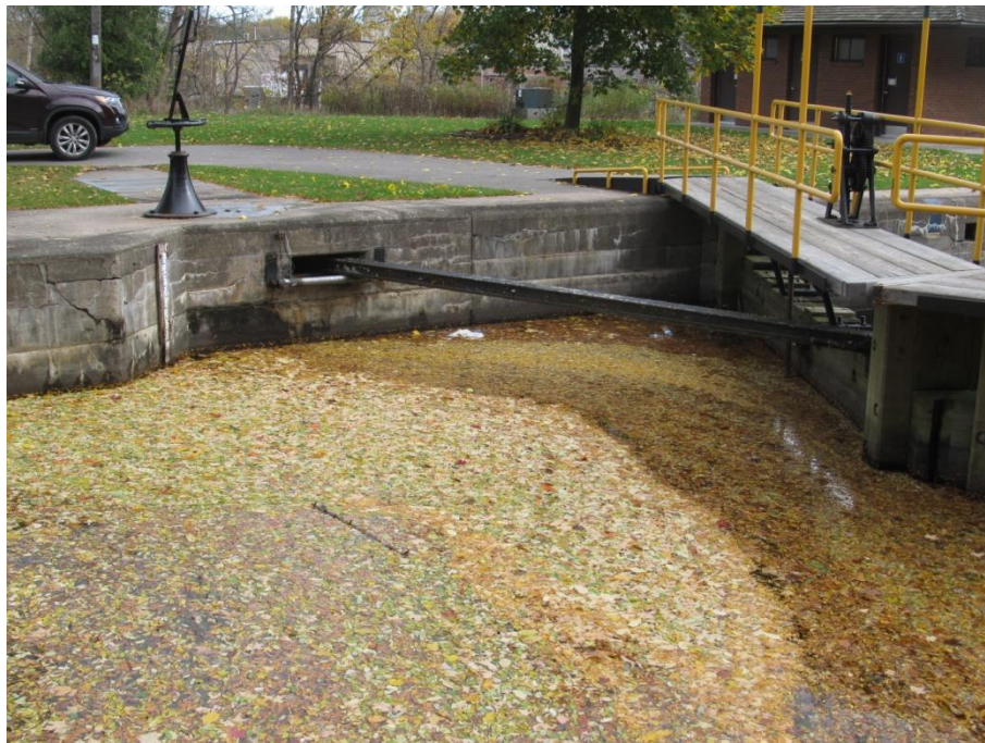
(P8) Lock 26 - NE Lock Gate Control Mechanism and Roller Bar
