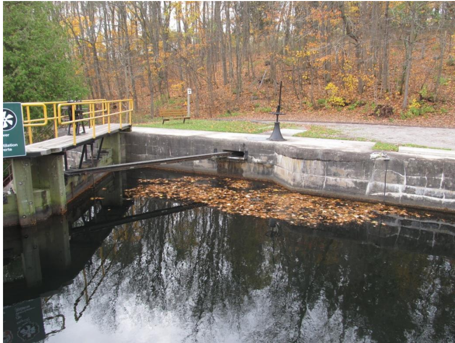
(P9) Lock 26 - SW Lock Gate Control Mechanism and Roller Bar
