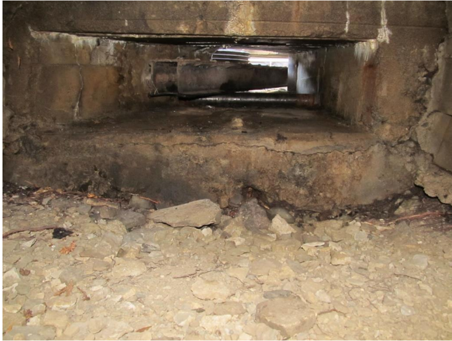
(P5) Lock 23 (SW Gate Control Mechanism)- Photo from within gate arm chase Photo taken from west side of control mechanism looking towards lock (to east).
