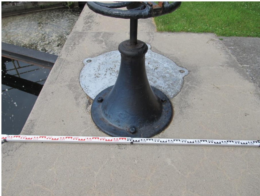
(P2) Lock 23 (SW Gate Control Mechanism)
