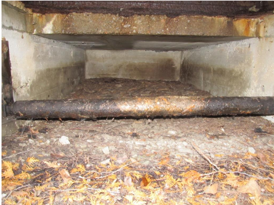
(P6) Lock 23 (SW Gate Control Mechanism)- Photo from within gate arm chase Photo taken from west side of control mechanism looking west .
