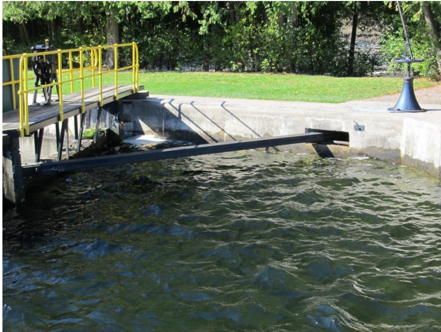
(P1) Lock 23 (SW Gate Control Mechanism)
