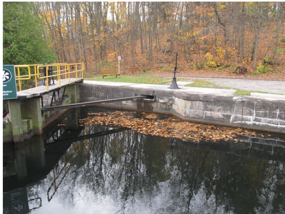
(P10) Lock 26 - NW Lock Gate Control Mechanism and Roller Bar
