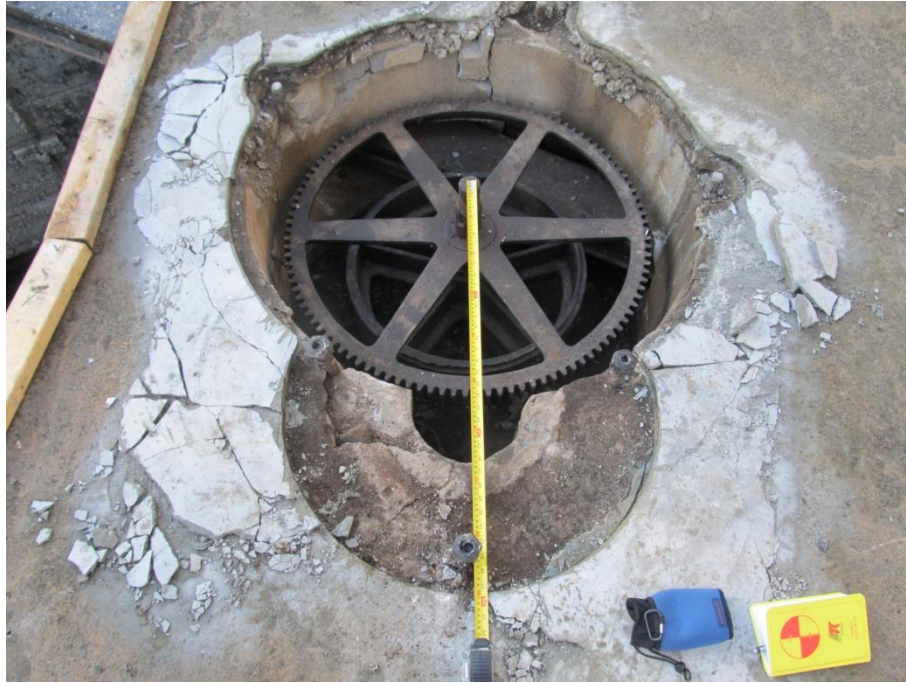
(P3) Lock 23 (SW Gate Control Mechanism)- Crank Cover Removed
