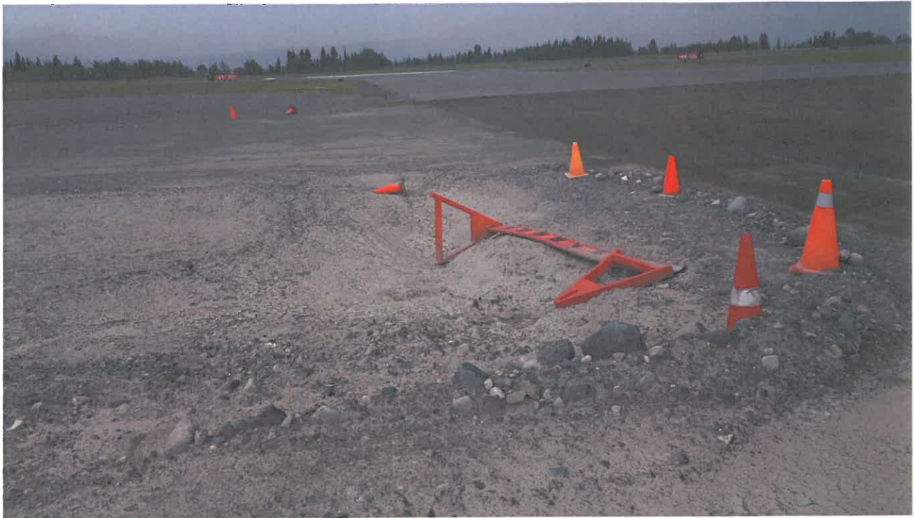
Photo 3: View of one of the subsidence areas within the footprint of the 2015 remedial excavation, which requires reparation during Phase I of the work program.
