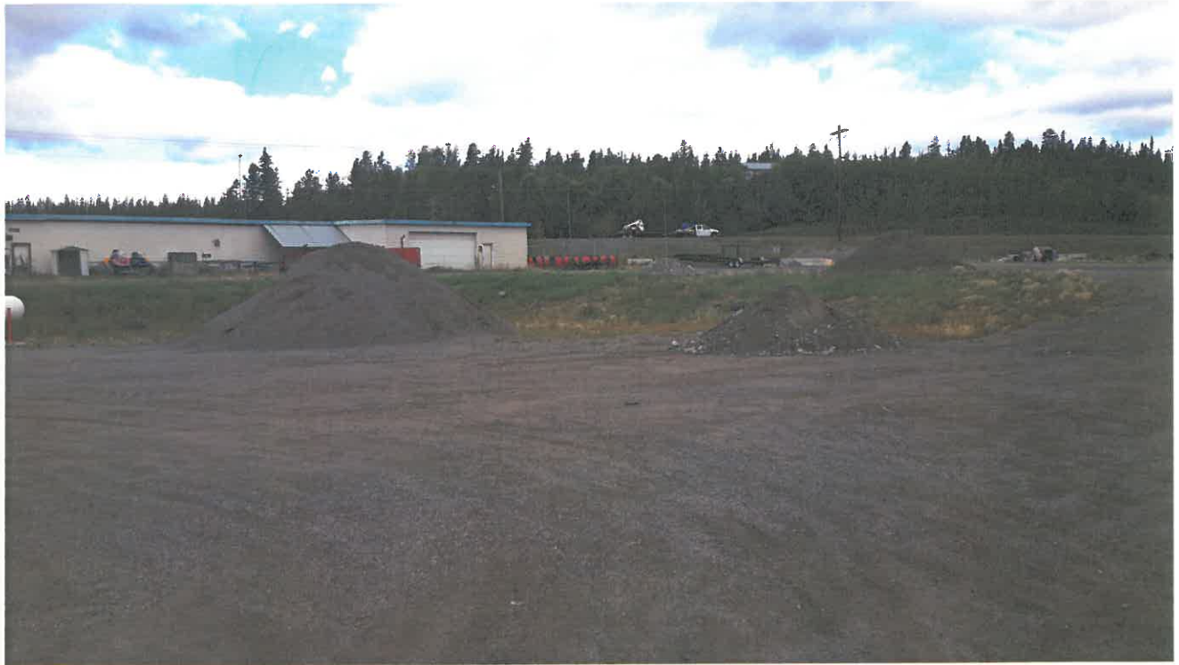
Photo 1: General view of the planned 2016 remedial excavation footprint located on the north apron of the Whitehorse International Airport.
