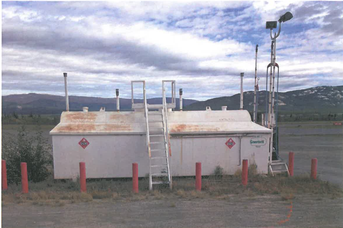
Photo 7: View of the fuel aboveground storage tank (AST) adjacent and southeast of the planned 2016 excavation footprint.
