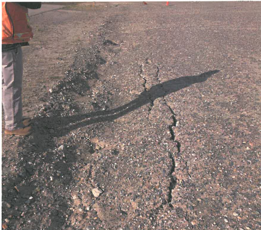
Photo 6: View of another of the subsidence areas within the 2015 remedial excavation footprint, which requires reparation during Phase I of the work program.
