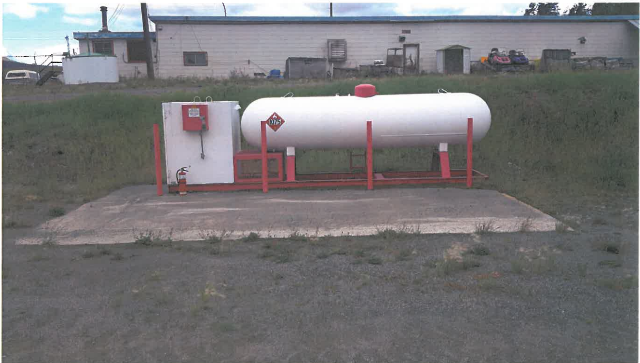
Photo 8: View of the propane tank in the centre section of the planned 2016 remedial excavation footprint. Concrete pad has dimension of 2.4 x 1.8m (8 x 6 feet).
