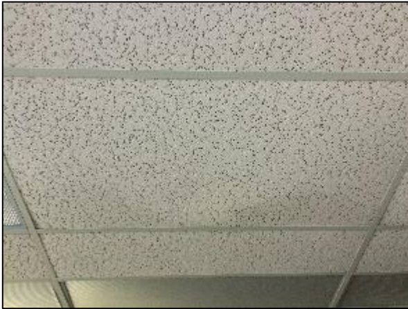
Photo 17 – 24"x48", lay in, pinhole with small random fissure
