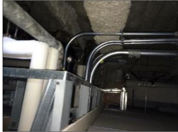
Photo 4 – Newer grey sprayed fireproofing in the print area – East Wing Phase 3A. Remnant asbestos-containing fireproofing was identified
