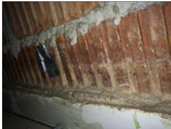
Photo 5 – Friable sprayed fireproofing debris on top of the perimeter plaster wall – West Wing Phase 2
