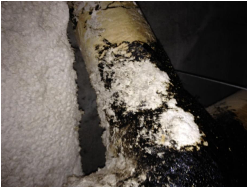
Photo 7: Black tar, observed on pipe straights, fittings and ducting, was identified as containing 3% Chrysotile asbestos.
