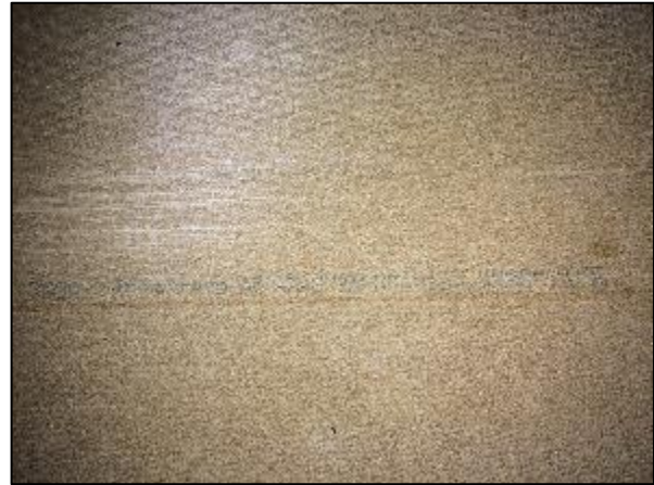
Photo 18 – 24"x48", lay-in, pinholes with small random fissures, date stamp 01/18/00
