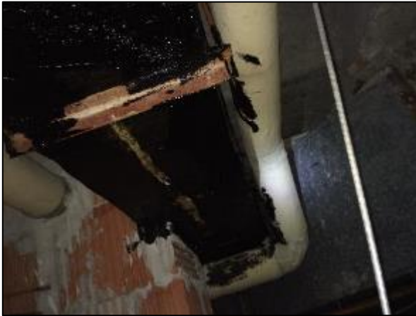
Photo 12 – Non-friable asbestos-containing black tar on square ducts
