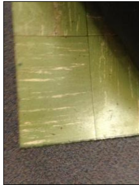
Photo 25 – Non-friable asbestos-containing 9"x9" vinyl floor tile, green with white streaks. Non-friable asbestos-containing mastic is present underneath tiles.
