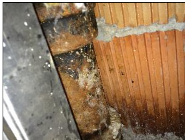
Photo 35 – Lead rope caulking may be present in bell and spigot fittings on cast iron pipes within the assessed areas.
