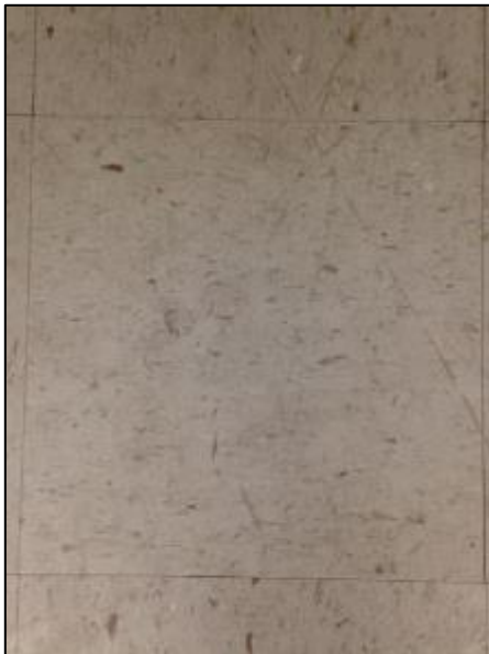
Photo 24 – Non-asbestos 12"x12" vinyl floor tile, rose with brown streaks. Non-friable asbestos-containing mastic is present underneath tiles.
