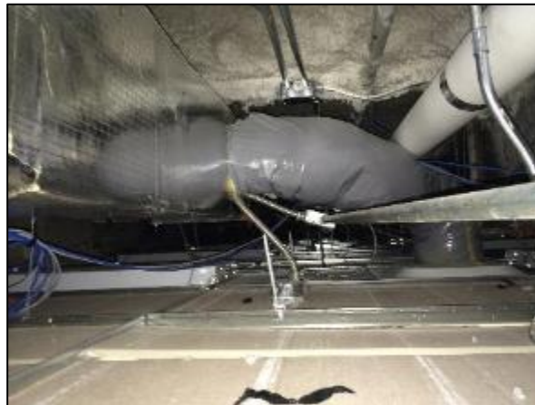
Photo 14 – Non asbestos fibreglass insulation on ducts.
