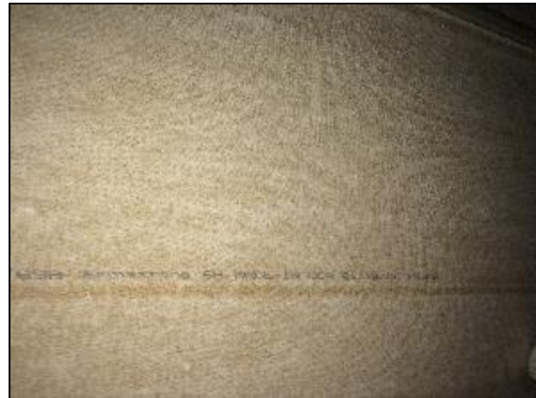
Photo 16 – 24"x48", lay-in, pinholes with small random fissures, date stamp 01/18/00
