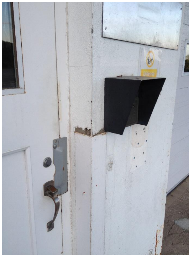
Photo 8: Approximately 20 square metres of a non-friable smooth cementitious finishing material (not stipple textured), containing 1% Chrysotile asbestos (DST sample 07A) was observed on the outer walls of the loading dock.
