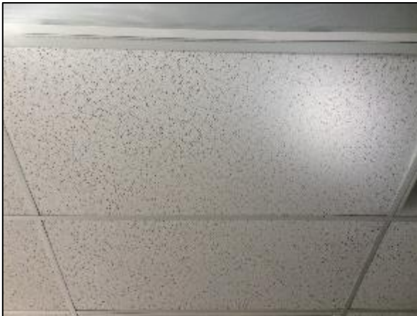
Photo 15 – 24"x48", lay in, pinhole with small random fissure
