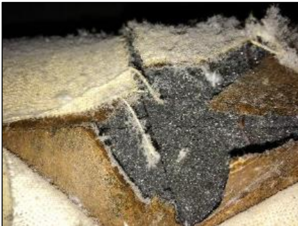
Photo 10 – Foamglass insulation on chilled water pipes in Phase 2.
