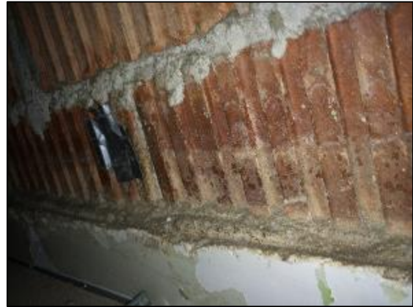
Photo 20 – Non-asbestos grey plaster with a white scratch coat – Phase 2. Sprayed fireproofing was identified on the top of plaster walls, ledges, etc. during the assessment.
