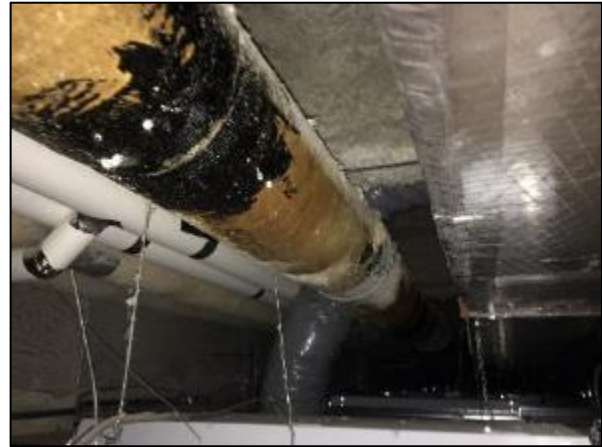
Photo 13 – Non-friable asbestos-containing black tar on circular ducts.
