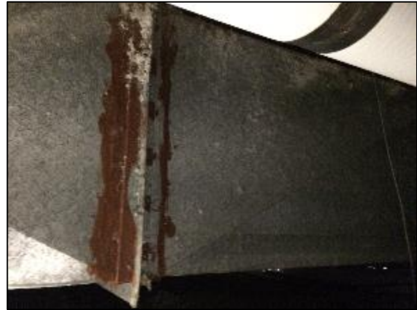
Photo 29 – Non-friable asbestos-containing burgundy sealant on ducts
