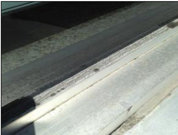
Photo 30 – Asbestos containing caulking is present on window sill flashings and as perimeter sealants around door and windows throughout the assessed area.
