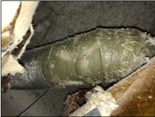
Photo 28 – Non-asbestos grey/green duct sealant
