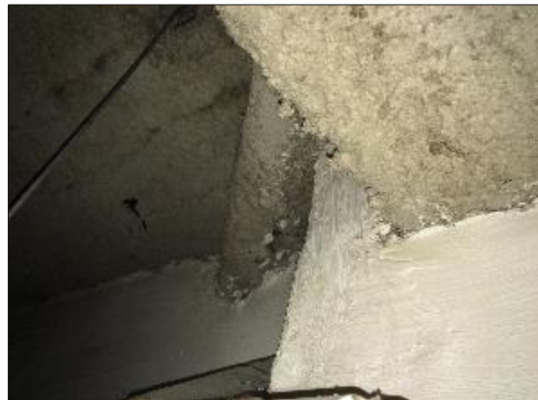
Photo 2 – Friable asbestos-containing sprayed fireproofing on structural beams with overspray on deck
