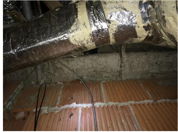
Photo 31 – Non-asbestos white duct sealant on foil over fibreglass insulated ducts in the pipe chases of Phase 3B.
