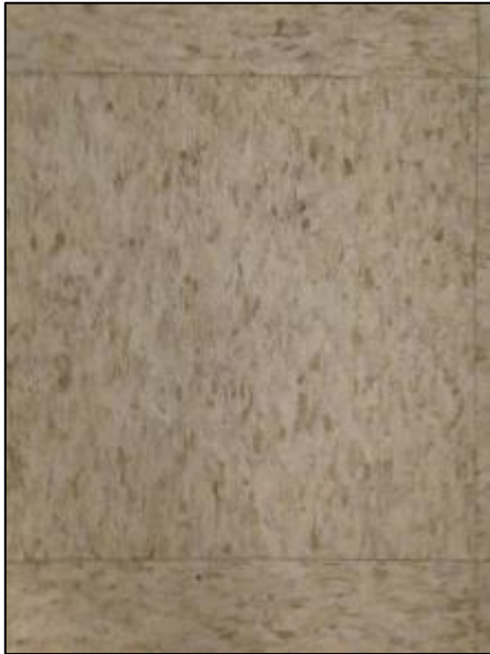
Photo 26 – Non-asbestos 12"x12" vinyl floor tile, beige with brown streaks. Non-friable asbestos-containing mastic is present underneath tiles
