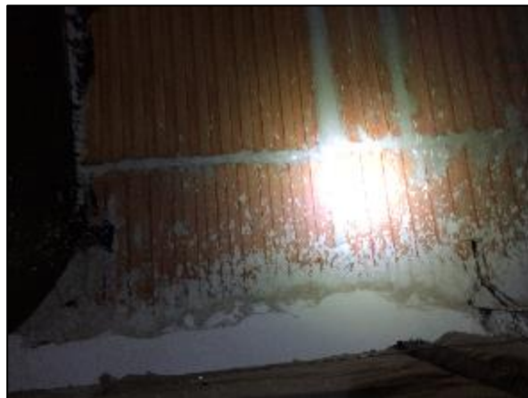
Photo 21 – Non asbestos grey plaster with a white scratch coat – Visually similar in Phases 3A and 3B. Sprayed fireproofing was identified on the top of plaster walls, ledges, etc. during the assessment.
