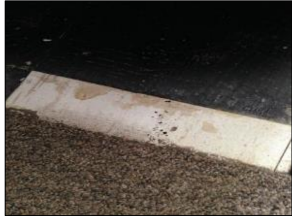
Photo 27 – Non friable asbestos-containing 9"x9" vinyl floor tile, white with brown streaks. Non-friable asbestos-containing mastic is present underneath tiles
