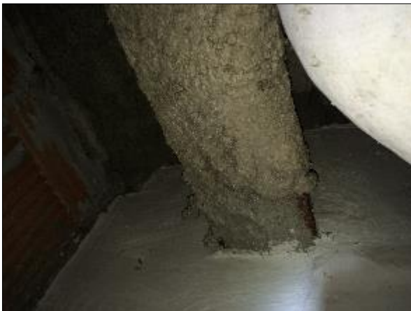
Photo 1 – Friable asbestos-containing sprayed fireproofing on structural beams
