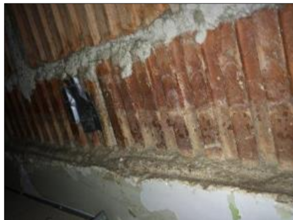
Photo 5 – Friable sprayed fireproofing debris on top of the perimeter plaster wall – West Wing Phase 2
