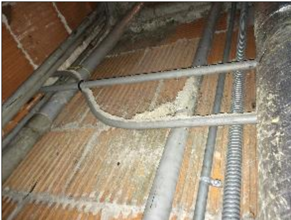
Photo 3 – Friable sprayed fireproofing in a riser – Phase 3B
