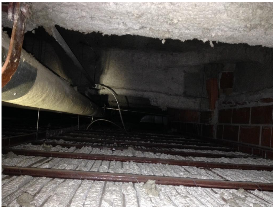
Photo 3: Spray-applied fireproofing was observed on the ceiling deck and structural beams throughout the ground floor south wing. Overspray and debris were also observed throughout.
