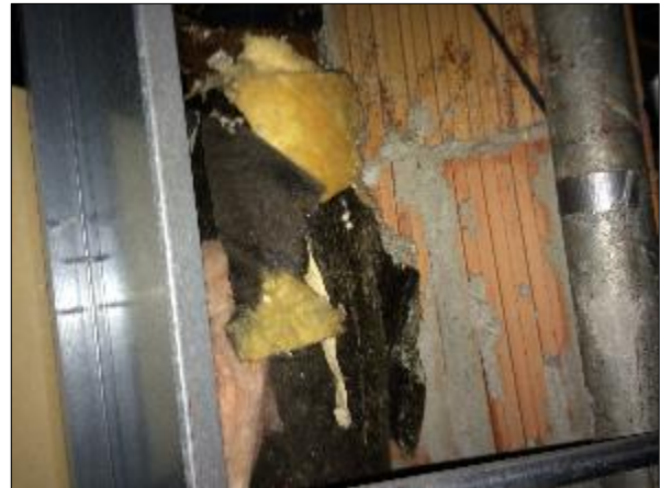
Photo 9 – Non-asbestos black tar paper over fibreglass insulation on pipe straights.
