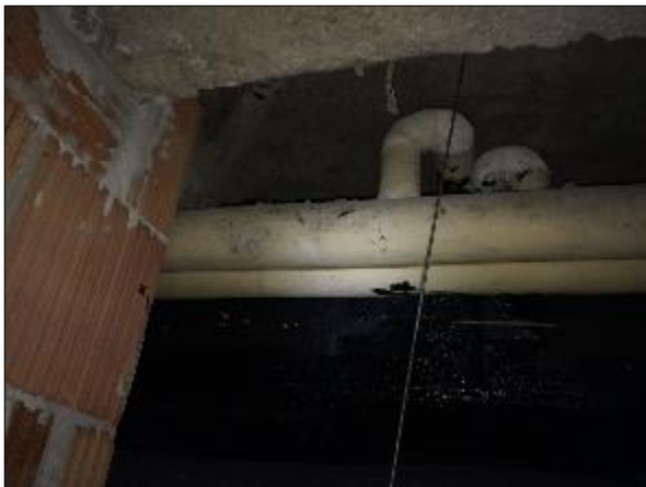
Photo 6 – Friable parging cement insulation on pipe fittings in ceiling space
