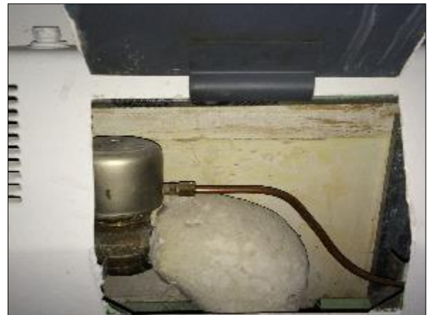
Photo 7 – Friable parging cement insulation on pipe fittings associated with the perimeter heating system.
