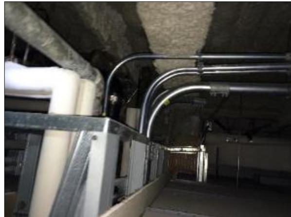
Photo 4 – Newer grey sprayed fireproofing in the print area – East Wing Phase 3A. Remnant asbestos-containing fireproofing was identified
