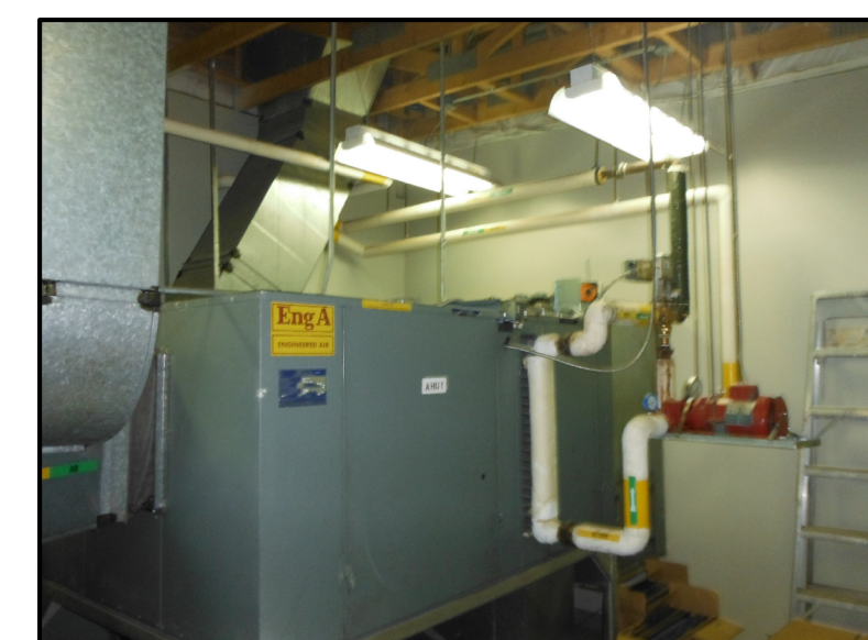
FIGURE 8: EXISTING AIR HANDLING UNIT TO BE REFURBISHED - MECHANICAL ROOM 205.
