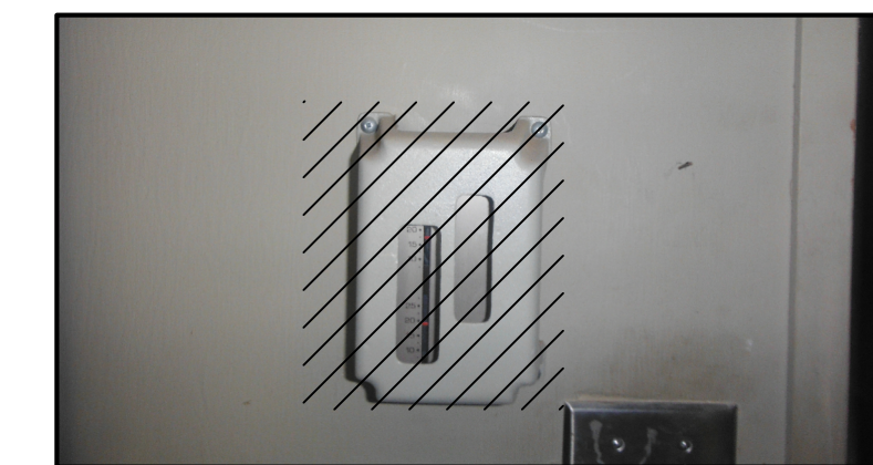
FIGURE 4: EXISTING THERMOSTAT TO BE REMOVED - CARPENTRY WORKSHOP 120.
