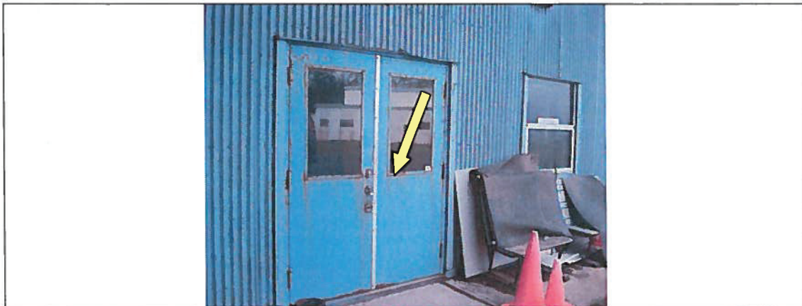
Typical asbestos-containing black window putty applied to glazing of the exterior man doors.
