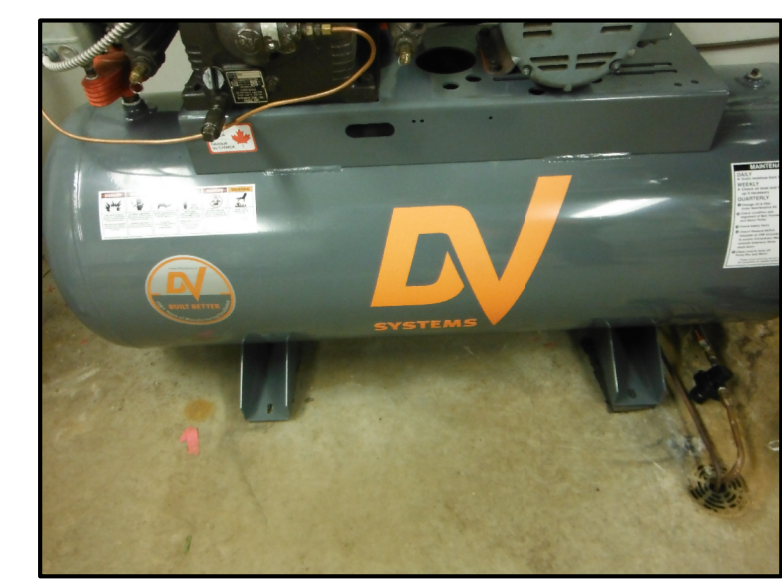
FIGURE 11: EXISTING COMPRESSOR TO BE SEISMICALLY RESTRAINED - MECHANICAL ROOM 205.
