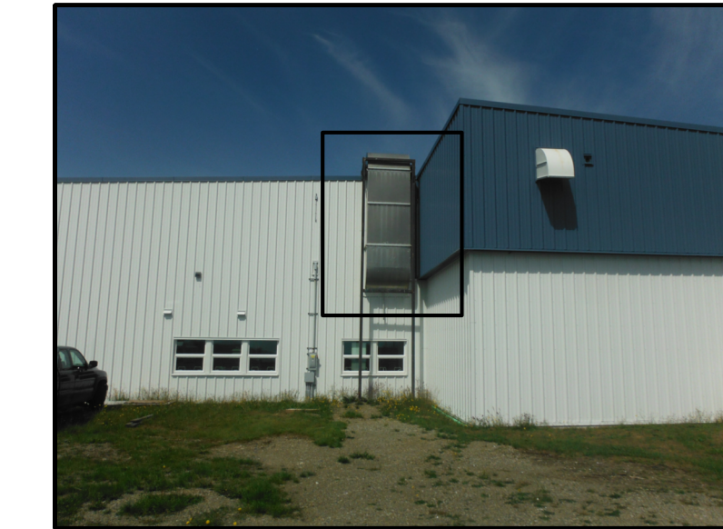
FIGURE 13: EXISTING O/A INTAKE. REINSULATE SECTION INSIDE OF BUILDING WITH 25 mm THERMAL INSULATION - EAST WALL.
