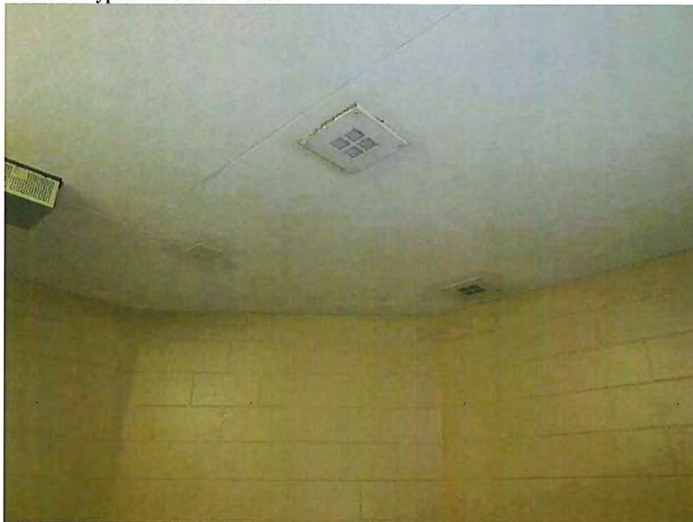
Photo 8 - Typical Ceiling Grills
