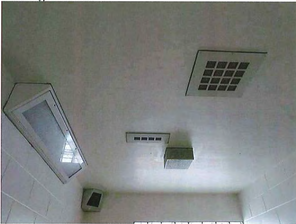
Photo 2 - Typical Ceiling Grills
