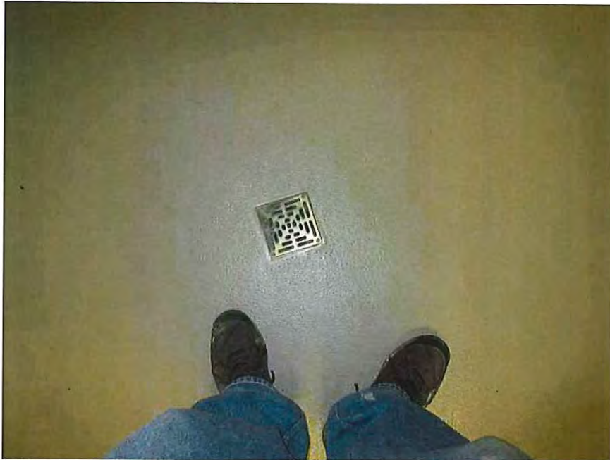
Photo 10 - Typical Floor Drain
