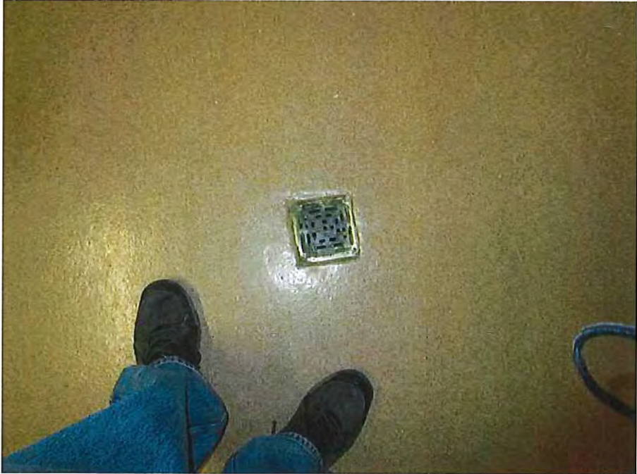
Photo 6 - Typical Floor Drain
