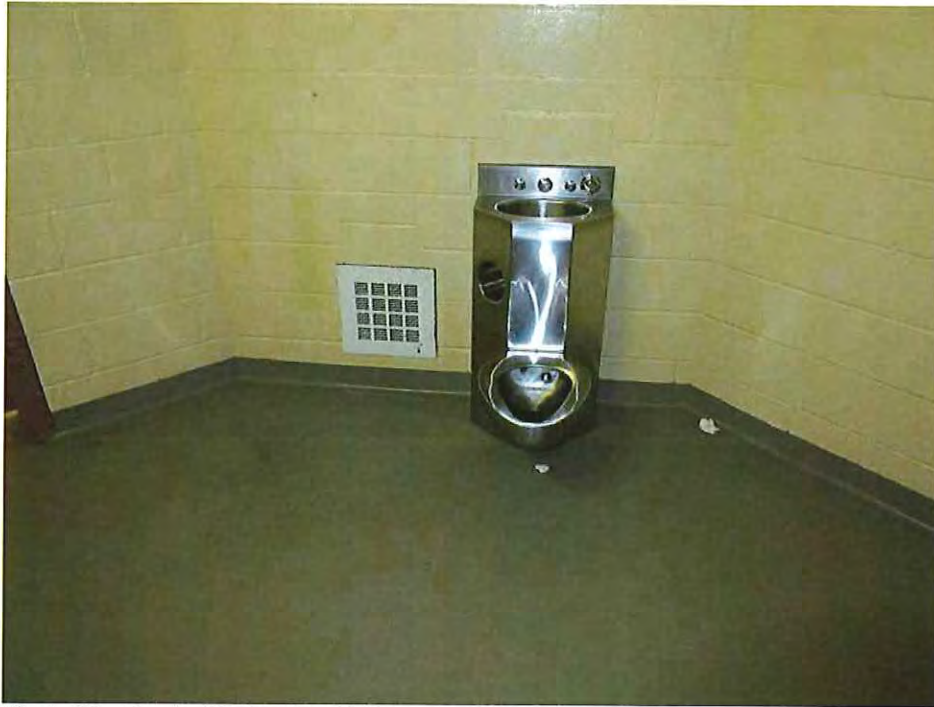
Photo 11 - Typical Detention Toilet
