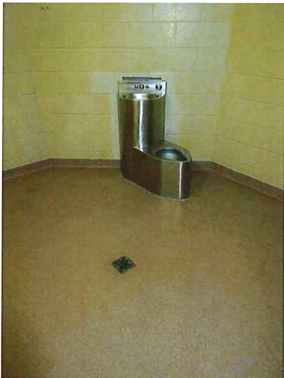
Photo 7 - Typical Detention Toilet
