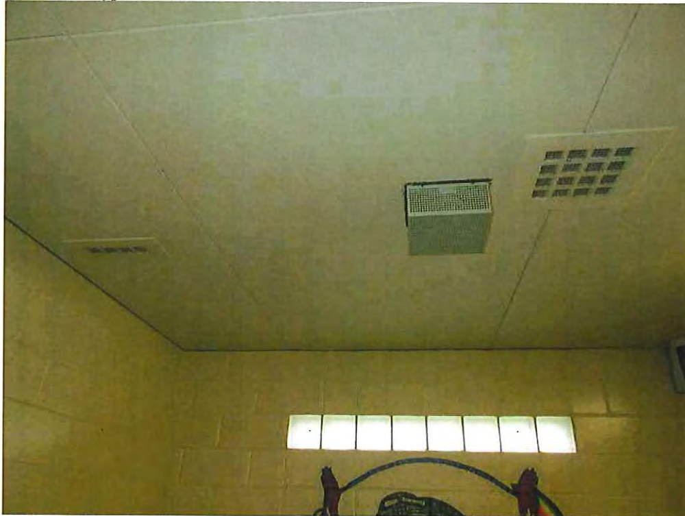
Photo 12 - Typical Ceiling Grille
