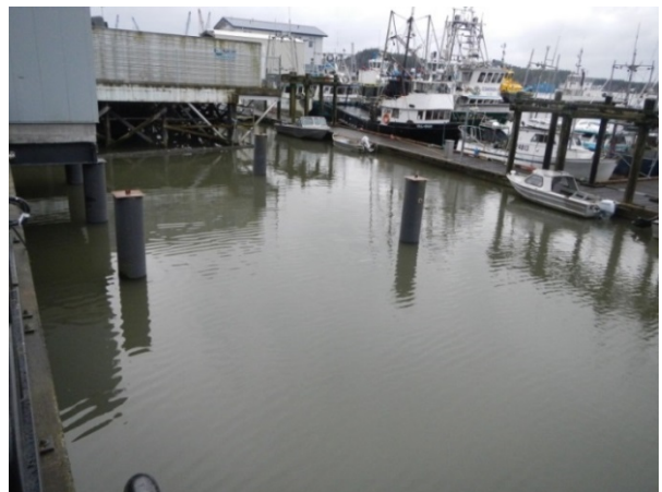
Photo 1-2 Project Site looking South showing Marina Floating Docks and Existing Steel Pilings
