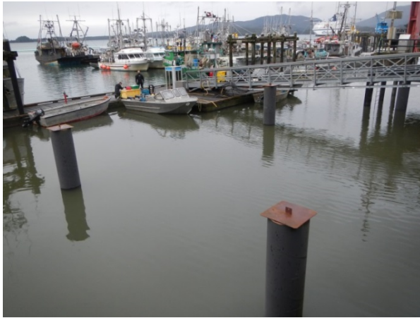
Photo 1-3 Project Site looking West showing Marina Floating Docks and Existing Steel Pilings
