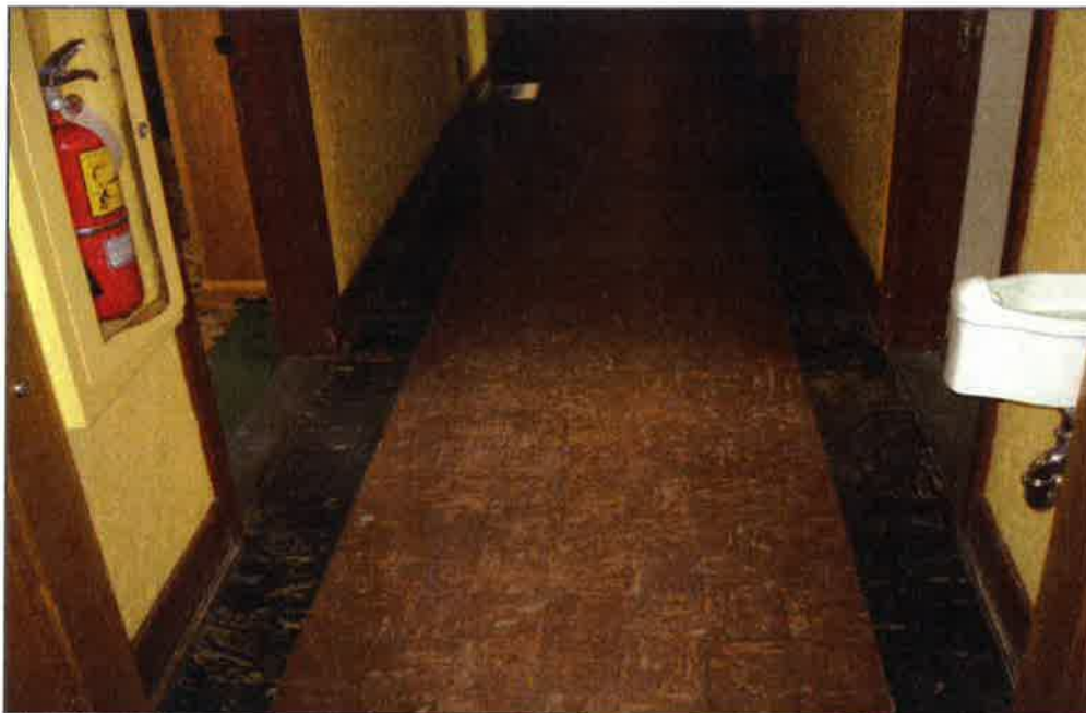
Photo 17: Asbestos containing 6"x6" brown vinyl floor tiles and 4"x4" black vinyl floor tiles as seen on the first floor. EBA sample No.Admin-004 and Admin-010.
