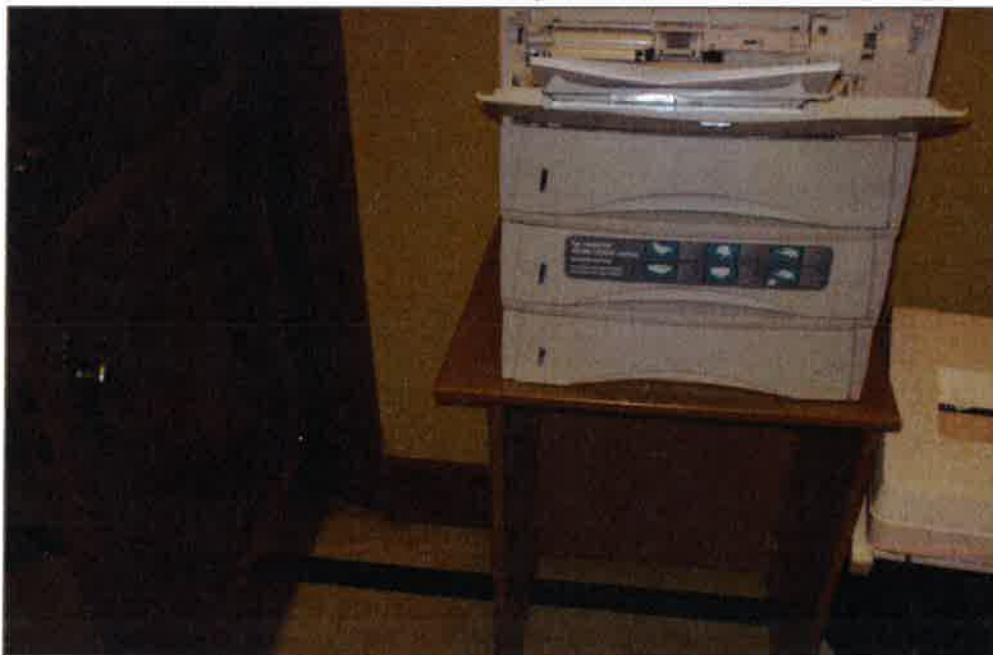
Photo 18: Asbestos containing texture coat on the wall of the Photocopy room on the main floor. EBA sample No.Admin-012.
