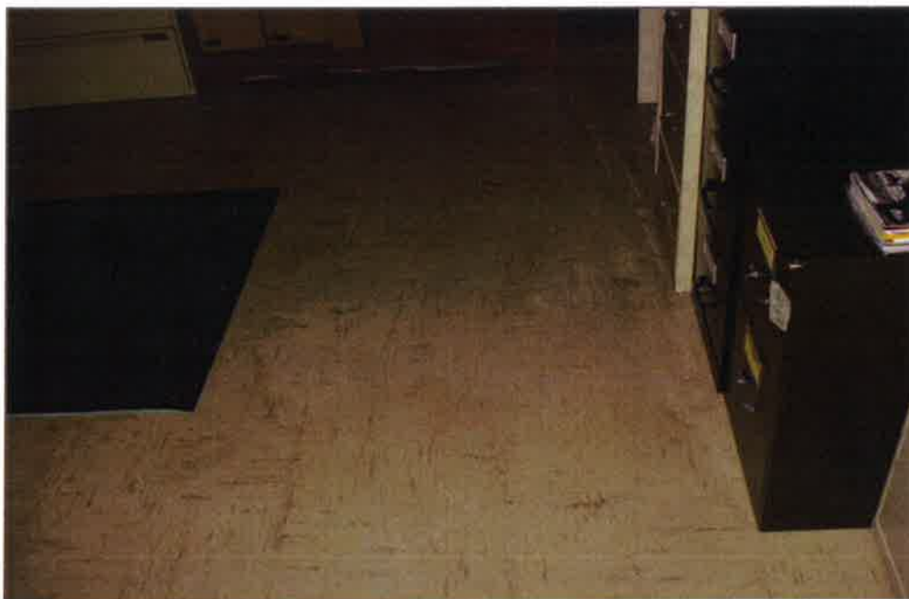
Photo 15: Asbestos containing 12"x12" dark beige vinyl floor tile located in the basement records room. EBA sample No.Admin-001.
