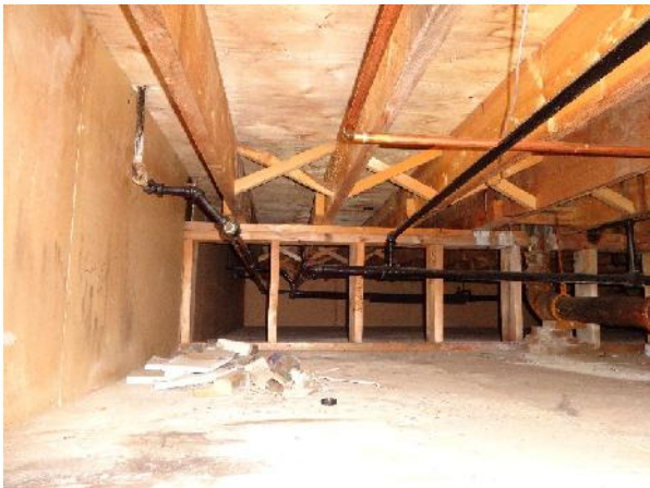
Photo 27: View of structural members within crawlspace of 18 Camsell Place. Crawlspace is approximately 0.9 m in height.
