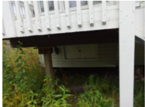
Photo 2: View of one of four exterior crawlspace entry points to 66/68 Alder Drive.
