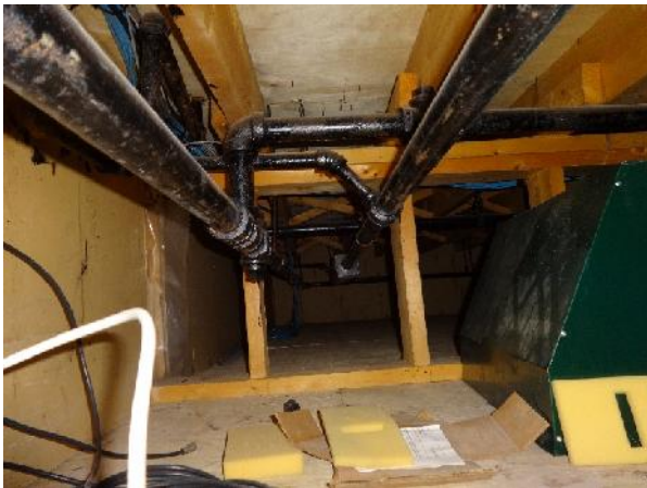
Photo 15: View of structural members within crawlspace of 15 Nanuk Place. Crawlspace is approximately 1.0 m in height.
