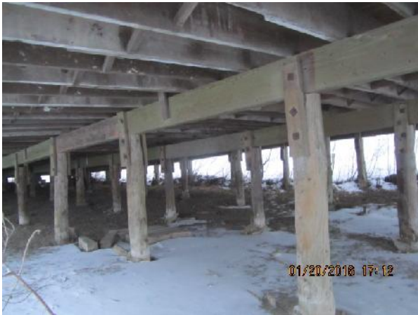
Photo 39: View of structural members under crawlspace of Warehouse #3. Approximately 1.0 m crawlspace height underneath building.
