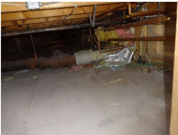
Photo 35: View of associated piping within crawlspace of 221 Mackenzie from exterior entry point.
