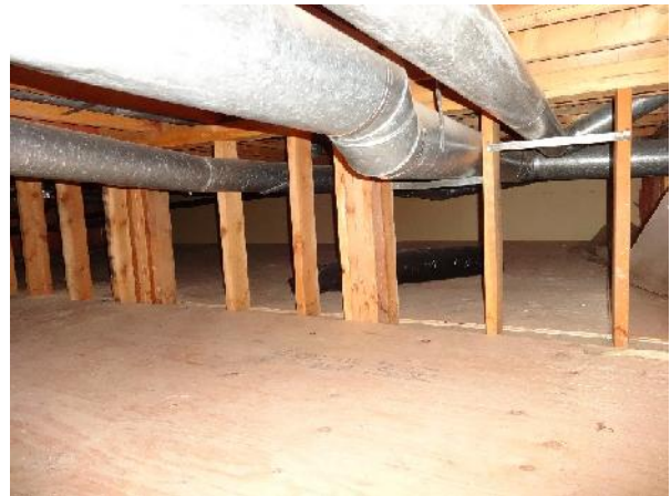
Photo 4: View of structural members and associated piping within crawlspace of 66 and 68 Alder Drive.
