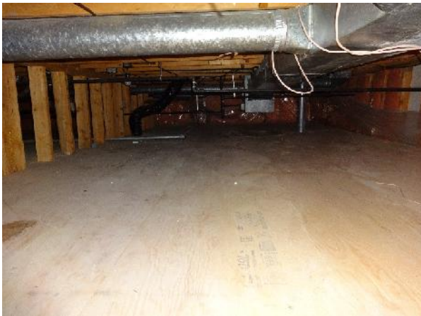
Photo 3: View of structural members and associated piping within crawlspace of 66 and 68 Alder Drive. Crawlspace is approximately 1.1 m in height.
