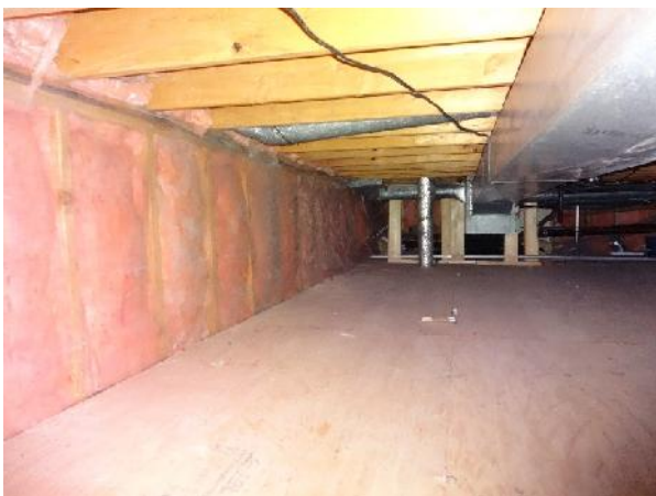
Photo 5: View of structural members and associated piping within crawlspace of 66 and 68 Alder Drive.
