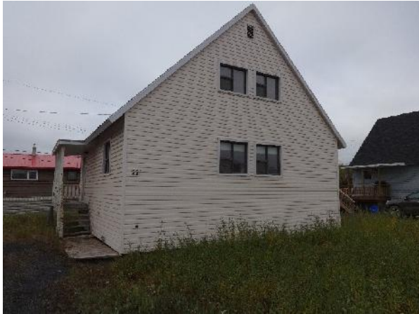
Photo 31: View of exterior 221 Mackenzie Road building. Attached overhead lines located on south side of building.
