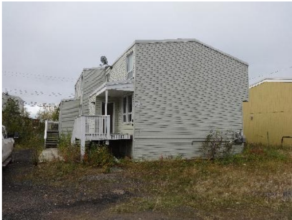
Photo 1: View of exterior 66/68 Alder Drive. Attached overhead lines located on south side of building.
