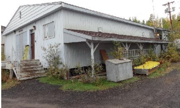
Photo 43: View of exterior Trade Shop building located in PWGSC compound. Approximately 1.0 m crawlspace height underneath building.
