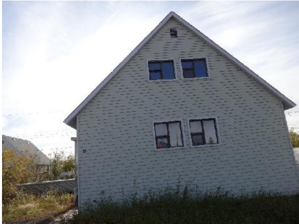
Photo 25: View of exterior 18 Camsell Place. Attached overhead lines located on south side of building.
