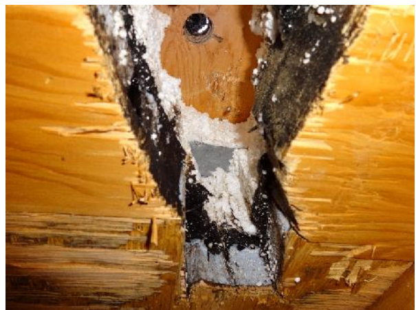
Photo 12: View of roof building material layers above initial interior plywood associated with the ceiling system at 66 and 68 Alder Drive. Building layers include from interior to exterior: plywood, sheeting insulation, asphalt paper, sheeting insulation, plywood and asphalt.
