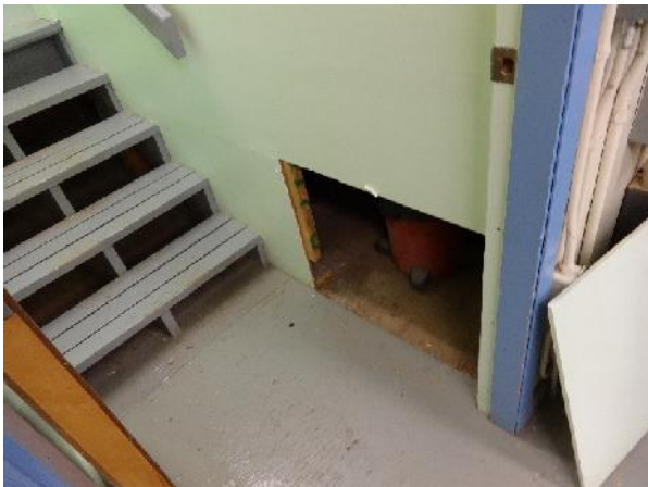
Photo 51: View of access point to interior crawlspace underneath bathroom in the Trade Shop. Crawlspace has an approximate height of 0.8 m. Bathroom is raised above main floor level of Trade Shop.
