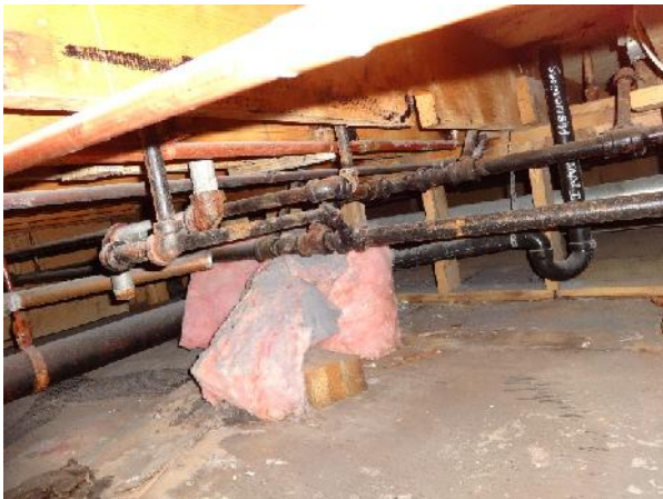
Photo 33: View of structural members and associated piping within crawlspace of 221 Mackenzie Road. Crawlspace is approximately 1.0 m in height.
