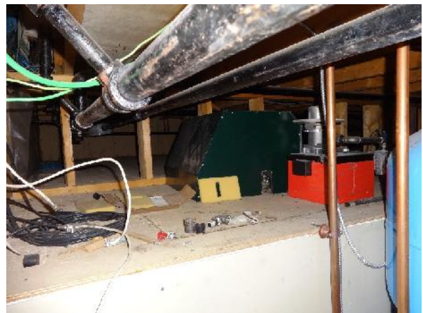
Photo 18: View of mechanical systems and associated piping located within crawlspace of 15 Nanuk Place.
