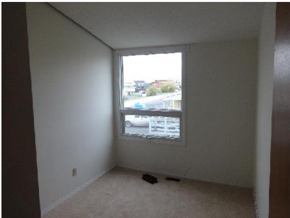
Photo 9: View of second floor bedroom at 66 and 68 Alder Drive with ceiling pitch and approximate ceiling height of 2.6 m.
