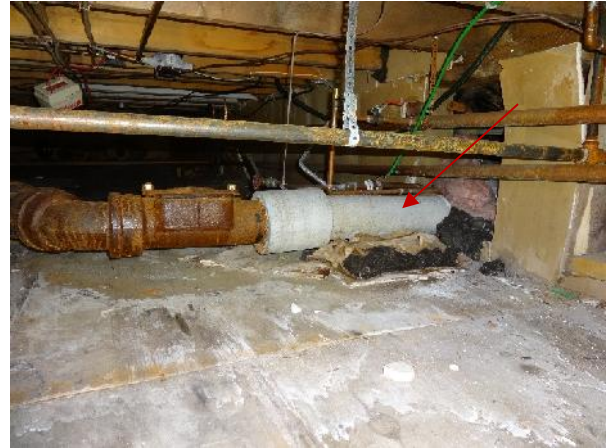
Photo 86: View of associated piping within crawlspace at 18 Camsell Place from exterior entry point..
