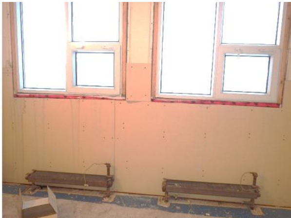
Photo 23: View of wall radiant heat fixtures in living room.
