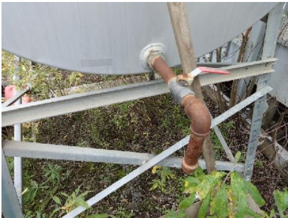
Photo 45: View of disconnected discharge line on AST south of Trade Shop. The AST has been disconnected and is a standalone containment used to store former heating diesel oil. No visual staining observed under AST.
