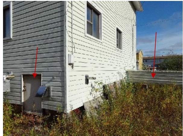
Photo 14: View of door access to crawlspace underneath building and utility corridor located on west and south side of 15 Nanuk, respectively.
