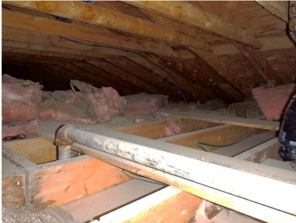
Photo 22: View of structural members and associated piping within attic space of 15 Nanuk Place.
