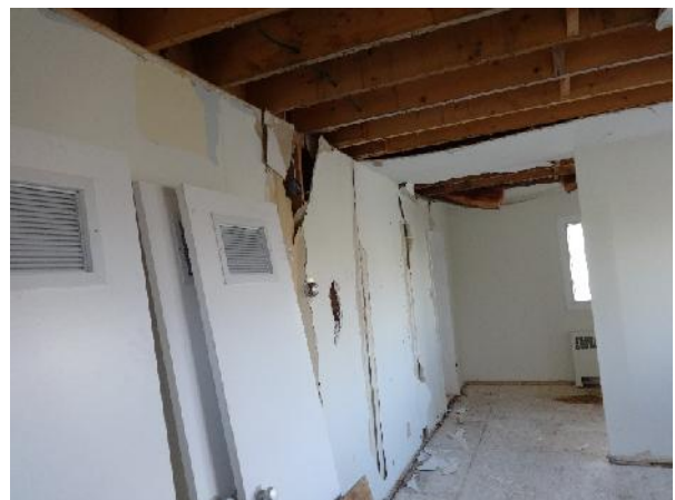
Photo 30: View of ceiling joists located in 18 Camsell Place. Ceiling height is approximately 2.4 m.
