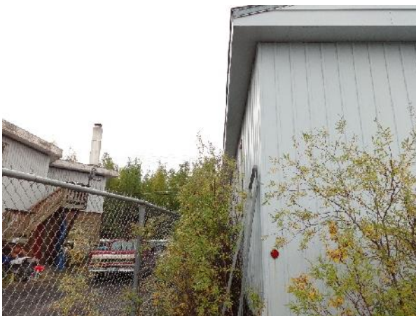
Photo 47: View of fence line for property boundary approximately 1.5 m north of Trade Shop building.
