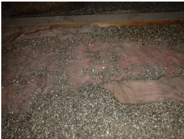
Photo 11: Samples ACM- 15, 16 and 17, vermiculite, were determined to contain Actinolite asbestos fibres.
