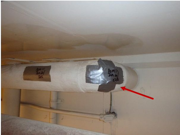
Photo 7: Sample ACM-12; Main Loop, East – West Line, pipe fitting insulation was determined to contain 2-60% Chrysotile asbestos fibres.
