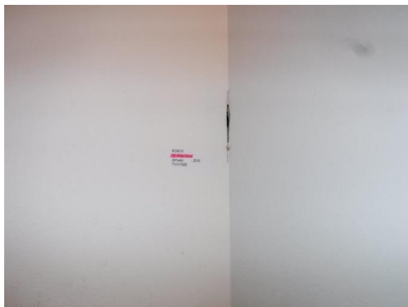
Photo 7: Sample ACM-01 – 68 Alder; Gypsum board joint compound in main floor bathroom was determined to contain 2% Chrysotile asbestos fibres.
