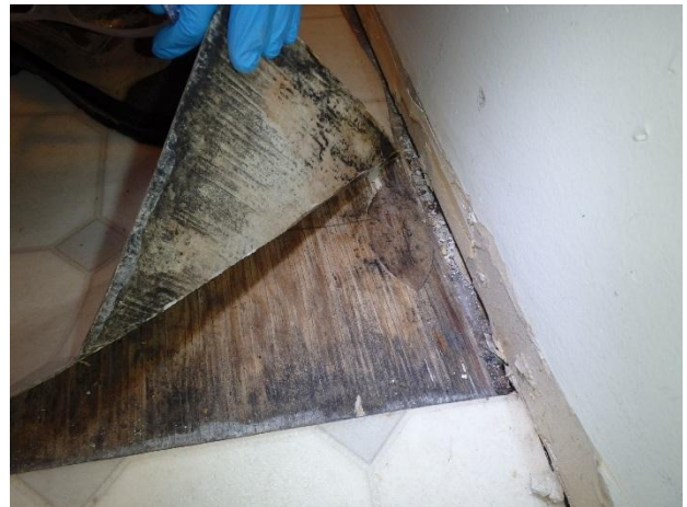
Photo 22: SVG observed on underside of flooring in side entrance.
