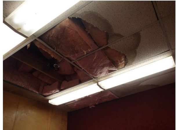
Photo 26: View of water damaged suspended ceiling tiles in the northeast office. Note the fluorescent light tubes suspected to contain mercury.
