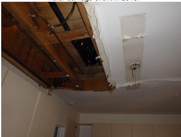
Photo 9: View of kitchen ceiling. Water damage in the building was a result of a leaking toilet on the second level.
