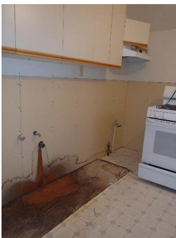
Photo 17: Water damage and SVG observed in kitchen.
