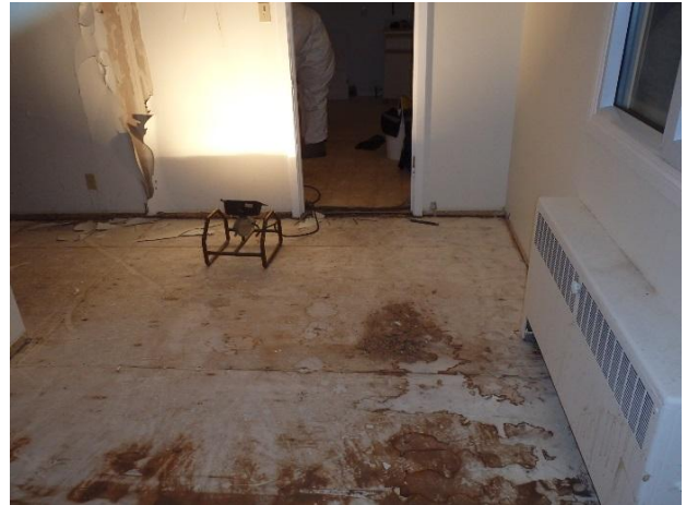
Photo 8: Most floors in building were observed to be have been stripped to the subfloor.
