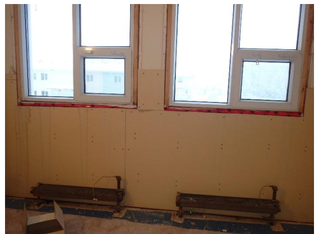
Photo 18: Water damage observed below bedroom windows on repaired sections of gypsum board.
