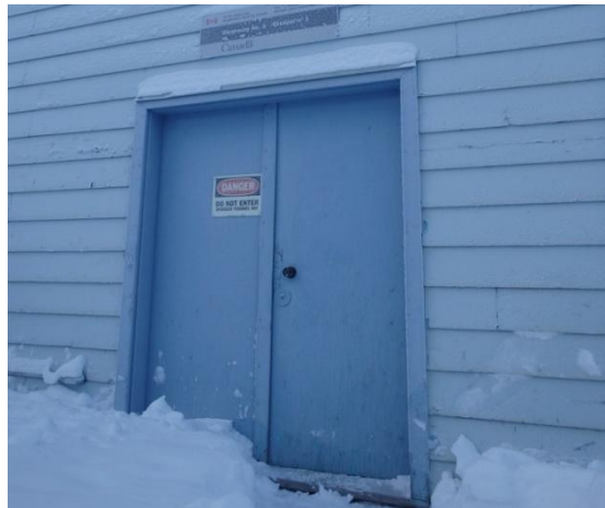
Photo 8: Sample PB01/ TCLP20 – 72 Franklin, four layers of paint on warehouse exterior doorways; grey, green, white, grey contains 12,100 mg/kg and 8.40 mg/l lead.
