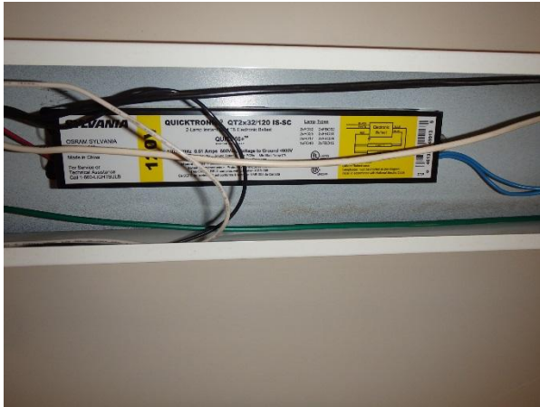
Photo 25: View of a typical fluorescent light ballast observed at the site with a manufacturer’s label noting “no-PCB”.
