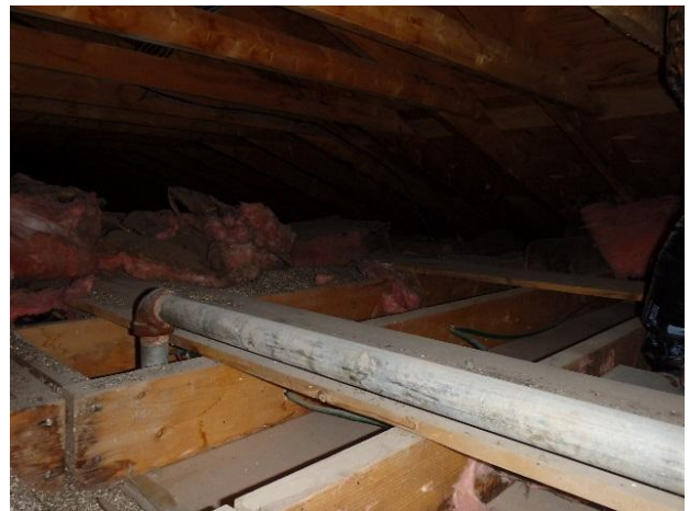
Photo 12: Vermiculite was observed to have been placed above (with traces below) pink fibreglass insulation.
