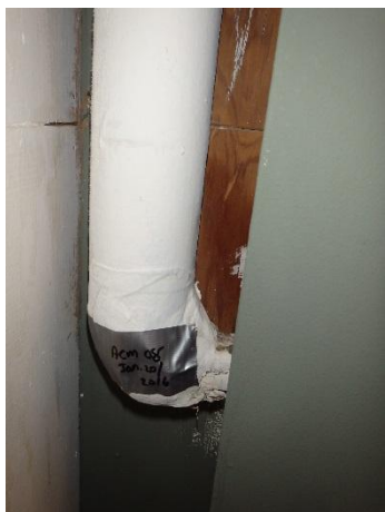
Photo 5: Sample ACM-08; Front Office, next to bottom rad, pipe fitting insulation was determined to contain 5-60% Chrysotile asbestos fibres.
