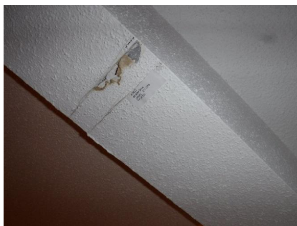
Photo 6: Sample ACM-22 – 66 Alder; Texture finish (stipple) on ceiling in 2 nd floor utility room was determined to contain 2% Chrysotile asbestos fibres.
