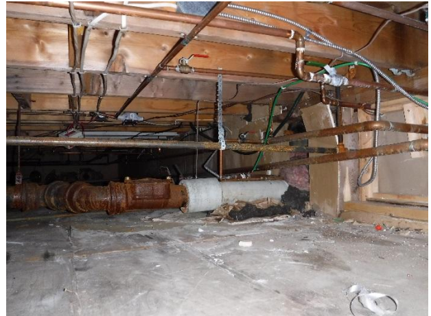
Photo 2: Sample ACM-26, crawl space, coupler connecting 152 mm dia. cast iron and cementitious waste-water pipes was determined to contain 30% Chrysotile and 5% Crocidolite asbestos fibres.
