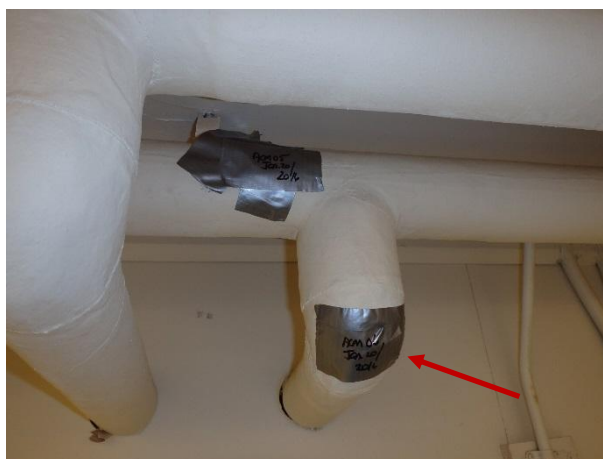
Photo 4: Sample ACM-06; Exiting South Line, Veering South, pipe fitting insulation was determined to contain 10-50% Chrysotile asbestos fibres.
