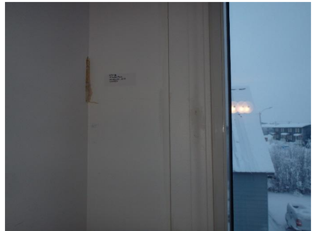
Photo 8: Sample ACM-12, GBJC, upstairs bedroom was determined to contain 5% Chrysotile asbestos fibres.
