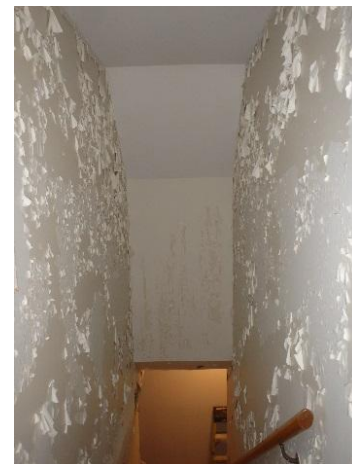
Photo 12: View of staircase walls showing extensive paint damage.
