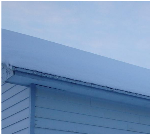
Photo 7: Samples ACM-01 and 02 – 72 Franklin, two layers of grey/black shingles on the warehouse roof. No asbestos fibres detected.
