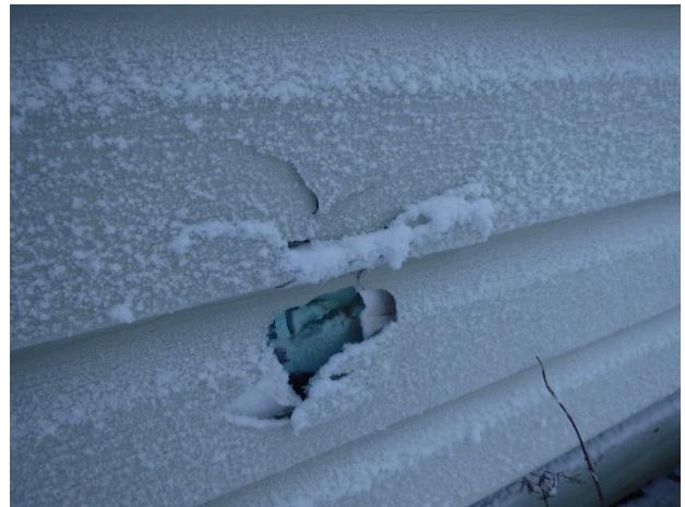
Photo 28: Damaged exterior siding, paper wrap house wrap Sample ACM-19, no asbestos fibres detected.
