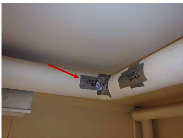
Photo 3: Sample ACM-04; Main Loop, NE Corner, pipe fitting insulation was determined to contain 5-65% Chrysotile asbestos fibres.
