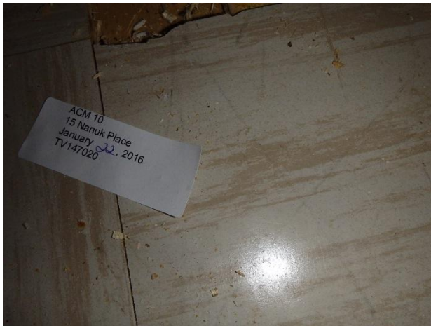
Photo 7: Sample ACM-10, vinyl floor tile 305 x 305 mm, master bedroom (and adjacent bedroom) was determined to contain 5% Chrysotile asbestos fibres.
