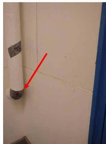
Photo 6: Sample ACM-10; Front Entrance pipe fitting insulation was determined to contain 10% Chrysotile asbestos fibres.
