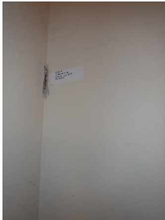
Photo 9: Sample ACM-13, GBJC, upstairs utility room was determined to contain 3% Chrysotile asbestos fibres.
