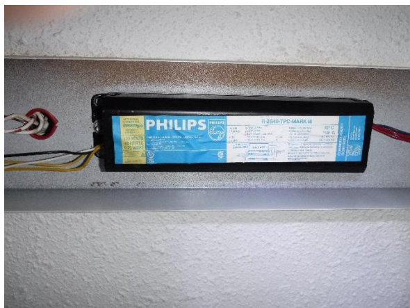
Photo 23: View of ballast associated with fluorescent light fixture in 66 Alder Drive, labelled as non-PCB.
