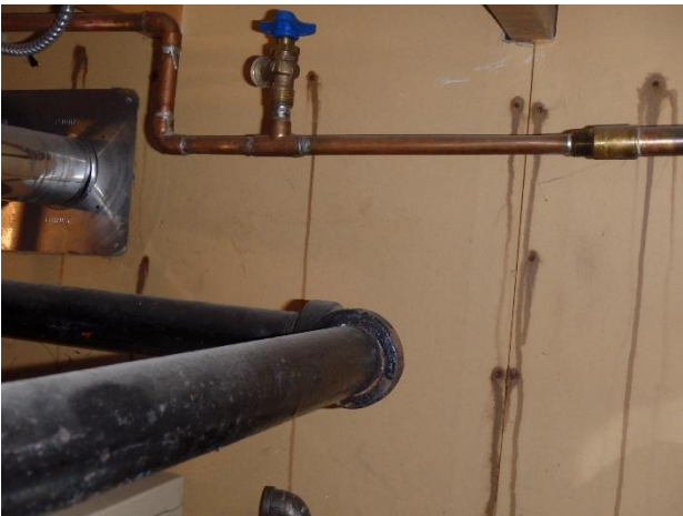
Photo 27: Cast iron piping observed in crawl space.
