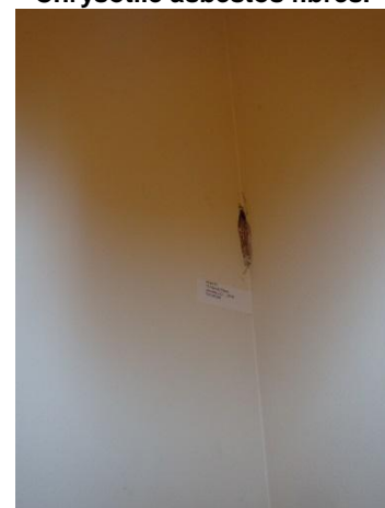
Photo 6: Sample ACM-07, GBJC – lower level entrance was determined to contain 5% Chrysotile asbestos fibres.
