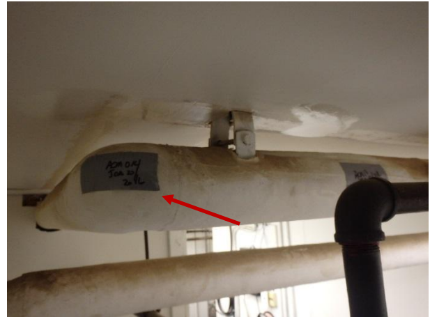
Photo 8: Sample ACM-14; Mechanical Room, 125mm pipe elbow insulation was determined to contain 10% Chrysotile asbestos fibres.
