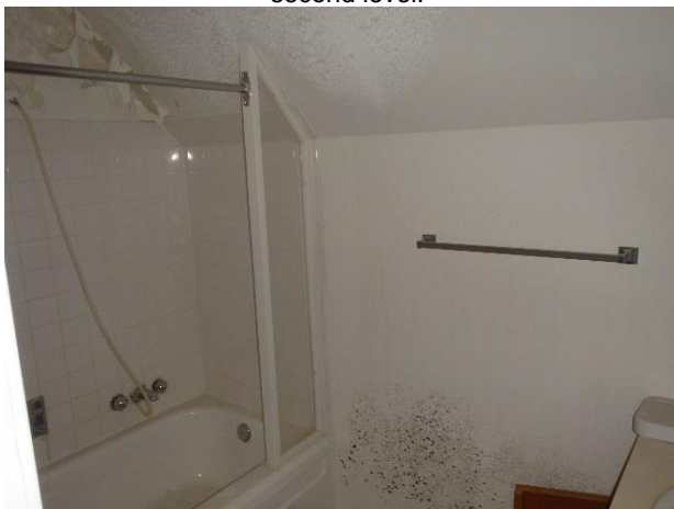
Photo 17: SVG observed to cover lower portion of wall in bathroom in former location of toilet.
