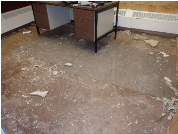
Photo 27: View of water damaged materials on the floor in the back office area.
