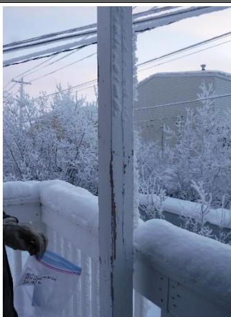
Photo 19: Sample PB-01 – 68 Alder; white paint located on exterior deck column was determined to have a total lead concentration of 223 mg/kg and a TCLP concentration of 0.225 mg/L.
