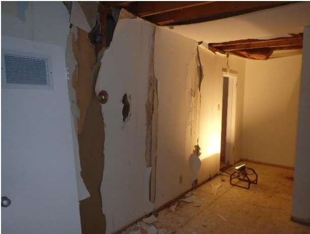
Photo 7: View of living room/dining room wall and ceiling. Site has had no heat and minimal electrical supply since water damage event in 2010.
