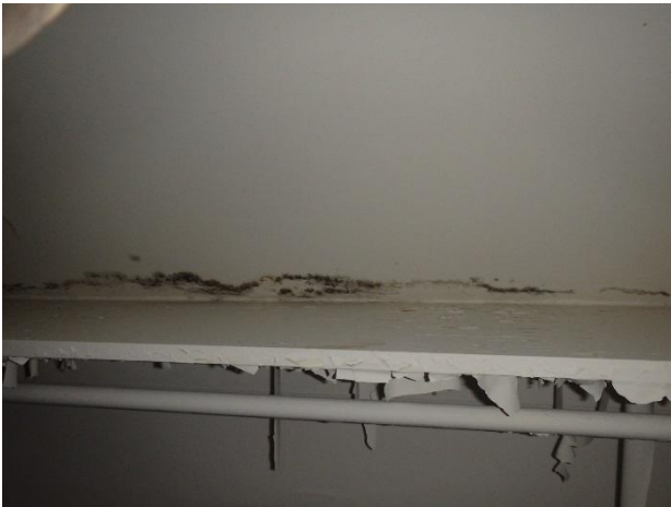
Photo 13: SVG observed in the master bedroom closet.
