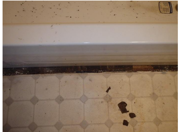
Photo 20: Water intrusion observed on sub-floor along tub in bathroom.
