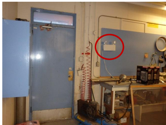
Photo 24: View of emergency lighting on wall suspected to contain a lead acid battery.
