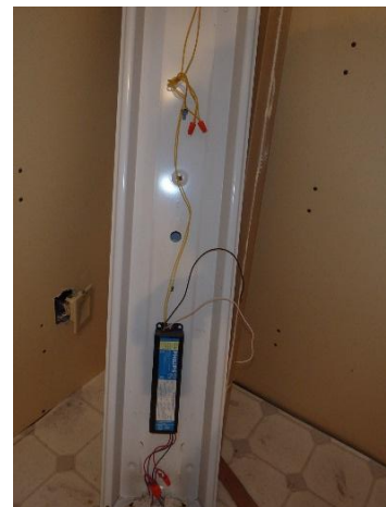
Photo 16: Ballast labelled "No PCBs" observed in fixture on floor in kitchen.
