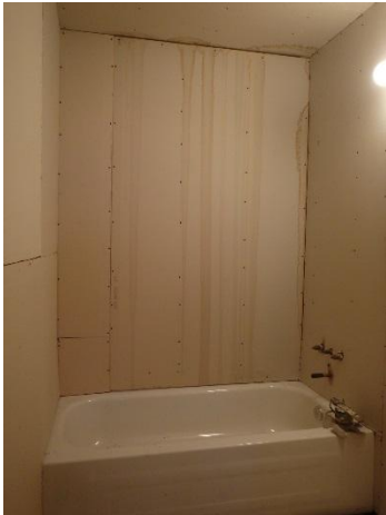
Photo 19: Water damage observed on walls and ceiling surrounding tub in bathroom.
