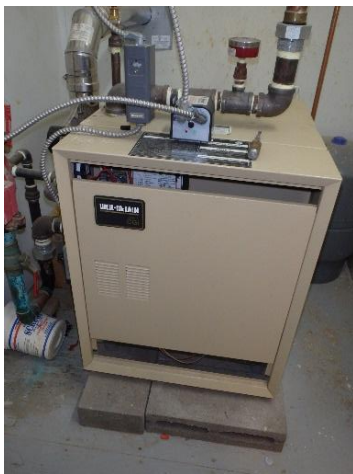
Photo 29: View of the gas fired boiler.
