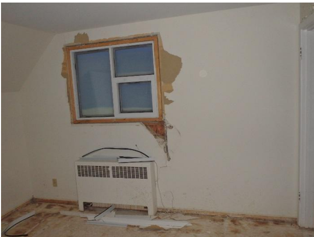
Photo 15: SVG and water damage observed to extend over most of the exterior wall in smaller bedroom on second level.
