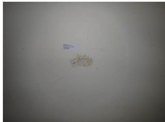
Photo 10: Sample ACM-18, GBJC on closet wall in Bedroom 2, was determined to contain 3% Chrysotile asbestos fibres.
