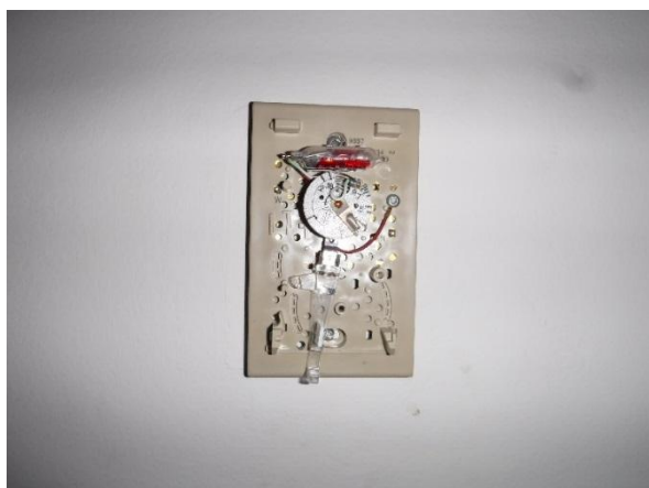
Photo 21: View of mercury containing thermostat observed in the living room of 68 Alder Drive.
