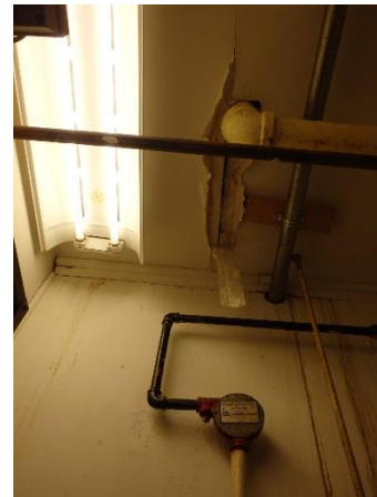
Photo 28: View of water damaged gypsum board ceiling the in boiler room.
