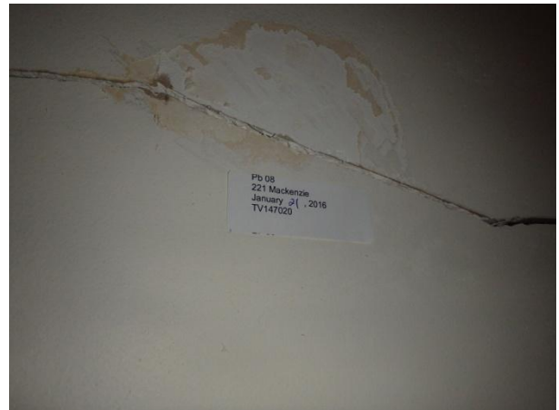
Photo 8: Sample ACM-13 GBJC from crack in stairway wall opposite lower level bedroom was determined to contain 2% Chrysotile asbestos fibres.
