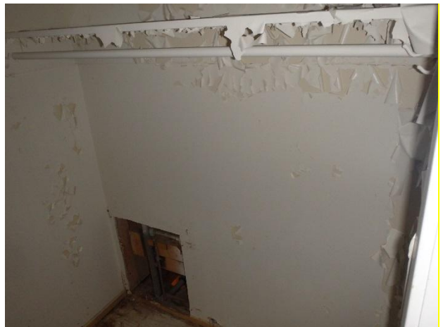
Photo 16: View of extensive paint damage in closet smaller bedroom on second level.
