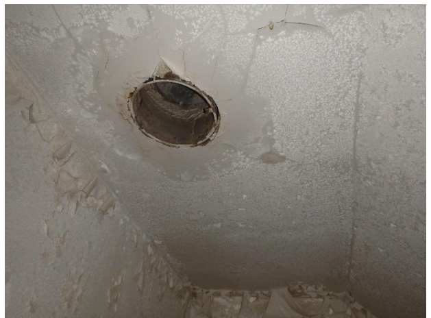
Photo 18: View of bathroom ceiling showing damaged paint and the presence on frost on the ceiling.
