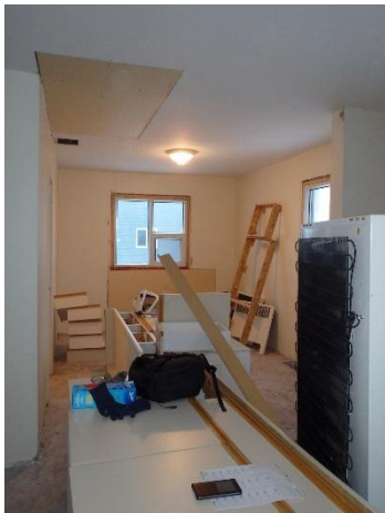
Photo 3: Dining room, wall and ceiling repairs visible.
