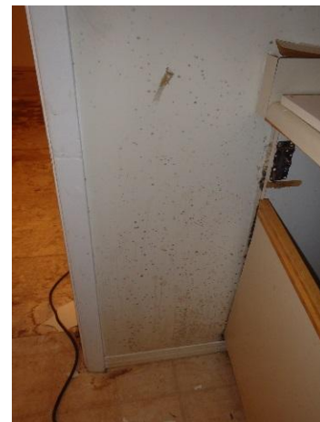
Photo 10: View of surface visible growth (SVG) adjacent to kitchen cabinetry.
