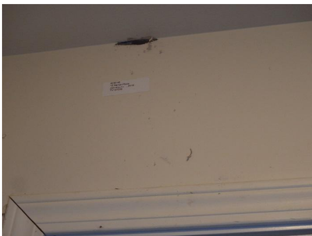
Photo 5: Sample ACM-06, gypsum board joint compound (GBJC), side entrance above exterior door was determined to contain 5% Chrysotile asbestos fibres.
