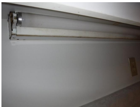
Photo 22: View of typical fluorescent light fixture located beneath kitchen cabinets, note the mercury containing light tube.
