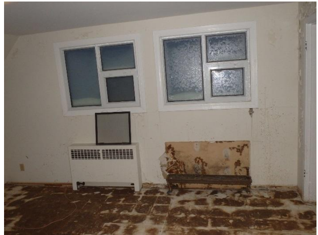
Photo 14: SVG and water damage observed to extend over most of the exterior master bedroom wall.
