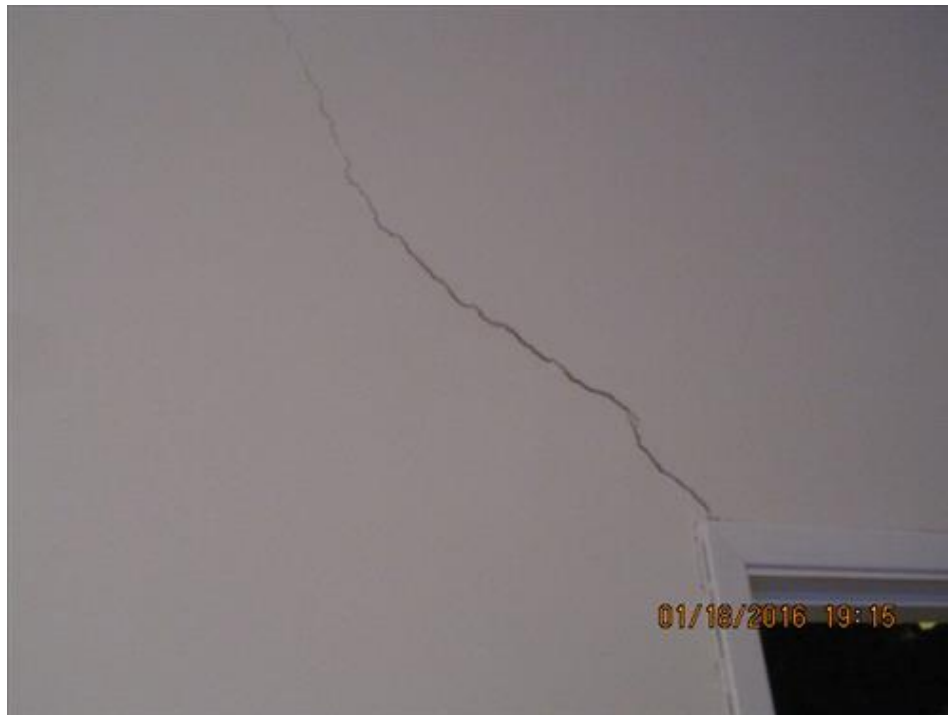
Photograph 92- Severe diagonal crack at the top corner of the south bedroom door on second floor-House #68
