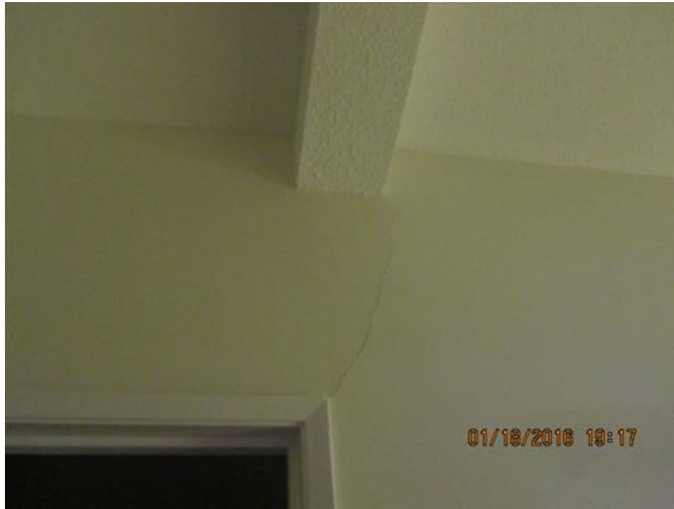
Photograph 95- Diagonal crack above the door to utility room on second floor, on hall side-House #68
