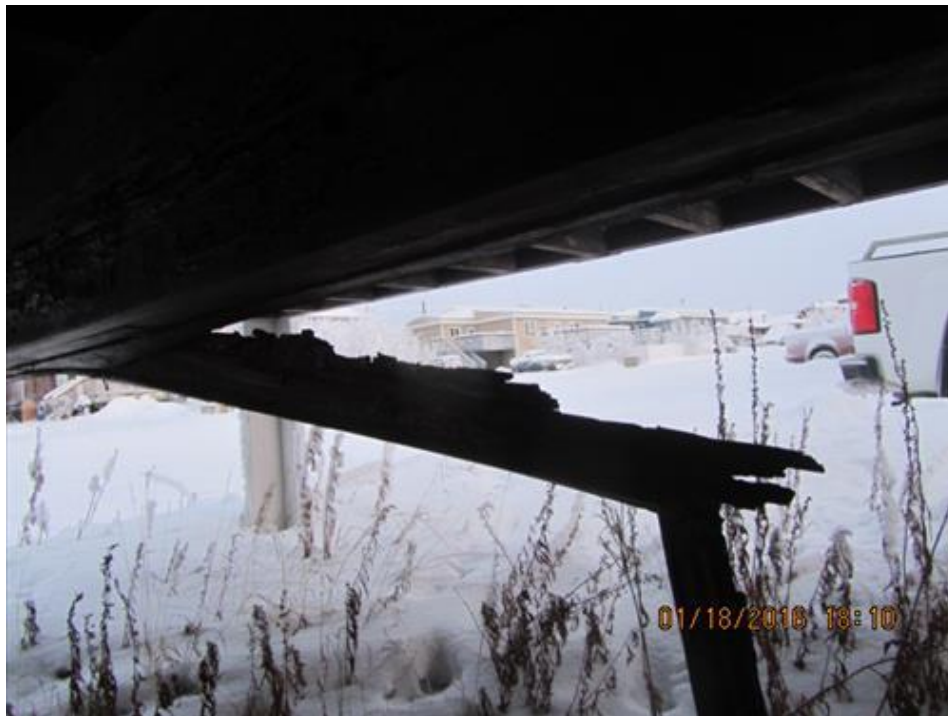
Photograph 42- Decayed and severely damaged beam under the front porch of House #66
