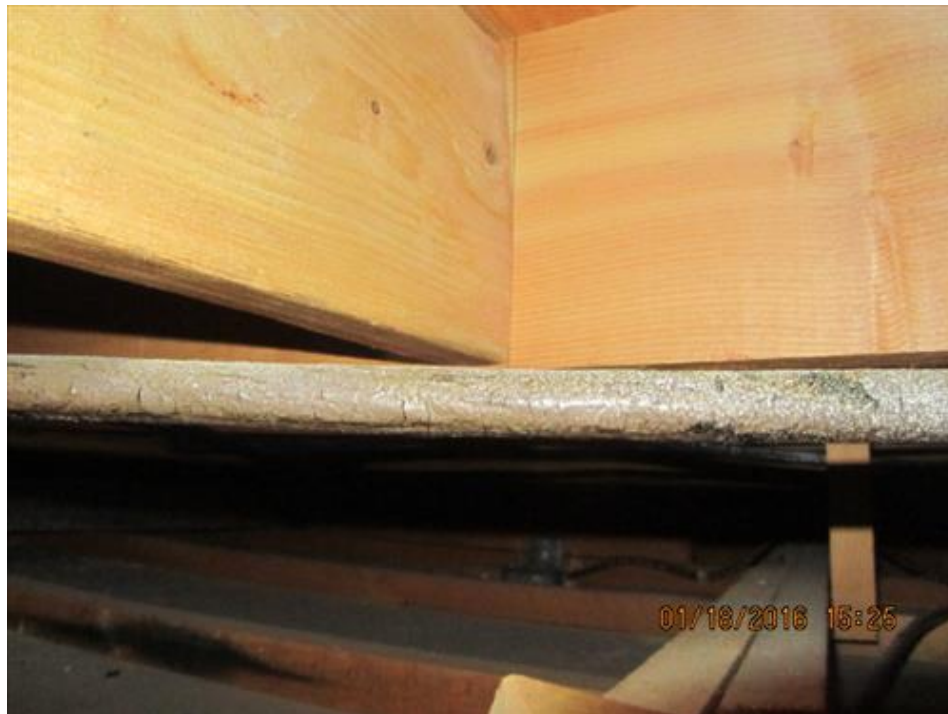
Photograph 30- Condition of second level floor joists, viewed through the plumbing maintenance hatch within the ceiling of kitchen in House #66
