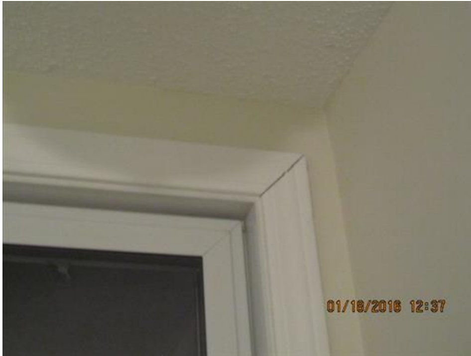
Photograph 73- Open joint within the wood mold around opening between the kitchen and dining room-House #66
