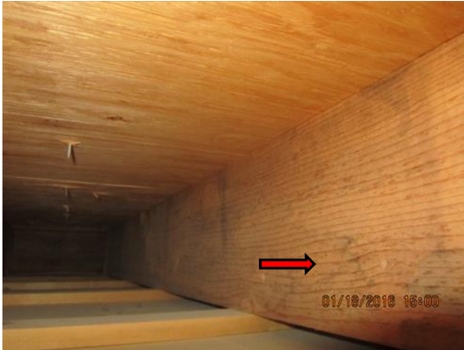
Photograph 37- Minor Water stain noted within the ceiling joist along the west wall of utility room on the second floor of House # 66
