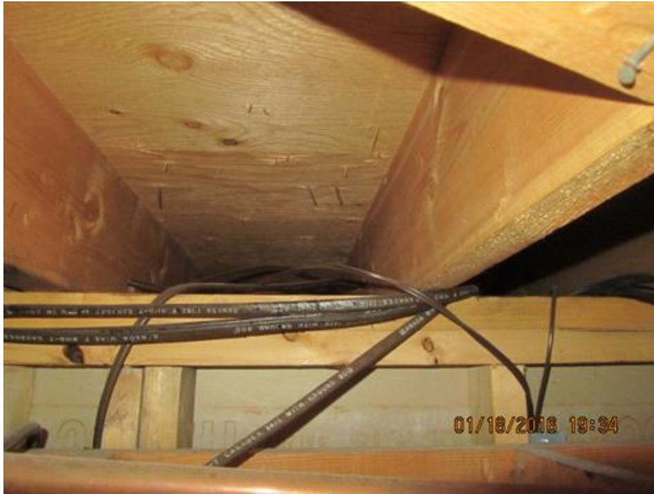
Photograph 31- Condition of second level floor joists and load bearing studs, viewed through the plumbing maintenance hatch within the ceiling of kitchen in House #68
