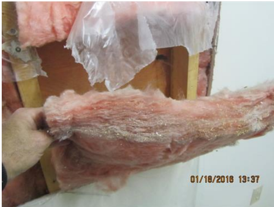
Photograph 26- Condition of studs and sheathing observed within the intrusive cut-out at ground floor level on north wall of House #66
