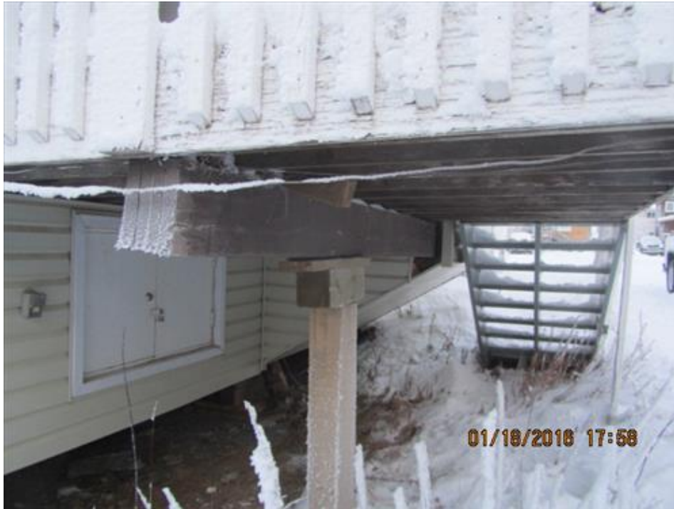
Photograph 41- Twisted main beam under the front porch of House #68
