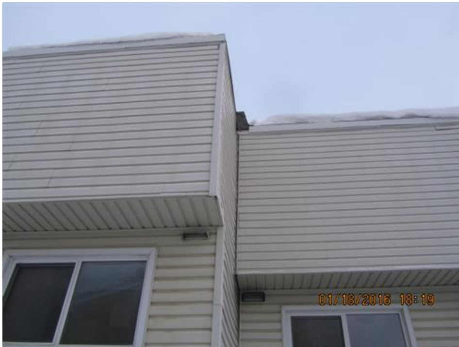
Photograph 38- Separation between Houses #66 and 68 at the top on west elevation
