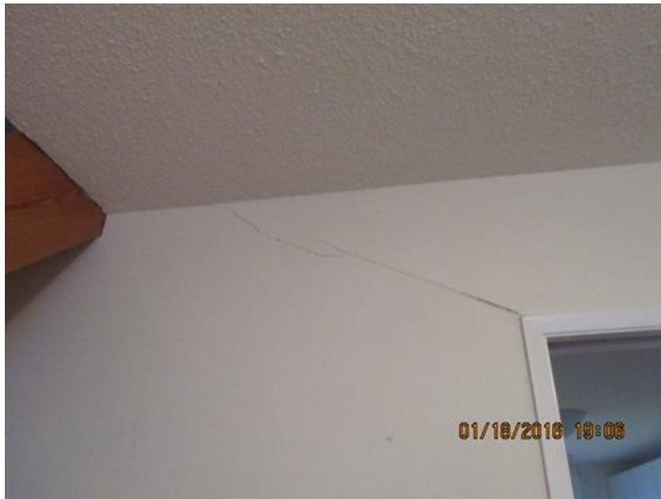
Photograph 84- Severe diagonal crack above the opening between the kitchen and dining room on dining room side-House #68
