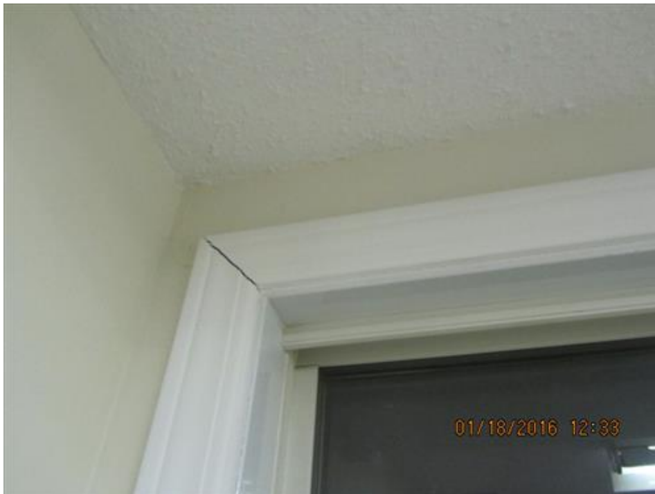
Photograph 74- Open joint within the window frame mold in furnace room-House #66
