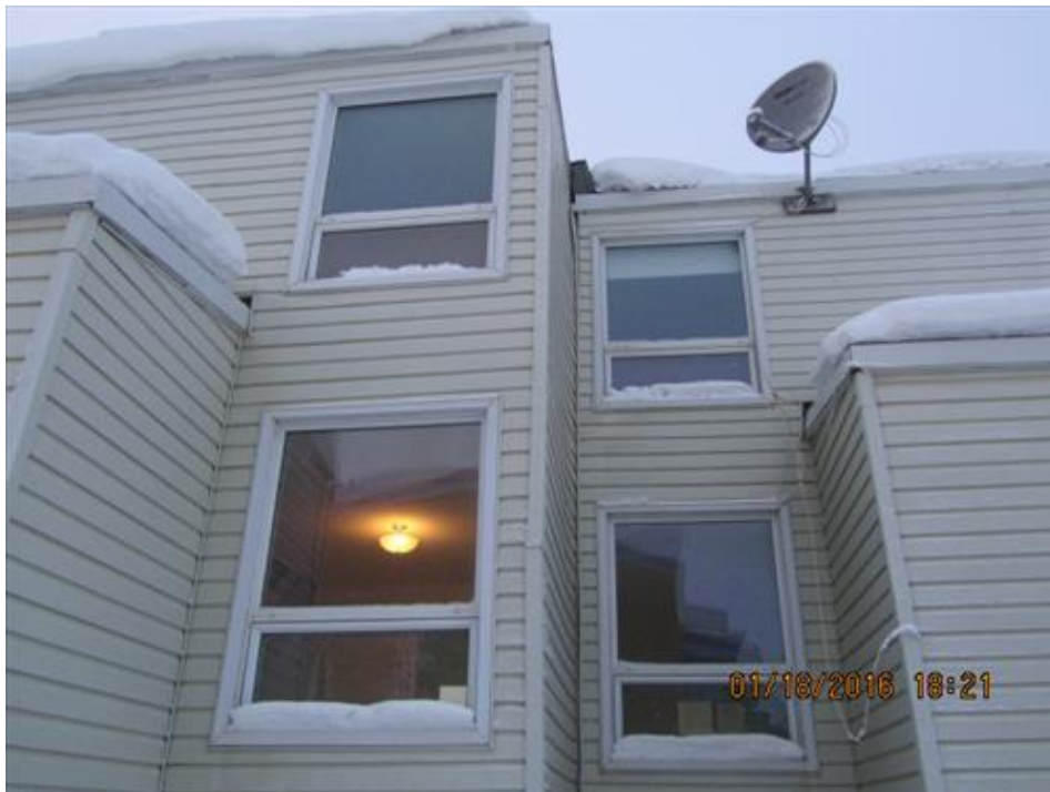
Photograph 40- Separation between Houses #66 and 68 at the mid height on east elevation
