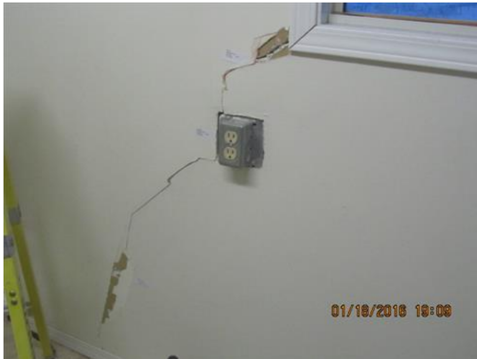
Photograph 88- Severe diagonal crack at the lower left corner of the window of the furnace room within the west exterior wall-House#68
