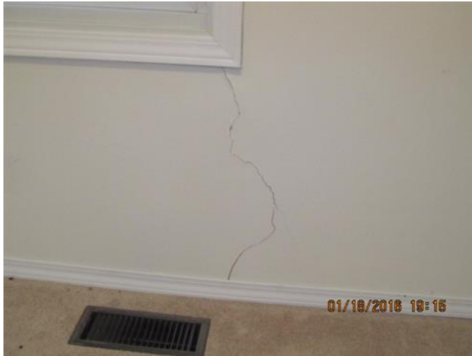
Photograph 93- Severe vertical crack at the lower left corner of the north bedroom window on second floor-House #68
