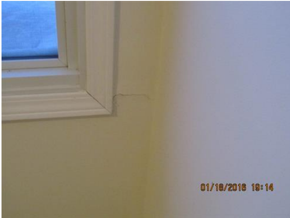
Photograph 91- Horizontal crack at the lower right corner of the window in south bedroom on second floor-House #68
