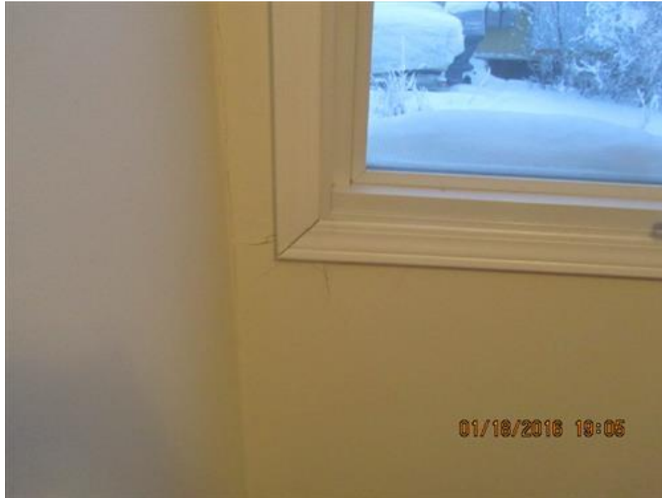
Photograph 83- Cracks at the lower left corner of north window within the east exterior wall, in sitting/living room-House #68
