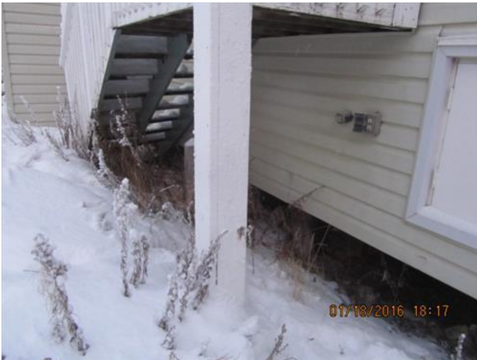
Photograph 16- Built-up wood column, supporting the rear (west) stairs and porch of House #68
