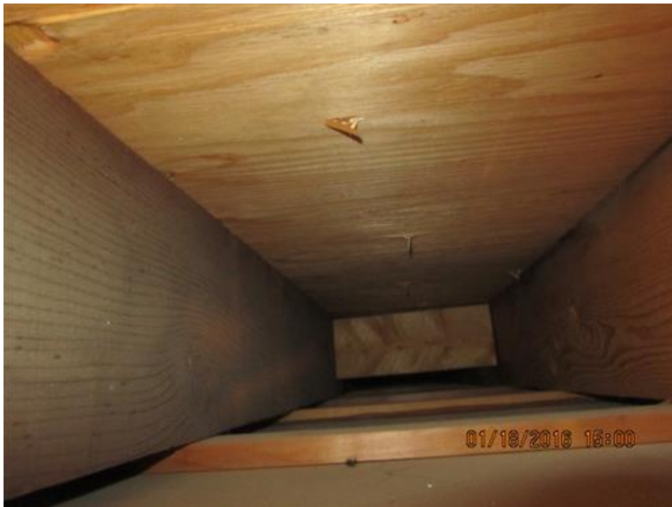
Photograph 28- Condition of ceiling joists and roof sheathing within the plenum of second floor utility room in House #66
