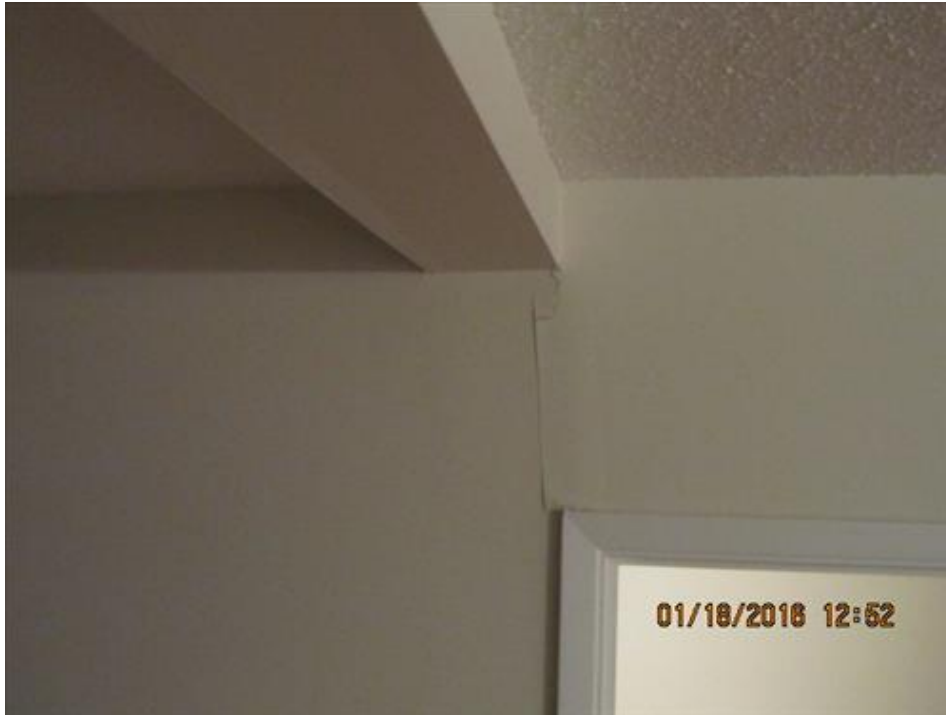
Photograph 69- Vertical crack within the interior loadbearing wall above the opening between the living/sitting room and back foyer and below the beam supporting the second floor-House #66
