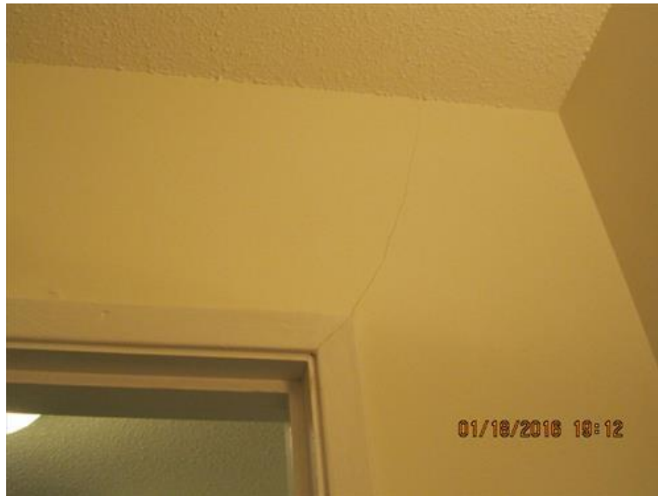
Photograph 90- Radial crack above the ground floor washroom door –House #68
