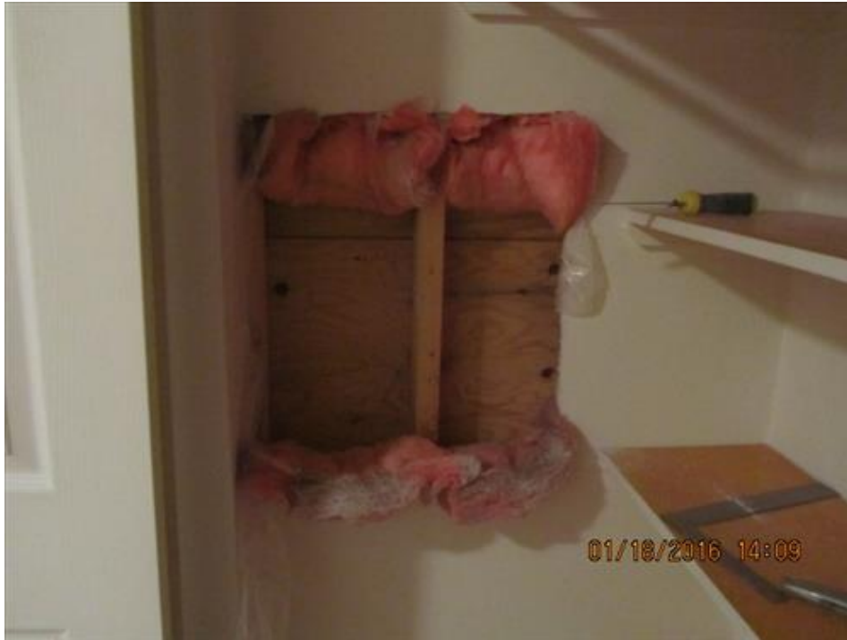
Photograph 27- Condition of studs and sheathing observed within the intrusive cut-out at the second floor level north wall of House #66
