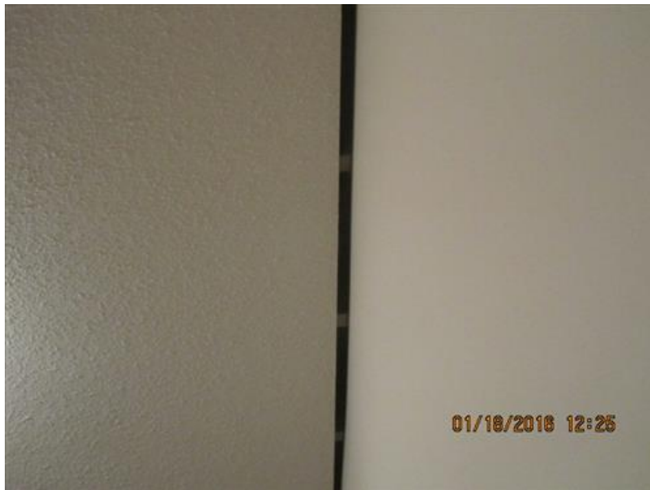
Photograph 104- Perimeter ventilation gap at the intersection of the wall and ceiling on second floor of House #66 (typical)
