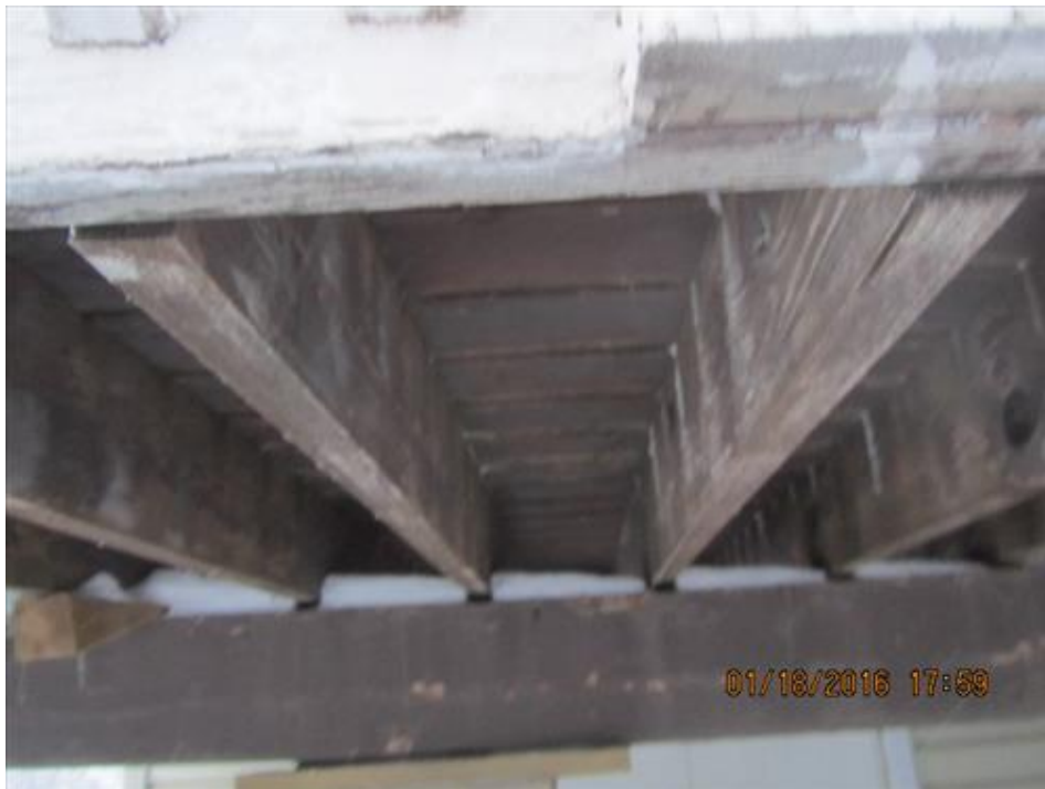
Photograph 14- Deck wood planks, joists, and beams of front porch of house #66, viewed from underside
