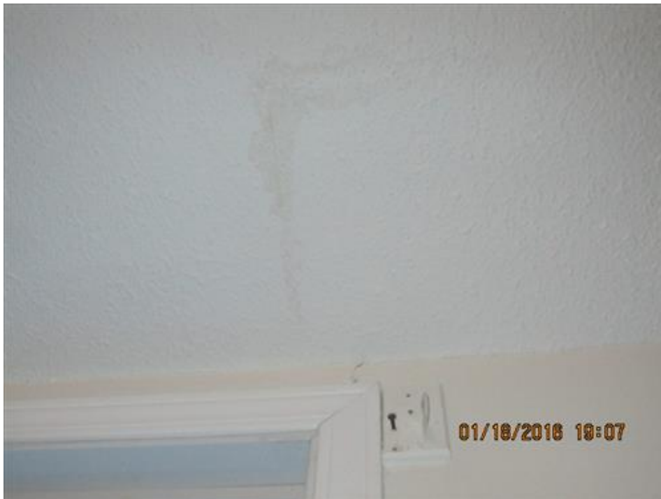
Photograph 86- Crack above the top right corner of the window in the kitchen and within the ceiling
