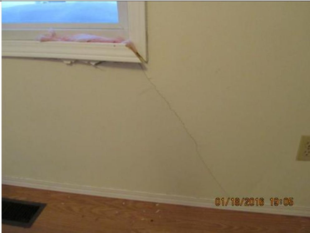
Photograph 82- Severe radial crack and bulging of wall at the lower right corner of north window within the east exterior wall, in sitting/living room-House #68
