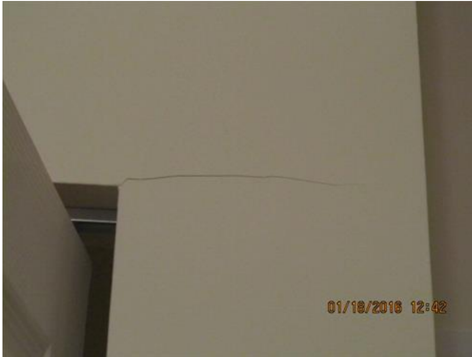
Photograph 67- Horizontal crack above the closet in second floor south bedroom-House #66
