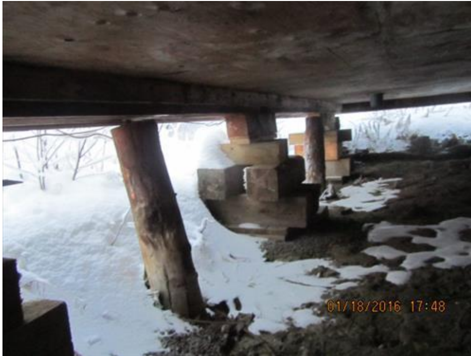
Photograph 17- Failed piles and temporary supports along the south end of House #68
