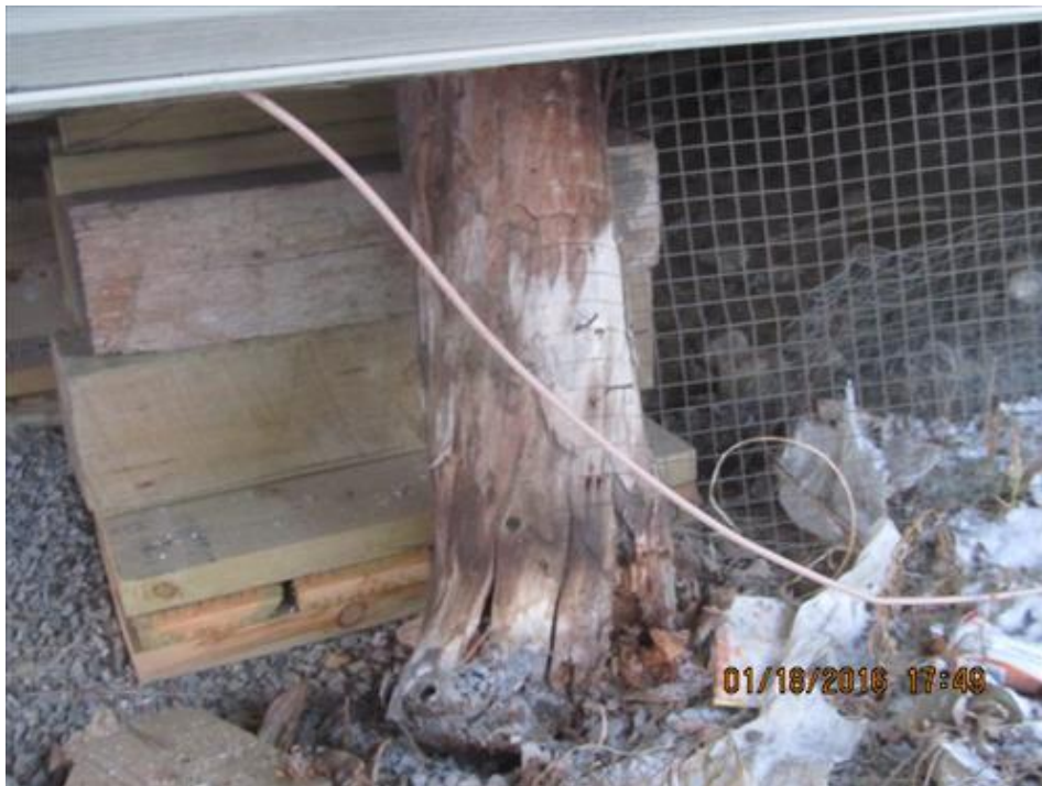
Photograph 24- Decayed pile at the southwest corner of House #66
