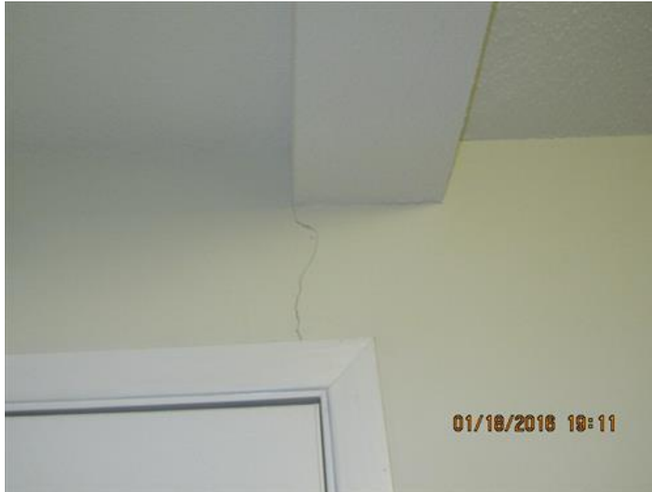
Photograph 89- Vertical crack below the beam and above the back door within the west exterior wall- House #68
