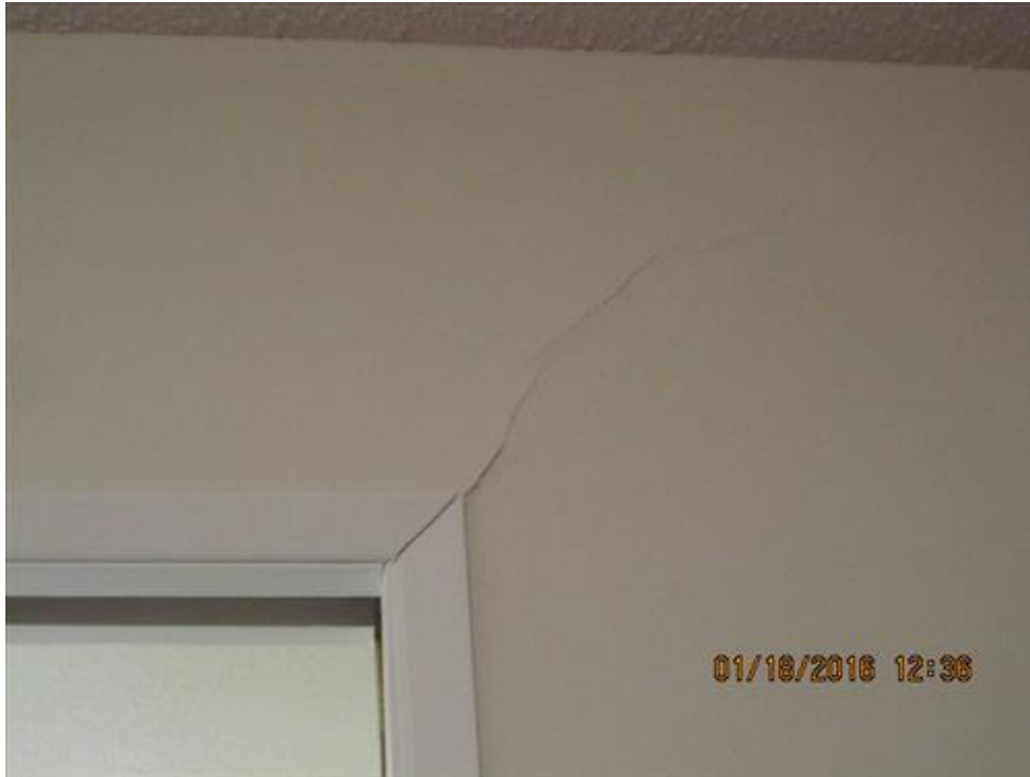
Photograph 65- Diagonal crack above the opening between the kitchen and dining room, on Kitchen side-House #66
