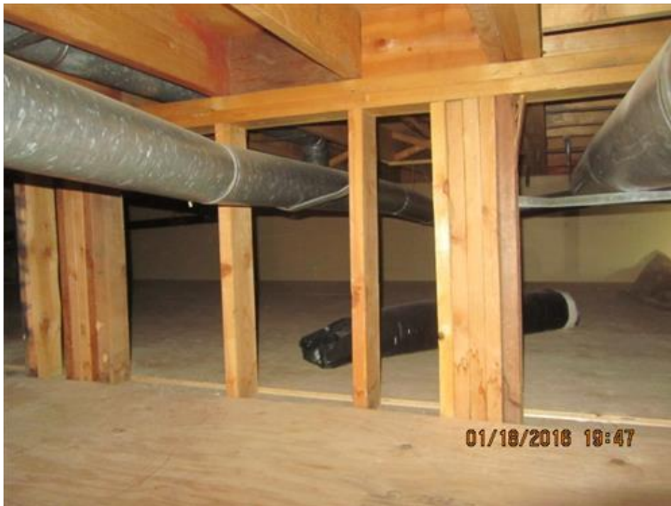
Photograph 8- Load bearing stud frame with built-up columns located at the mid span within the raised enclosed crawl space under the building
