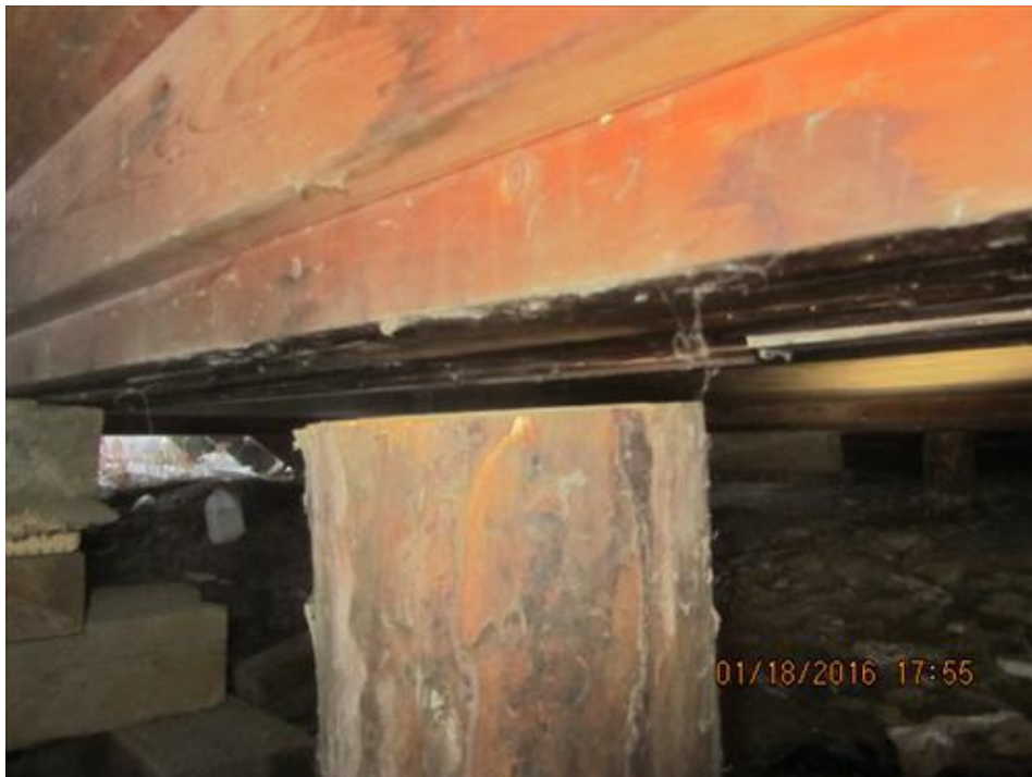
Photograph 22- Wide gap between top of the existing pile and the unsupported beam
