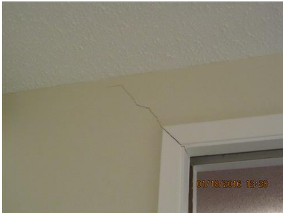
Photograph 64- Diagonal crack above the opening between the kitchen and dining room, on dining room side-House #66
