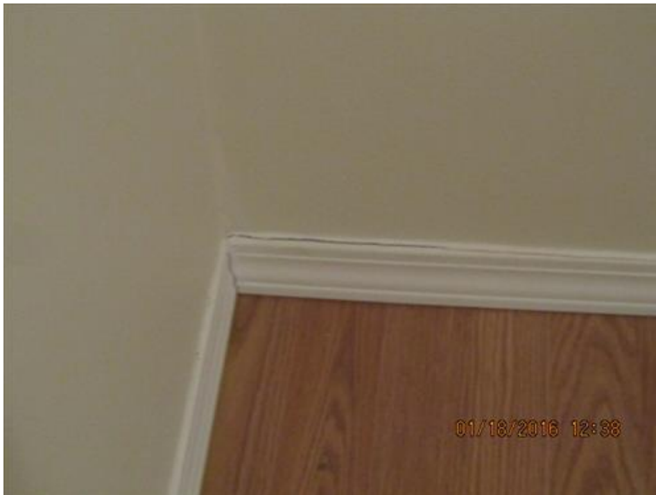
Photograph 76- Separation within the baseboard at the northwest corner of the second floor north bedroom-House #66
