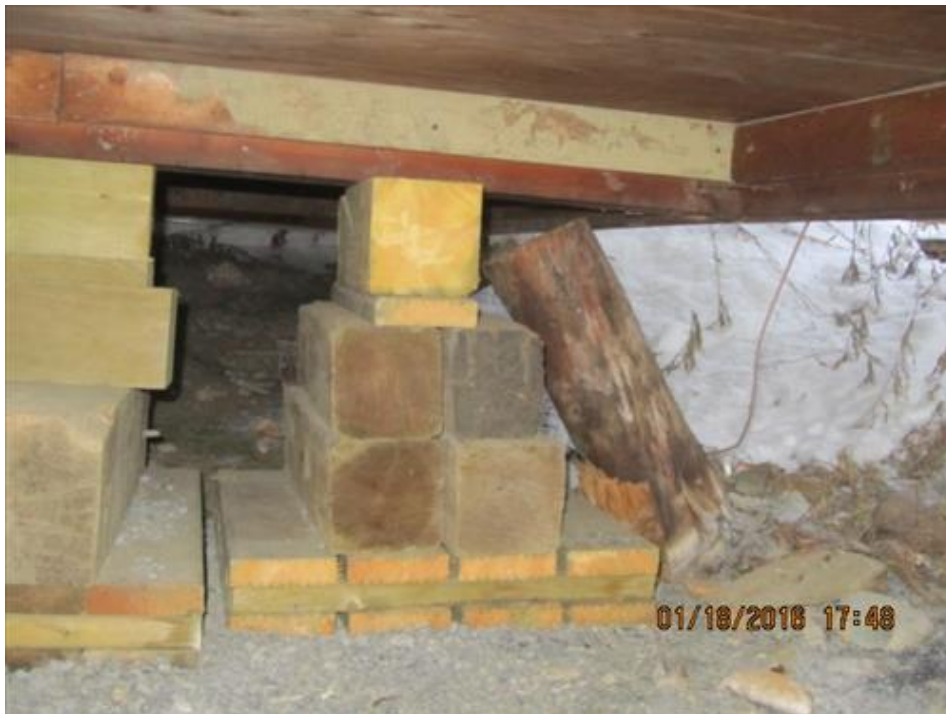
Photograph 18- Failed pile along the east edge of House #68 and constructed temporary support
