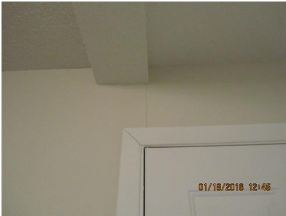
Photograph 68- Vertical crack within the east wall above the main entrance door and below the beam supporting the second floor-House #66
