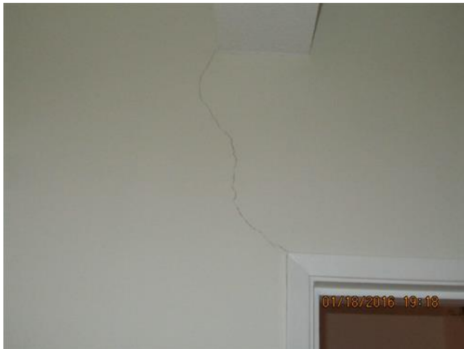
Photograph 96- Diagonal crack under the ceiling beam and above the door of utility room on second floor, on utility room side-House #68
