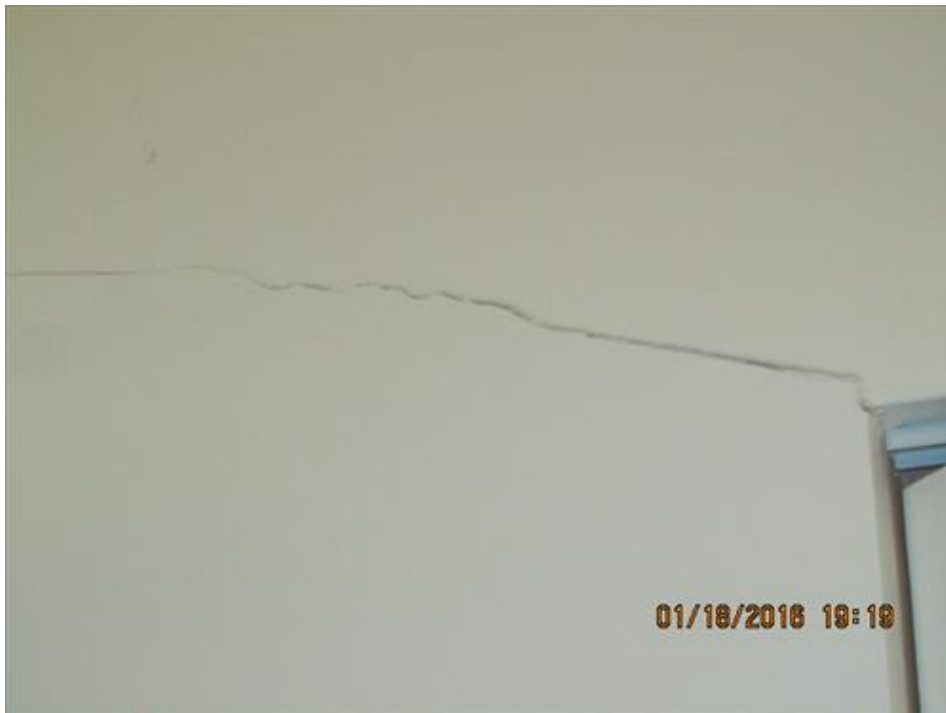
Photograph 100- Severe horizontal crack at the corner of closet door of the bedroom, located at the southwest corner of second floor-House # 68
