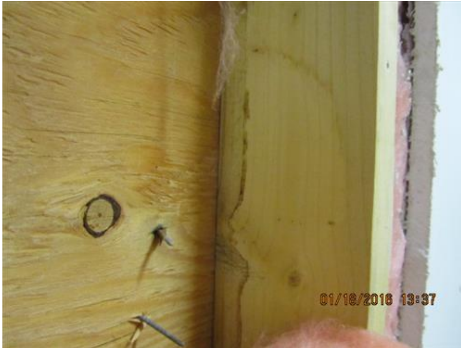
Photograph 35- Water stain at the intersection of the stud and exterior plywood sheathing, noted within the cut-out in the laundry room of house #66
