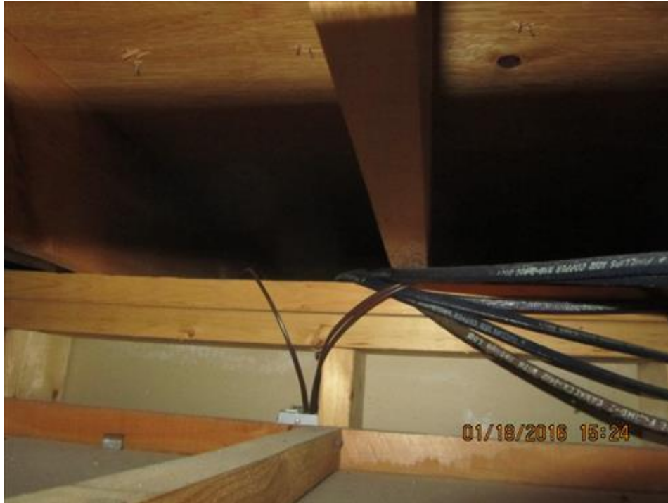
Photograph 29- Condition of second level floor joists and load bearing studs, viewed through the plumbing maintenance hatch within the ceiling of kitchen in House #66
