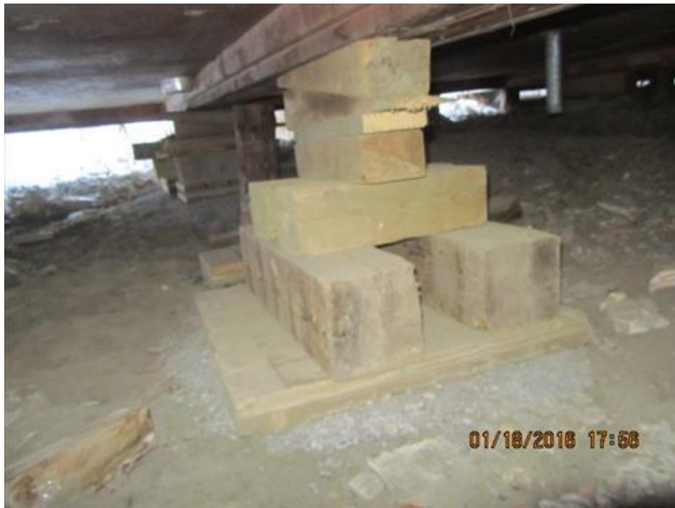
Photograph 20- Failed piles replaced with temporary blocking, placed on wood pallets, bearing onto prepared granular pad-Typical
