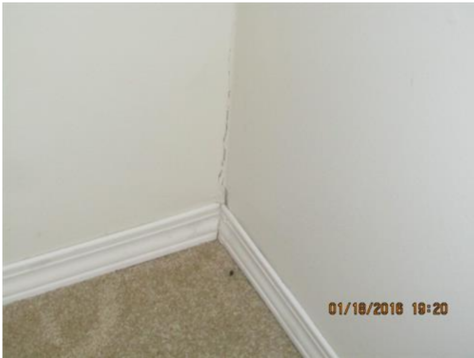
Photograph 102- Severe vertical crack at the south west corner of the located at the southwest corner of second floor-House # 68
