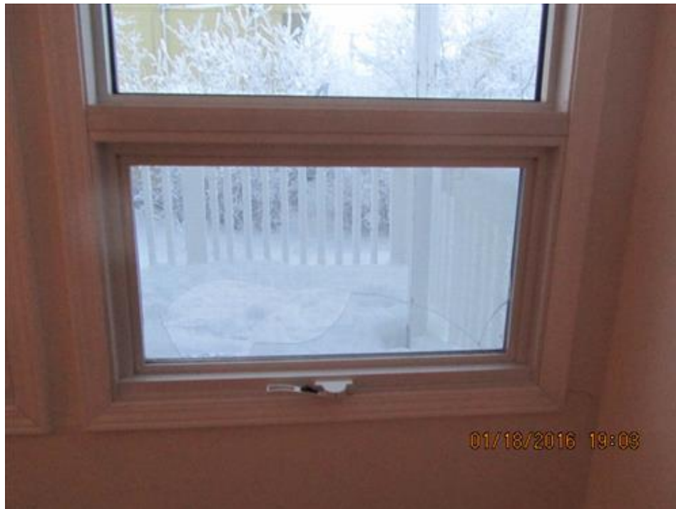
Photograph 50- Broken glass of the window located in sitting/living room of House #68
