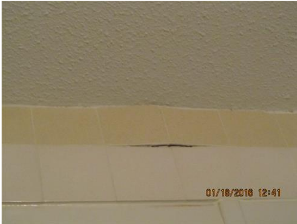
Photograph 77- Bulging of the loadbearing west interior wall, below the ceiling and above the door of the second floor north bedroom-House #66
