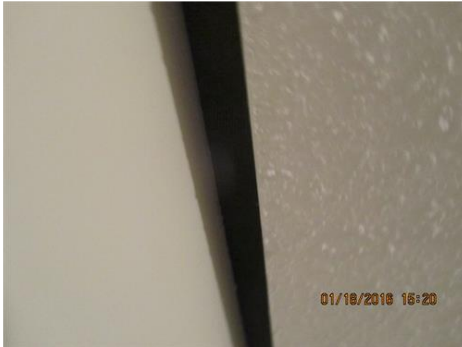
Photograph 105- Close-up of perimeter ventilation gap at the intersection of the wall and ceiling on second floor of House #66 (typical)
