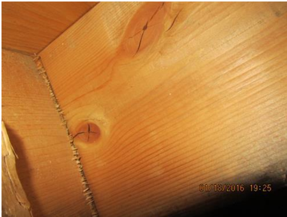
Photograph 34- Cracks and splitting in the second floor joist of House # 68
