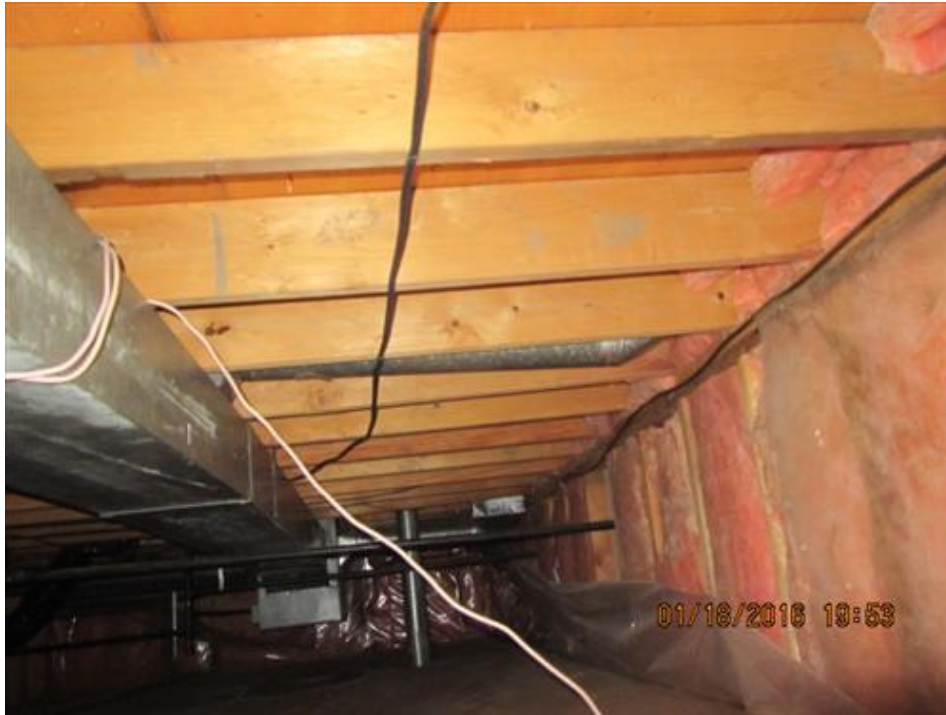
Photograph 7- Insulated perimeter studs within the raised enclosed crawl space under the building
