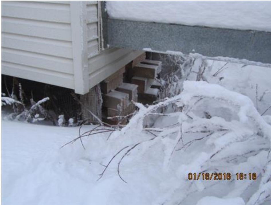
Photograph 19- Failed pile at the southwest corner of House #68, with temporary placed crib blocking support
