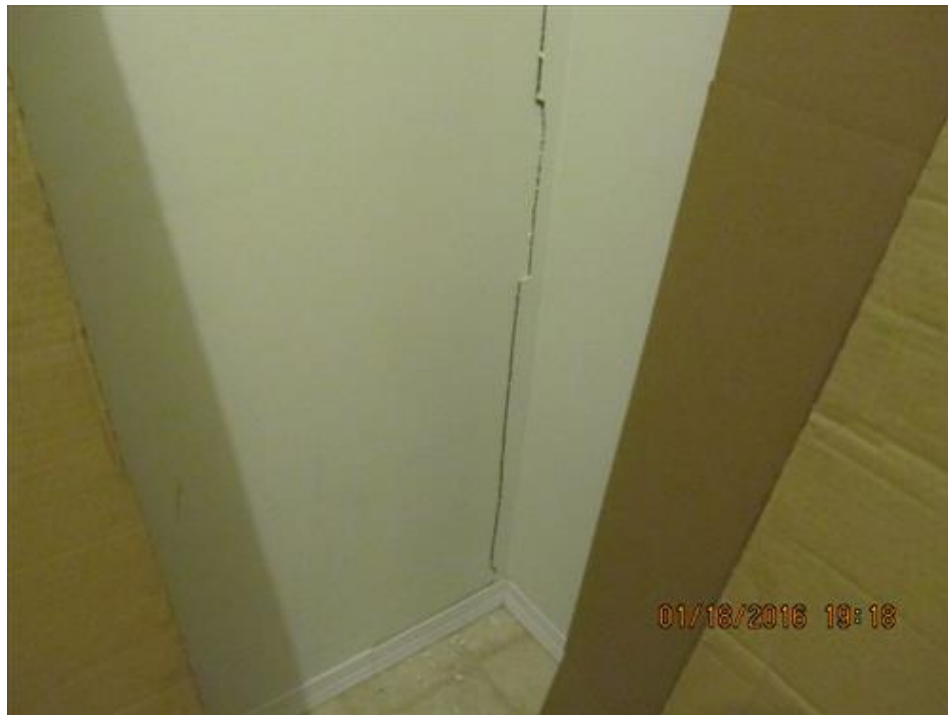
Photograph 98- Close-up of severe vertical crack at the northwest corner of utility room on second floor-House #68 (location of separation in party wall with House #66)
