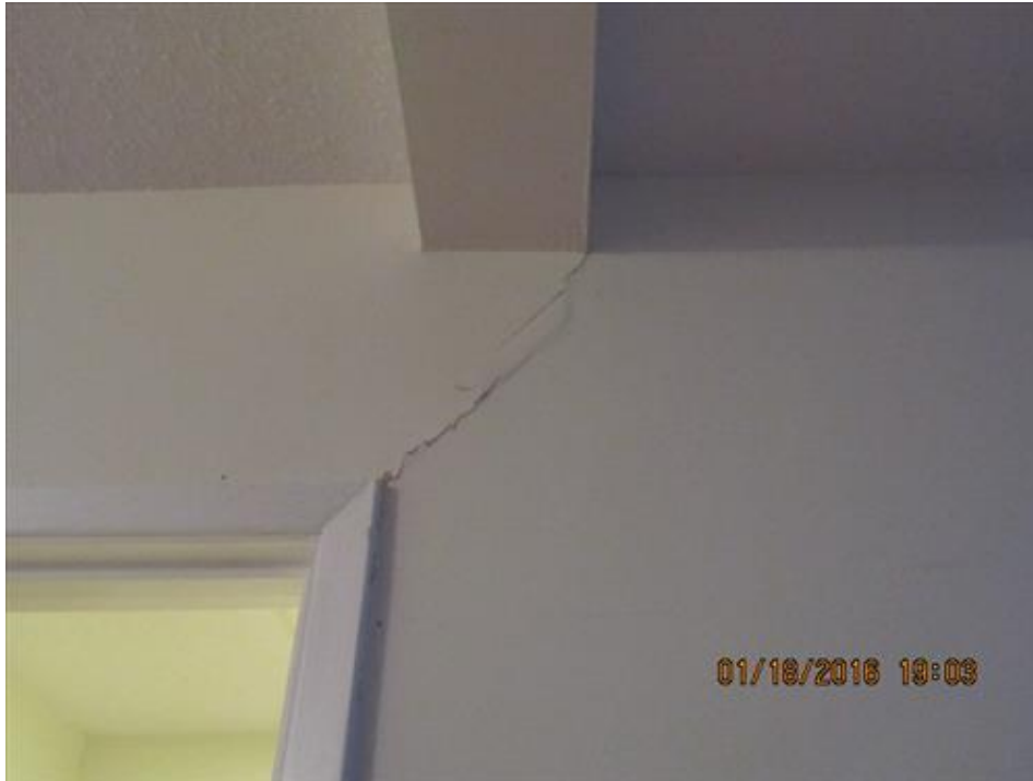
Photograph 79- Diagonal crack under the second floor beam and door opening from foyer to living/sitting room-House 68
