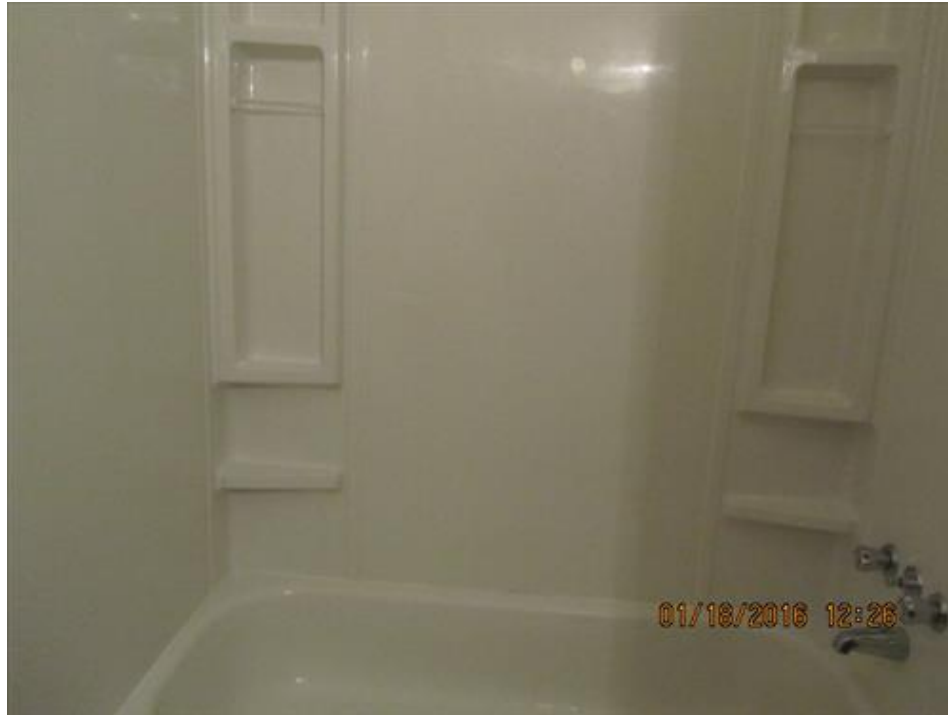
Photograph 57- Vinyl inserts around bathtub
