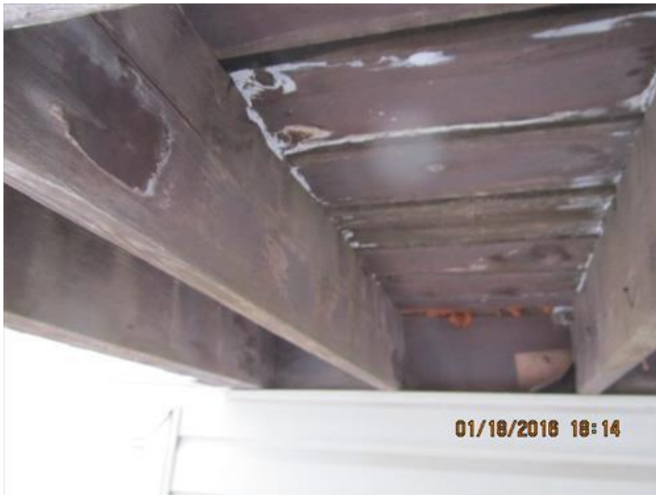
Photograph 44- Condition of beams and joist under the rear porch
