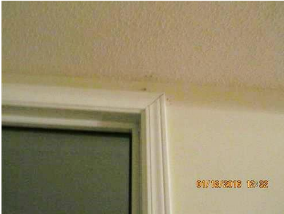
Photograph 71- Open window frame mold joint at the top right corner of window in sitting/living room-House #66
