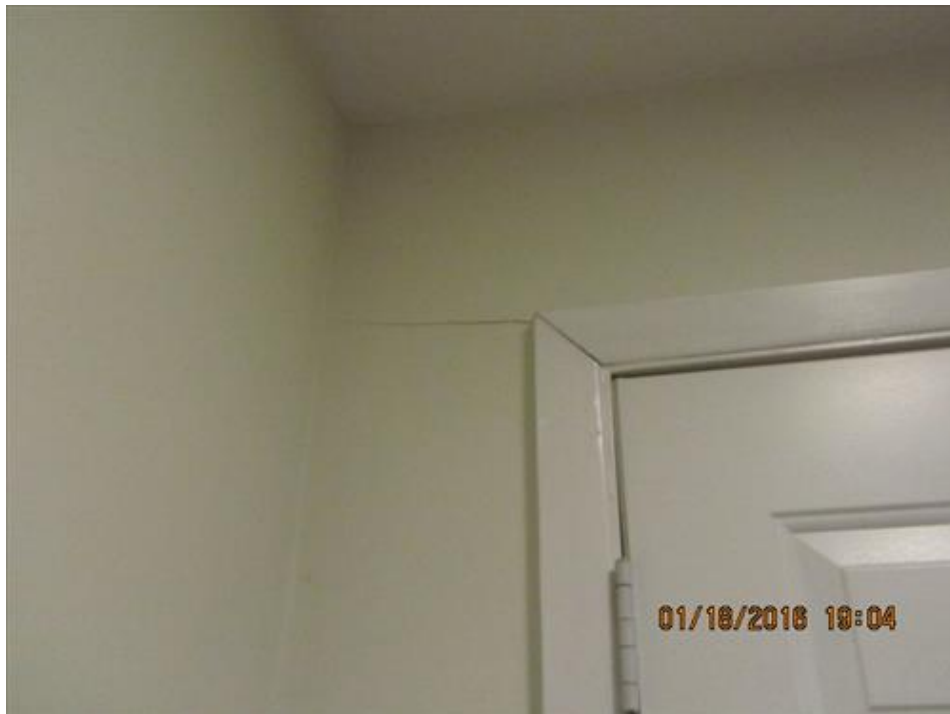
Photograph 80- Horizontal crack at the corner of the main entrance door to front foyer – House 68
