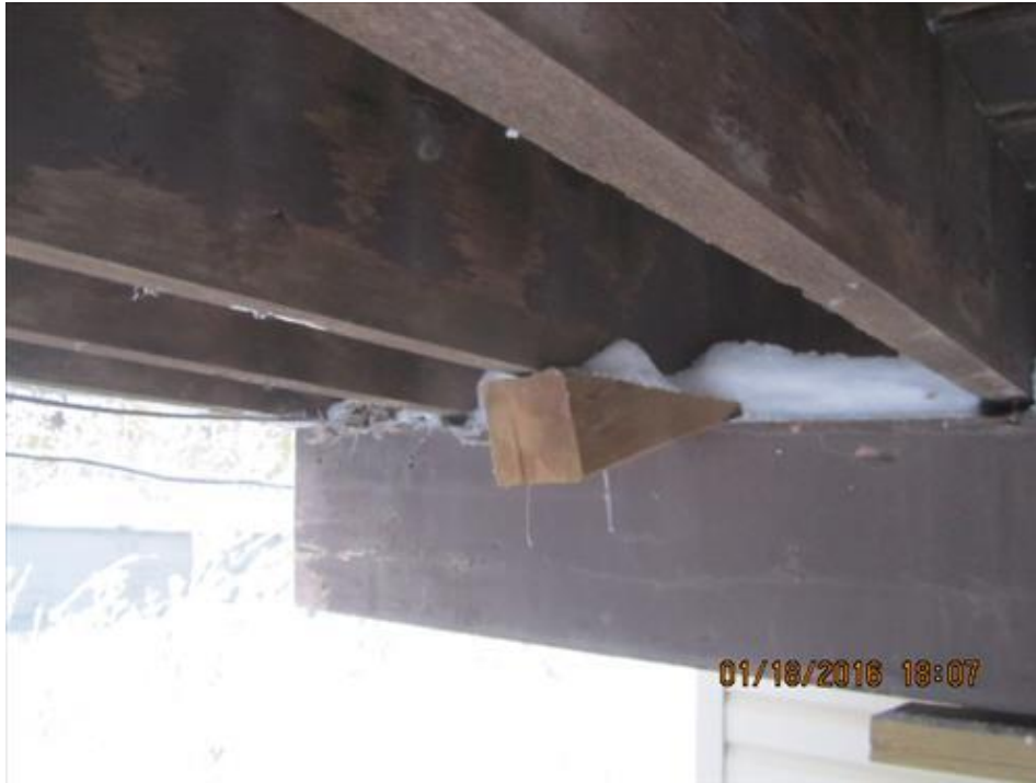
Photograph 43- Condition of joist supporting the front porch of House #68. Note the wedge placed due to the twist of the beam
