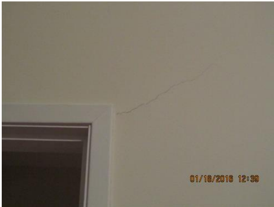
Photograph 66- Diagonal crack above the door of second floor north bedroom-House #66
