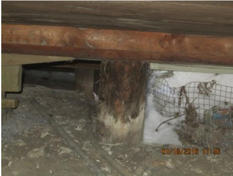
Photograph 23- Severe exposure to elements and heavy staining of the perimeter piles
