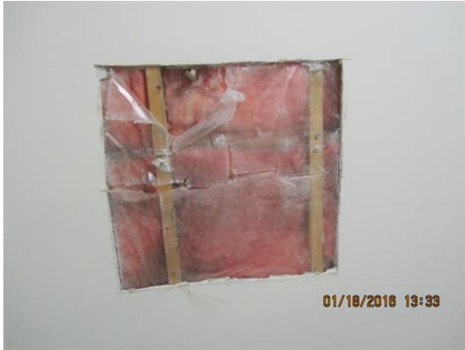
Photograph 47- Exterior wall components noted within the cut-out in ground floor laundry room
