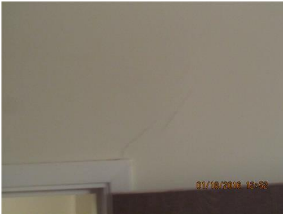
Photograph 70- Diagonal crack above the secondary door to outside within the west exterior wall
