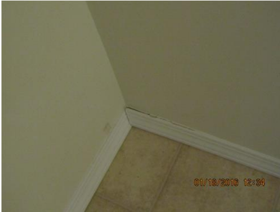
Photograph 75- Separation within the baseboard at the corner of the back foyer-House #66
