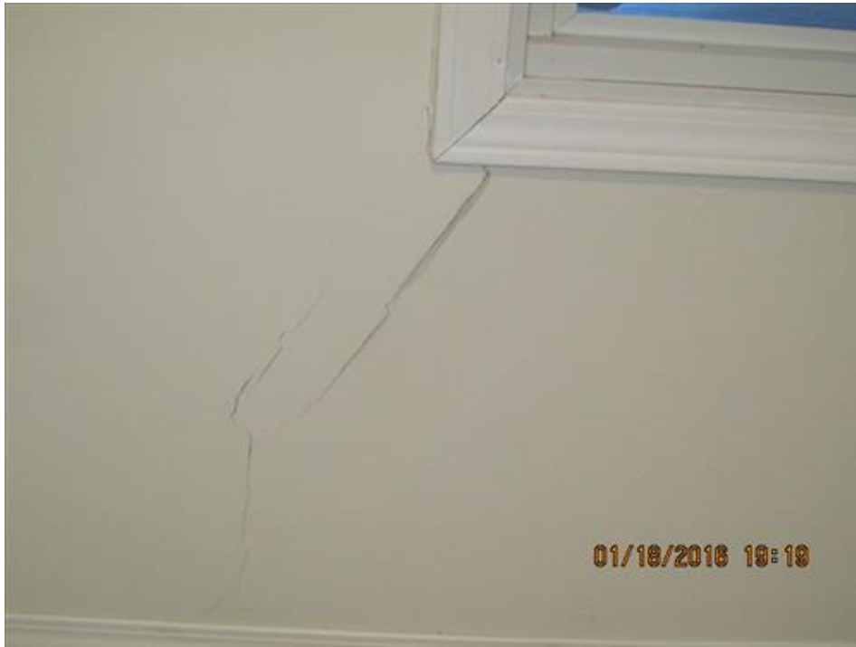
Photograph 101- Severe diagonal cracks at the lower left corner of the window, located at the southwest corner bedroom on second floor-House # 68
