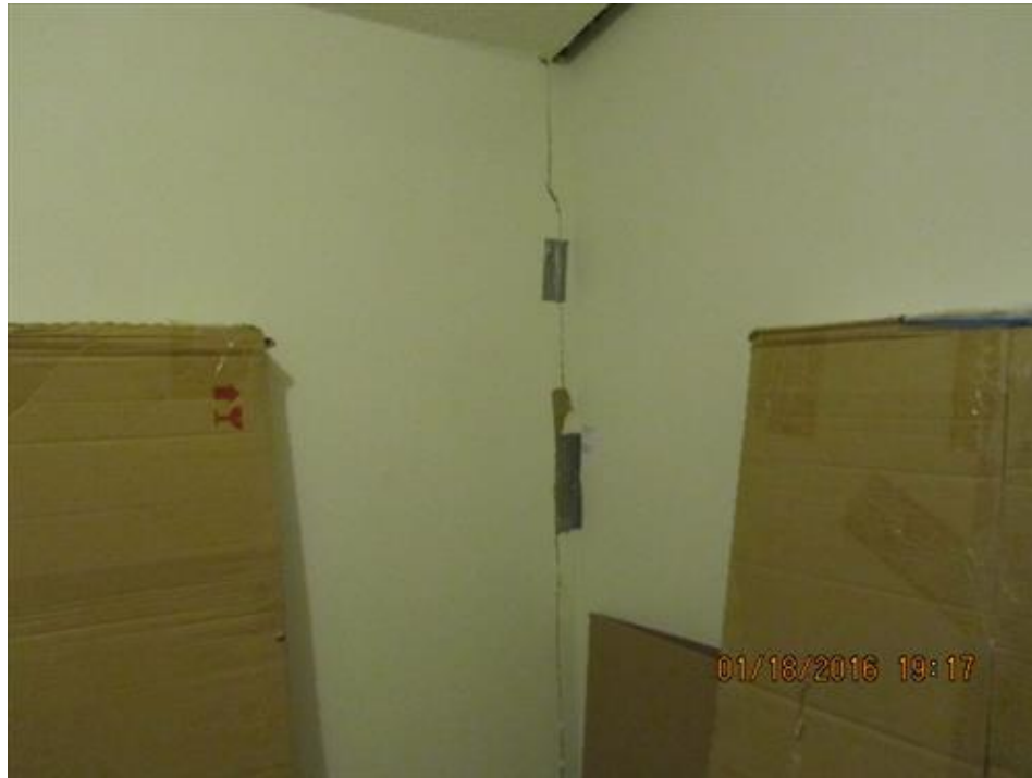
Photograph 97- Severe vertical crack at the northwest corner of utility room on second floor-House #68 (location of separation in party wall with House #66)
