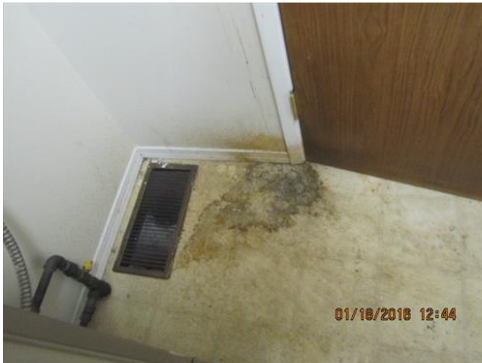
Photograph 78- Heavy stain within the furnace room floor, adjacent to the furnace-House #66
