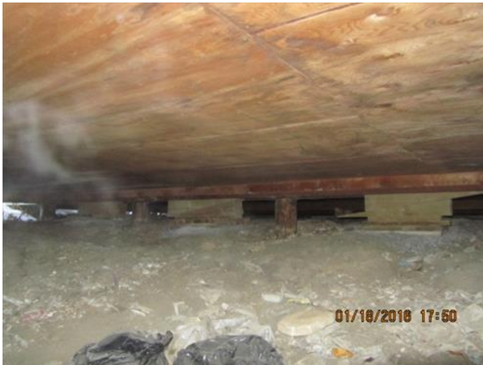
Photograph 4 -General view of shorter piles and ply wood cover under House #66, located on the north side
