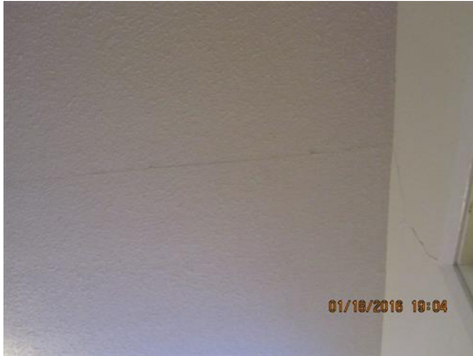
Photograph 81- Vertical crack above the door from front foyer and within the ceiling-House 68
