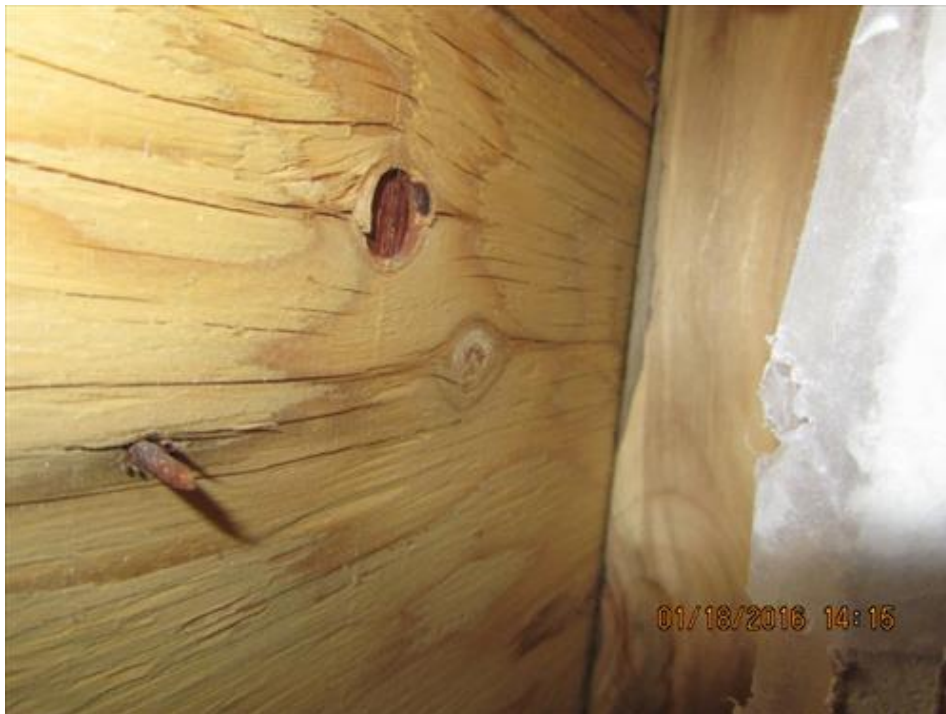
Photograph 36- Minor water stain and aging exterior plywood sheathing, noted within the cut-out in the second floor bedroom of house #66
