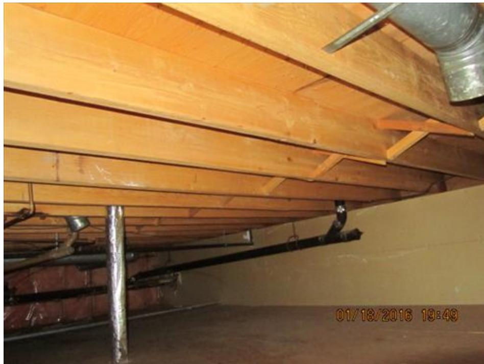
Photograph 10- Joists and cross bracing noted within the crawl space supporting the ground floor
