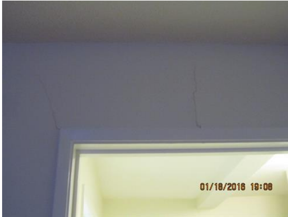
Photograph 87- Vertical and diagonal cracks above and at the corner of the door between the middle hall and back foyer-House #68
