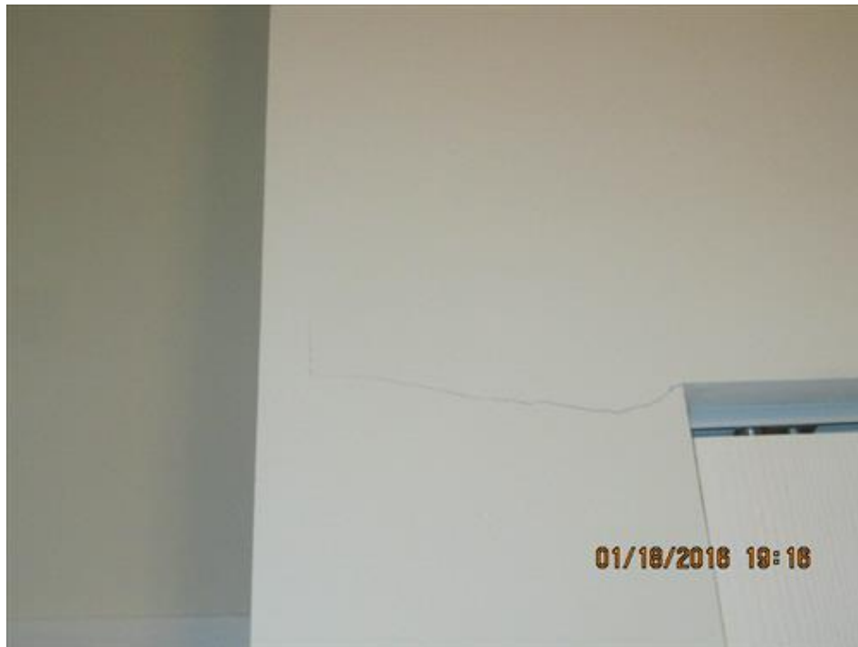
Photograph 94- Horizontal crack at the top left corner of the closet within the north bedroom on second floor-House #68
