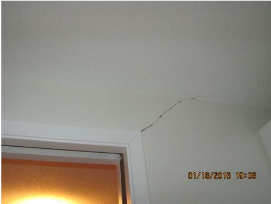
Photograph 85- Severe diagonal crack above the opening between the kitchen and dining room on kitchen side-House #68
