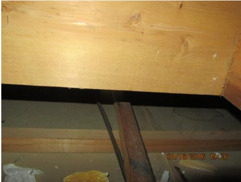
Photograph 33- Condition of second level floor joists, viewed through the plumbing maintenance hatch within the kitchen ceiling of House #68
