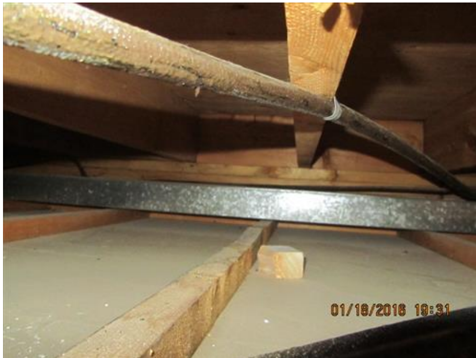
Photograph 32- Condition of second level floor joists and loadbearing studs, viewed through the plumbing maintenance hatch within the ceiling of kitchen in House #68
