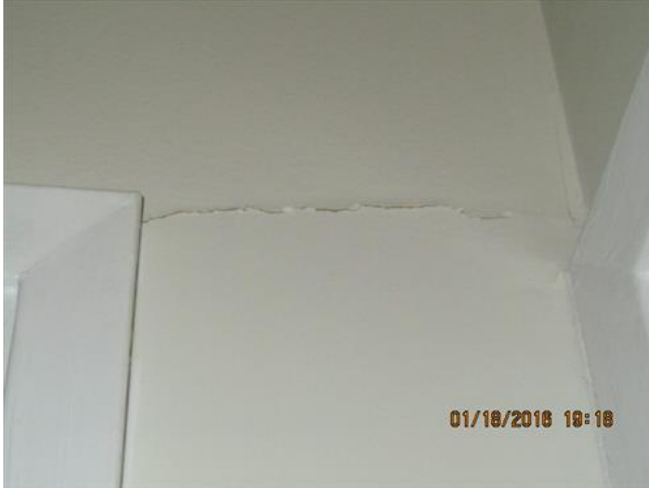
Photograph 99- Severe horizontal crack at the corner of the door of the bedroom, located at the southwest corner of second floor-House # 68
