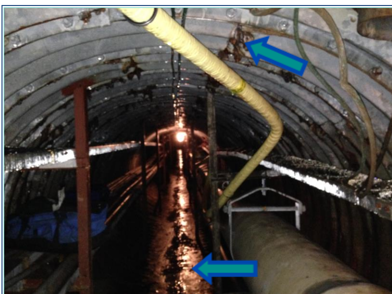
Photo 5: visible pooled water at the base of the tunnel during the May 2016 site visit, and precipitation along the tunnel walls are indicated by arrows in the photo above
