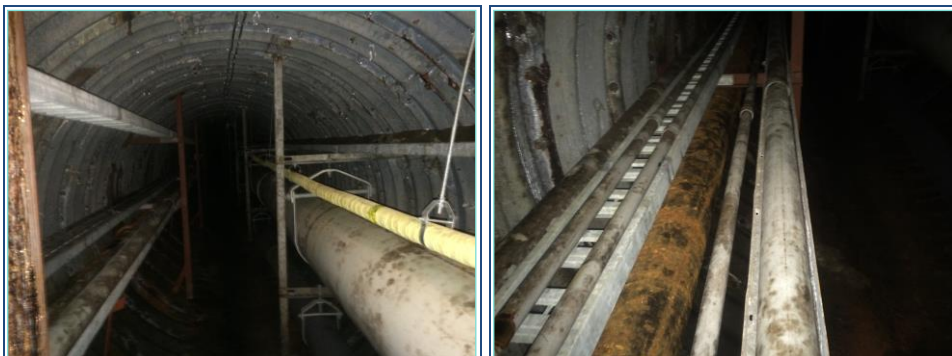
Photo 3 (left) and Photo 4 (right): staining observed along the pipes within the service tunnel as sampled in tape lift sample Tape4
