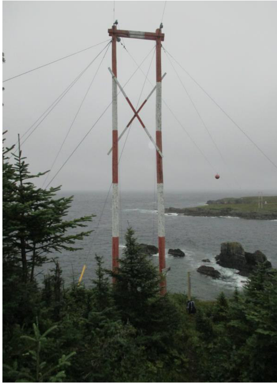
Photo A1: H Frame Structure (Catalina Side)
