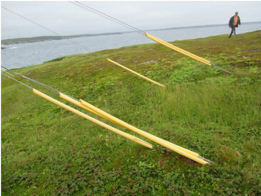
Photo A4: Typical Guy Anchors
