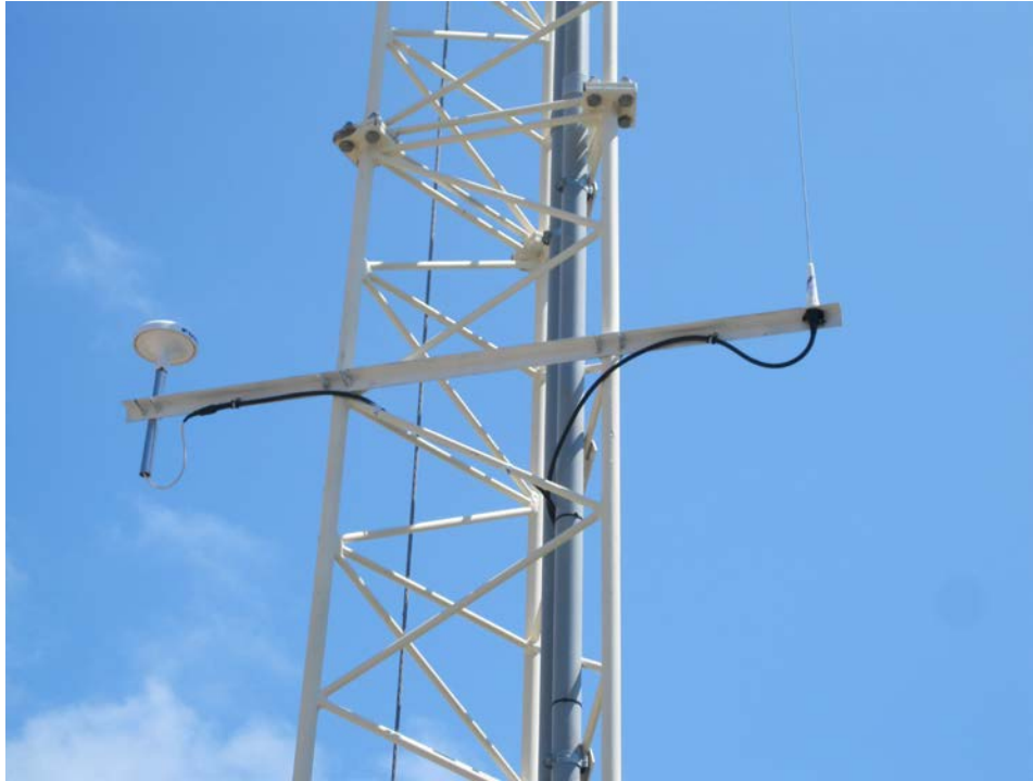
Figure 8: Example of Antenna Support Bar to be installed 9.15 m [30 ft] above ground level.
