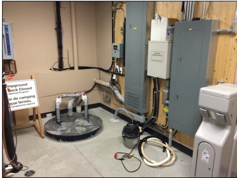
Photo 7 - View inside Maintenance Building Electrical Room looking northeast. Normal power distribution panel is to the left and emergency distribution panel is to the right. Automatic transfer switch is between both panels. New fuel system power to be obtained from normal panel. Fuel tank monitoring system to be mounted on wall adjacent to panels or at a location selected by the Site Supervisor.
