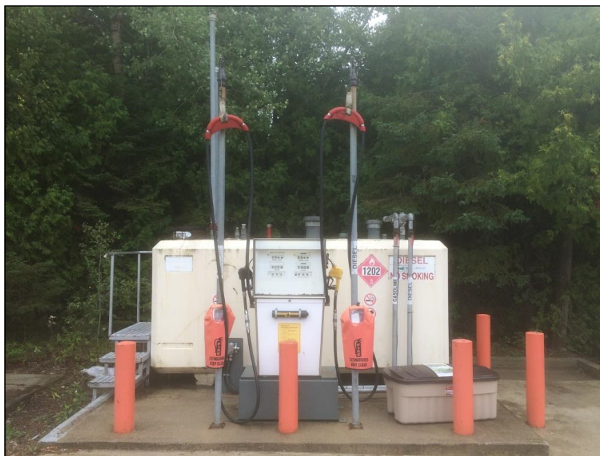
Photo 4 - View looking southwest at existing "Convault" split-product fuel tank, access stairs, pump, sump, high-hose retractor assemblies, and concrete tank pad/apron to be removed.
