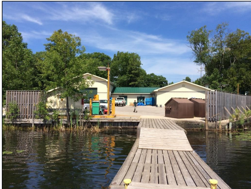
Photo 1 – View looking north from end of fuelling dock. Existing fuel pump island, bollards, fuel pump, hose reel, light standard and shed to left of dock to be removed. Maintenance Building in background. Existing “Convault” fuel tanks to be removed are located to the right of the waste bins behind the wood fence.
