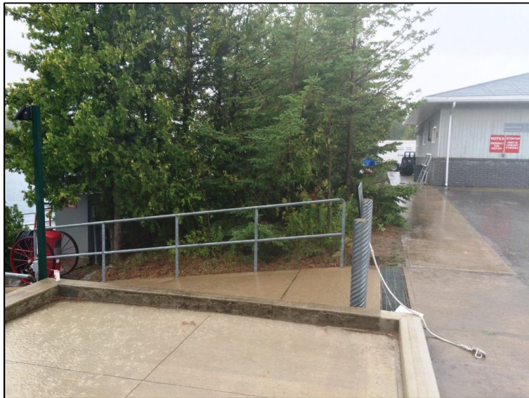
Photo 6 – View from existing product transfer area dike looking southwest towards Maintenance Building. Existing fuel pump E-Stop and sign visible on building outer wall. Electrical room is located opposite the E-Stop. Power for new fuel system to be obtained from existing distribution panel in electrical room.
