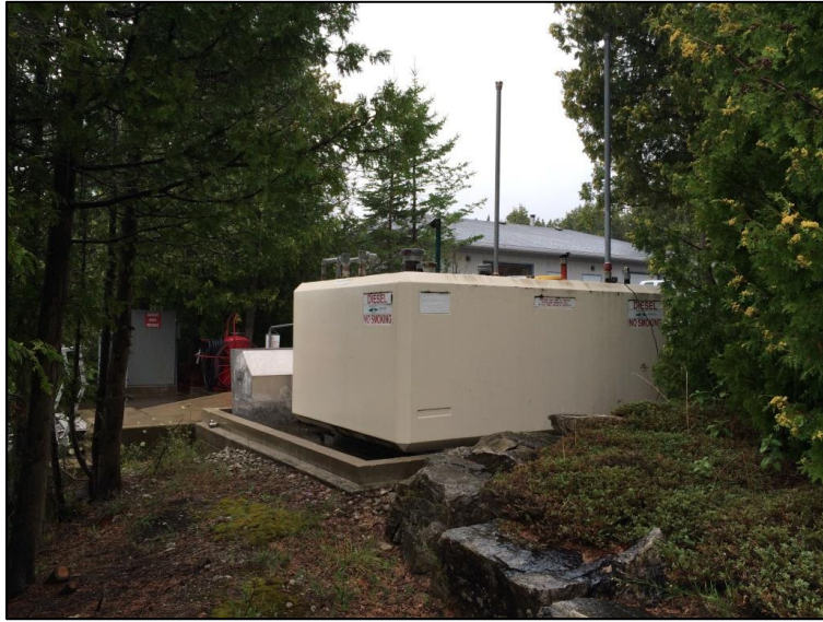
Photo 5 – View looking west at existing aboveground fuel tank system to be removed. Electrical distribution panel for watercraft battery system recharging is located inside grey electrical box to left of fuel tank. Maintenance Building visible in background behind fuel tank.
