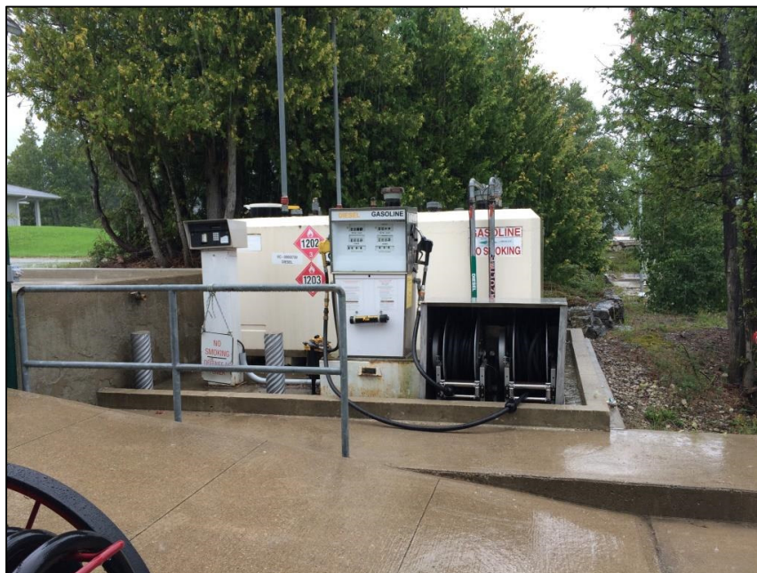
Photo 4 - View looking northeast at existing "Convault" split-product fuel tank, pump, sump, hose reel assembly and cardlock pedestal to be removed. Concrete tank dike and all other concrete visible in the photo to remain.
