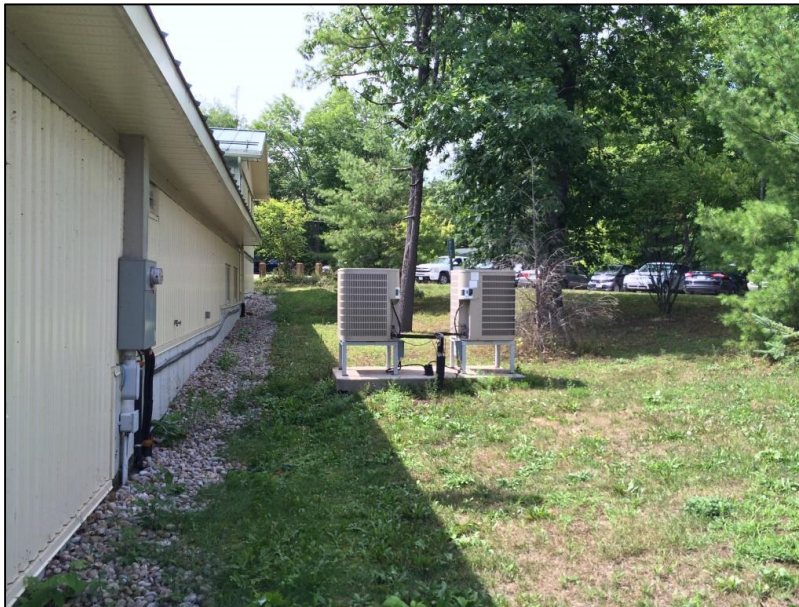
Photo 6 – View looking west at the rear of the Maintenance Building (north building wall) showing location of hydro meter. Building electrical room is located opposite the hydro meter.
