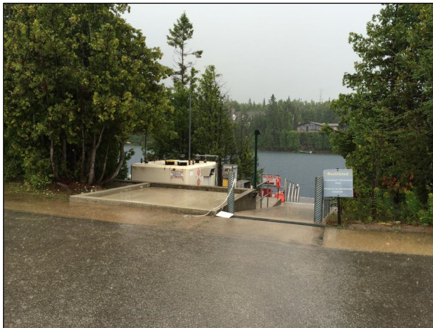
Photo 2 - View looking southeast at existing aboveground fuel tank system to be removed. Existing concrete product transfer area dike in foreground to remain.
