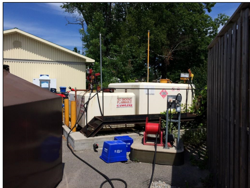
Photo 4 – View looking northwest at existing “Convault” fuel tanks and steel platform to be removed. Underlying concrete tank dike and bollards to remain. Concrete hose reel island and hose reel assembly in foreground to be removed.
