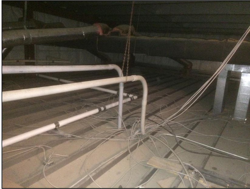
Photo 7 - View inside Maintenance Building above suspended ceiling looking southwest. The two electrical conduits shown in the photo are connected to the distribution panel shown in Photo 6.
