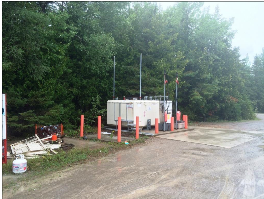
Photo 3 - View looking west at existing aboveground fuel tank system to be removed and concrete fuelling apron/tank pad and bollards to be removed. Concrete island and bollards in the foreground (to the left of the tank in the photo) are to be removed.
