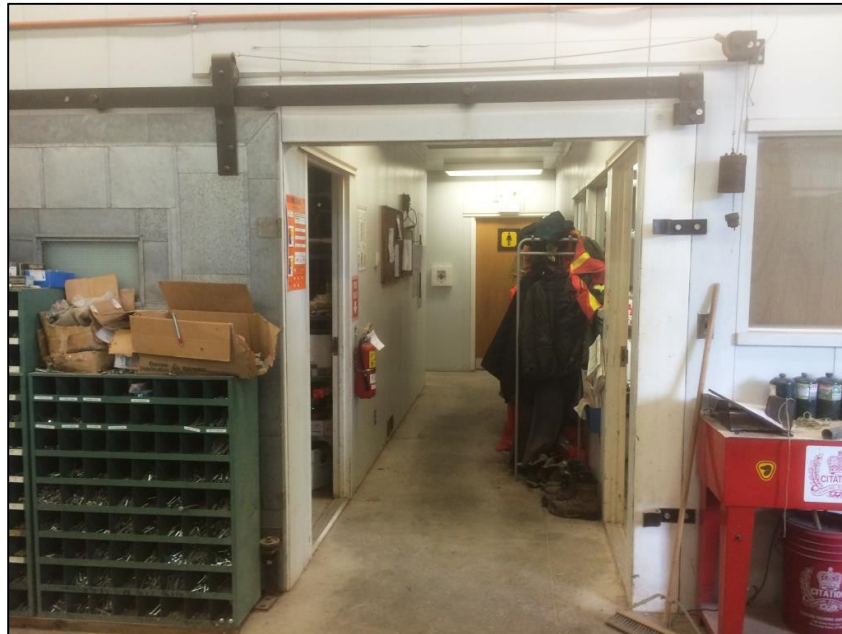
Photo 6 - View inside Maintenance Building looking southeast. Electrical distribution panel from which new fuel system power will be obtained is located on the left-side of the hallway (recessed into wall) just beyond the bulletin board. Existing tank overflow alarm to be removed is mounted on hallway wall just above bulletin board.
