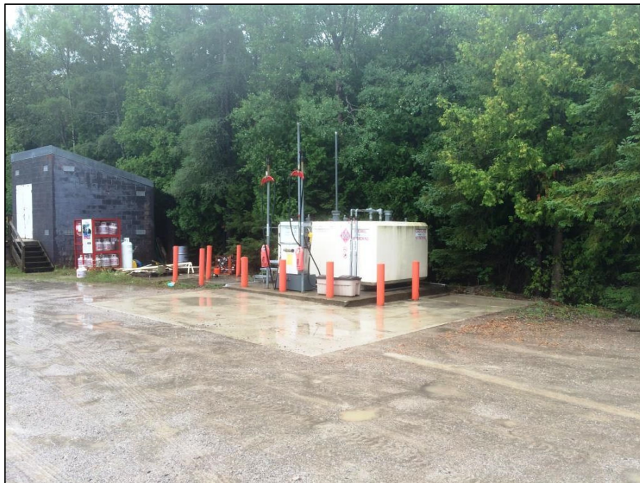
Photo 2 - View looking south at existing aboveground fuel tank system to be removed and concrete fuelling apron/tank pad and bollards to be removed.
