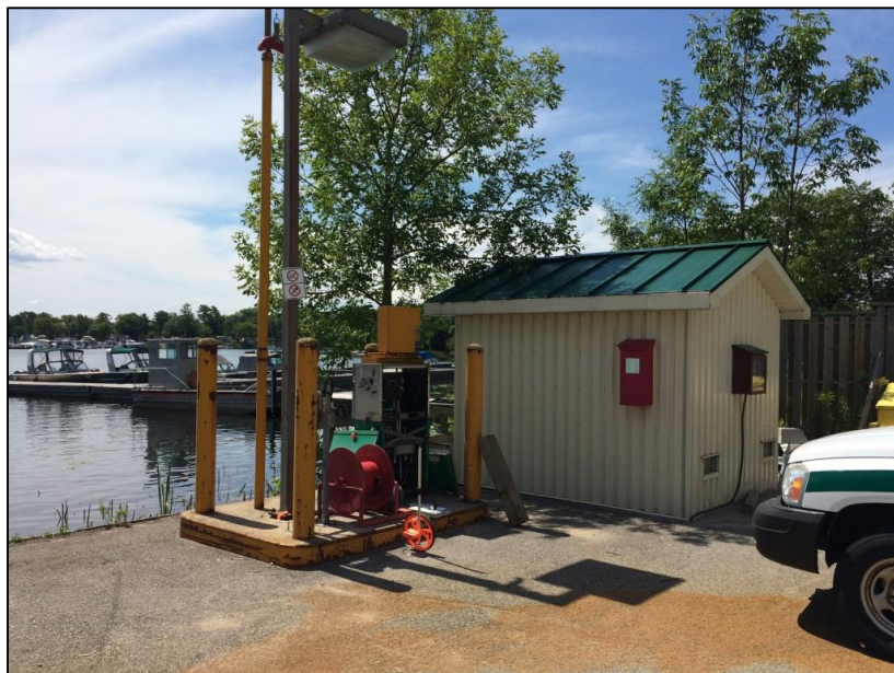
Photo 2 – View looking southwest at existing fuel pump island, bollards, fuel pump, hose reel, light standard and shed to left of dock to be removed.
