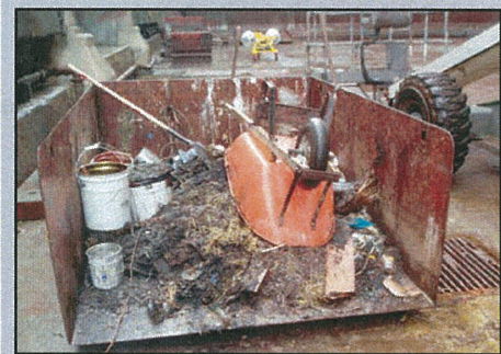
INADEQUATE waste grit storage.
