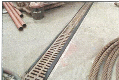
Prevent deleterious substances entering marine environment by placing filter cloth in the trench drains.
