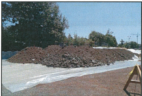
INADEQUATE stockpile of contaminated soil. Soil should be covered to prevent exposure to elements, runoff and people.
