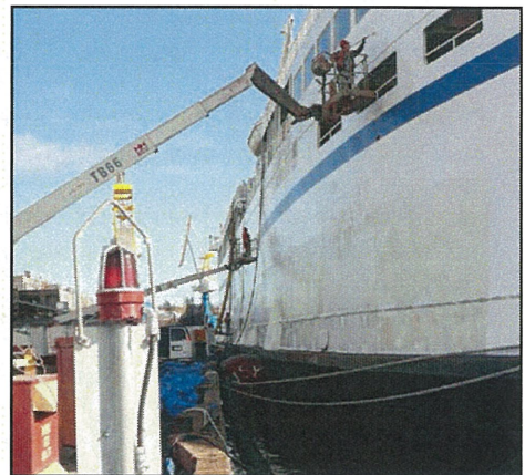
While painting vessels docked alongside the wharves or jetties, do not spray paint. Take sufficient measures to prevent paint from entering the marine environment.
