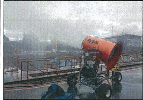
Dust suppression unit in operation.
