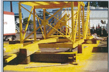
INADEQUATE containment. Ensure tarps are in place to prevent overspray impacting the surrounding work area.
