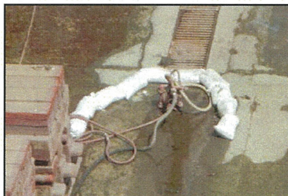
Sand bags used on dock bottom to divert and filter excess water.
