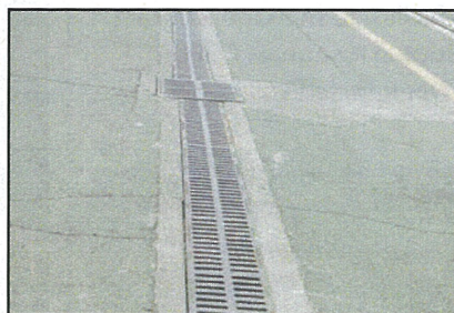
UNAUTHORIZED Sanitary Sewer Discharge point (i.e. trench drains).
