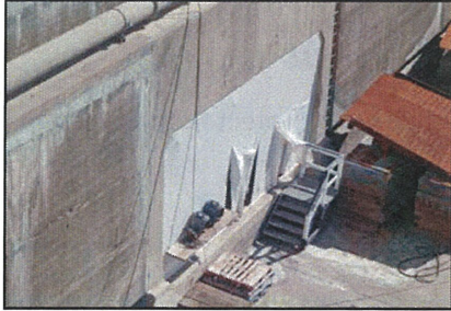
ADEQUATE containment on stabilizer pocket doors.
