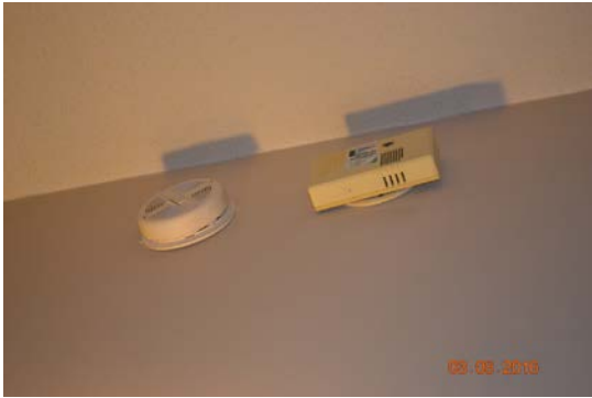
V008 – CO/Smoke detector.
