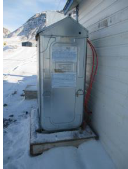
Photo 4: Outdoor tank and piping
