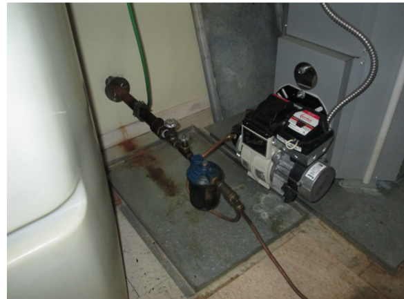
Photo 4: Interior piping and accessories
