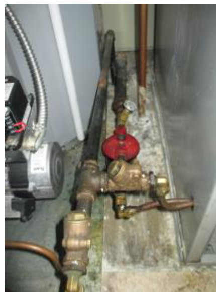
Photo 4: Interior piping and accessories
