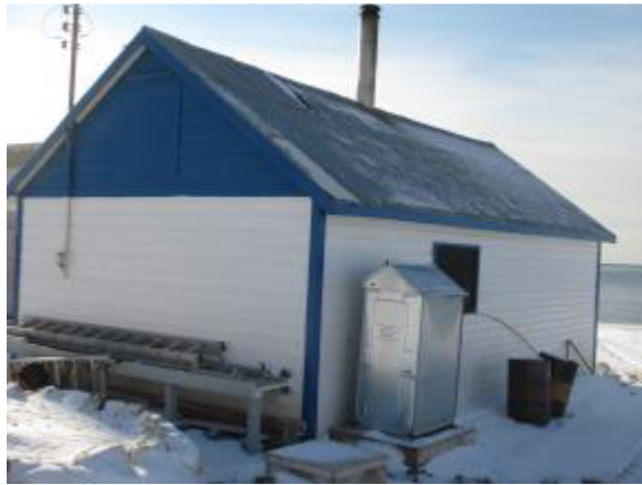
Photo 1: Outdoor above ground fuel tank
