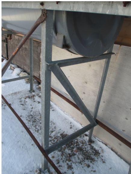
Photo 1: Outdoor above ground fuel tank and stand
