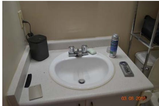
G007 – replace taps. Hand sink & bathtub
