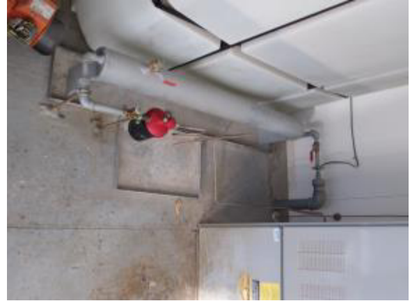
Photo 2: Indoor piping and accessories
