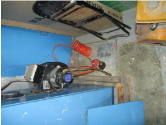
Photo 3: Burner and piping
