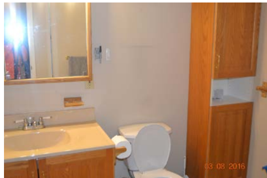
V008 – bathroom, replace taps – hand sink and bath-tub faucets.
