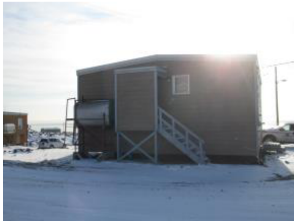
Photo 1: Outdoor above ground fuel tank and stand
