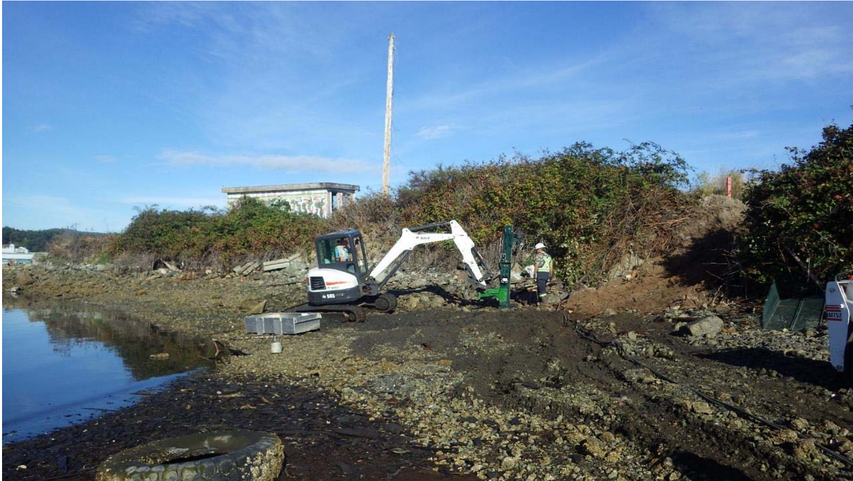
Photograph 3: Looking west at the excavator-mounted auger rig set up on the foreshore area.
