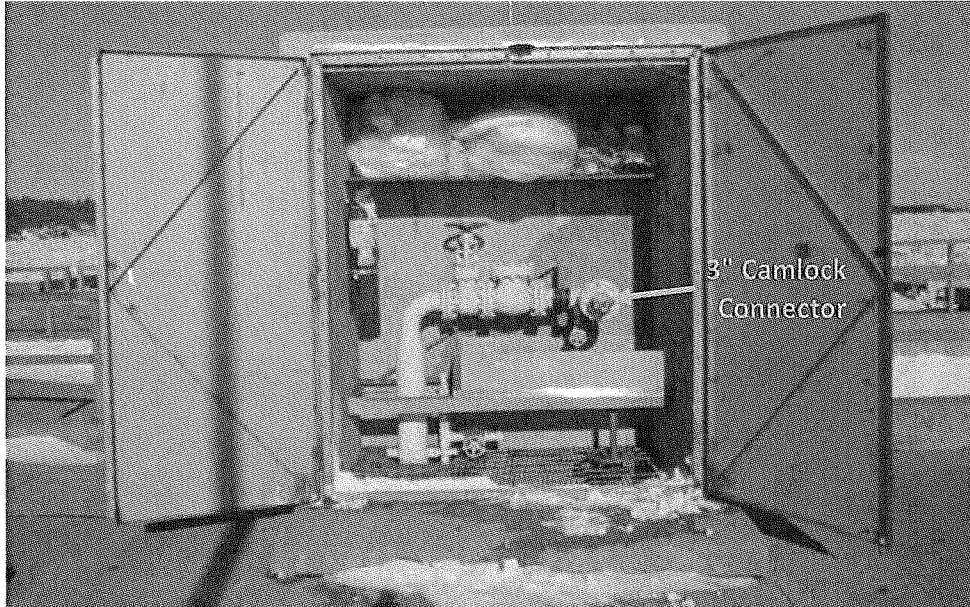
Diesel refuelling station at the wharf
