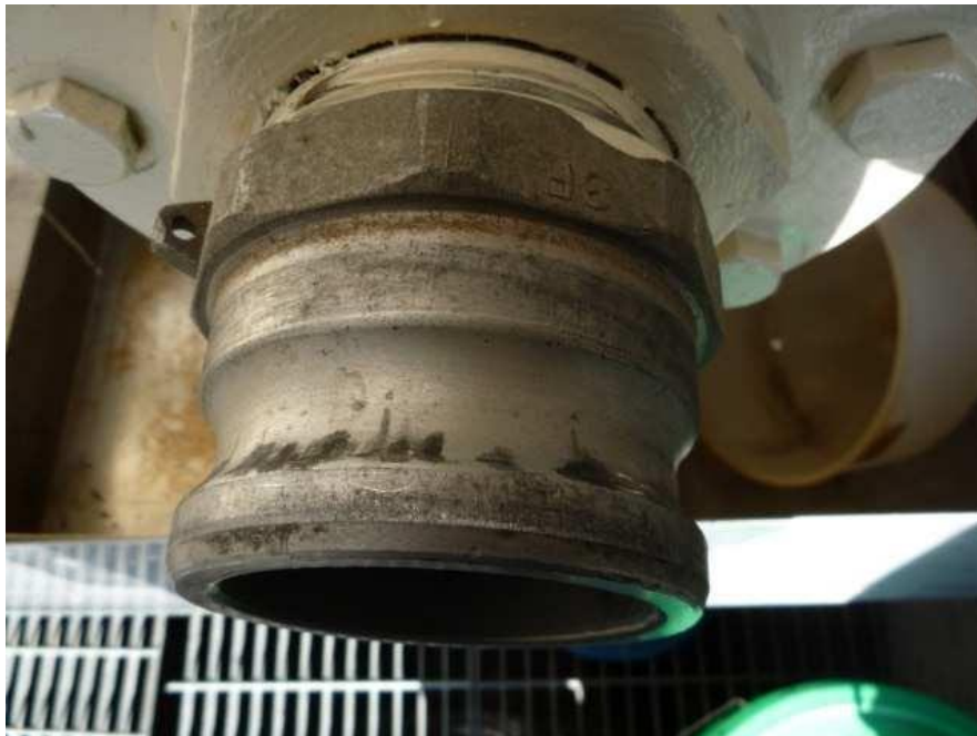
3" Camlock connector at the wharf refuelling station
