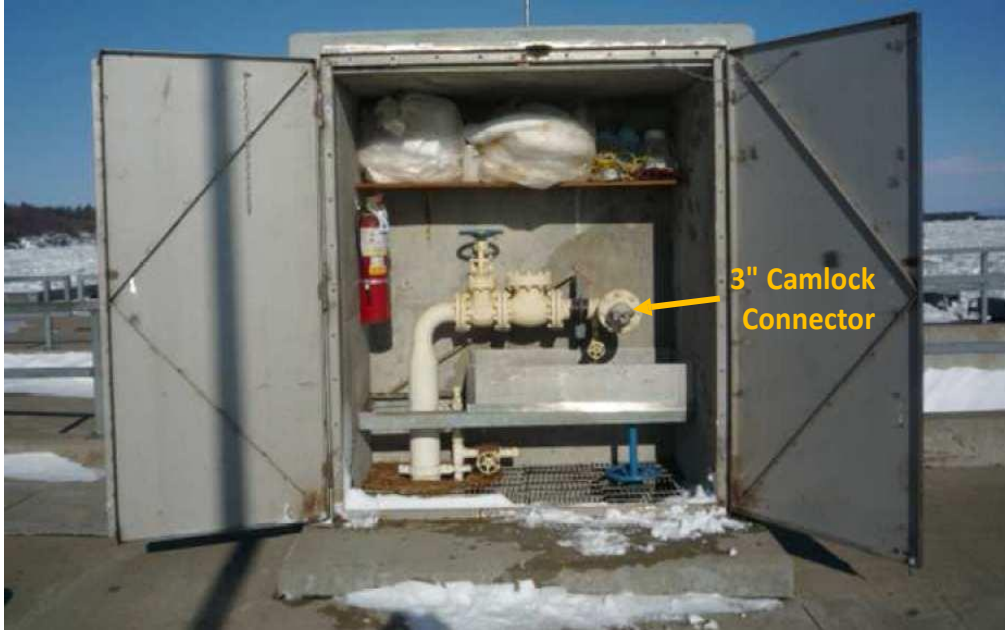
Diesel refuelling station at the wharf
