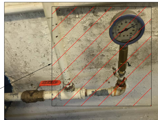
PILOT SYSTEM SUPPLY
