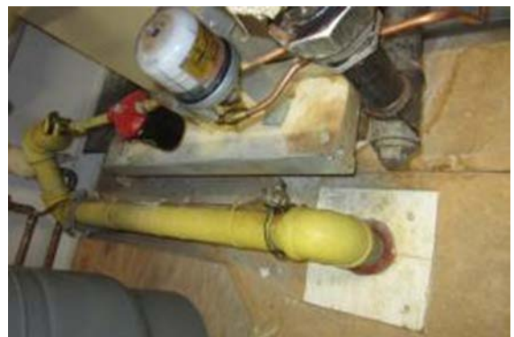
Photo 8: Fuel Main and Filter
