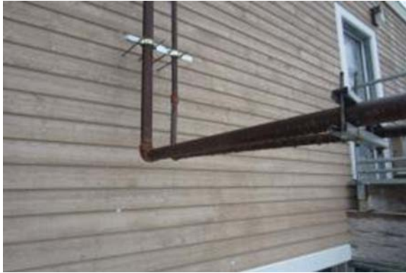
Photo 3: Exterior Piping along Wall
