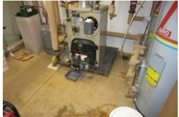
Photo 6: Boiler in Mechanical Room
