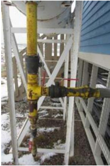
Photo 3: Exterior Piping and Valves
