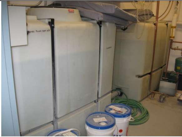
Water tanks at detachment ( 2 x 325 gal)
