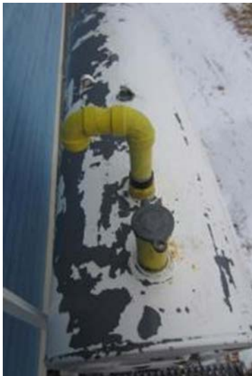
Photo 5: Fill and Vent Terminations
