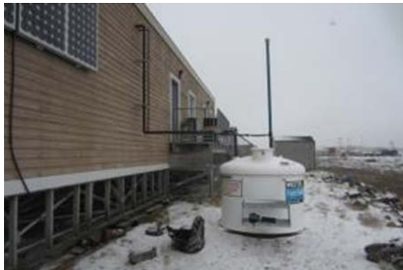
Photo 1: Outdoor above ground fuel tank
