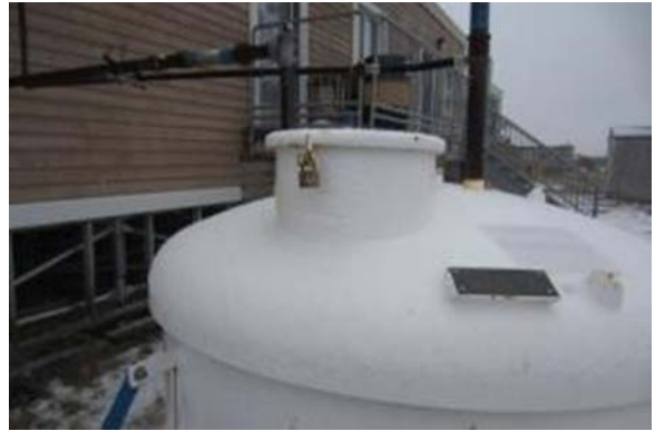
Photo 4: Supply and Return Lines at Exterior Tank
