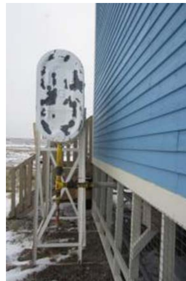
Photo 2: Outdoor above ground fuel tank
