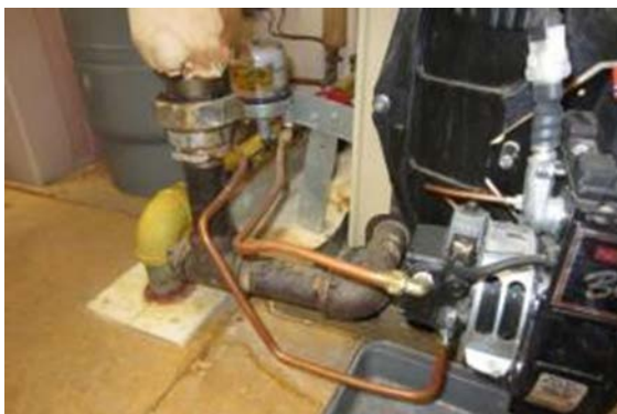
Photo 7: Fuel Piping At Boiler
