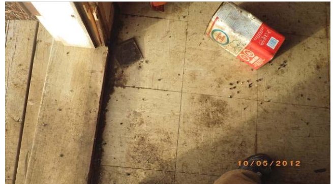
Photo 28. Close up view of dead flies, general debris and floor linoleum (Sample TK-ACM-3).
