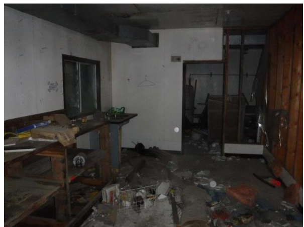
Photo 24: View of miscellaneous debris in lab and storage building.
