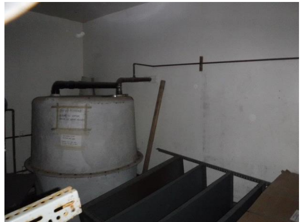
Photo 22: View of lines running from miscellaneous tanks in NW room/utility room.
