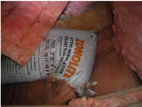
Photo 17: Bag of vermiculite observed in attic (2016).
