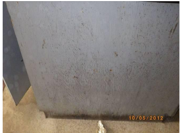
Photo 10: Close up view of mould on cabinets inside lab and storage building.
