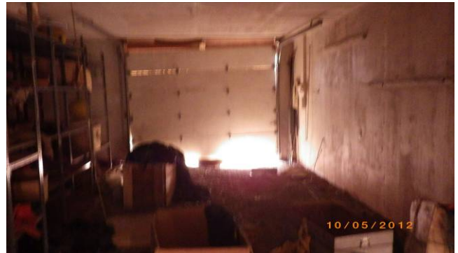
Photo 24. Interior view of garage portion of the subject building, east side of building.
