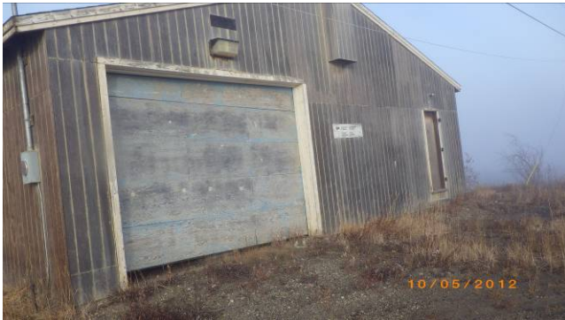
Photo 33. Looking west at on-site building and location of samples TK-LP-1 (garage door) and TK-TH8 (soil).
