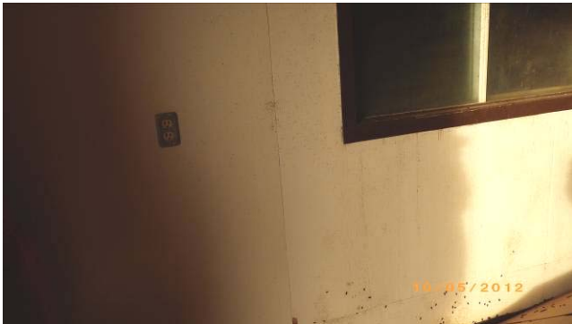
Photo 29. Close up view of mould on the wall inside the subject building.
