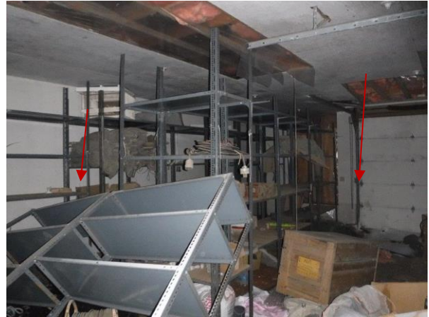
Photo 14: View of shelving units knocked over in garage area (2016).
