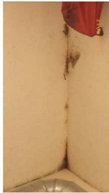
Photo 21. View of mould on wall inside subject building.
