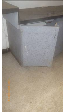
Photo 25. View of floor linoleum inside subject building (Sample TK-ACM-3) and mould on cabinets.
