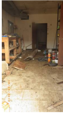
Photo 19. Interior view of the subject building, looking north. View of floor linoleum (Sample TK-ACM-1) and lagging (Sample TK-ACM-2).
