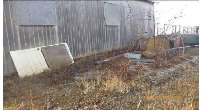
Photo 32. Looking at the south side of the subject building, including debris.
