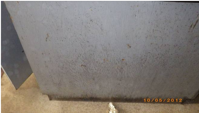
Photo 27. Close up view of mould on cabinets inside subject building (laboratory area).
