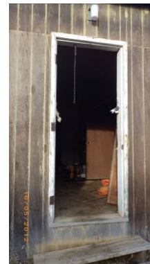
Photo 12. Close up view of missing door on the north side of the building.
