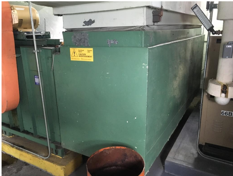
Photo 1: Grey cement compound was observed on AHUs and ducting, including in solid-board form (pictured).
