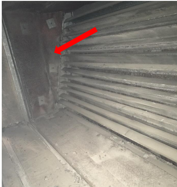
Photo 5: Maroon-coloured burlap covering over asbestos-containing grey parging, inside ducting associated with AHU in Room 257. The ducting traverses down to connect to air diffusers in DST Rooms 49 and 50.
