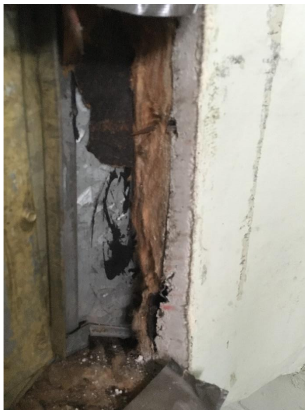
Photo 2: Black mastic, applied to the AHUs and associated ducting to adhere the grey cement compound outer insulation contains 11.22% Chrysotile asbestos.
