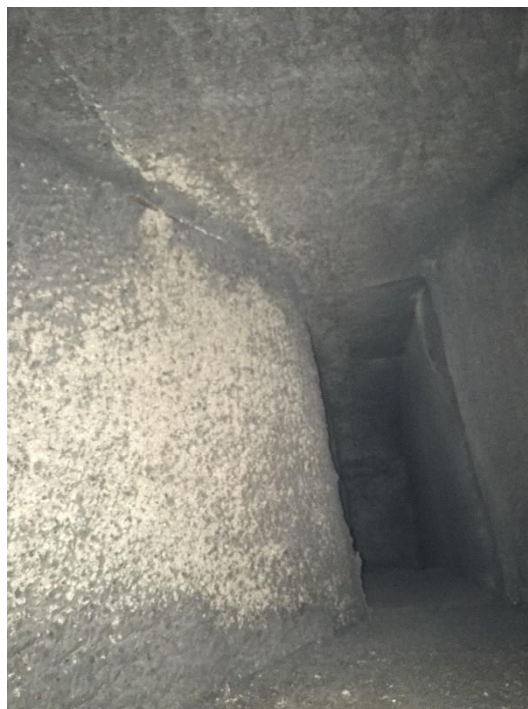
Photo 6: Suspected mould-impacted tar-paper (non-asbestos) over fibreglass acoustic panels, inside ductwork associated with AHU03 in the Penthouse.
