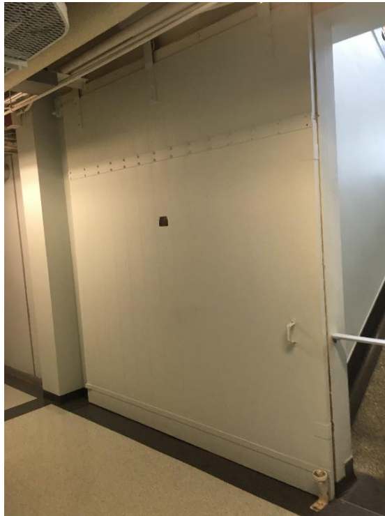
Photo 3: The internal, concealed lining of the fire door (suspect ACM), that separates the 1 st floor stairwell to 2 nd floor lobby.
