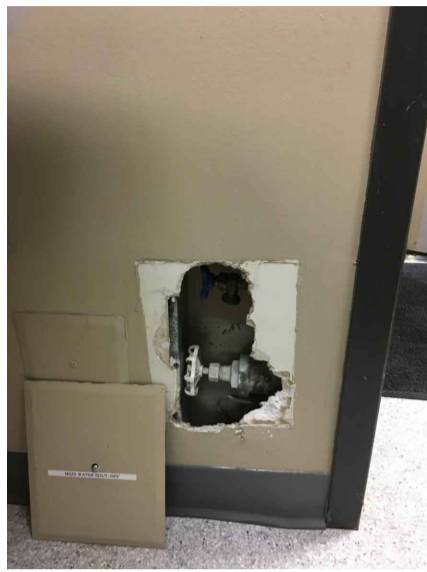
1A M102 INCOMING WATER LINE
