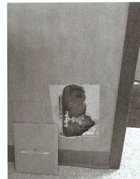
1A M102 INCOMING WATER LINE
