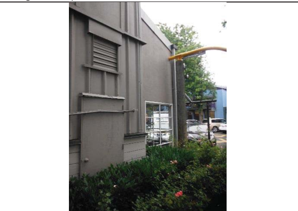
Photo 6: Sample B3-S15 of caulking material present at the exterior wall (northeast portion) was found to be asbestos containing.
