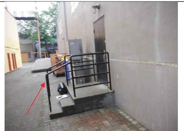
Photo 4: View of west portion of the building. Sample B3-L5 of black on yellow paint present at the steel railings. The paint contains more than 0.06% lead.
