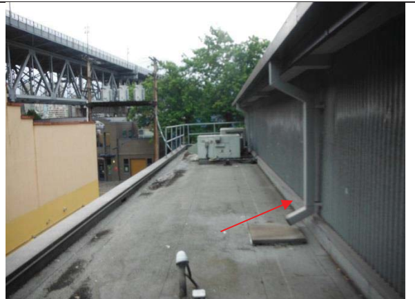
Photo 2: View of the theatre roof (west side). The caulking material present at the walls is found to be asbestos containing (0.25% Chrysotile).
