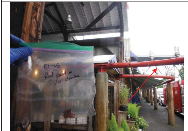
Photo 5: View of the red paint applied on the steel structure present at the exteriors. The paint sample is found to contain greater than 0.06% lead.
