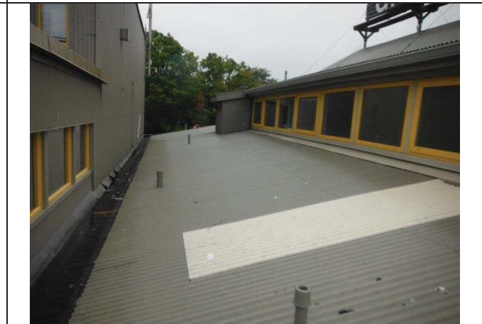
Photo 4: View of lead containing the wash room exhaust boots, present at the roof of the building.
