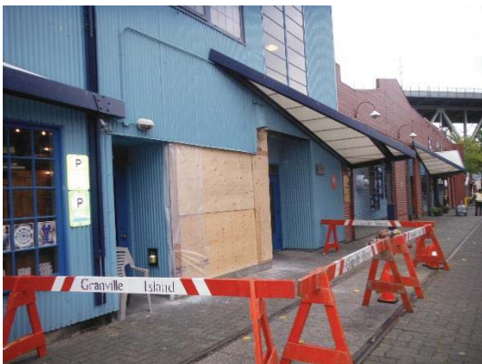
Photo 5: View of the south portion of the building that was damaged in the vehicle accident.
