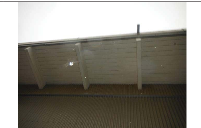
Photo 6: View of the white paint applied on the ceiling of the building structure. The paint sample is found to contain greater than 0.06% lead.
