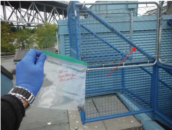
Photo 3: View of paint sample location B2-L2 of dark blue paint sample applied on the steel structure. The paint is found to contain more than 0.06% of lead.
