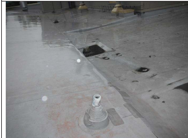
Photo 3: View of lead containing the washroom exhaust boot, present at the roof of the building.
