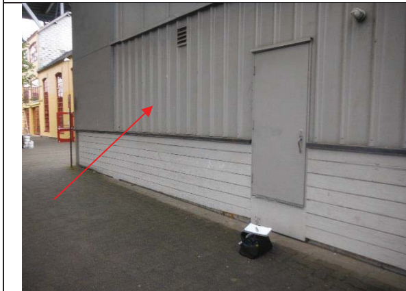
Photo 5: View of the rear portion of the building. The corrugated cement panels present on the exterior walls were assumed to be asbestos containing. The white paint contains more than 0.06% lead.
