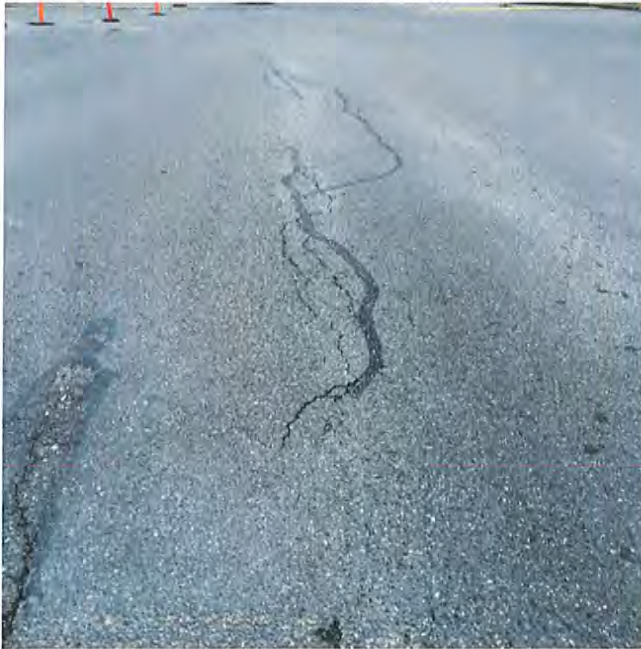
Photo 1: Longitudinal and alligator cracks
