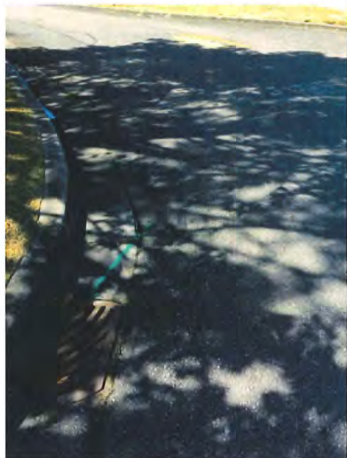
Photo 7: Long patch in the exit lane after inspection area
