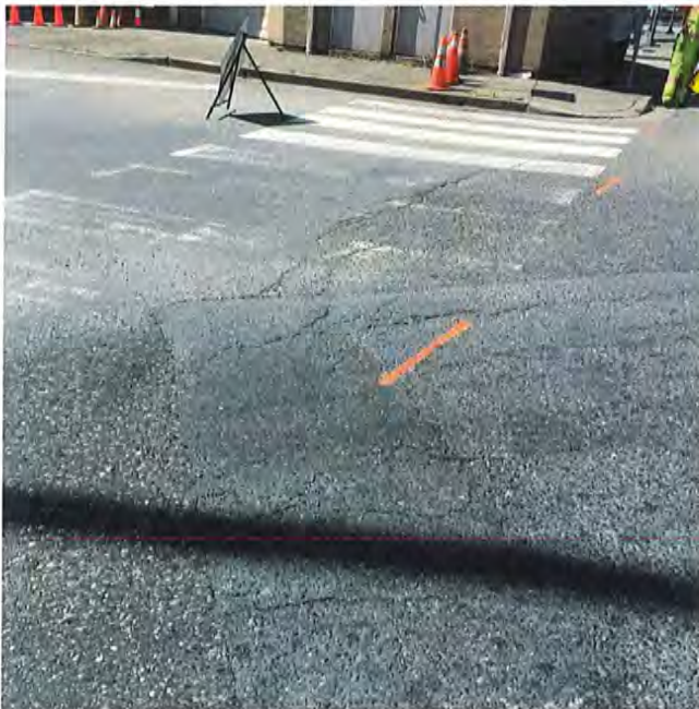
Photograph 3 – Cracked asphalt of commercial lane
