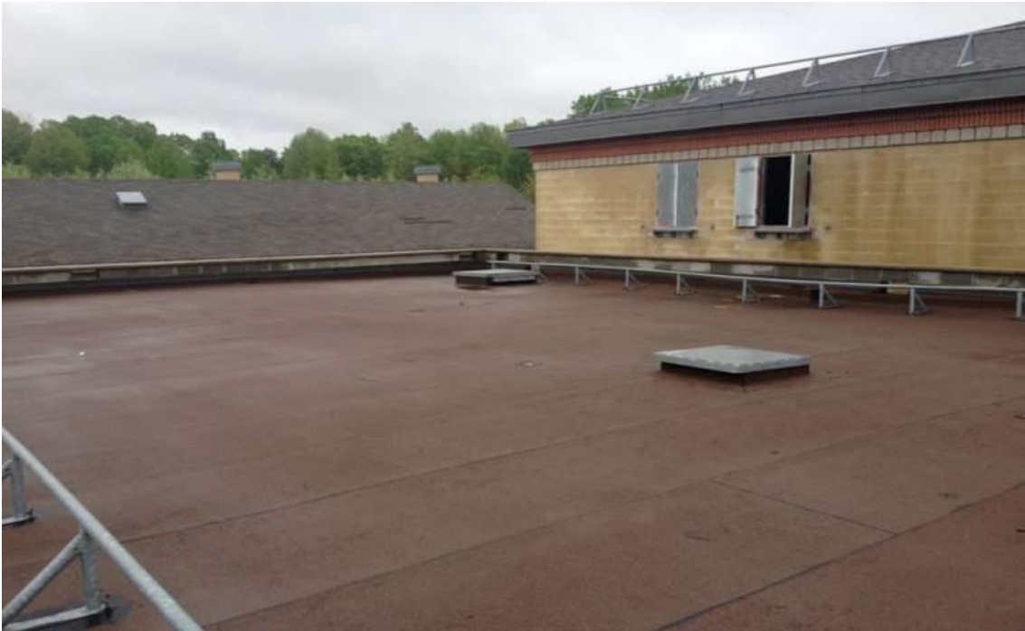
Rooftop with Anchors for Customized Training
