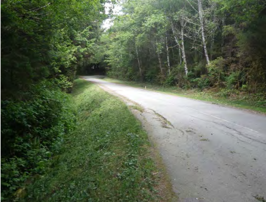
Wick Road Slope – oversteepened fill slope on downhill side of road.
