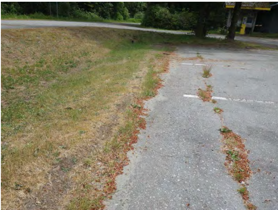
Photo 6: Cracking and built up vegetation adjacent to swale (27-May-2016)
