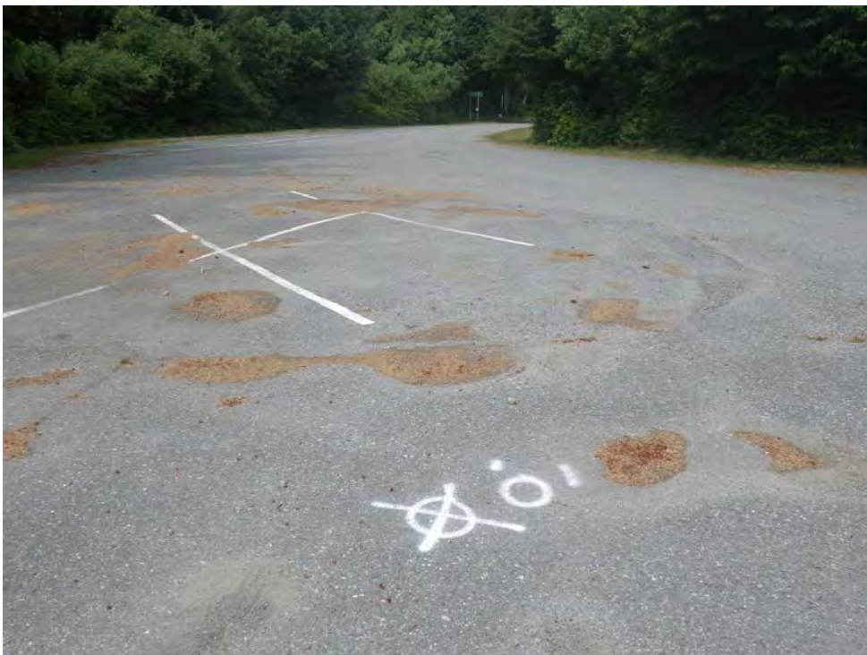
Photo 8: Kwisis Visitors Centre parking lot – note pot holes (27-May-2016)
