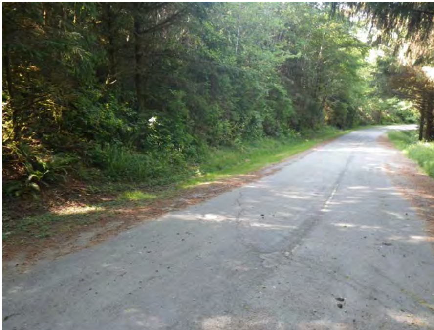
Wick Road Slope – pavement cracking and settlement where the road transitions from cut to fill construction.
