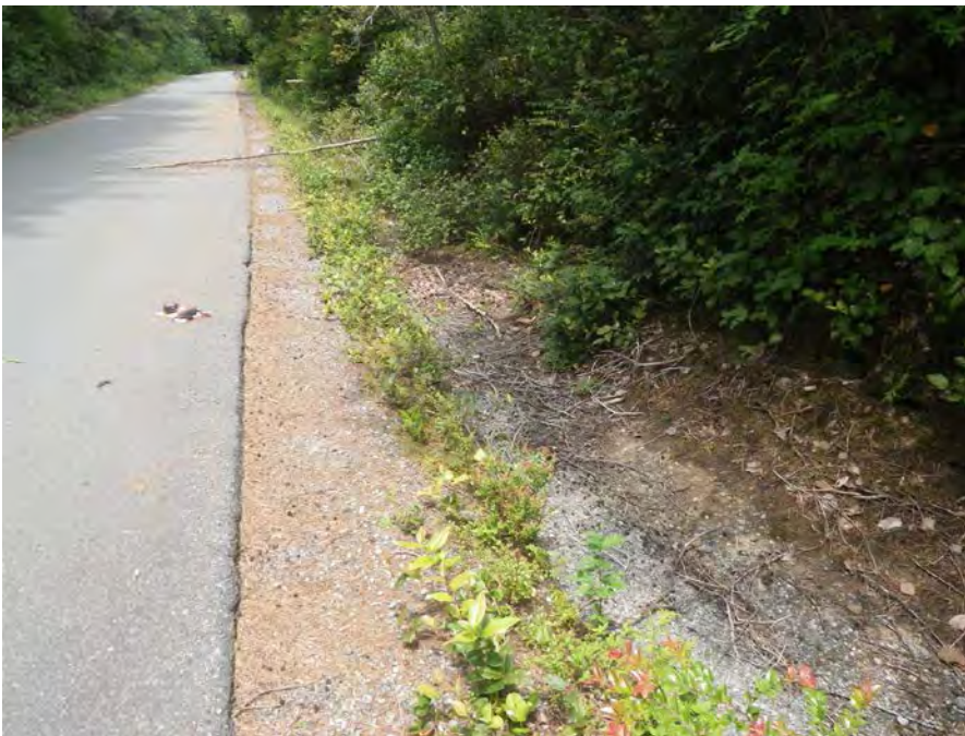
Florencia Bay Access – unsupported edge of pavement and inadequate ditching.
