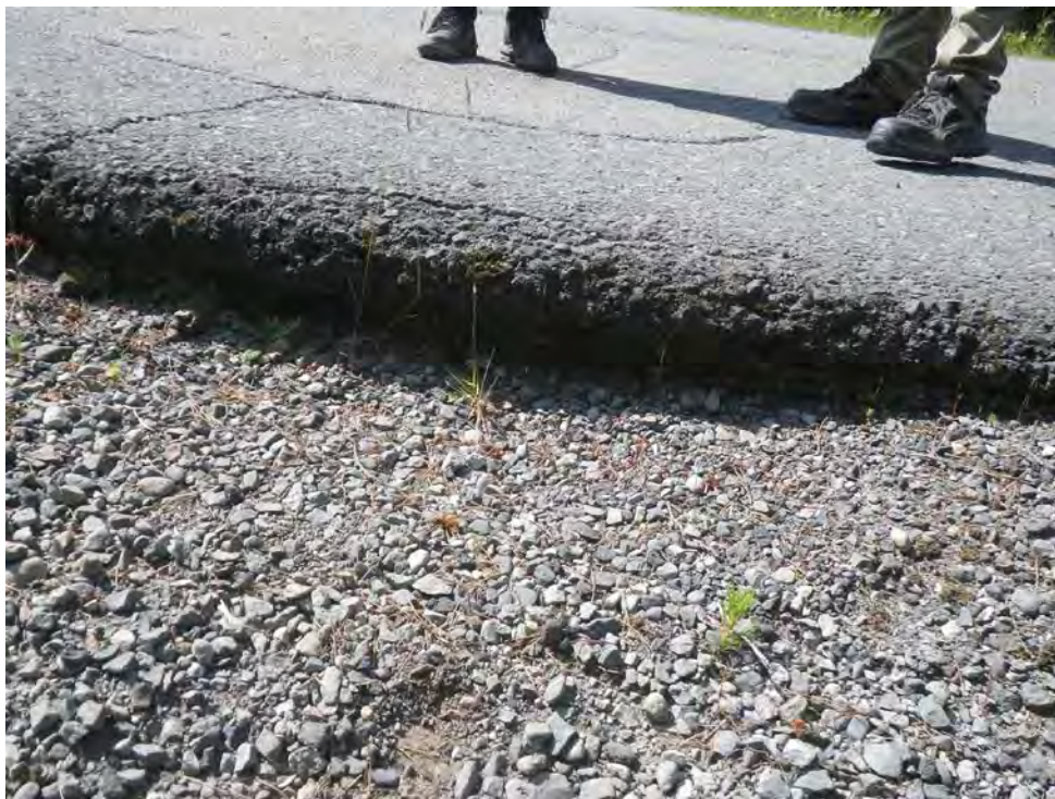
Photo 2: Undermined asphalt at north shoulder of Wick Road (27-May-2016)
