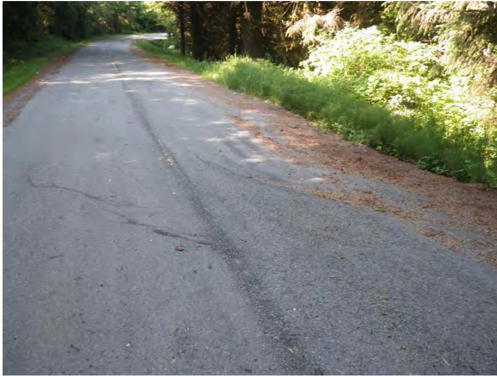
Photo 3: Wick Road cracking and subsidence at ~Sta. 0+150 (27-May-2016)
