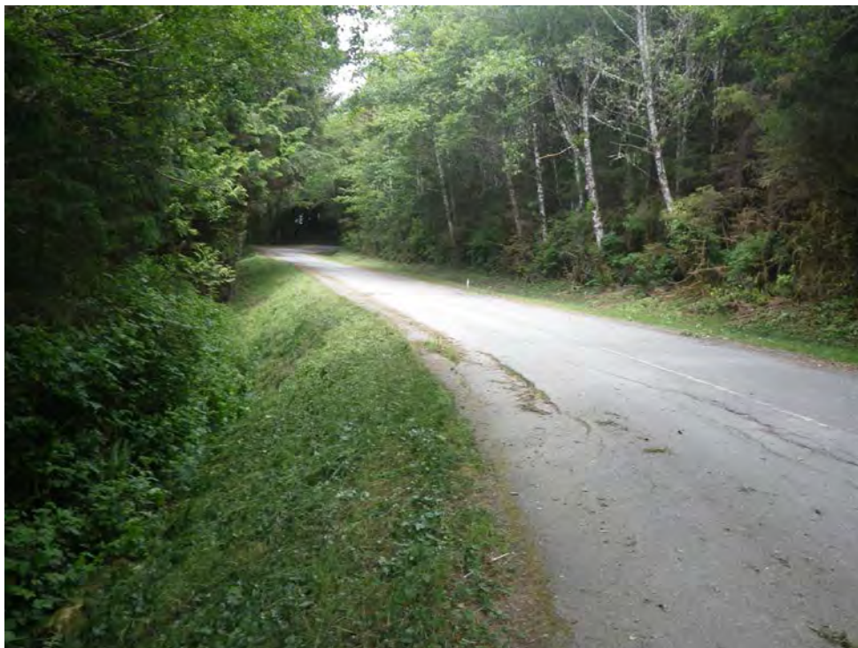
Photo 4: Steep embankment slope at Wick Road ~Sta. 0+090 (27-May-2016)
