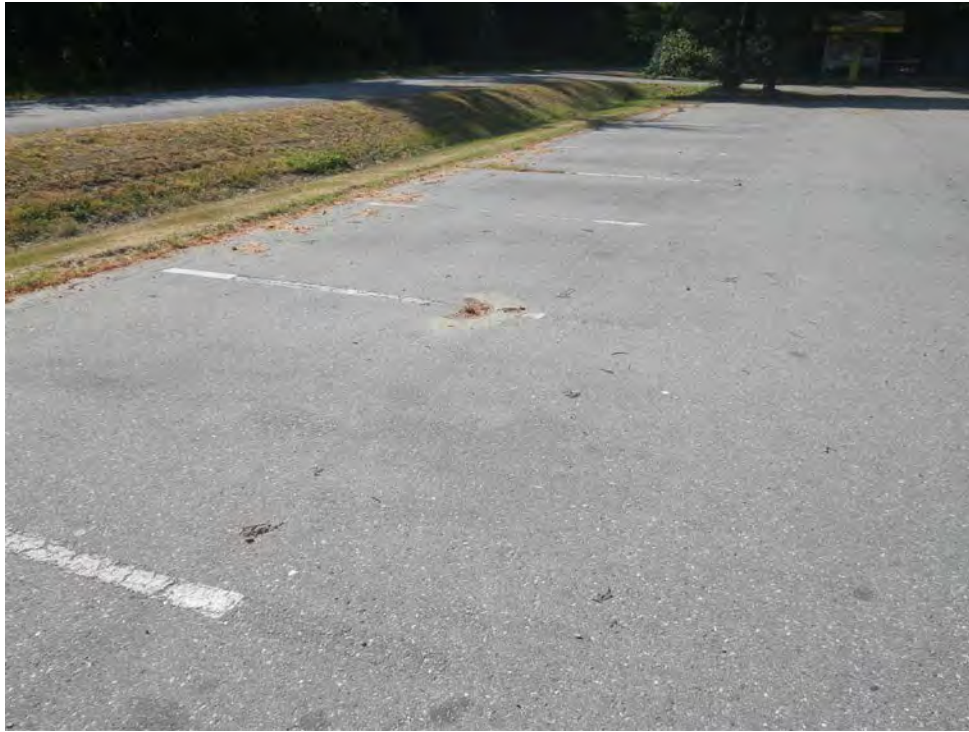
Photo 7: Localize pot hole adjacent to paving joint (27-May-2016)
