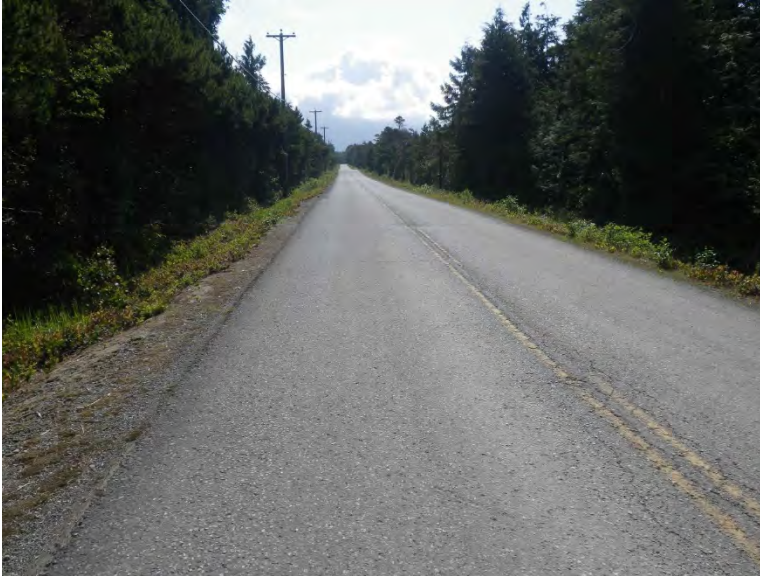
Wick Road – note longitudinal cracks at centreline and surface weathering
