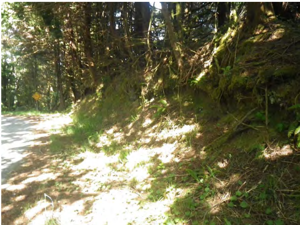
Photo 10: Undermined trees at Sta. 0+200 Wick Road (27-May-2016)
