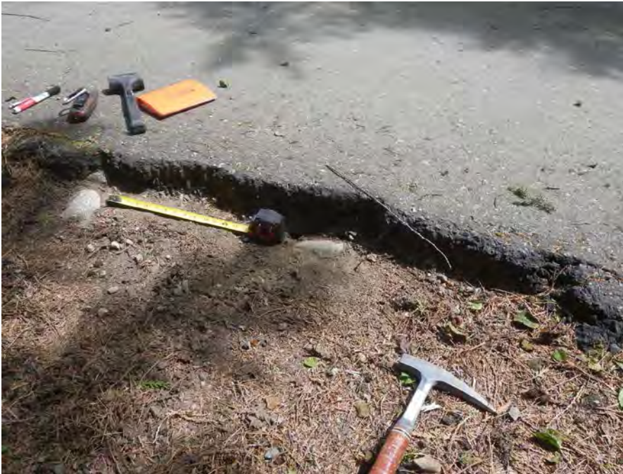
Florencia Bay Access – edge of pavement failure due to inadequate shoulder fills. Note cobbly embankment fill.
