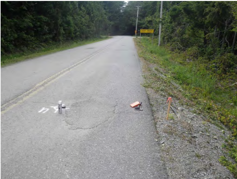
Wick Road – patched pothole and unsupported edge of pavement
