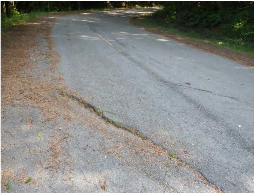
Wick Road Slope – pavement cracking and settlement within fill section of embankment.
