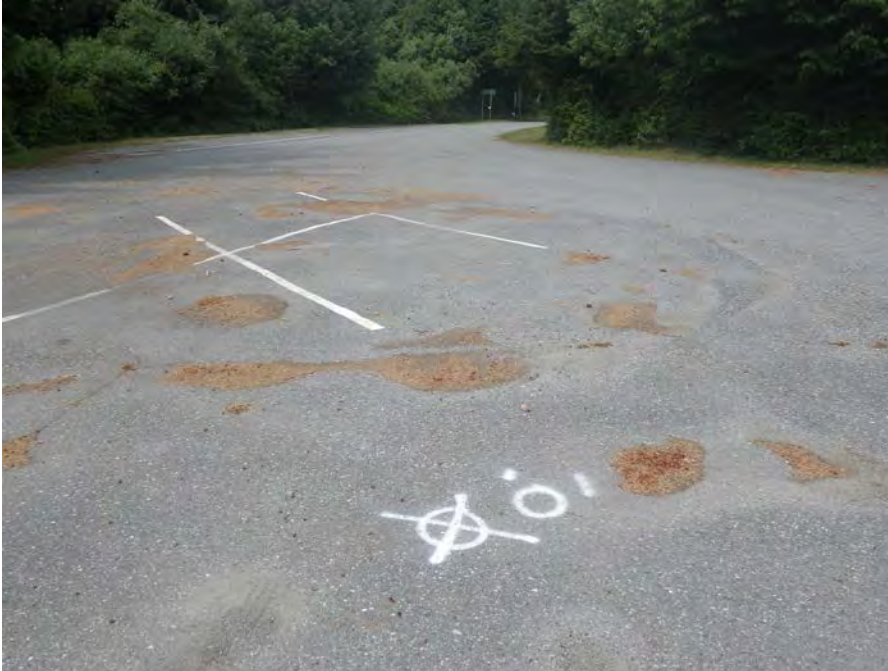
Kwisitis Parking Lot – numerous potholes/depressions within and around the perimeter of a former planter area.
