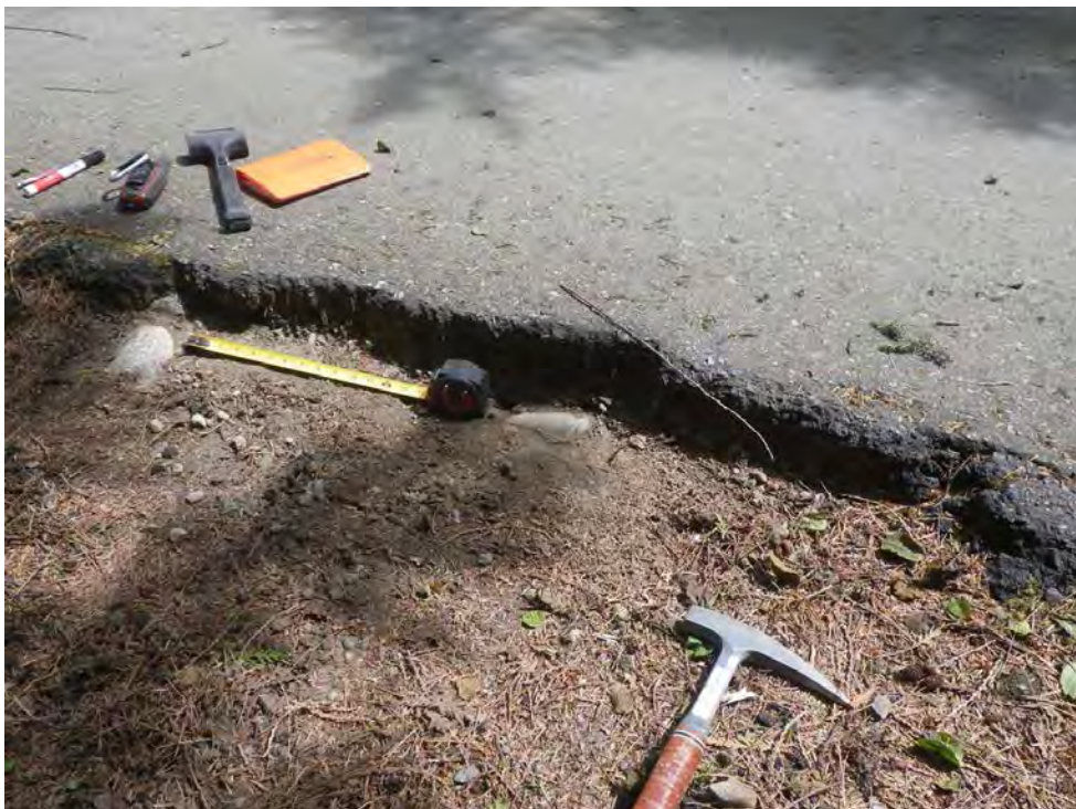
Photo 12: Florencia Bay Access Road – note unsupported asphalt and cobbly embankment fill materials. (27-May-2016)
