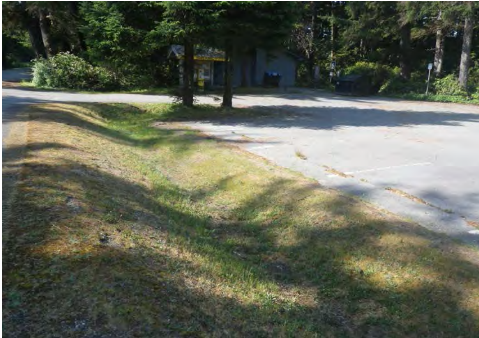
Beach Parking Lots - note longitudinal cracks and vegetation in swale and along edge of pavement
