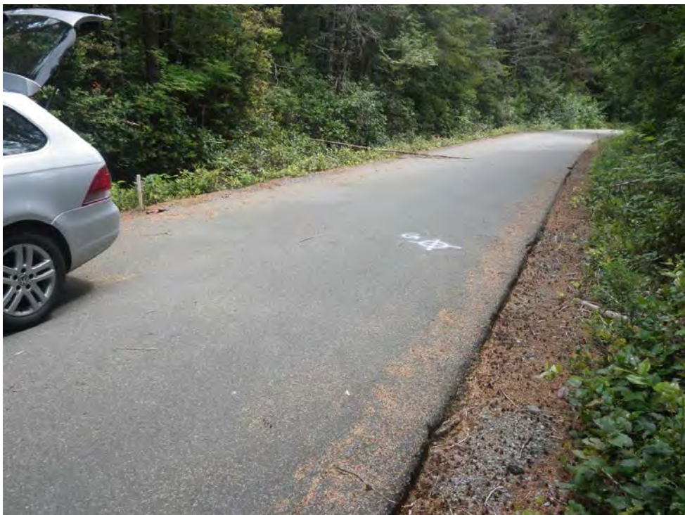
Photo 14: Florencia Bay Access Road – inadequate shoulder (27-May-2016)
