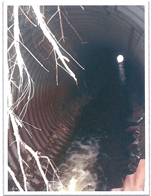
Figure 1 Existing 2.2m culvert with corroded base.
