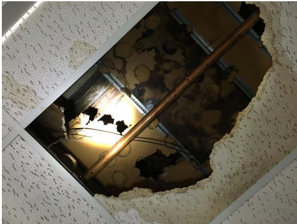
Photo 4: View of the mould impacted drywall with asbestos-containing drywall joint compound observed in Location 26 in the Storage Room of the ground floor.
