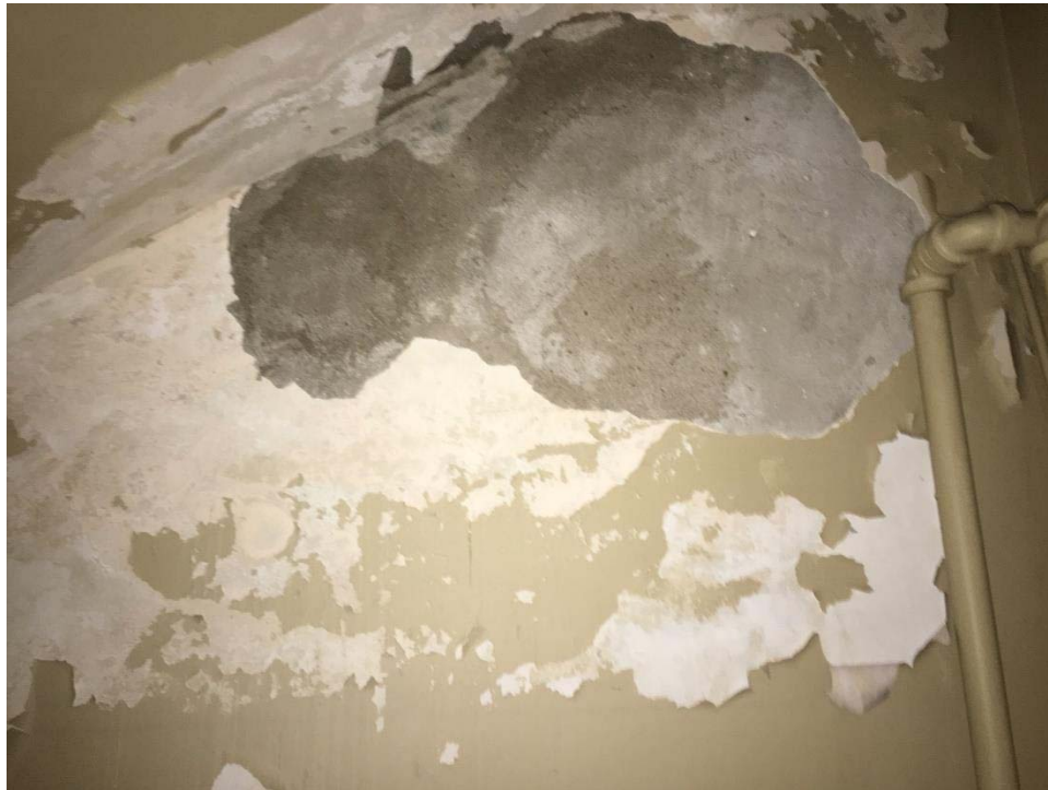
Photo 1: View of the poor condition asbestos-containing plaster observed in Location 43 in the Stairwell of the basement.
