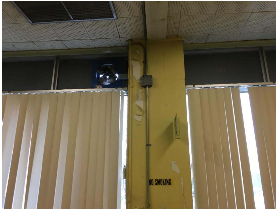
Photo 3: View of the damaged lead-containing paint observed in Location 45 in the Environment Canada Office of the second floor.
