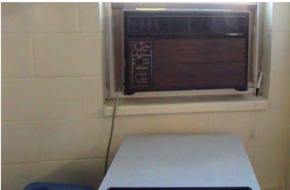
Photograph 12: Typical alternate style window mounted air-conditioning unit present in offices. Unit contains halocarbons.
