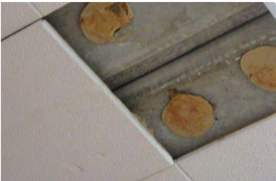
Photograph 8: Room 108 Brown/beige ceiling tile glue (sample C2A) present under tiles in office.
