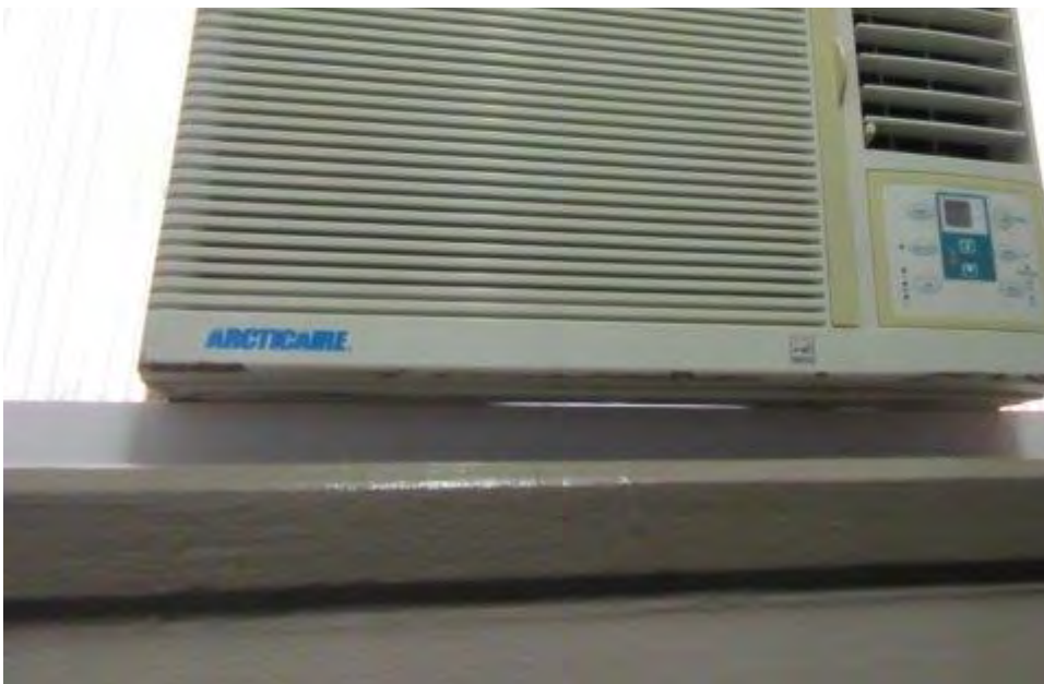
Photograph 4: Typical window mounted air-conditioning unit present in all offices (approximately 10). Units contain halocarbons.
