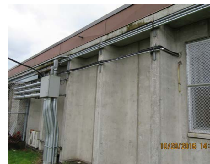
(PHOTO 3) EXISTING EXTERIOR JUNCTION BOX & CONDUITS SCALE NTS
