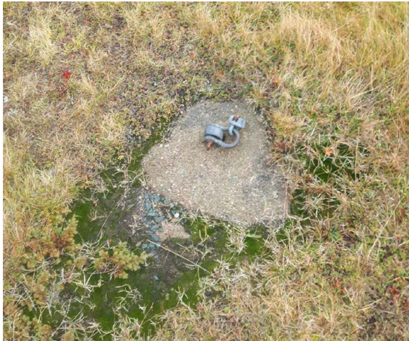
Fig. 3. Anchoring ring of the old mast located on the southwest side of the lighthouse and its concrete base. (Photo: Newfoundland East Field Unit).
