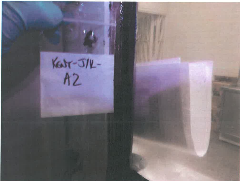
Photograph 4: Non-Asbestos grey mastic between the window pane and frame on the door facing Living Unit J kitchen.
