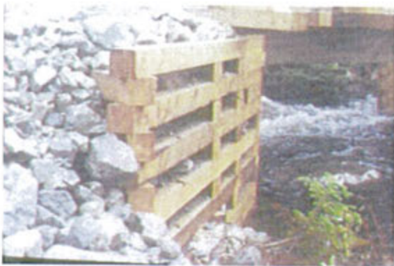
Figure 1: Infill material for timber cribs should be blocky, angular and free of fines or sediment.
