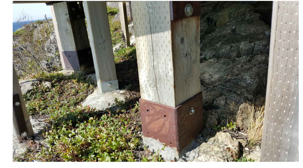
VIEW OF MISSING POST BOLTS (TYP.)
