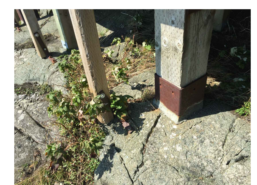
VIEW OF MISSING SUPPORT BOLTING ADD LAG SCREWS
