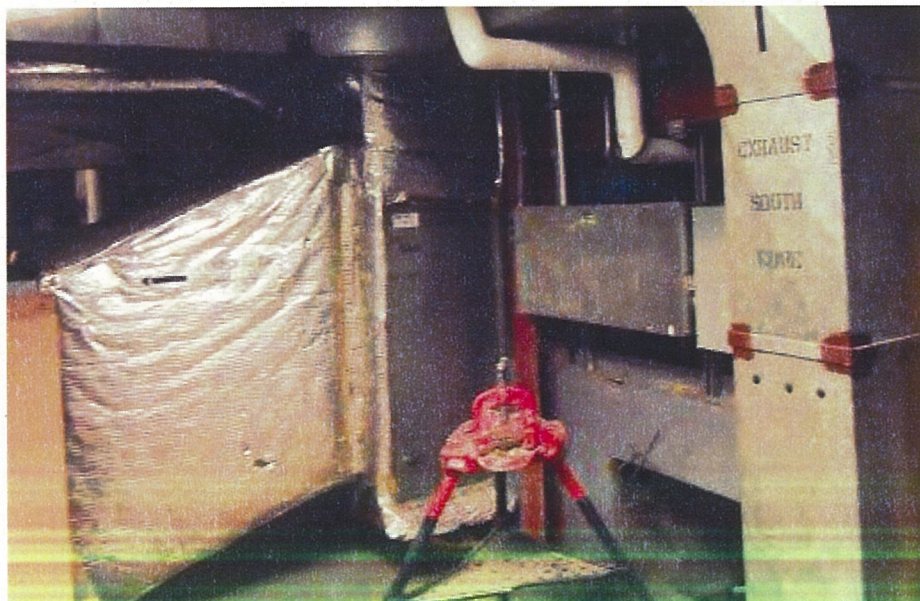
Photograph 9: Non-asbestos fiberglass thermal insulation with foil wrap applied to air ducts.
